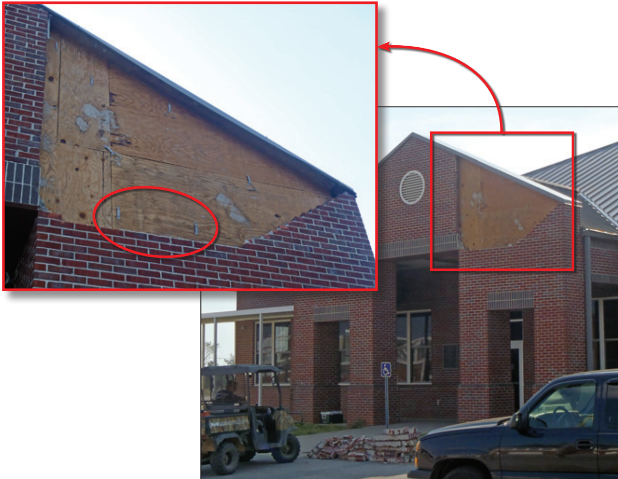
Figure 3-5: Brick veneer blew off this high school cafeteria during the tornado in Phil Campbell, AL. Note that brick ties do not appear to be at the correct spacing, which may have contributed to the failure (shown in red circle in inset).
