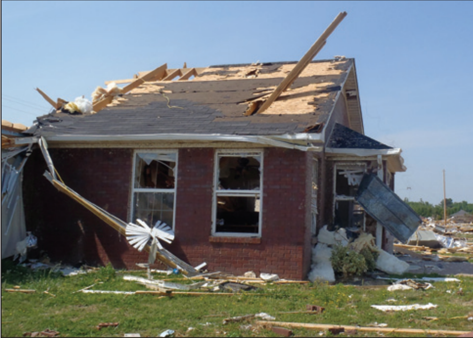
Figure 3-9: Large roof beam penetrated the roof of this home (Athens, AL)
