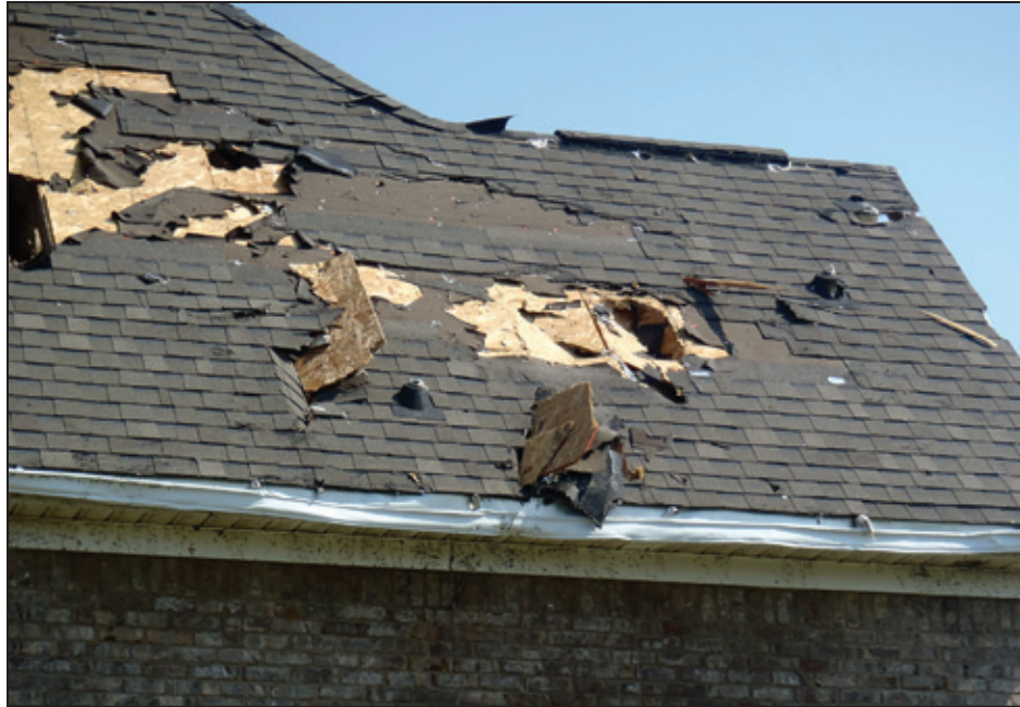
Figure 3-11: Small pieces of OSB debris penetrated the roof of a home (Harvest, AL)
