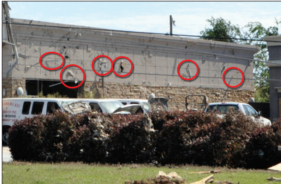
Figure 3-16: Numerous missiles struck the outer wall of this non-residential building, including several that remained embedded (indicated by red circles) (Tuscaloosa, AL)
