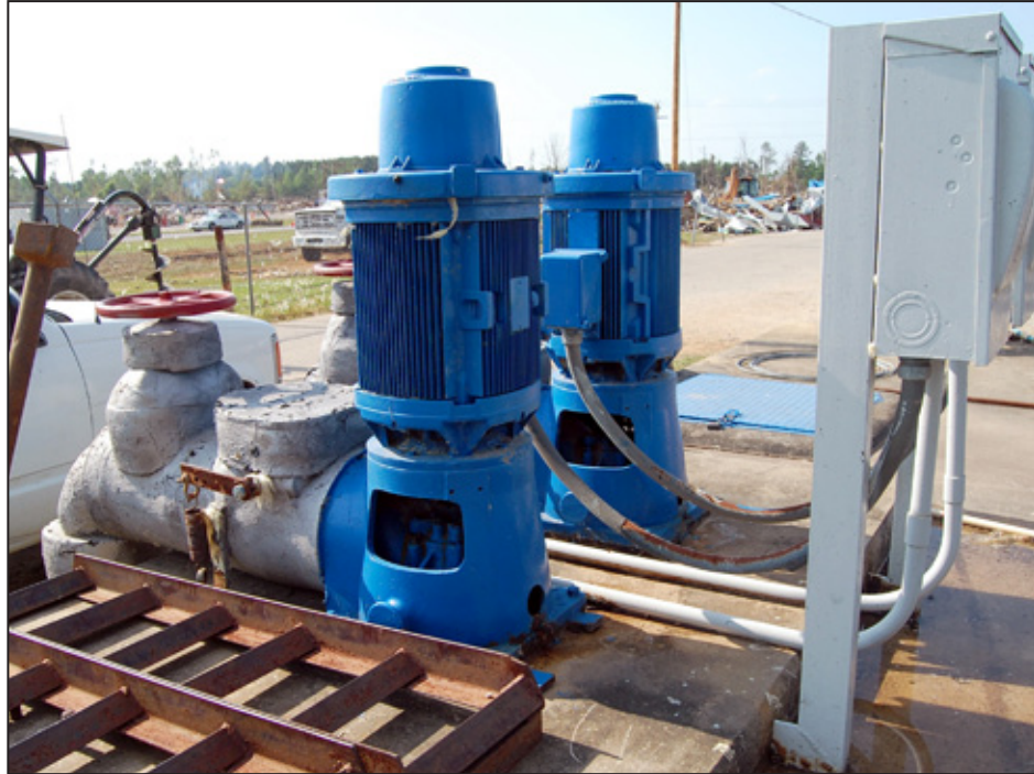
Figure 8-11: Lift pumps and controls of the Smithville, MS, water plant were exposed, but not damaged
