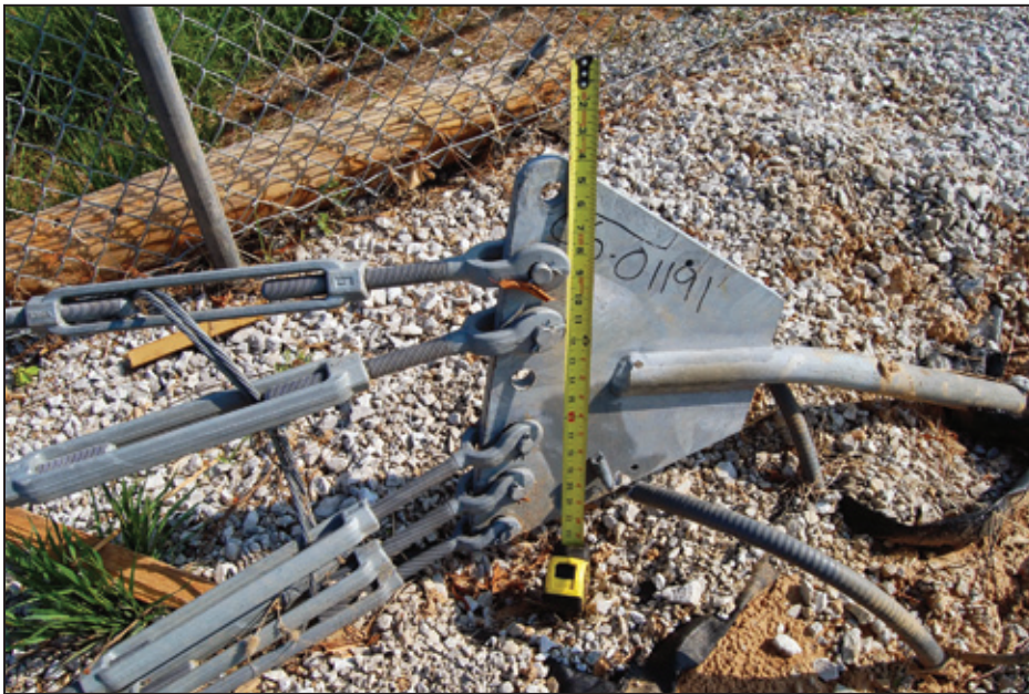
Figure 8-28: Guy attachment plate, turnbuckle, and anchor shaft (Smithville, MS)
