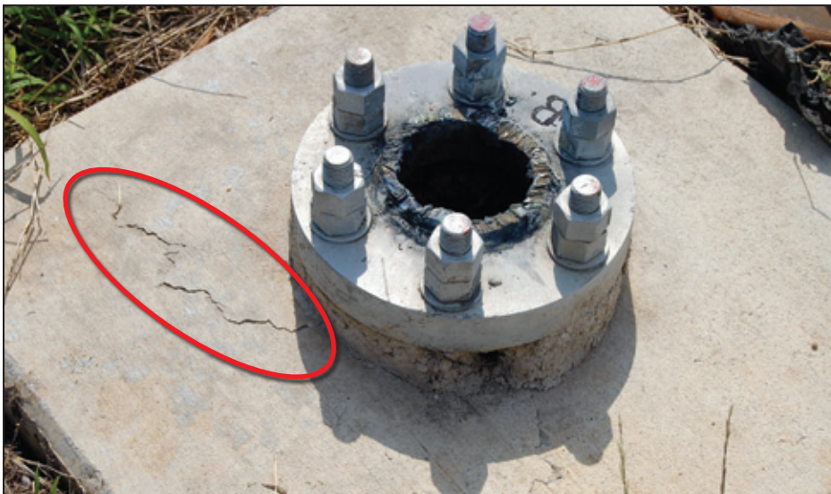
Figure 8-17: Photograph shows the six-bolt tower base with cracks in concrete foundation cap (red oval) (Tuscaloosa, AL)
