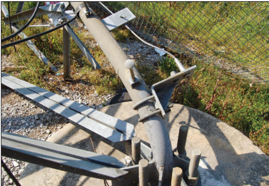
Figure 8-19: Base for 300-foot latticed cellular tower (Tuscaloosa, AL)
