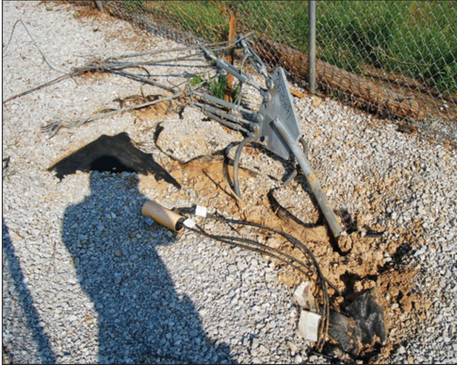
Figure 8-31: The anchor securing one guy was dragged several feet through the ground (Smithville, MS)
