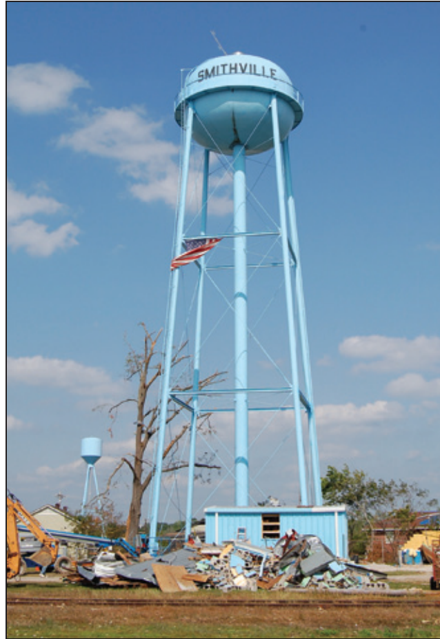
Figure 8-7: Water tower after the tornado (Smithville, MS)
