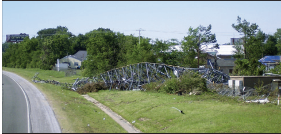
Figure 8-20: View of the 300-foot latticed cellular tower that collapsed during the tornado event (Tuscaloosa, AL)
