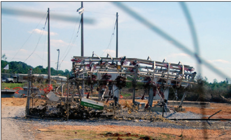
Figure 8-4: Representative damage to overhead electrical lines and substations along the tornado path (Tuscaloosa, AL)
