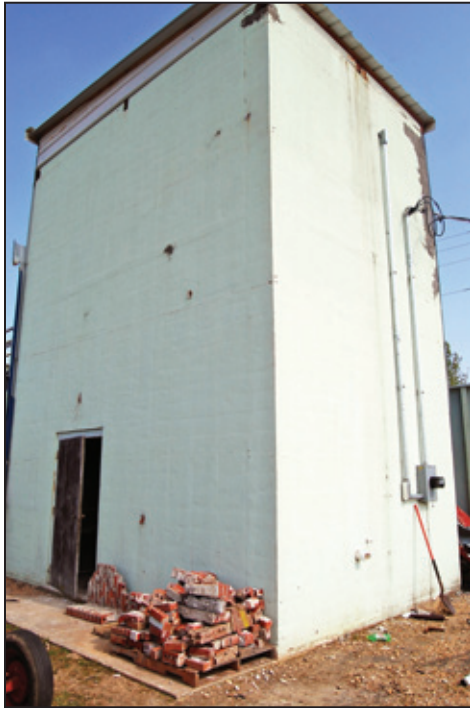
Figure 8-9: Reinforced CMU building housing control equipment (left) and undamaged water treatment control equipment (right) (Smithville, MS)
