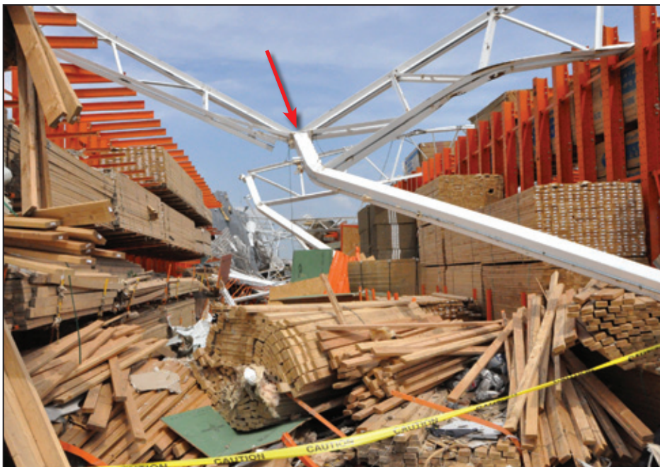
Figure 5-7: Joist girder and column failure. The column-to-joist girder is shown by the red arrow (Joplin, MO).
