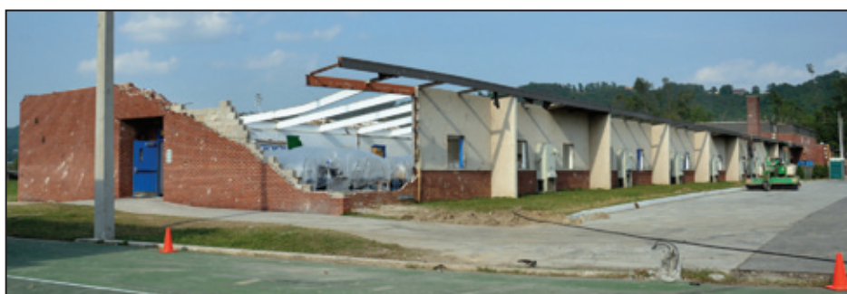
Figure 6-35: This wing lost most of its roof decking, and a portion of the brick veneer and unreinforced CMU collapsed (Ringgold, GA)
