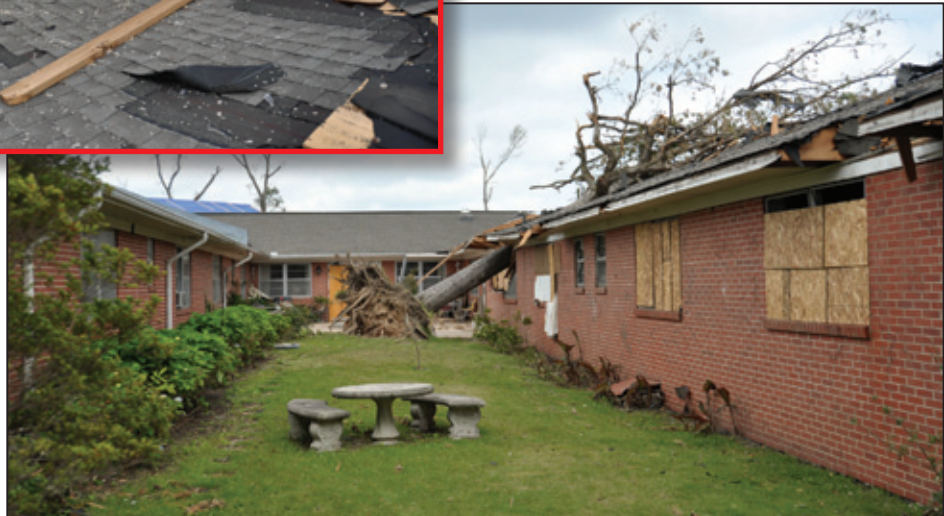
Figure 7-14: Tree-fall damage. Note the boarded-up broken windows. The inset shows a close-up of the tree-fall damage (Tuscaloosa, AL).
