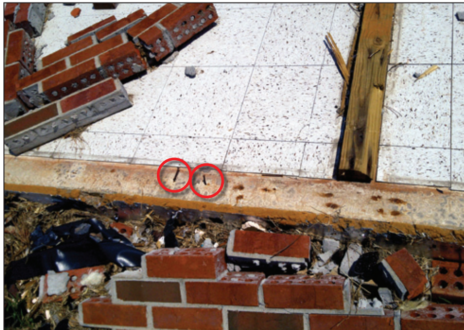
Figure 4-29: Wall-to-foundation connection failure where concrete nails remained in stained concrete slab and bottom plate (missing) pulled over the heads of the nails (red circles) (Hackleburg, AL) [MAT EF Rating = 3]
