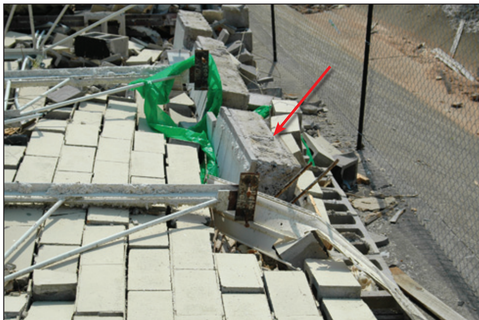
Figure 5-23: Steel joists with joist seat and bond beam on top of collapsed wall (red arrow). Wall fragmentation shows lack of reinforcement in the wall (Tuscaloosa, AL).
