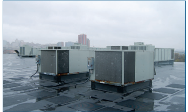
Figure 10: ACC units vulnerable to wind and wind-borne debris
