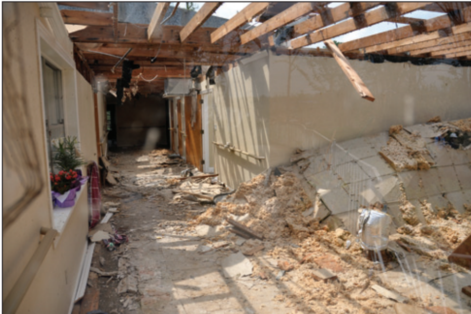
Figure 7-12: Interior damage as a result of roof structure blow-off (Tuscaloosa, AL)
