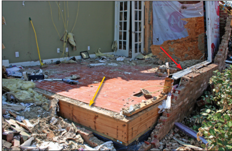
Figure 4-26: Example of DOD 6 showing under-braced framed sunroom wall failure. Note long window bottom on right (red arrow) and the failure of nailed wall-to-floor connection on left wall (yellow arrow) (Harvest, AL). [MAT EF Rating = 2]
