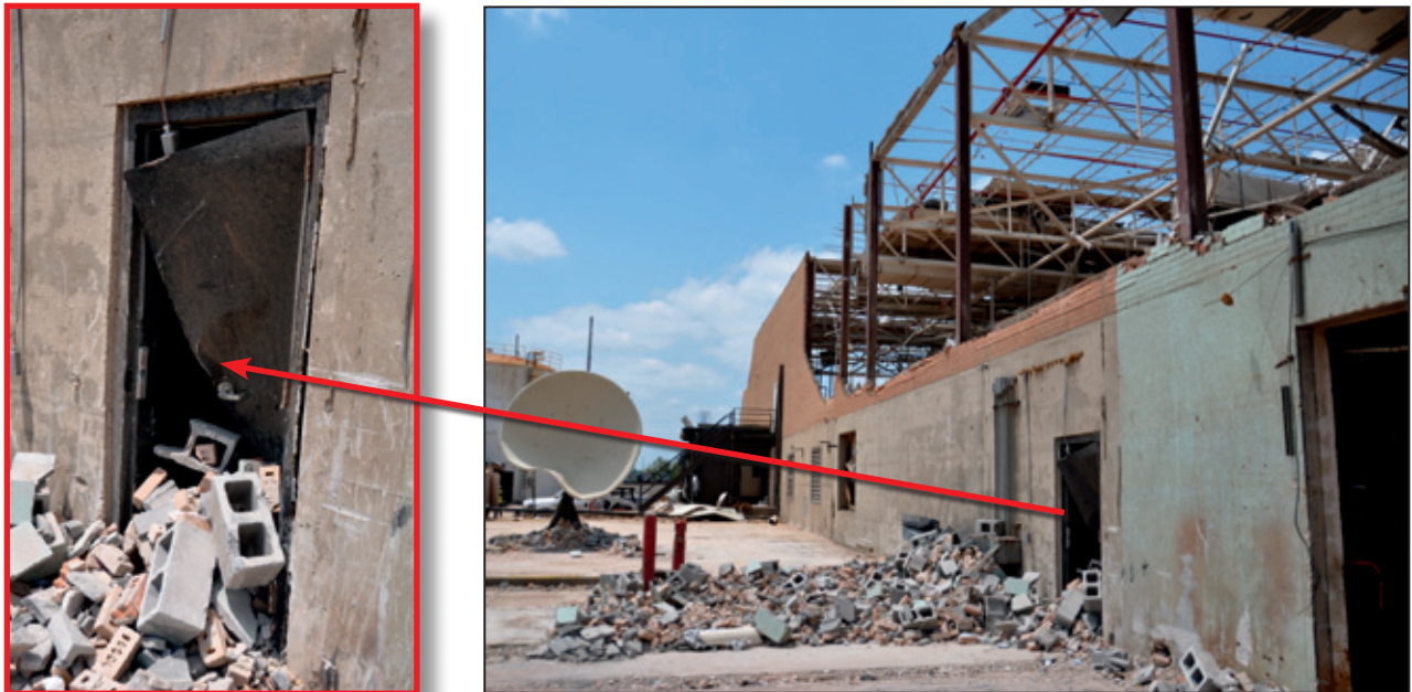
Figure 7-60: Part of the southern portion of the building. The inset shows a metal door that buckled inward (Tuscaloosa, AL).
