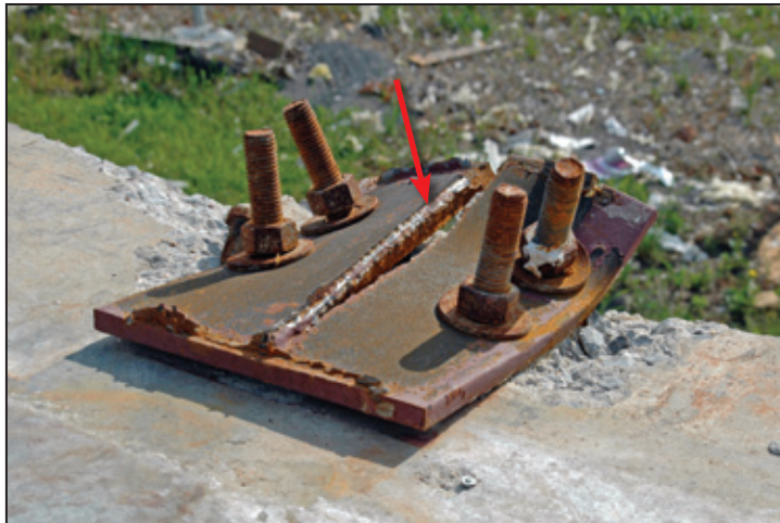
Figure 5-49: Ductile end column at southwest corner of building (red arrow). The anchor bolts remained attached to both the foundation and the column (Tuscaloosa, AL).
