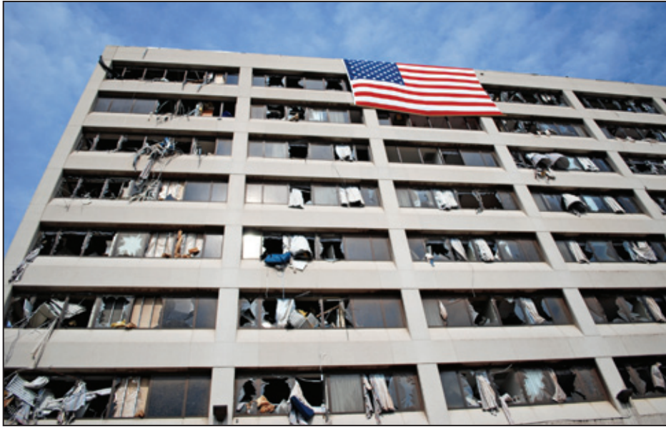
Figure 7-22: View of the glazing damage at patient rooms (Joplin, MO)
