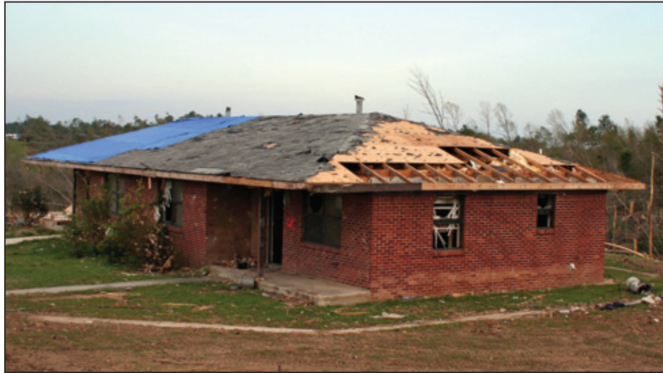
Figure 4-14: Example of DOD 4 showing roof decking removed at wide eaves on hip roof (Phil Campbell, AL) [MAT EF Rating = 1]
