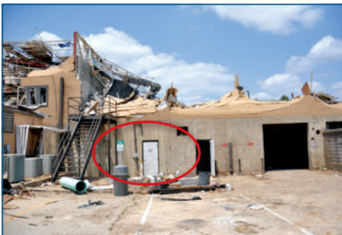
Figure 9: An EOC in Tuscaloosa, AL, that remained intact even though the story above it collapsed (Tornado 2011)
