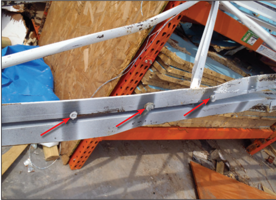
Figure 5-6: Failed puddle welds that connected the metal roof deck to the top chord of the joist (red arrows) (Joplin, MO)
