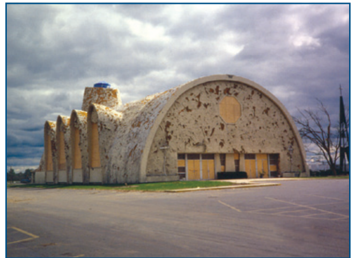
Figure 6: Although struck by a strong tornado, the SPF roof system of this Plainfield, IL, building did not blow off (1990 Tornado)
