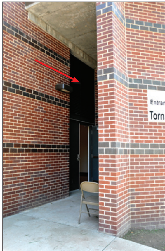
Figure 9-44: Outside doors and louvers (red arrow) protected by alcoves at the Seneca Intermediate School community safe room
