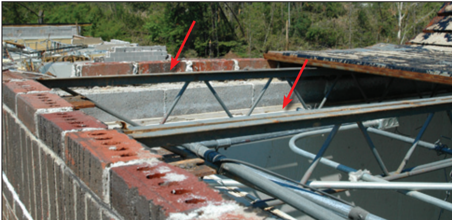
Figure 5-27: Failed roof deck with no connections between the roof deck and the joists (red arrows) (Birmingham, AL)
