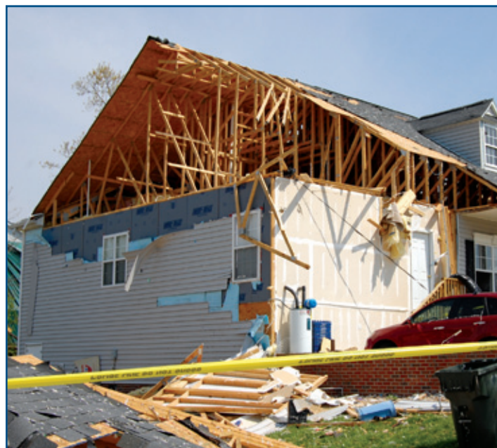
Figure 1: A house that lost large sections of the roof and the garage due to internal pressurization.
