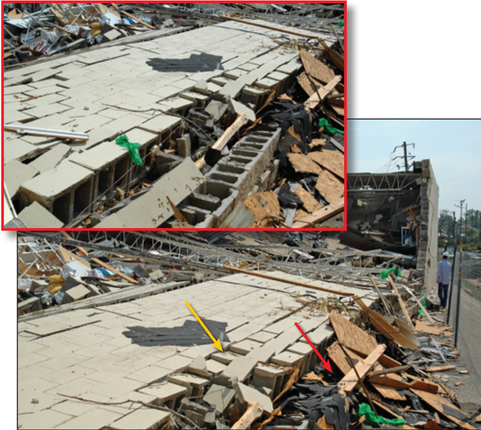
Figure 5-21: Global wall instability failure. The CMU blocks are lying loosely on the ground and many have rotated (yellow arrow) due to the complete separation of all the blocks. Note lack of reinforcement in the wall and especially between wall and footing (red arrow). Inset shows a close-up view of the separation of the blocks (Tuscaloosa, AL).
