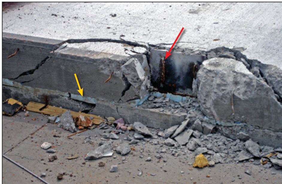
Figure 5-11: Joist support pocket at top of a precast wall. The red arrow points to weld marks from the connection to the framing member seat on the embedded plate. The yellow arrow points to the light blue insulation layer between the concrete shells (Joplin, MO).
