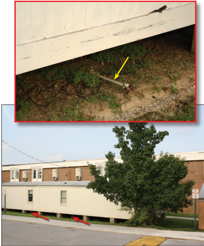
Figure 6-25: View of one of the portable classrooms. The red arrows indicate anchor straps. The strap shown in the inset had corroded through (yellow arrow) (Ringgold, GA).
