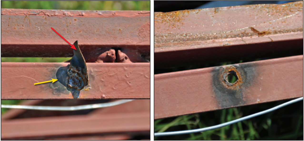
Figure 6-21: Red arrow shows a strong weld attaching a piece of decking to the joist (the dark area shown by the yellow arrow is a shadow). The photo on the right shows a weak deck attachment where the weld burnt through the joist (Tuscaloosa, AL).
