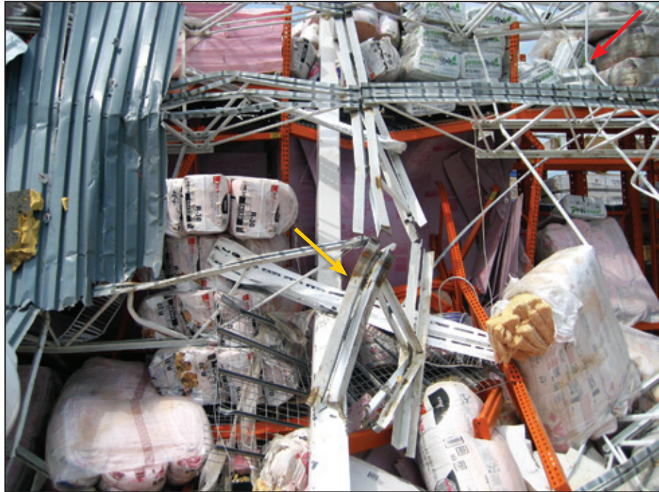
Figure 5-12: Failure of joist-to-joist girder connection shown by broken welds (yellow arrow); red arrow shows location where bridging angle is touching insulation bundles (Joplin, MO)
