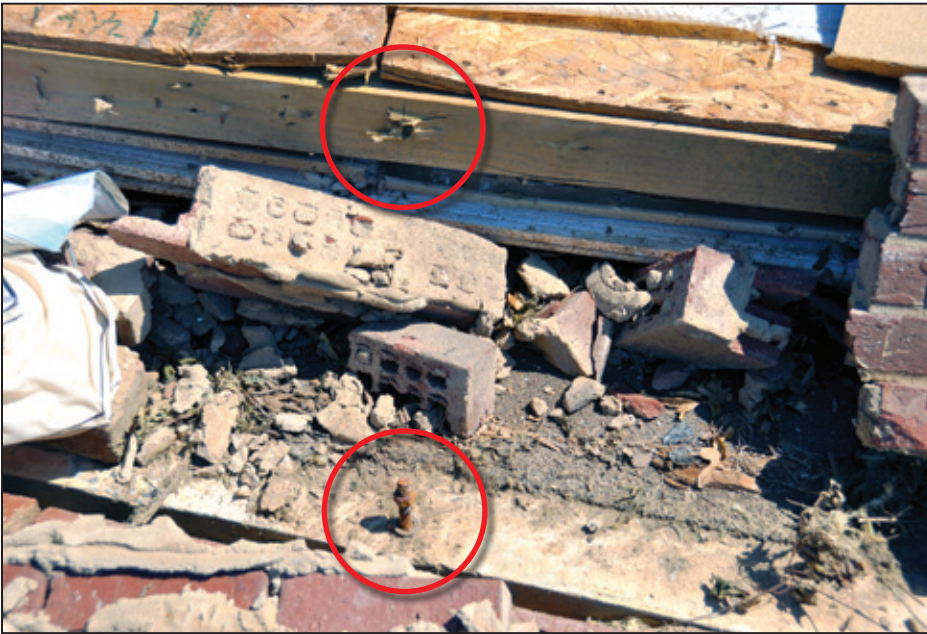
Figure 4-39: Two-story Chastain Manor Apartment slab with bottom plate pulled over remaining anchor bolt and 1-inch diameter washer; red circles indicate where bolt and plate were connected prior to damage
