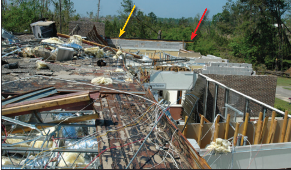
Figure 5-26: Roof joist lifted off front (red arrow) and folded over rear half of building (yellow arrow) (Birmingham, AL)
