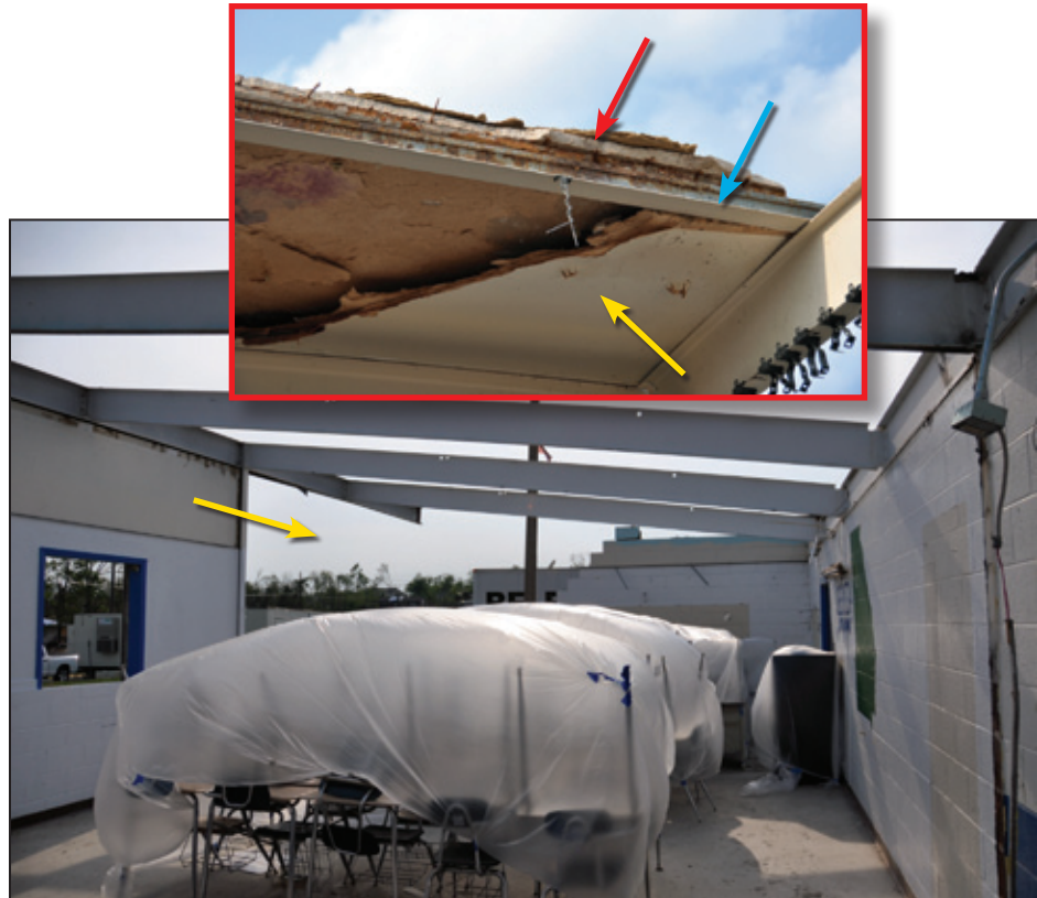
Figure 6-36: View from within a classroom. The yellow arrow shows the area of the collapsed wall that is shown in Figure 6-35. In this area, the deck bulb-tees also blew off. The inset shows an area of this wing where some form-board (yellow arrow), a bulb-tee (blue arrow), and the gypsum deck (red arrow) were still in place (Ringgold, GA).
