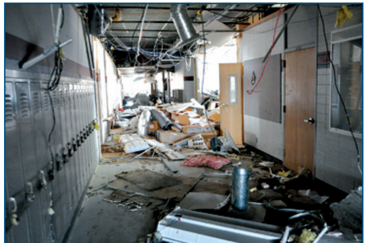
Figure 1: Debris in a school corridor in Joplin, MO (2011 Tornado)
