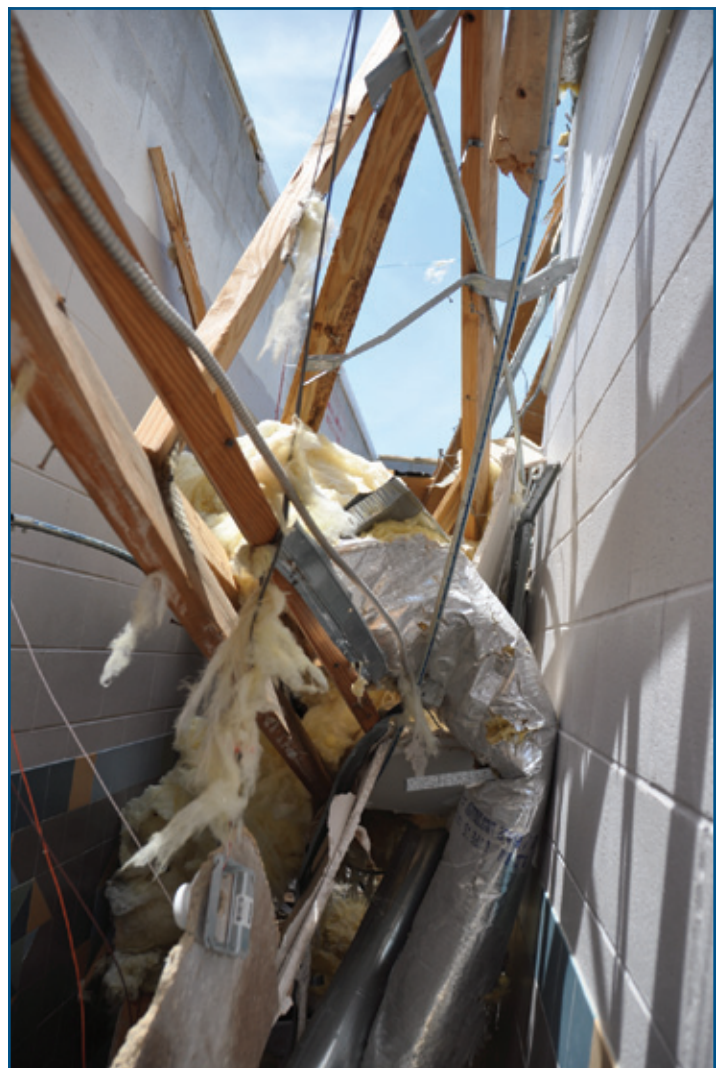
Figure 2: Debris in an elementary school restroom in Tuscaloosa, AL (Tornado 2011)
