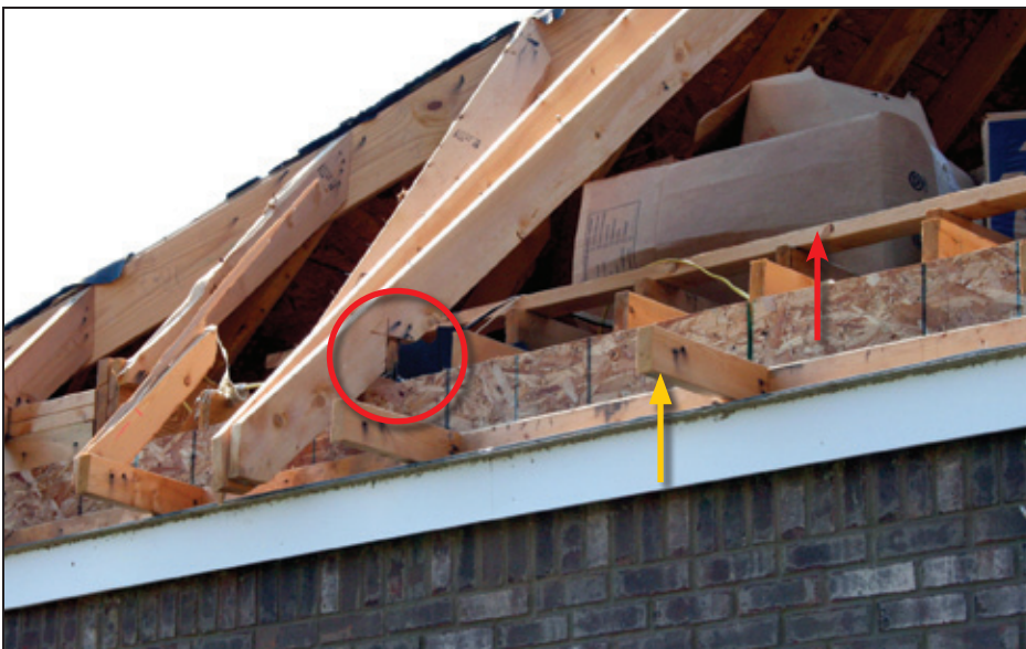
Figure 4-19: Example of roof-to-wall connection failure facilitated by non-code-compliant construction: notched rafters, known as “bird’s mouth,” (red circle) displaced when roof-to-wall connections failed; red arrow indicates rafter bearing plate, yellow arrow indicates outlooker (Harvest, AL) [MAT EF Rating = 1]
