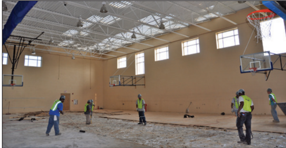
Figure 6-29: The loss of the roof covering shown in Figure 6-28 led to water intrusion that damaged the floor below. The damaged floor needed to be removed and replaced (Ringgold, GA).
