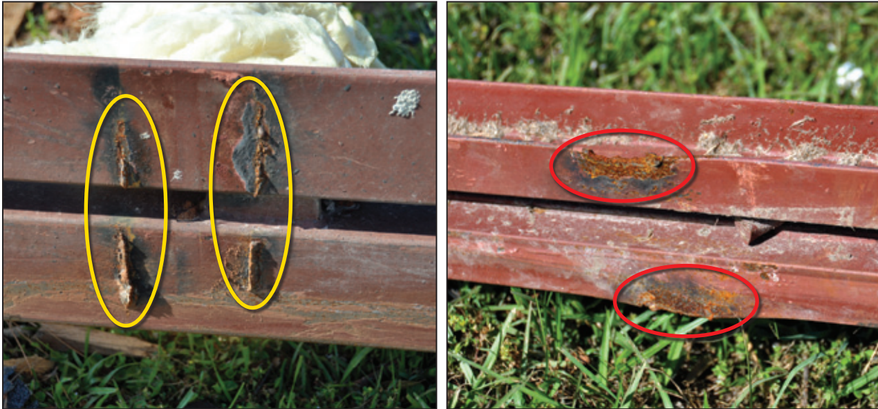
Figure 6-20: The yellow ovals on the left photograph show weld remnants where a joist was attached to the girder. The red ovals on the right photograph show weld remnants where a joist was attached to a bearing plate at a bond beam (Tuscaloosa, AL).
