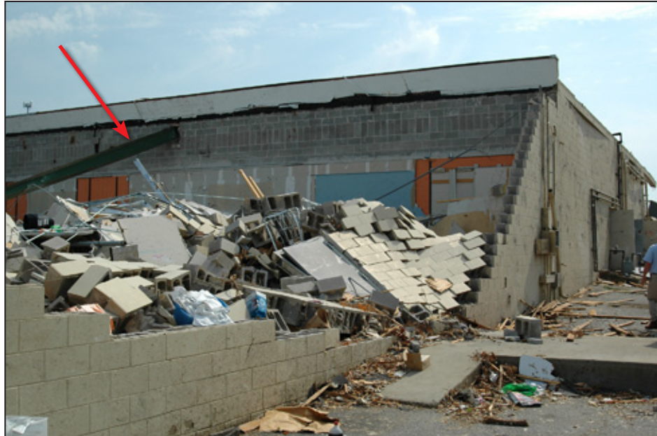
Figure 5-19: Solid steel hot rolled sections (red arrow) left in beam pockets of CMU building section. These supported the steel joists shown in Figure 5-18. Also note lack of reinforcement in the wall and wall-to-foundation connection (Tuscaloosa, AL).
