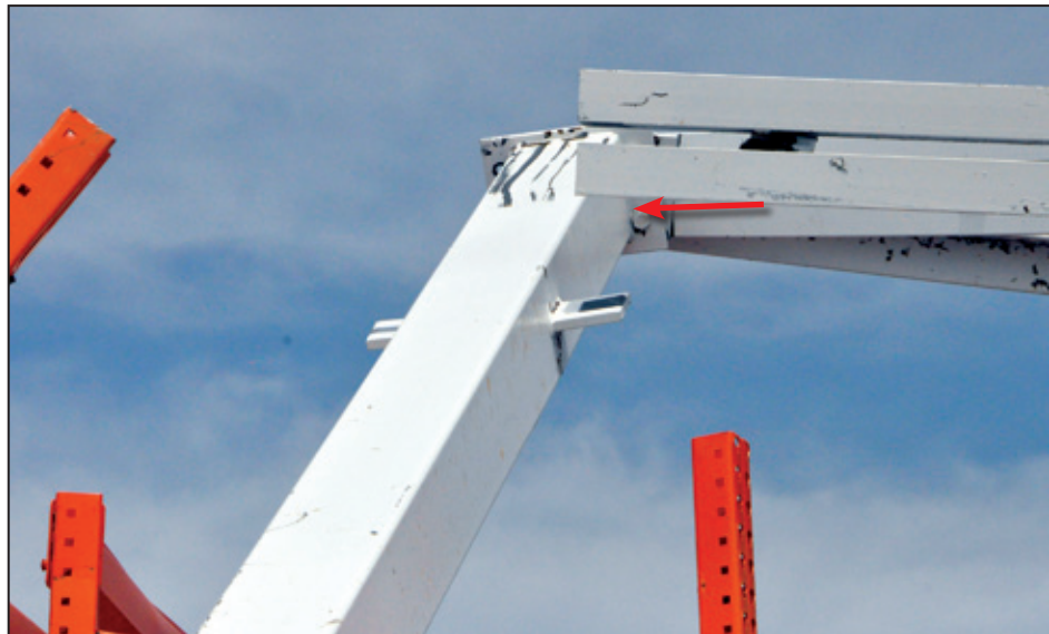
Figure 5-8: Separation at bottom chord to stabilizer plate (red arrow) (Joplin, MO)
