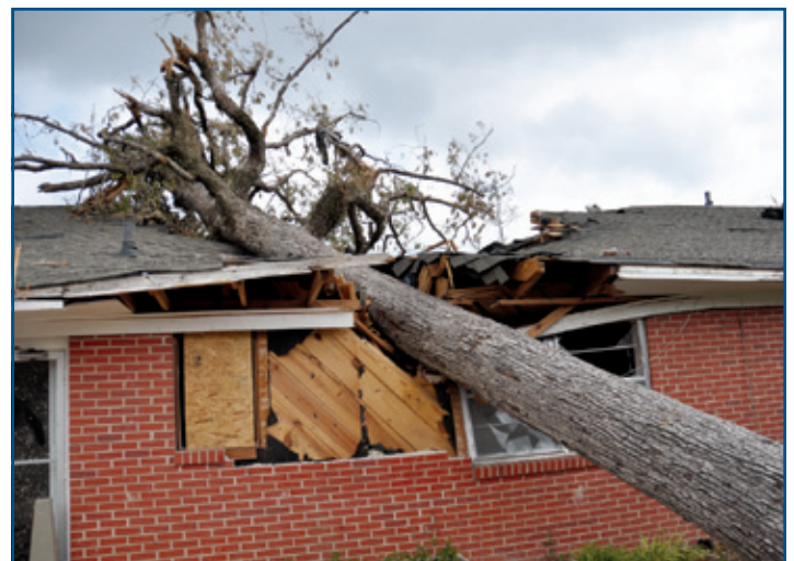
Figure 5: Tree-fall damage at a critical facility in Tuscaloosa, AL (2011 Tornado)
