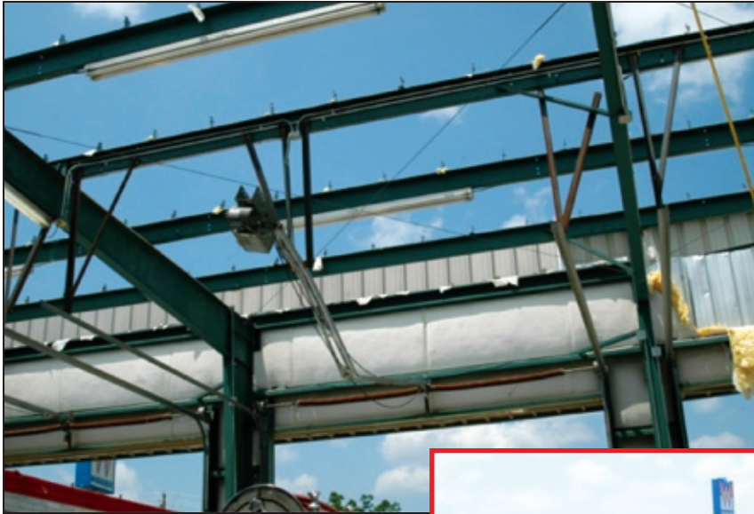
Figure 7-32: The metal roof panels blew off the apparatus bay of the fire department. The panels unlatched from the clips, shown at another angle in the inset (Fultondale, AL).
