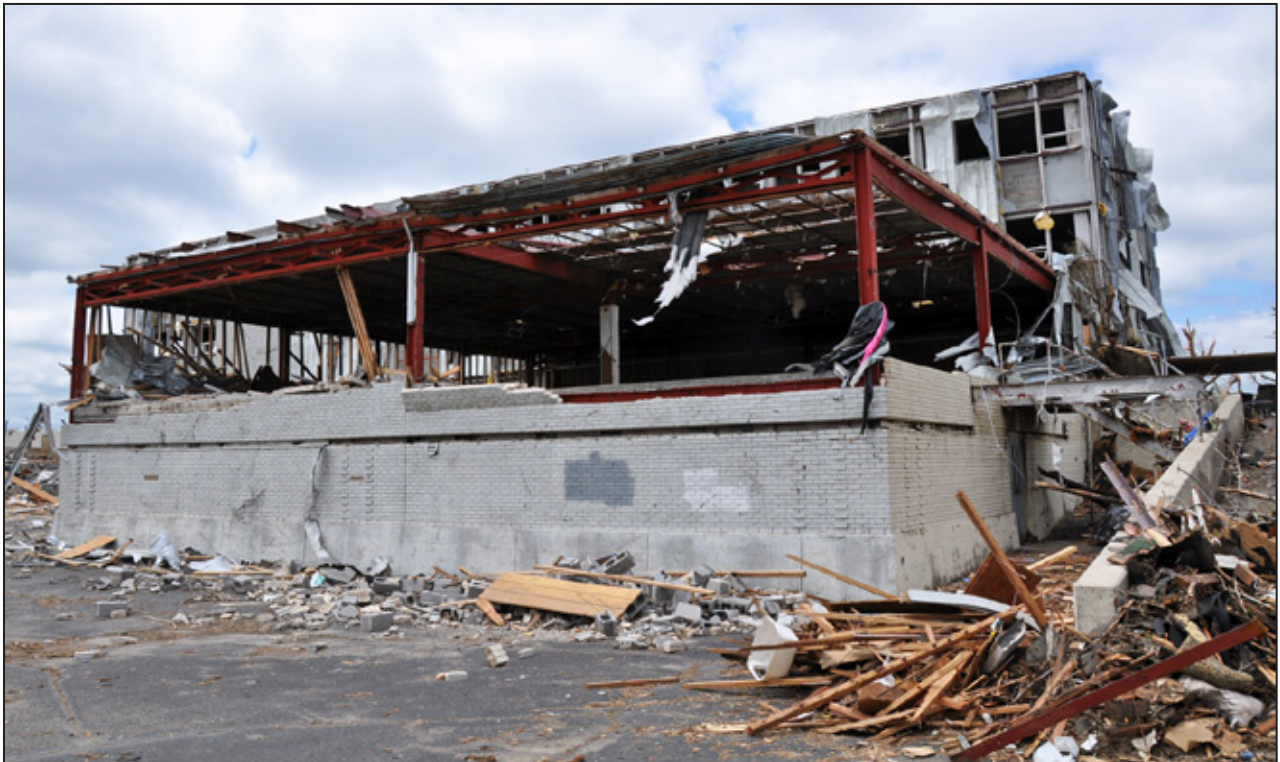
Figure 5-56: East elevation from northeast corner of building. The structural core of the taller building performed well, as did the CMU infill. The wing in the nearside of the figure is a two-story extension. Wood wall-framing debris can be seen in the foreground (Joplin, MO).
