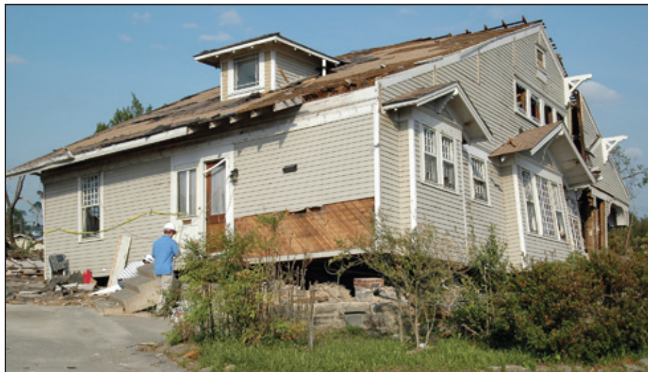
Figure 4-17: Example of DOD 5 showing residential building shifted off masonry piers (Cullman, AL) [MAT EF Rating = 2]
