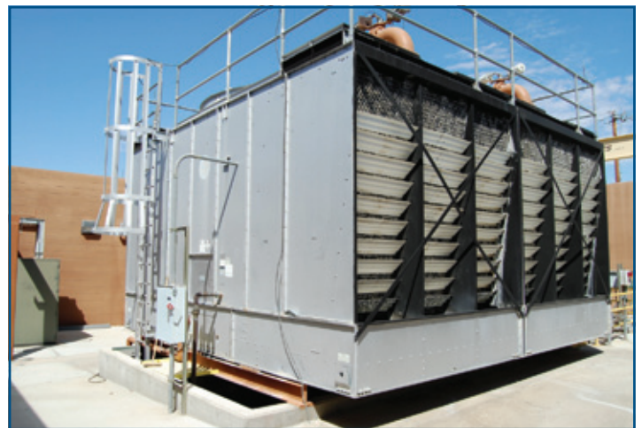
Figure 11: Cooling tower vulnerable to wind and wind-borne debris
