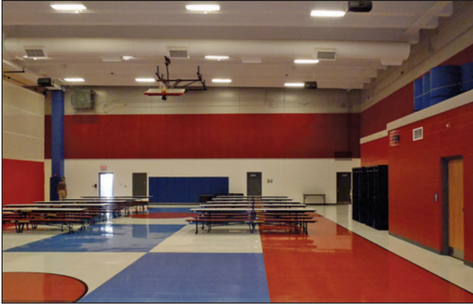
Figure 9-41: Seneca Intermediate School safe room in the cafeteria
