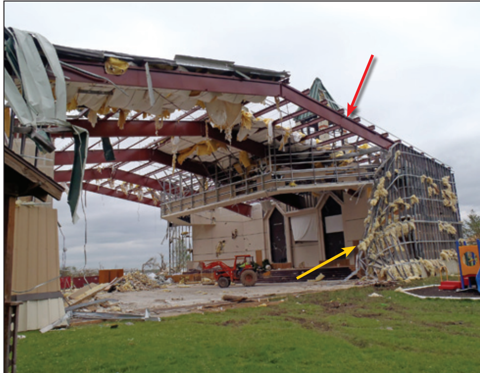
Figure 5-53: Secondary framing (light gage infill walls) failed (yellow arrow) while the main frames survived (red arrow) (Joplin, MO)
