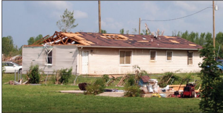
Figure 4-16: Example of DOD 4 showing damage to gable end of simple gable roof (Harvest, AL) [MAT EF Rating = 1]
