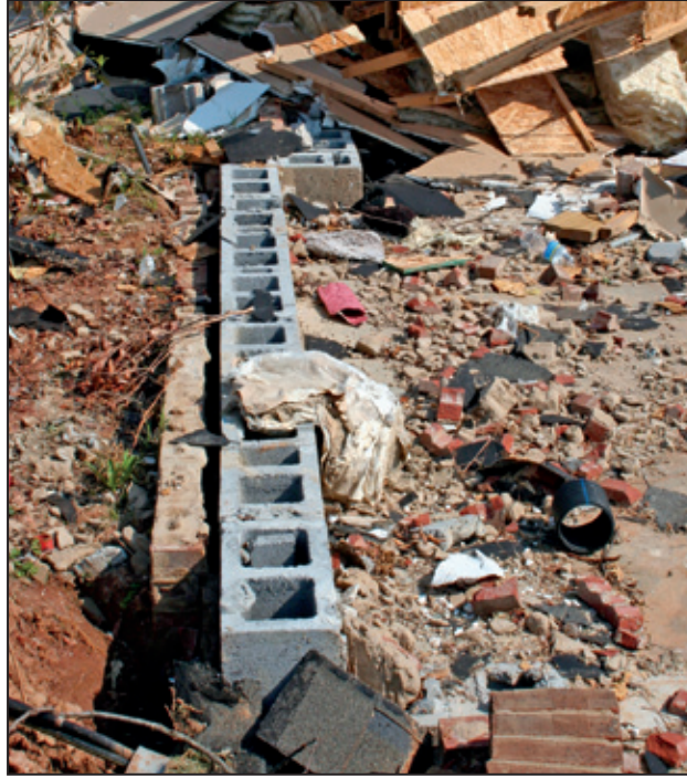
Figure 4-27: Example of wall framing- to-foundation connection failure. Wall and bottom plate separated from foundation where anchorage of collapsed framed wall failed because anchors lacked embedment in grout. Note CMU wall with no reinforcement or solid grout (Harvest, AL). [MAT EF Rating = 2]
