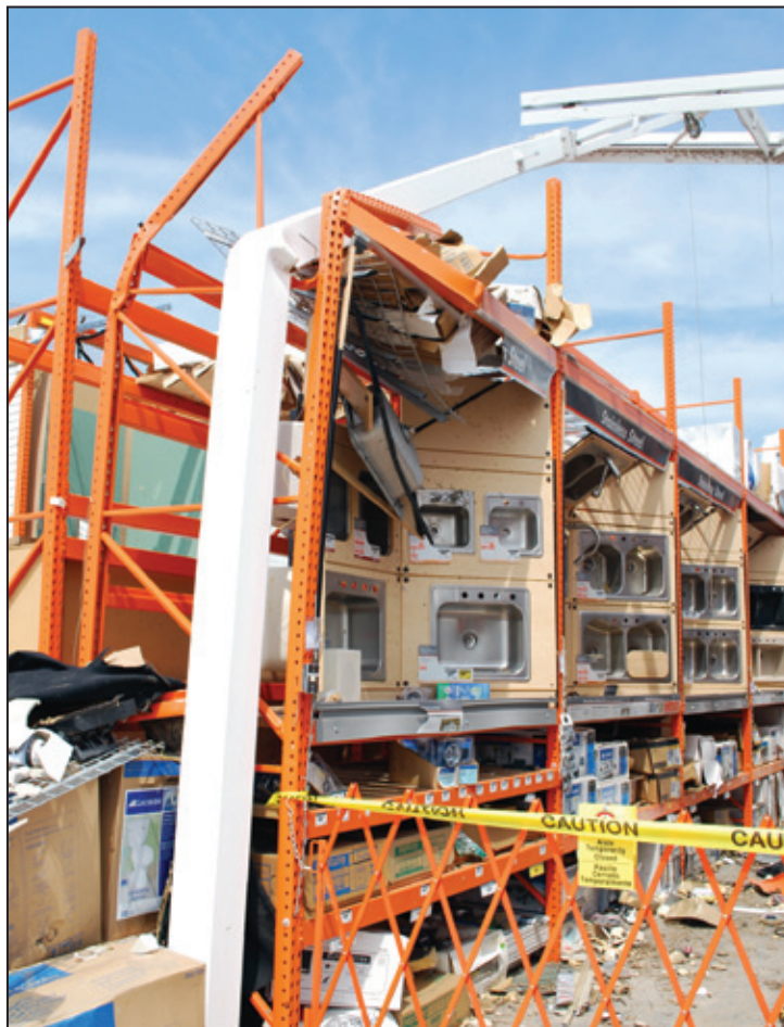
Figure 5-9: Buckled column (Joplin, MO)
