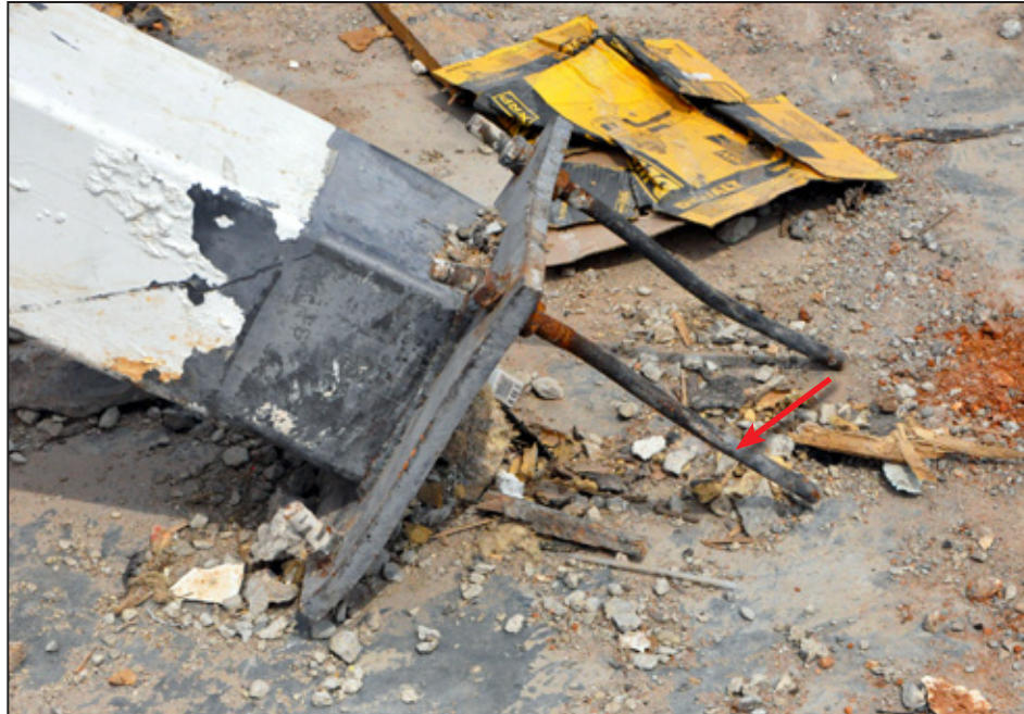
Figure 5-10: Bolt failure at interior column resulting from shear and tension. The hooked anchor bolts pulled out of the slab (red arrow) (Joplin, MO).
