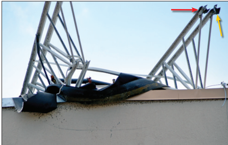
Figure 5-13: The joist seats came free of their bearing locations when both the seat-to-joist weld (yellow arrow) and the seat-to-embed plate weld (red arrow) broke (Joplin, MO)
