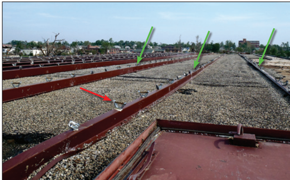
Figure 5-58: Roof of the third-story main building. The roof overbuild purlins are shown with green arrows while the roof clips that unlatched are shown by red arrow (Joplin, MO).
