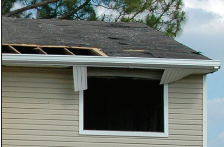
Figure 4-13: Example of DOD 4 showing where roof decking lifted and blew off above damaged soffit in roof Zone 2 (see Figure 4-12) (Birmingham, AL) [MAT EF Rating = 2] 4
