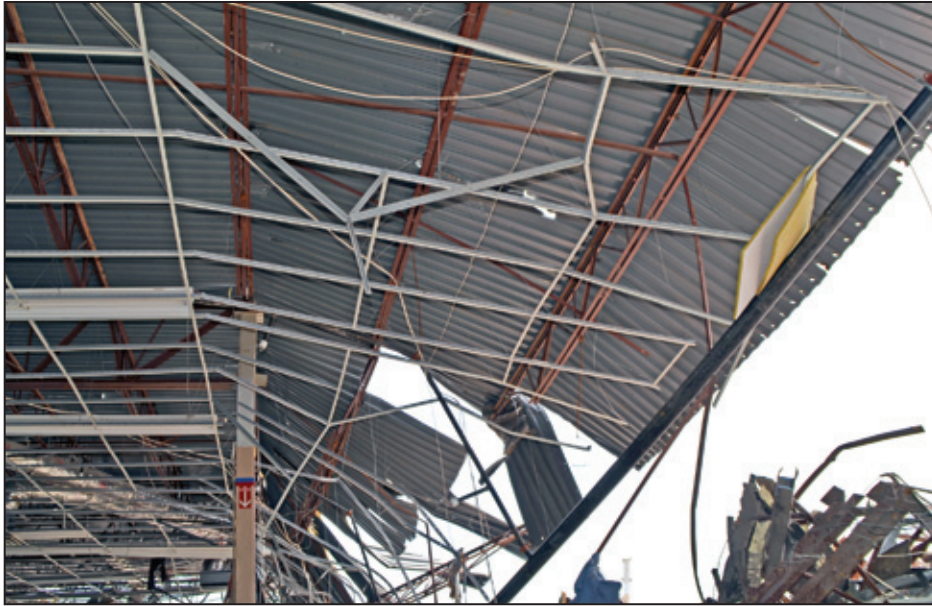
Figure 5-36: Interior view from the south half of the building looking toward the east. This shows the boundary of roof damage to the south portion of the building. Note deck supported by steel joist (Joplin, MO).
