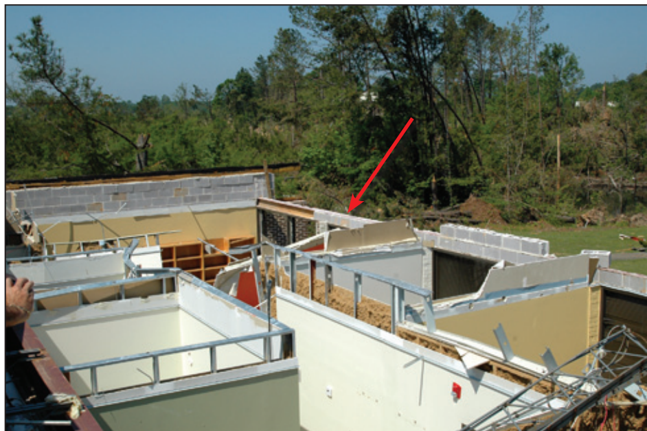
Figure 5-25: Failed bond beam-to- structural steel connection over front windows (red arrow) (Birmingham, AL)
