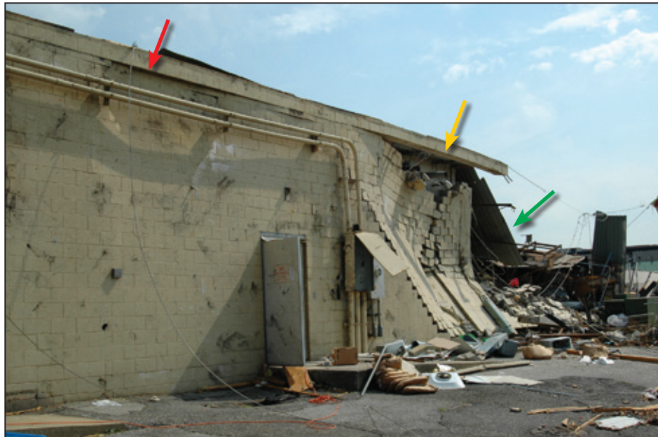
Figure 5-20: Sequence of failure for CMU wall at the dry cleaner building: wall buckling and initial separation (red arrow) was followed by complete separation of wall from bond beam (yellow arrow) and then by collapse of wall (green arrow) (Tuscaloosa, AL)
