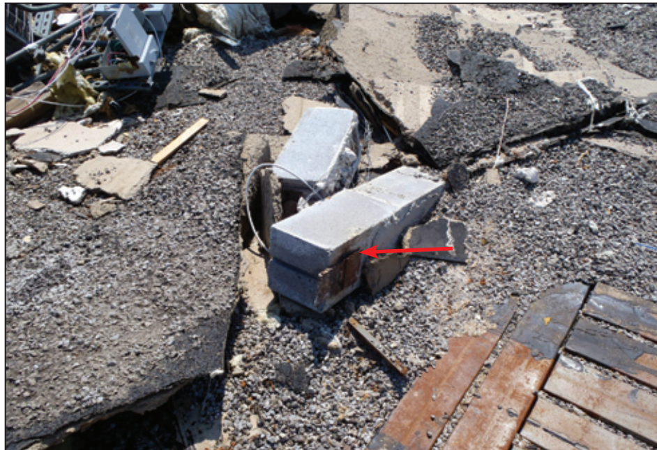
Figure 5-30: Embed plate with bond beam cell (red arrow) on roof (Birmingham, AL)
