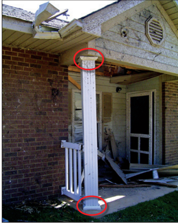
Figure 4-34: One-story Chastain Manor Apartment unanchored porch column that rotated at top and bottom of column (red circles)
