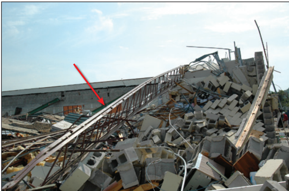
Figure 5-18: Steel joist (red arrow) in midst of collapsed unreinforced masonry wall at the dry cleaner store (Tuscaloosa, AL)
