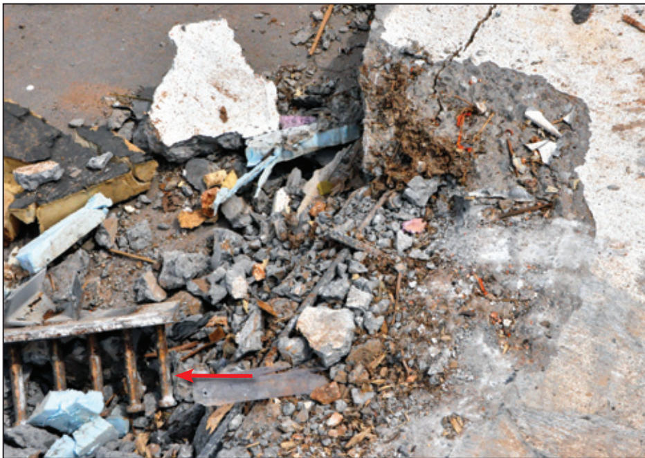
Figure 5-15: The panel at the weld plate failed (red arrow) (Joplin, MO)
