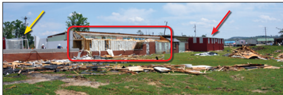
Figure 7-47: View of the back of the building. The old apparatus bay is shown by the yellow arrow and the new bay by the red arrow. Roof structure and wall damage occurred within the red box. The debris in the foreground is from the multipurpose room roof and the old apparatus bay (Wellington, AL).
