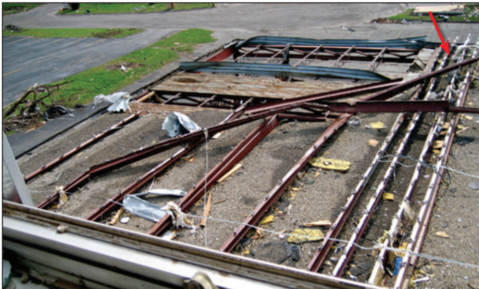
Figure 5-60: View of roof of the two-story extension observed from the third floor. Note the failed decking at the corner (red arrow) (Joplin, MO)
