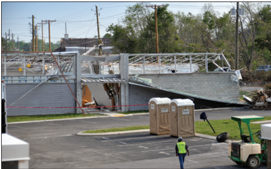
Figure 6-31: The roof covering was blown off of the 2008 art center. The metal wall covering and insulation was also blown off the CMU. The art center was subsequently demolished (Ringgold, GA).
