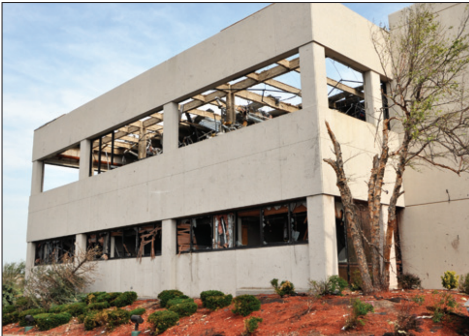
Figure 7-26: Metal decking blow-off and glazing damage in the administrative area (Joplin, MO)
