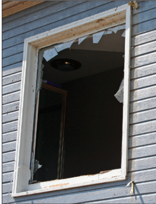
Figure 4-7: Example of DOD 3 showing window with shattered double-glazing (Harvest, AL) [MAT EF Rating = 2] 1
