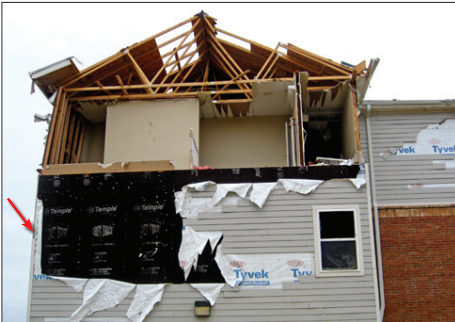
Figure 4-44: Damage to the gable end wall at south stair tower end. Note third floor wall is missing and second floor wall is bowed outward (red arrow).
