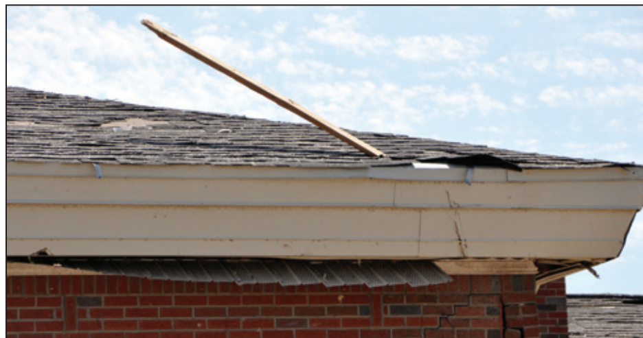
Figure 3-8: Medium-sized missile that struck the roof of a school building (Tuscaloosa, AL)
