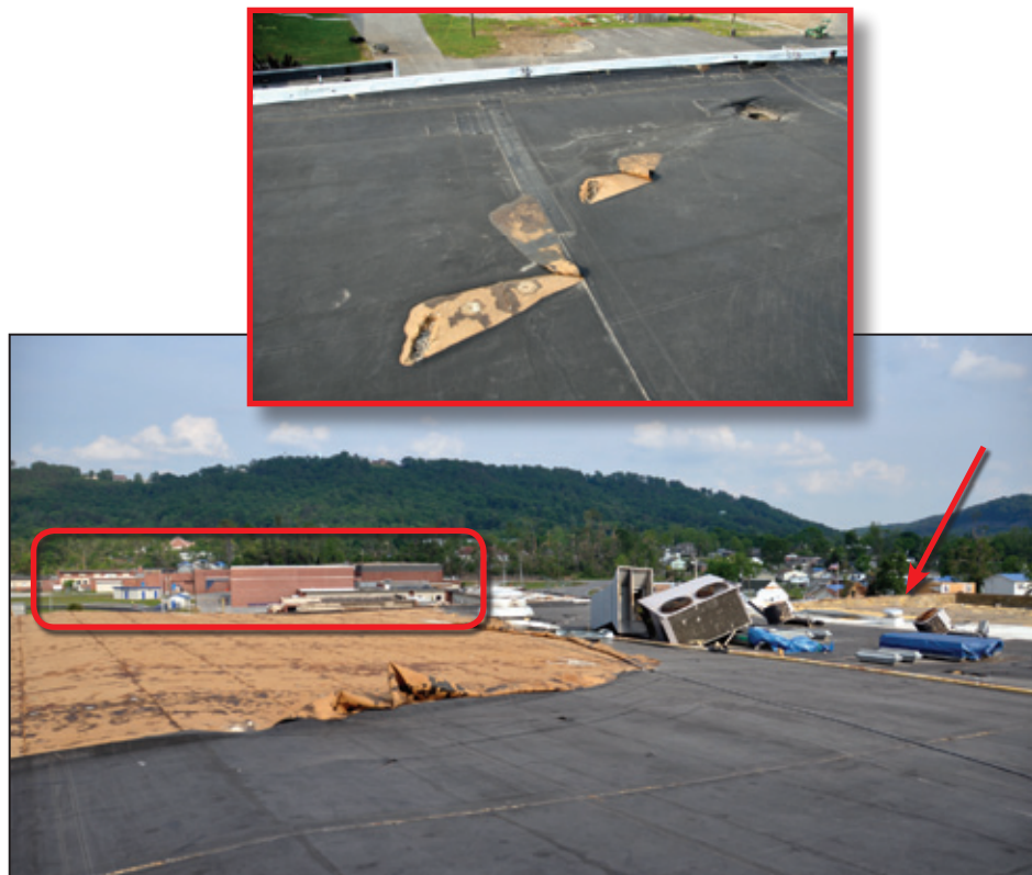
Figure 6-27: View of the two gymnasium roofs. The red arrow shows the 2008 auxiliary gymnasium (see also Figures 6-26 and 6-28). The EPDM (black) membrane is over the original gymnasium. Note the displaced rooftop equipment. The red box shows a portion of the middle school beyond. The inset shows wind-borne debris damage to the EPDM roof (Ringgold, GA).
