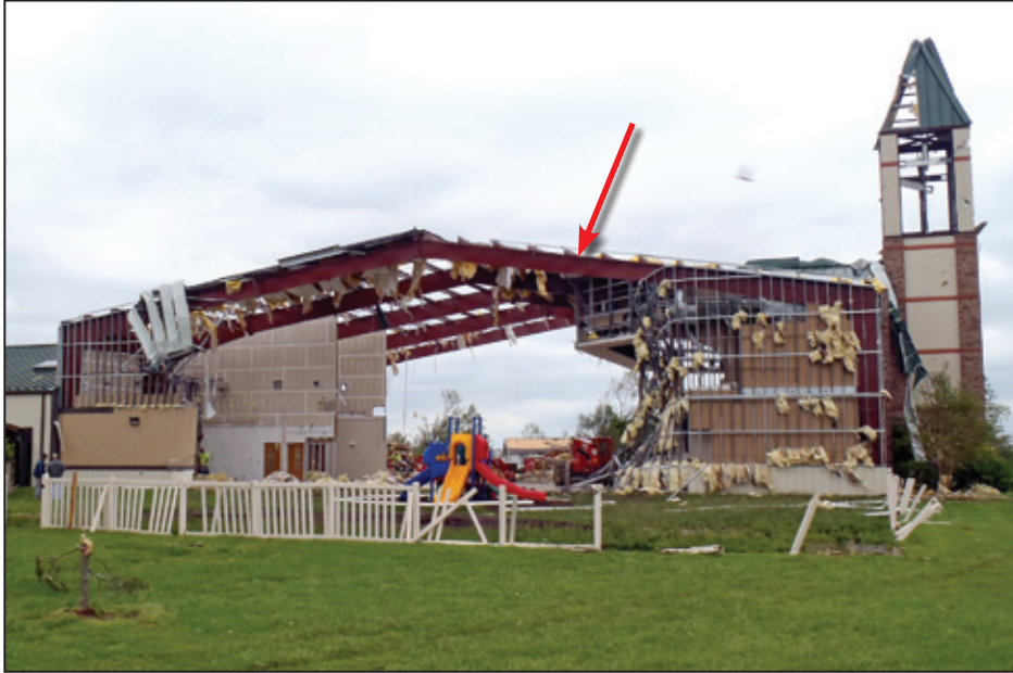
Figure 5-51: Intact PEMB main frames (red arrow) (Joplin, MO)
