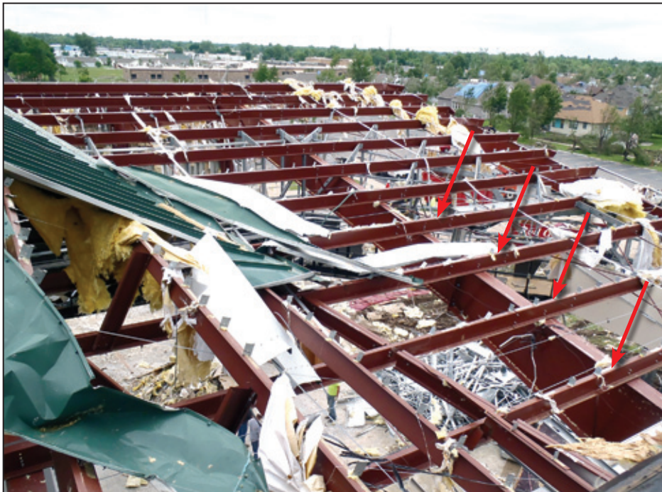
Figure 5-52: Roof system purlins intact with metal roof clip released (red arrows) (Joplin, MO)
