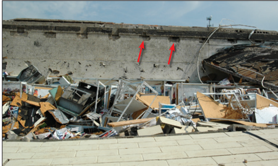
Figure 5-22: View of steel joist pockets in CMU wall where joists pulled out (red arrows); the exterior CMU wall fell inwards, shown in the foreground (Tuscaloosa, AL)
