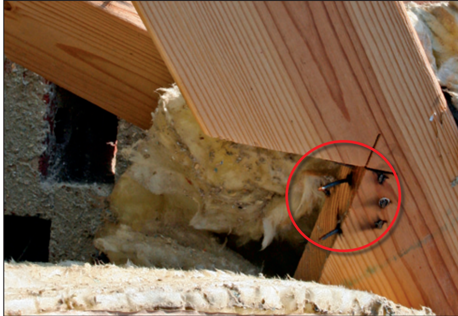
Figure 4-20: Over-notched rafter found on ground with two toe nails withdrawn from plate (red circle) (Harvest, AL) [MAT EF Rating = 1]
