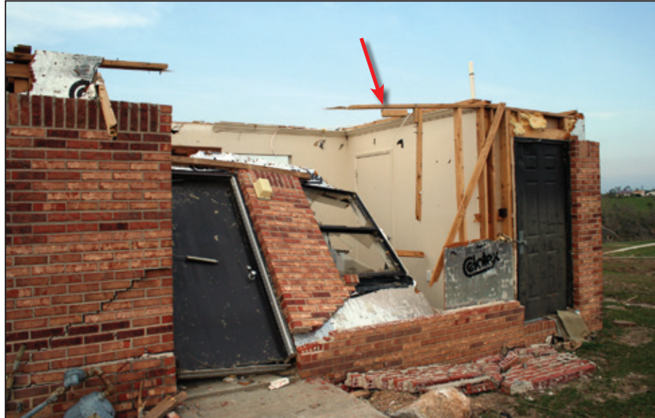
Figure 4-23: Example of DOD 6 showing failure of roof framing that resulted in loss of lateral support for the top of this wall (red arrow) (Phil Campbell, AL) [MAT EF Rating = 2]
