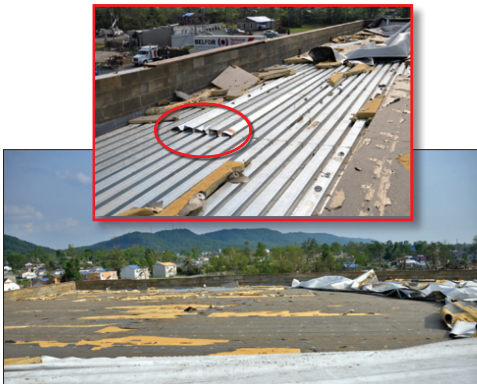
Figure 6-28: View of the roof of the 2008 auxiliary gymnasium (see also red arrow in Figure 6-27); inset shows lifted decking (red circle) (Ringgold, GA)
