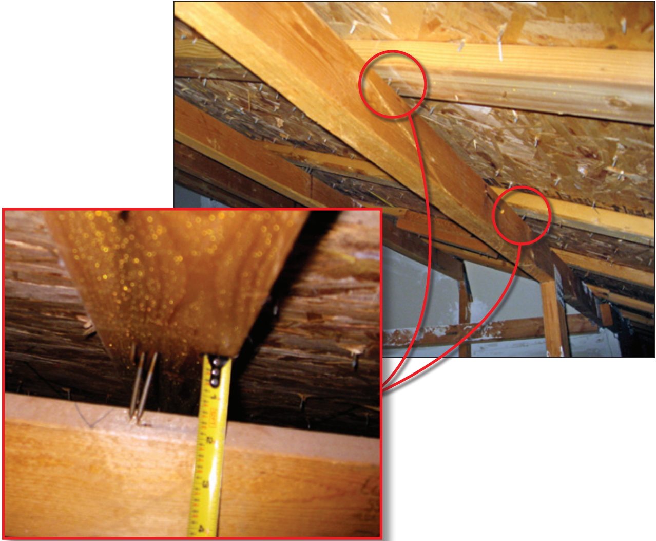
Figure 4-46: Nails through roof sheathing and nail plates have separated from roof trusses (red circles) because of wind pressures. Inset shows close-up of 2-inch nail withdrawal where nail plates separated from the roof truss.
