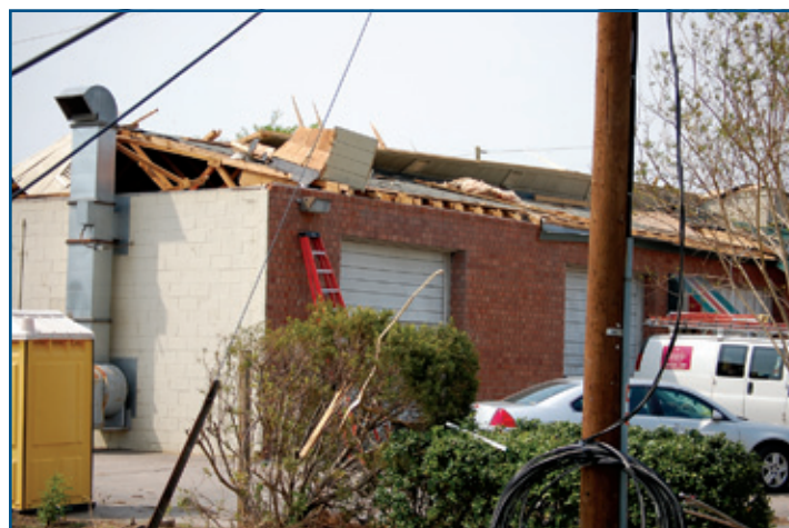
Figure 1: A business damaged by roof damage and water intrusion from a weak tornado
