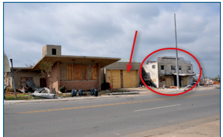
Figure 7: Fire station with a cast-in-place concrete roof deck in Tuscaloosa, AL. The apparatus bay doors (red arrow) collapsed and the adjacent building (red circle) was damaged (2011 Tornado).
