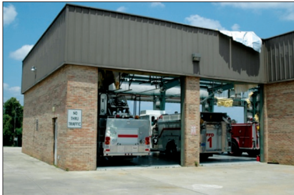
Figure 7-31: The apparatus bay doors of the fire department collapsed (Fultondale, AL)
