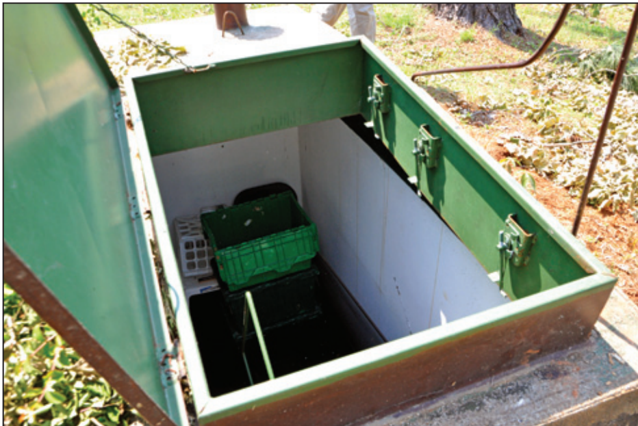
Figure 9-28: Below-ground FEMA- funded residential safe room (Tuscaloosa, AL)
