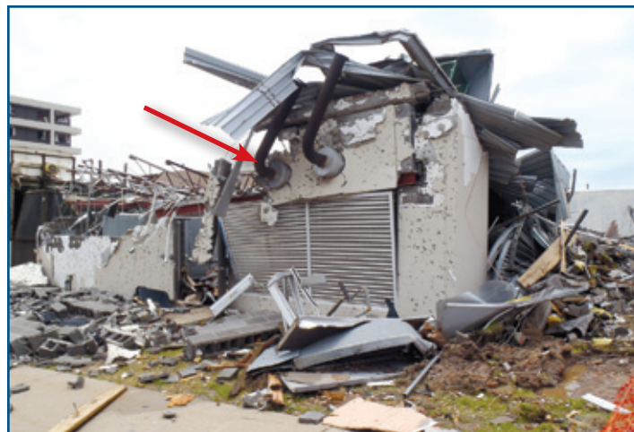
Figure 13: The steel deck/steel joist roof structure and unreinforced CMU walls of this Joplin, MO, building collapsed onto the emergency generator (2011 Tornado)
