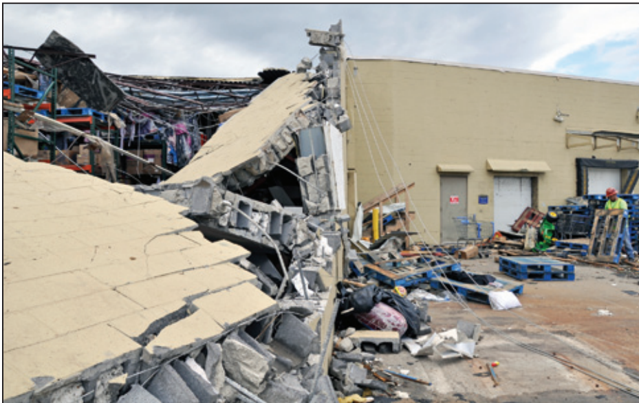
Figure 9-13: Close-up view of the damage at the Walmart store in Joplin, MO
