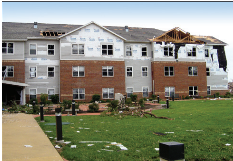
Figure 4-45: Damaged glazing on the interior courtyard of north wing building; majority of glazing was damaged
