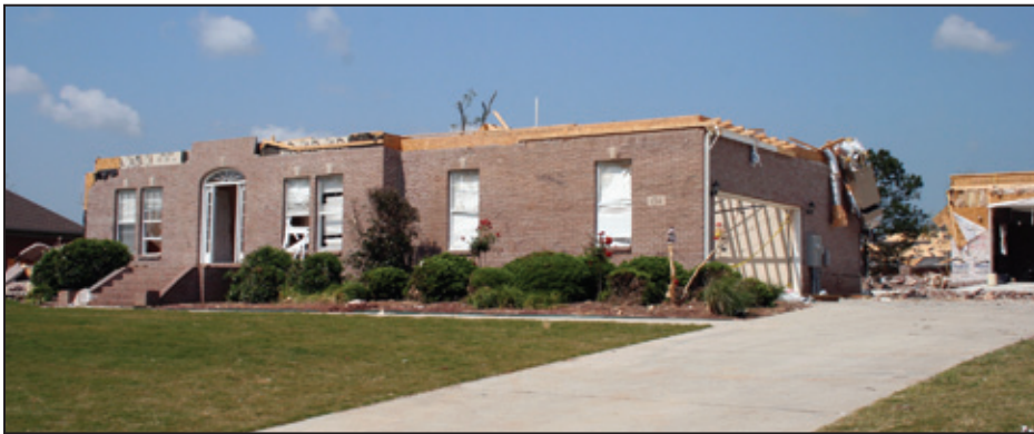
Figure 4-18: Example of DOD 6 showing failed roof-to-wall connections that resulted in loss of roof structure (Harvest, AL) [MAT EF Rating = 2]
