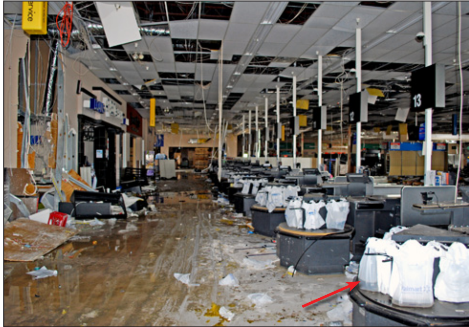
Figure 5-35: Interior of the north half of building showing water infiltration collected in bags (red arrow) (Joplin, MO)
