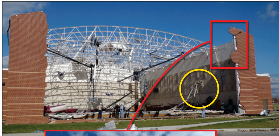
Figure 6-43: View of the gymnasium. The red box in the inset shows where the truss was attached to the wall. The yellow circle indicates the end of the collapsed truss shown in Figure 6-45 (Joplin, MO).
