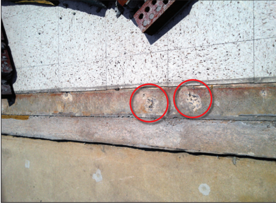
Figure 4-30: Wall-to-foundation failure where bottom plate and concrete nails were pulled out by high winds. Shallowly embedded concrete nails pulled small cones of concrete up with bottom plate (red circles) (Hackleburg, AL). [MAT EF Rating = 3]
