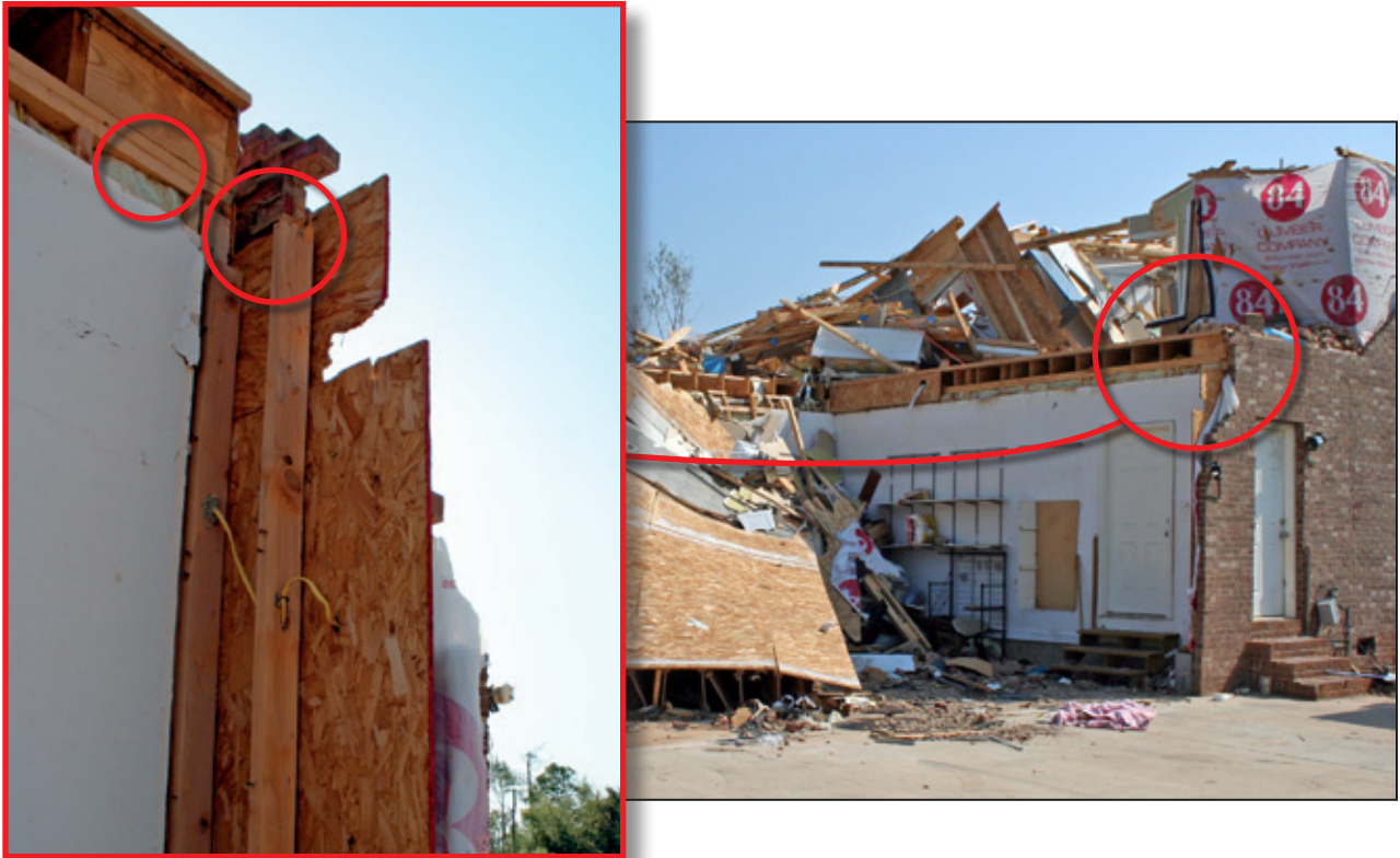
Figure 4-24: Example of DOD 6 showing pressurization of this garage from failure of the garage door/wall removed the support for the second story floor system (red circle). Inset shows where top plate of garage entry wall separated with floor or wall (red circles). Note former location of entry wall top plate—separated and missing from top of studs—is lower than the interior wall top plate due to deeper floor system (Harvest, AL). [MAT EF Rating = 2]
