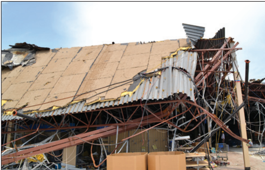
Figure 5-37: View of the south half of the building looking north showing roof damage. Note the missing roof membrane (Joplin, MO).
