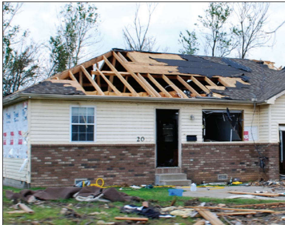
Figure 4-11: Example of DOD 4 showing roof decking blown off along eaves and hip (Zone 2 in Figure 4-12), where uplift pressures are greater than in the field of the roof (Joplin, MO) [MAT EF Rating = 2] 3
