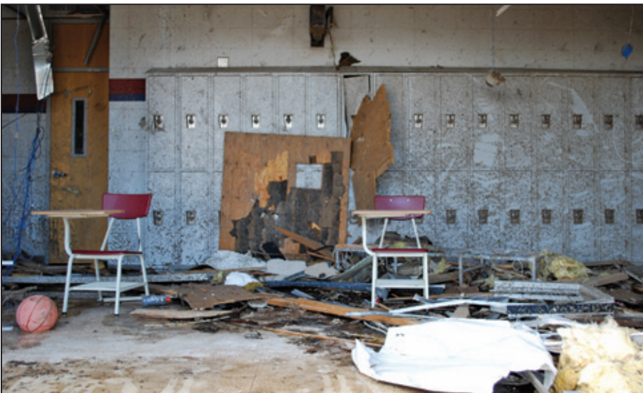
Figure 3-10: OSB damaged the first floor locker in Joplin High School (Joplin, MO)
