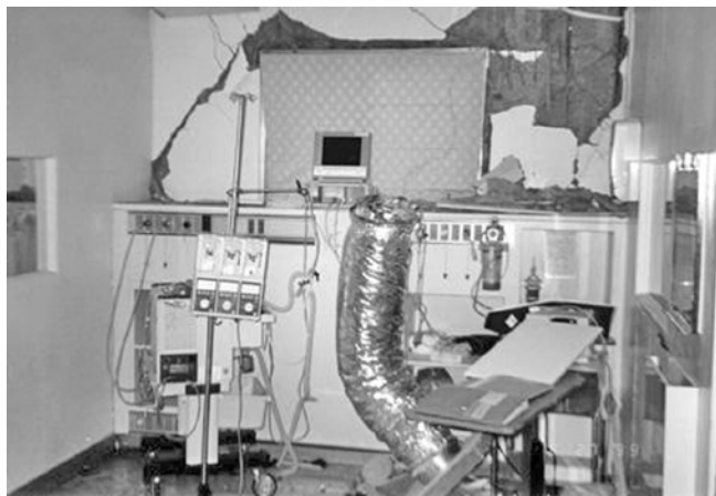
FIGURE C13.1-3 Collapsed Duct and HVAC Diffuser
