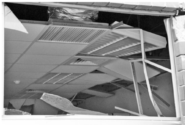
FIGURE C13.1-4 Damaged Ceiling System
