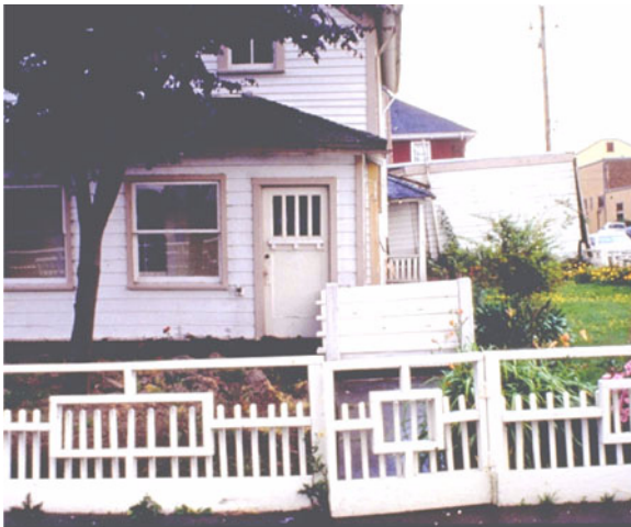
Figure F-10 This house has settled to the ground due to collapse of its post and pier foundation.
