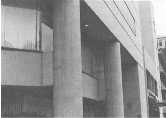
Figure E-42 Typical precast column cover on a steel or concrete moment frame.
