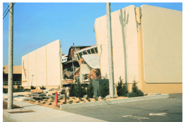
Figure E-39 Result of failure of the roof beam anchorage to the wall in tilt-up building.
