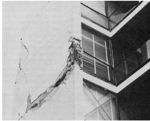
Figure E-22 Close-up of exterior shear wall damage during a major earthquake.
