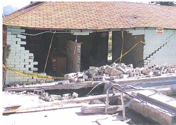
Figure E-54 Damaged URM building, 1992 Big Bear earthquake.
