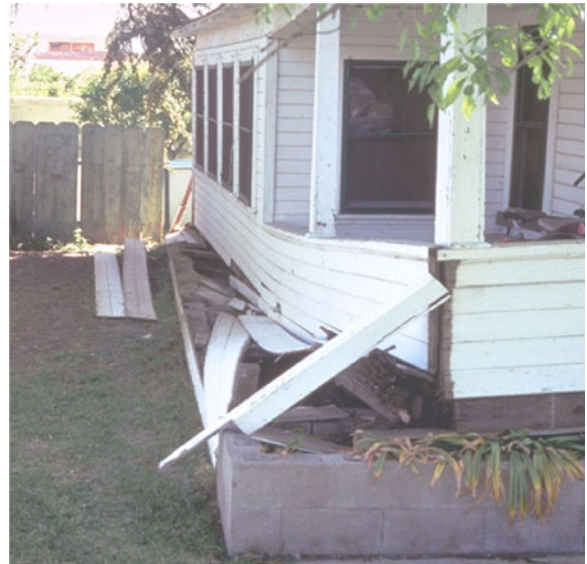
Figure E-7 House off its foundation, 1983 Coalinga earthquake.
