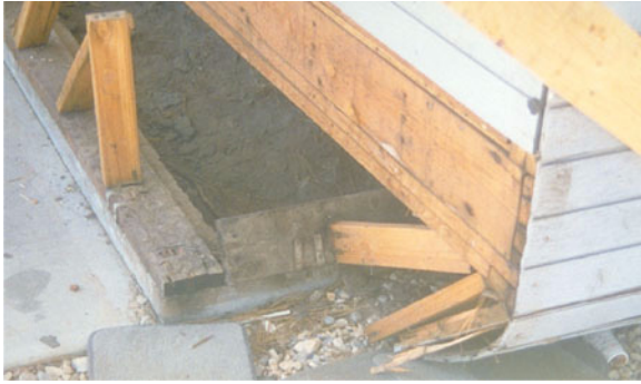
Figure E-8 Failed cripple stud wall, 1992 Big Bear earthquake.
