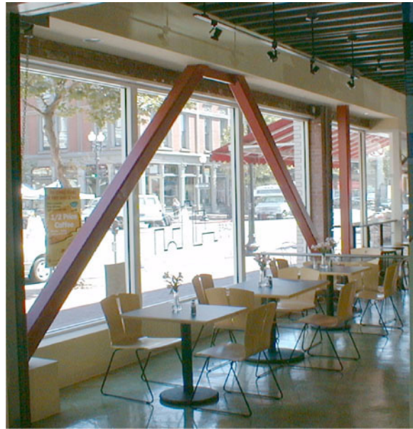
Figure E-16 Use of a braced frame to rehabilitate an unreinforced masonry building.
