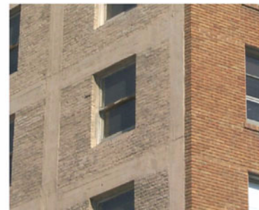
Figure E-34 Blow-up (lower photo) of distant view of C3 building (upper photo) showing concrete frame with URM infill (left wall), and face brick (right wall).
