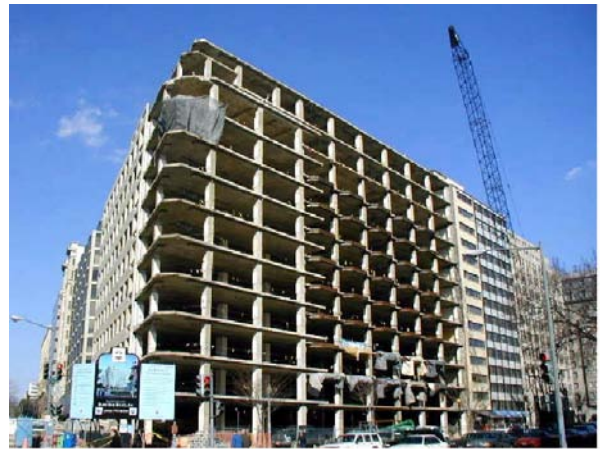
c. New precast facade units being applied to reinforced concrete frame buildings.
