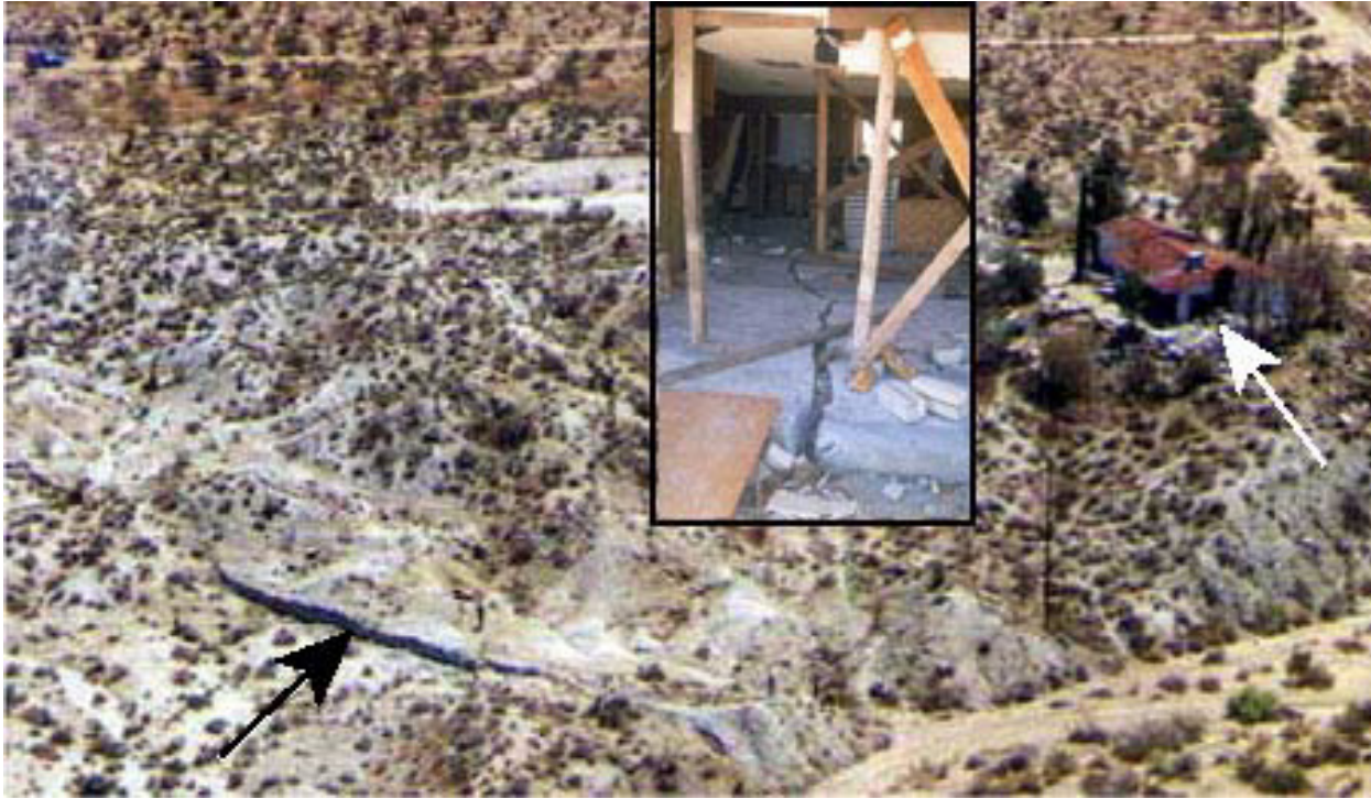
Figure F-6 Near-field effects, 1992 Landers earthquake, showing house (white arrow) close to surface faulting (black arrow); the insert shows a house interior.
