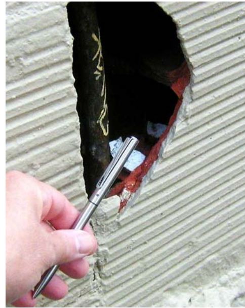
Figure D-14 Hollow clay tile wall with punctured tile.
