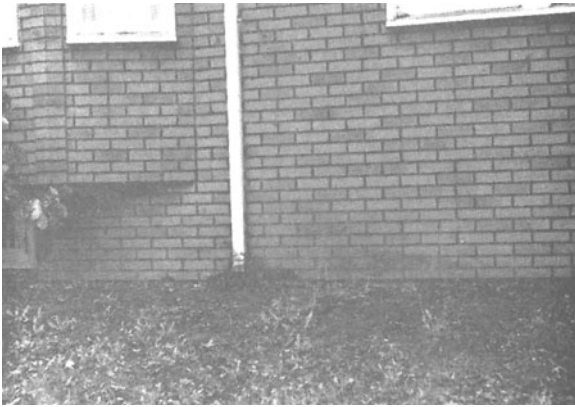
Figure D-16 Asphalt siding with brick pattern.
