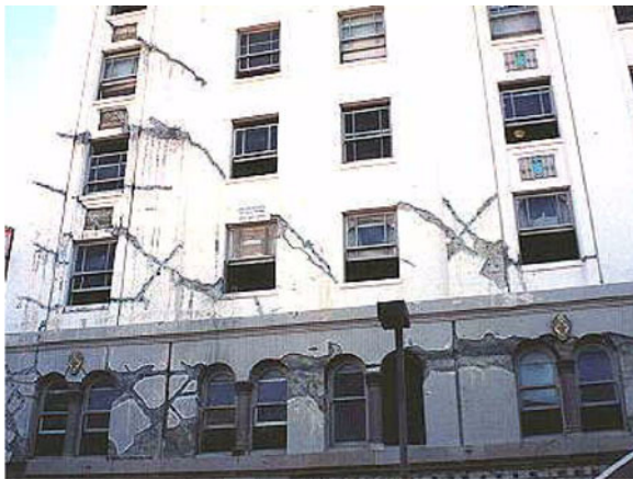
Figure E-32 Shear-wall damage, 1989 Loma Prieta earthquake.
