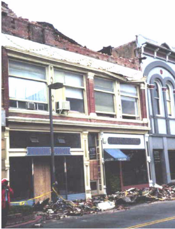
Figure E-53 Parapet failure leaving an uneven roof line, due to inadequate anchorage, 1989 Loma Prieta earthquake.
