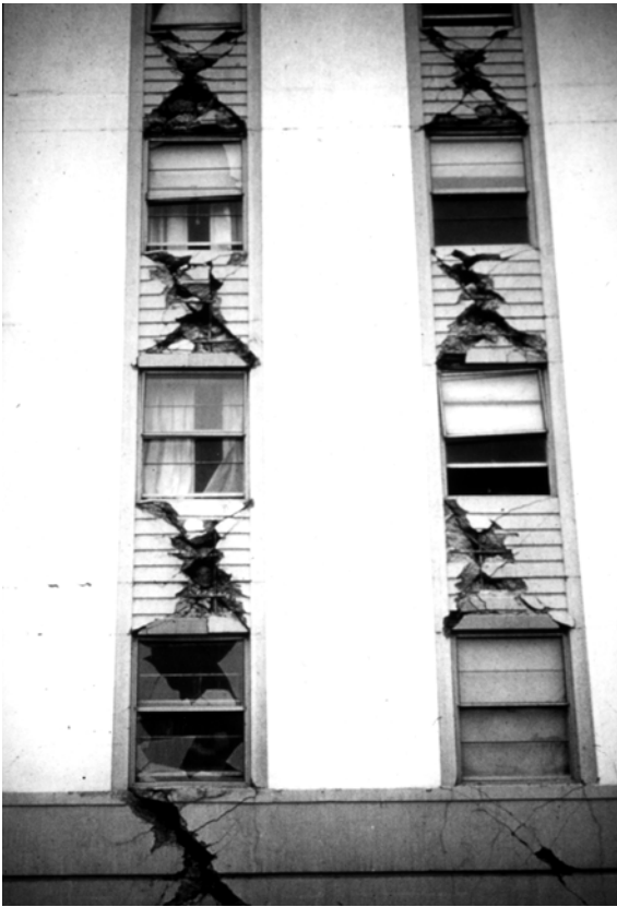
Figure E-31 Tall concrete shear-wall building: walls connected by damaged spandrel beams.
