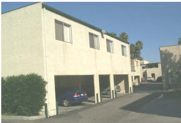
Figure 3-16 Example of soft story conditions, where parking requirements result in large weak openings.
