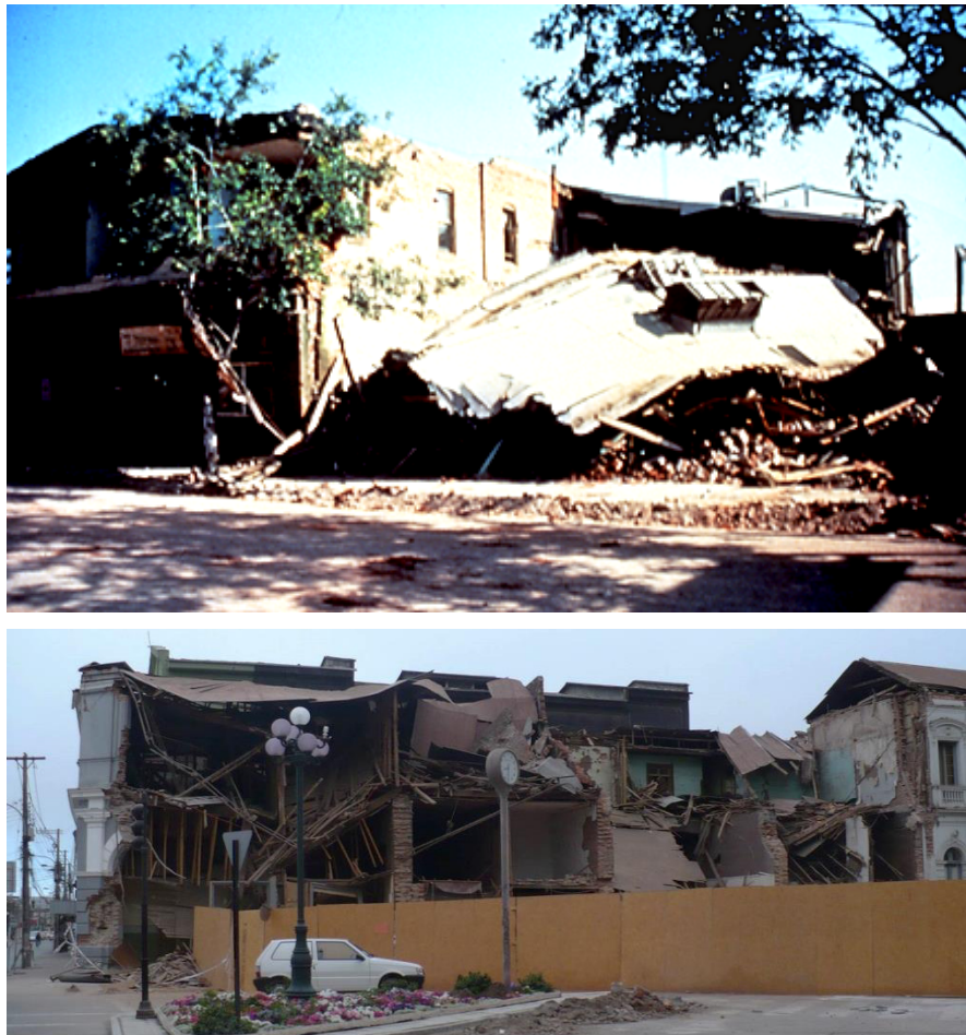
Figure 4-1 Examples of collapse and partial collapse.
