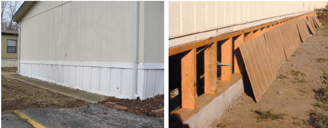
Figure 3-3 Photographs of a metal skirt and pony-wall perimeter covering systems.
