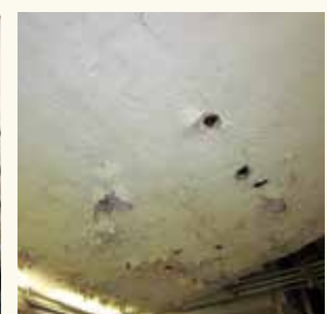
PHOTO 2: Ceiling damage resulting from roof leaks.
