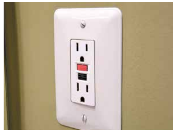
PHOTO: GFCI outlets are safer than other types of outlets in wet areas.
