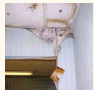
PHOTO 4: Mold behind vinyl wallpaper.
