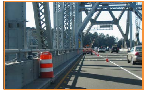
Deployment of a PTMD in a construction barrel in California to support traffic monitoring for bridge work.
