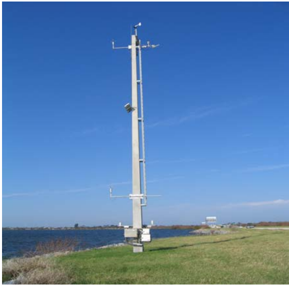
Figure 2. Road Weather Information System (RWIS) Environmental Sensor Station (ESS)
