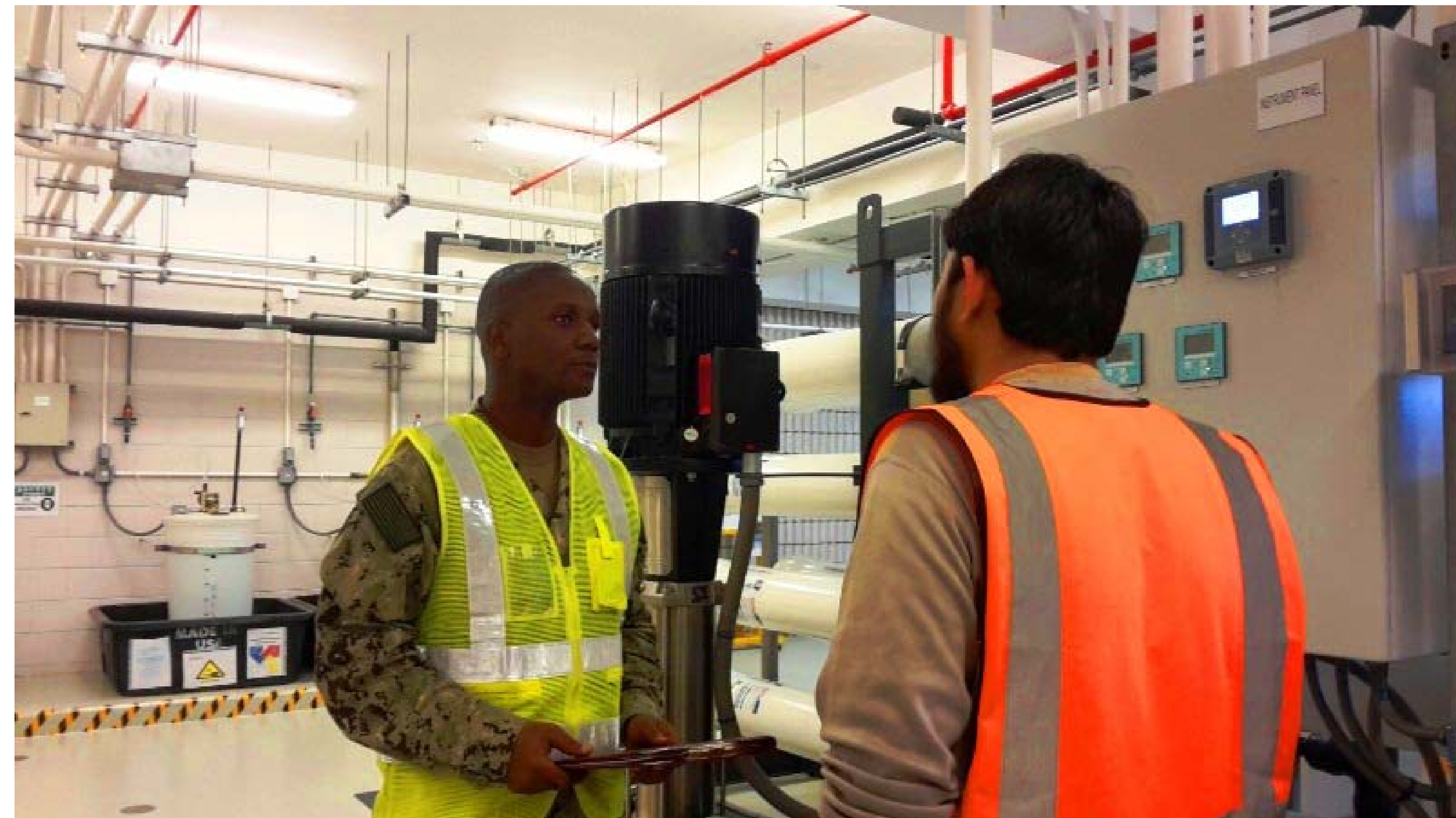
EA1 Sean Barezi listens as a G4S contractor explains reverse osmosis (RO) plant operation during his scheduled performance assessment. The RO plant supplies water for all of NSA 2; it is crucial that it is run efficiently and effectively. (U.S. Navy photo by NSA Bahrain/Released)
