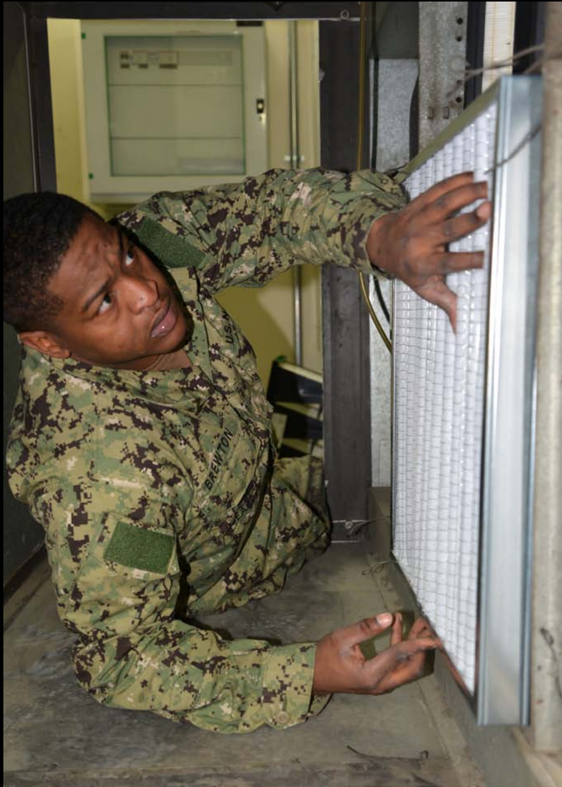
Construction Electrician Constructionman Apprentice Darien Brewton of Public Works Department (PWD) Naples, Italy replaces filters in the air handler units at Naval Support Activity Naples Feb. 4, 2015. PWD Naples provides a full range of NAVFAC construction, engineering, facility maintenance, utilities, transportation and environmental services to NSA Naples and tenant commands. (U.S. Navy photo by Mass Communication Specialist 2nd Class Eva-Marie Ramsaran/Released)
