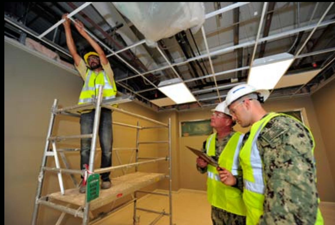
CE1 (SCW) John Hoodenpyle (left) and LTJG Erwin Rodriguez (right) perform a quality inspection on the acoustical ceiling installation at the new dry storage warehouse project at Camp Lemonnier, Djibouti, Africa. The new warehouse will provide increased covered storage, eliminating the need for CONEX box containers aboard Camp Lemonnier. (U.S Navy photo by MC1(SW/AW) Julia A. Casper/Released)
