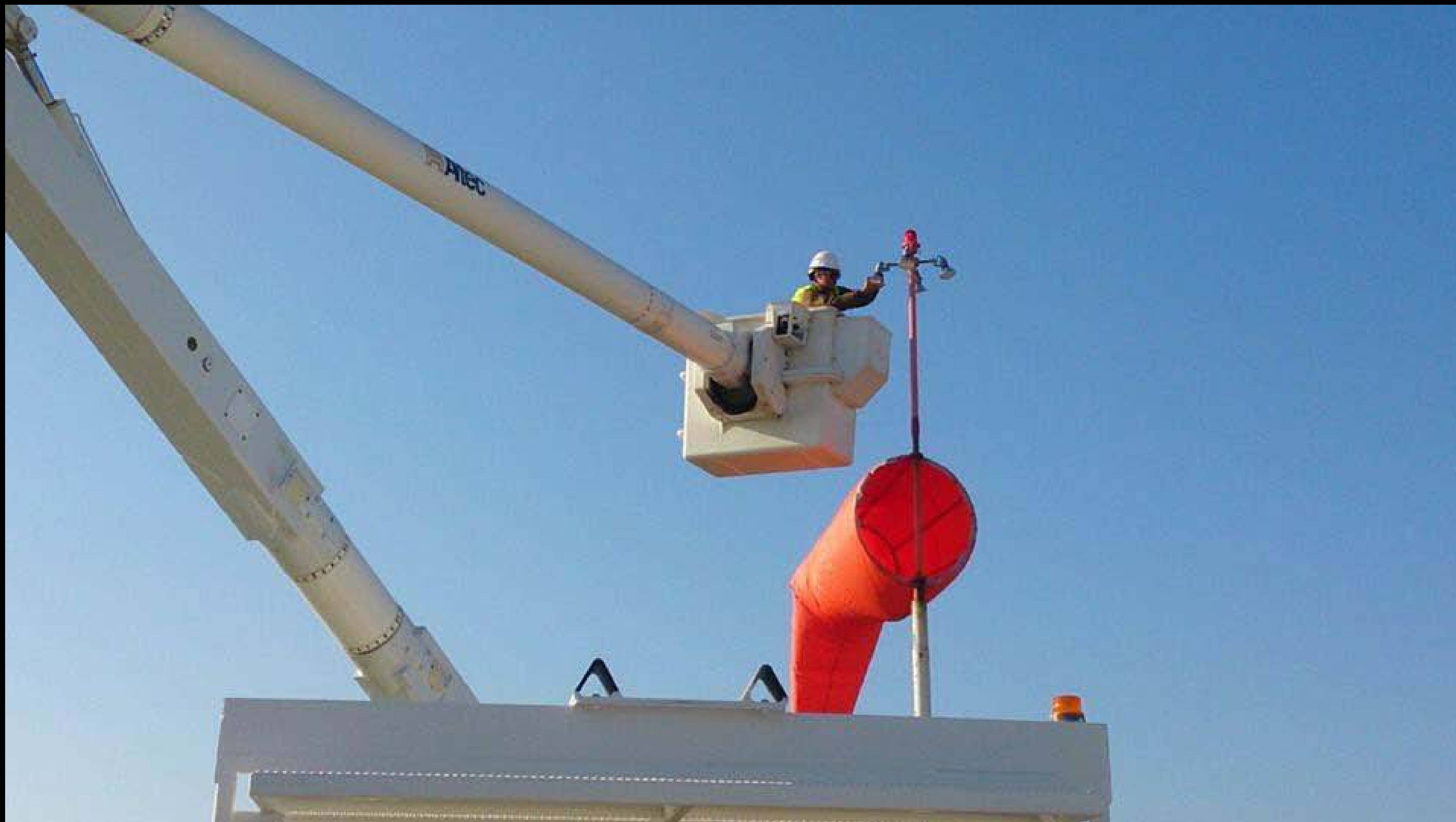
CE3 Daniella Acevedo Inspects Runway Approach lighting onboard Naval Station Rota, Spain in order to ensure continued operations. (U.S Navy photo by CMC Leslie Walton)
