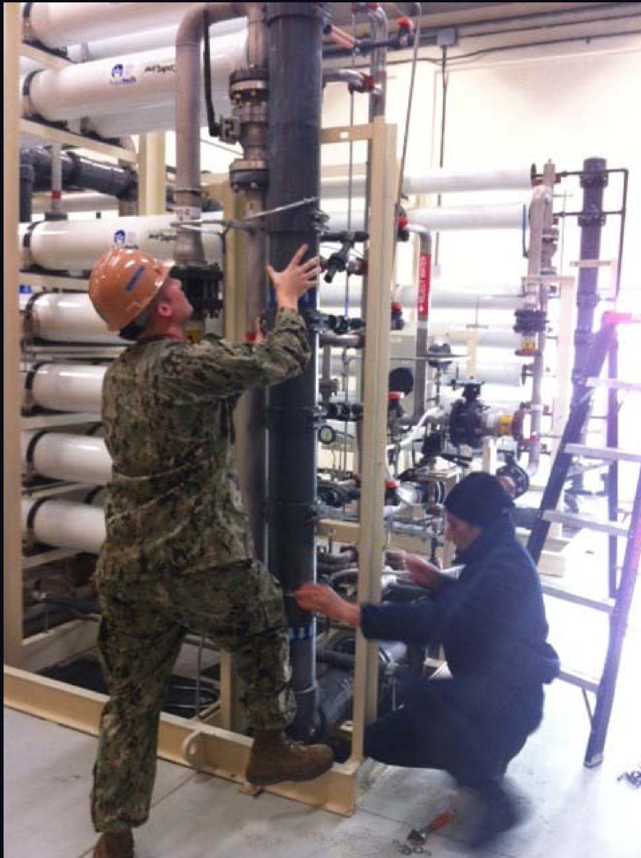
UTCA Books and Fabio Calabrese of the NASSIG PWD Plumbing shop begin the replacement of a ruptured six inch PVC pipe on the NAS 2 Water Treatment Plant's permeate line. The line was replaced with Electrofusion pipe which use special fittings that have built-in electric heating elements fusing the pipe together. (U.S Navy Photo by Utilitiesman 1st Class Daniel Goodwin/Released)
