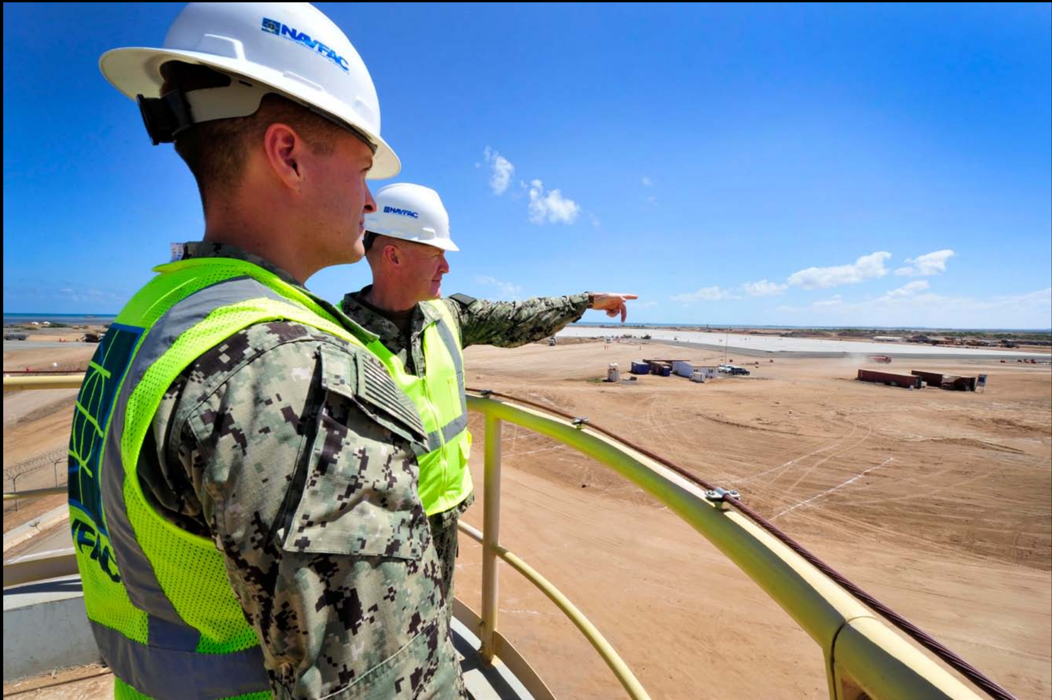
LTJG Jack Schenker and BUCS(SCW) Tom O'Connor inspect the Combat Armament Loading Apron project from atop a newly installed guard tower. The project installed 46 acres of 11 inch thick concrete to be used for aircraft parking. (U.S Navy photo by MC1(SW/AW) Julia A. Casper/Released)
