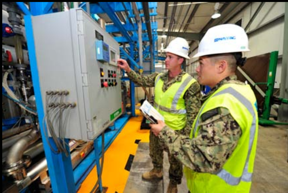
CE1 (SCW) Fernando Marquez (right) provides oversight of a relay installation for the power generation units at Camp Lemonnier, Djibouti, Africa. The 17 megawatt power plant supplies all Camp electricity ensuring mission accomplishment for the Camp and tenant commands. (U.S Navy photo by MC1(SW/AW) Julia A. Casper/Released)
