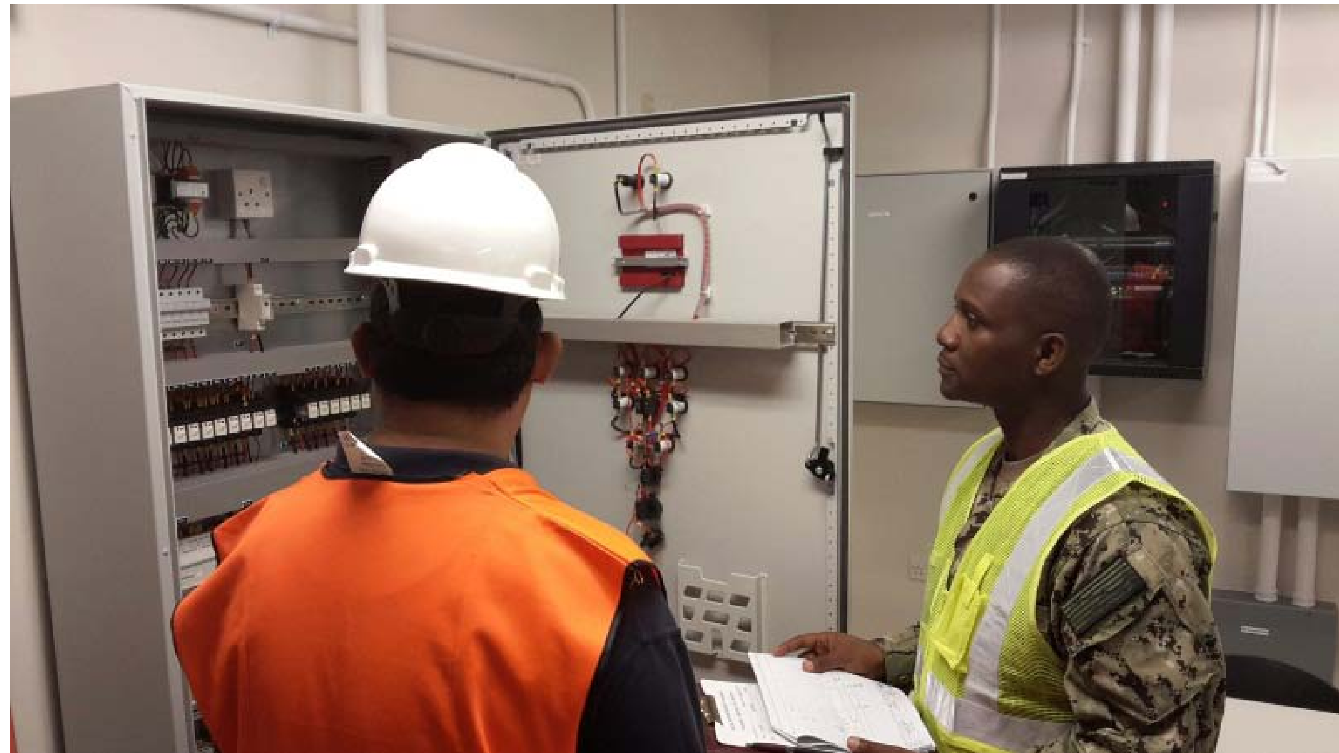
EA1 Barezi inspects the AHU-2 panel inside the Pass & ID building during contractor scheduled maintenance. G4S conducts weekly and monthly maintenance on HVAC equipment to ensure they are fully operational. The team is instrumental in the support of the 98 tenant commands onboard NSA Bahrain. (U.S. Navy photo by NSA Bahrain/Released)
