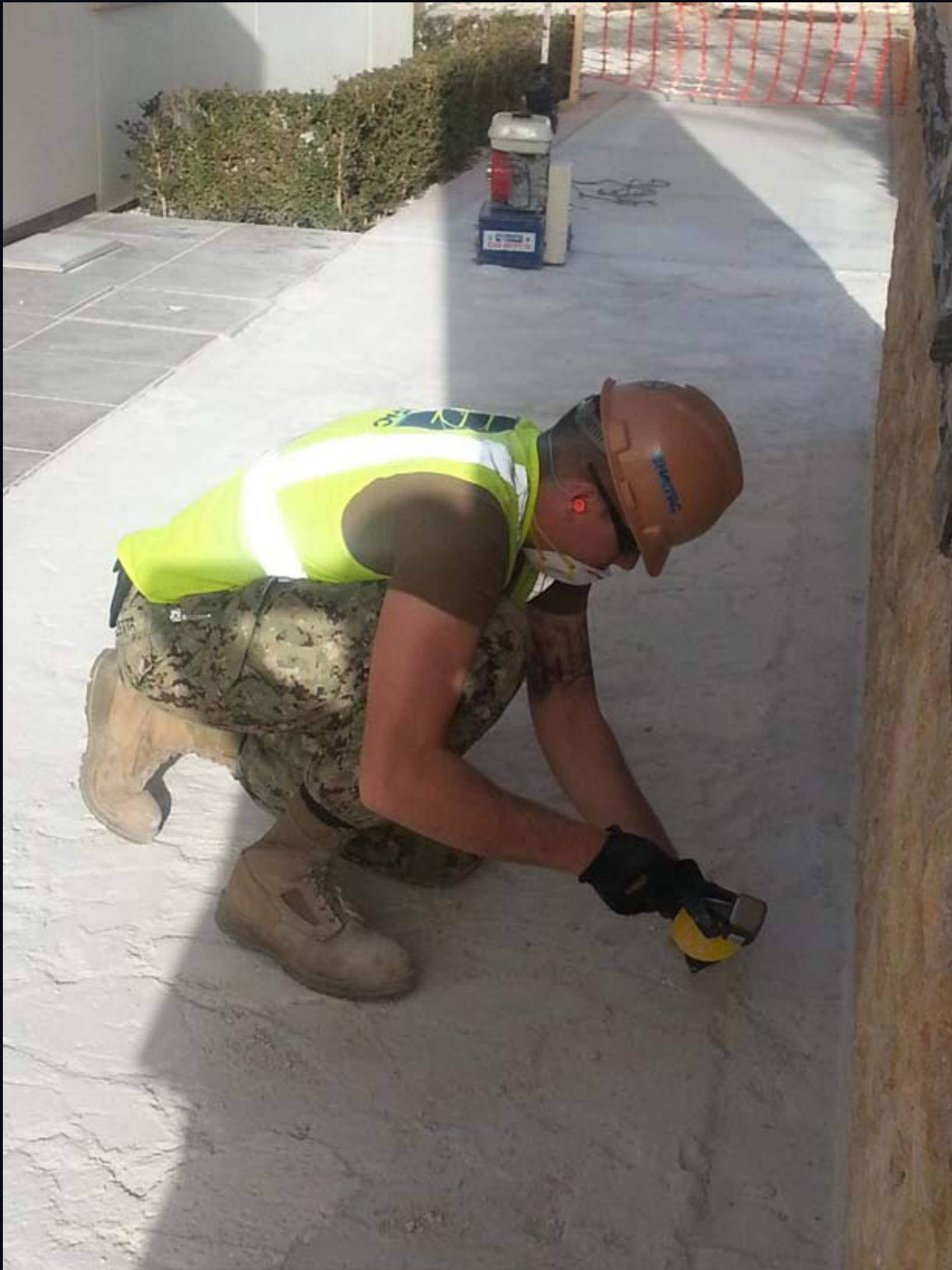
Crew Members from NSA Souda Bay's Public Works Department Builder shop Prepare Concrete surface at Building One for the placement of tile. (U.S. Navy Photo by BU2(SCW) Whittaker/Released)
