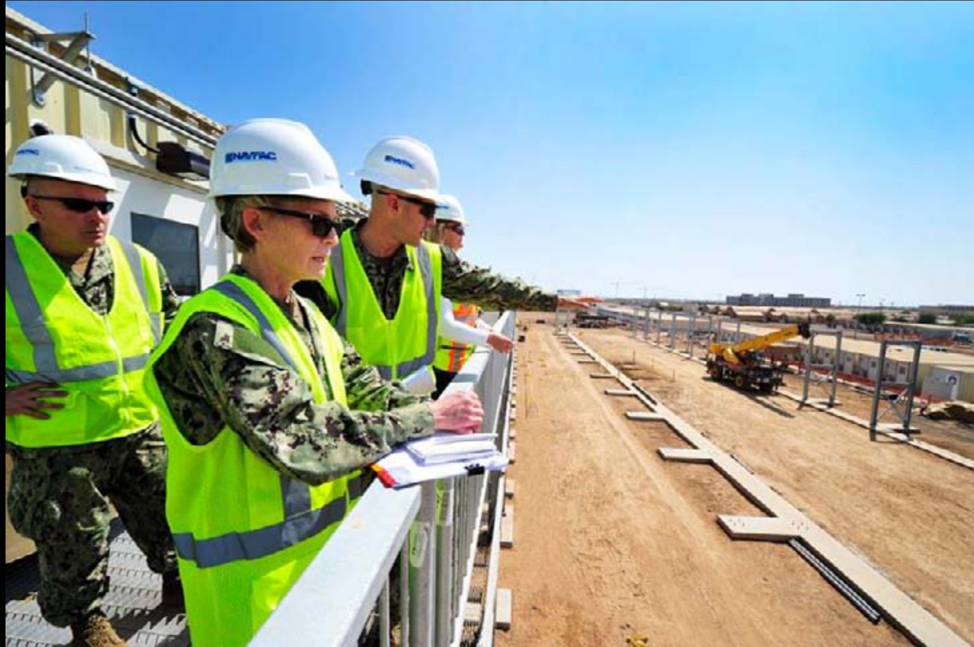
Chief of Civil Engineers, Rear Adm. Katherine Gregory, 2nd from left, discusses a building construction development plans with Lt. Erwin Rodriguez, a Camp Lemonnier construction site manager. Gregory and Seabee Force Master Chief Christopher Levesque are conducting site visits throughout the European Region to assess various engineering support facilities and bases. (U.S. Navy photo by Mass Communication Specialist 1st Class Julia A. Casper/Released)
