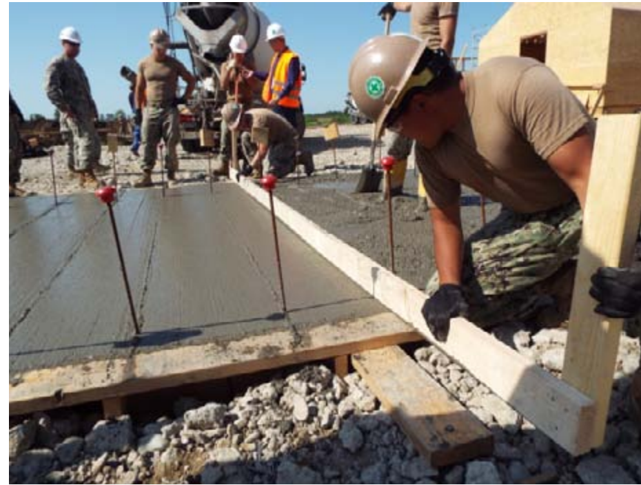
DEVESELU, ROMANIA -- Sailors level a cement foundation during construction of the base's land-based ballistic missile defense (BMD) facility. The BMD facility will utilize a system nearly identical to those used on Navy Aegis-capable guided missile destroyers and cruisers. (U.S. Navy photo by CTF-68/Released)
