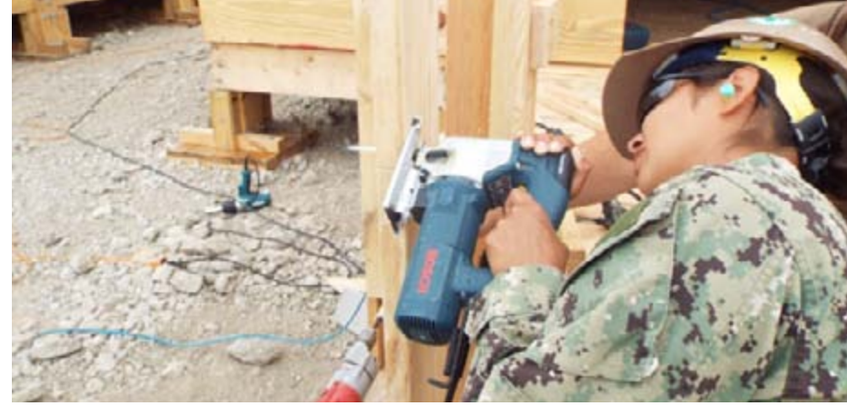
DEVESELU, ROMANIA -- A sailor cuts a stud during construction of the base's land-based ballistic missile defense facility. (U.S. Navy photo by CTF-68/Released)
