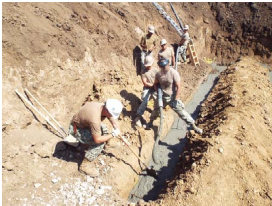
DEVESELU, ROMANIA -- Sailors pour cement during construction of the base's land-based ballistic missile defense (BMD) facility. The BMD facility will utilize a system nearly identical to those used on Navy Aegis-capable guided missile destroyers and cruisers. (U.S. Navy photo by CTF-68/Released)
