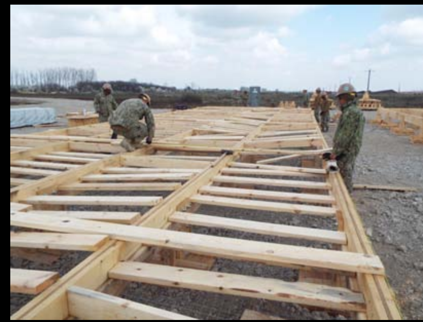
Builder 1st Class Jose Andino, right, assigned to Naval Mobile Construction Battalion (NMCB) 74, oversees the quality and progress of a project. Seabees from NMCB 74 are constructing a security force camp in support of the Aegis Ashore ballistic missile defense facility in Deveselu. (U.S. Navy photo by Utilitiesman Constructionman Sydney Thorne/Released)
