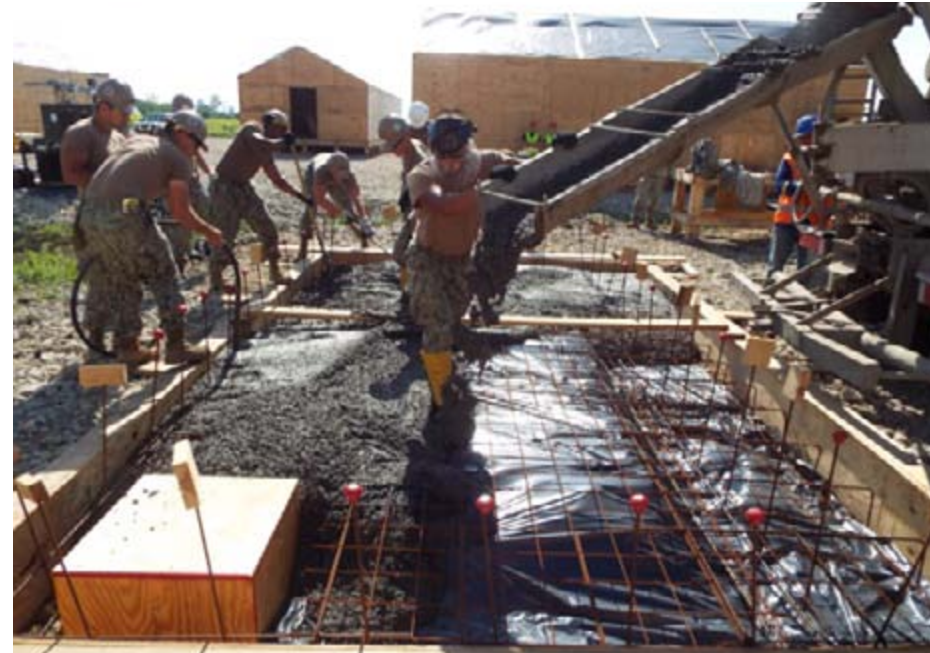
DEVESELU, ROMANIA -- Sailors pour cement foundations during construction of the the base's land-based ballistic missile defense facility. (U.S. Navy photo by CTF-68/Released)
