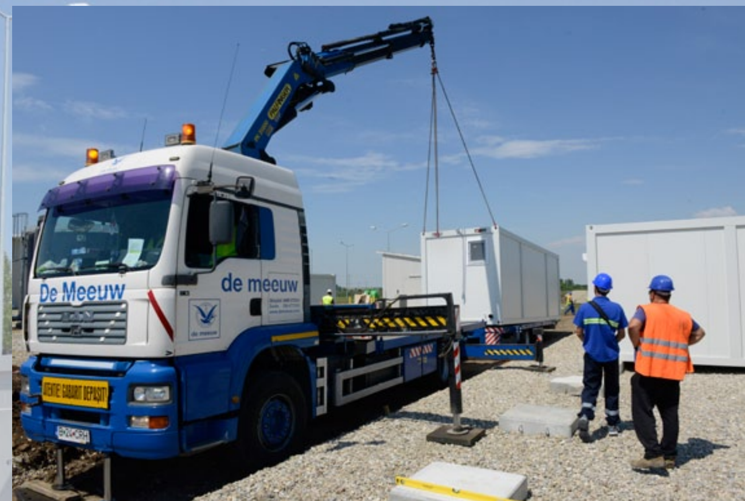
A contractor uses a truck-mounted crane to swing a containerized housing unit (CHU) into position at Naval Support Facility (NSF) Deveselu, Romania, June 10, 2015. The CHUs are single-occupancy units with a full bathroom, furnished like a small apartment, and will be continue in use as additional housing after the permanent installation housing/dining facility is completed later this year. (U.S. Navy photo by Lt. Cmdr. Mike Billips/Released)
