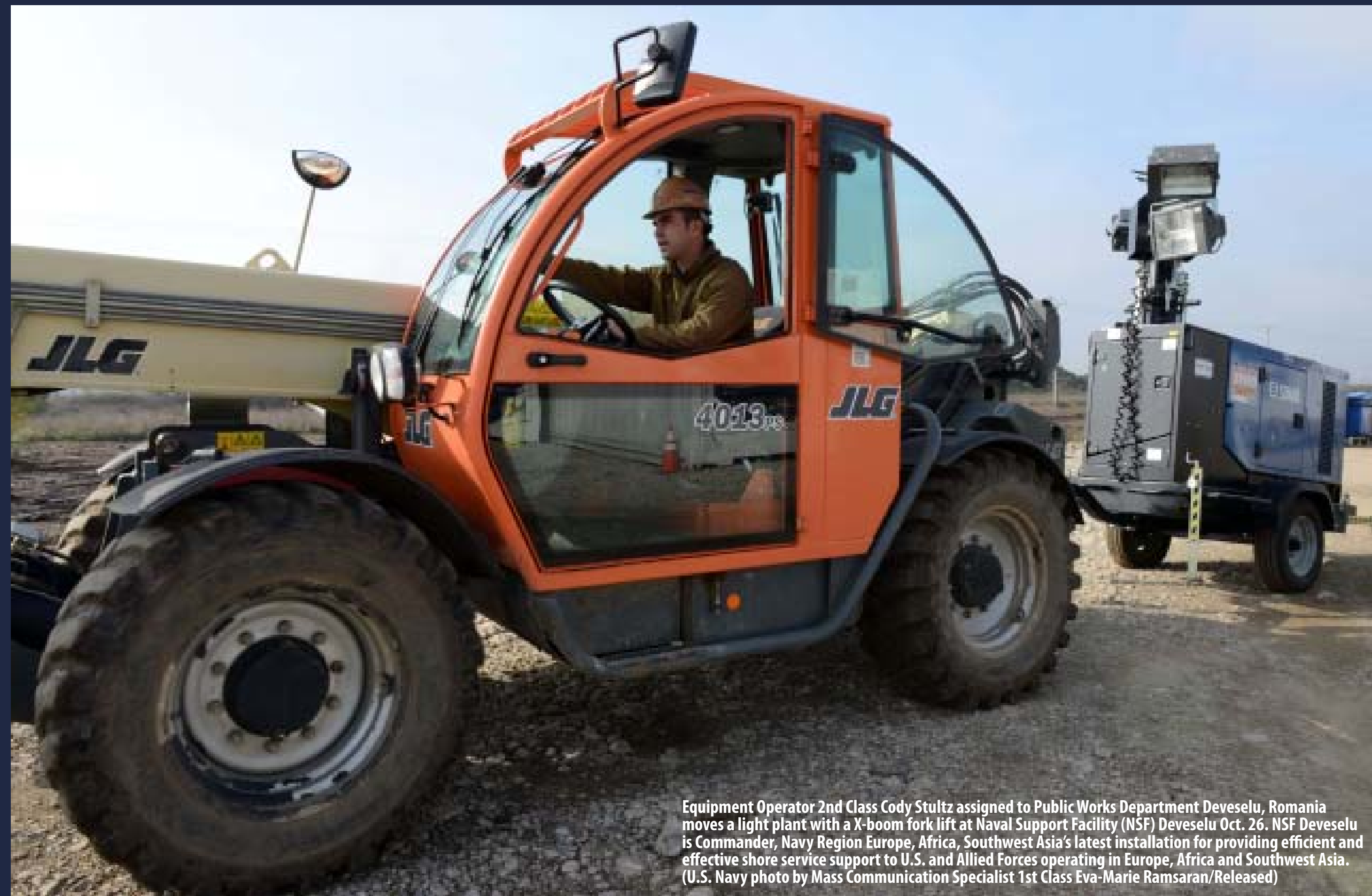
Seabees assigned to Public Works Department Deveselu, Romania work together to lift a light plant onto a X-boom fork lift hitch to be moved at Naval Support Facility (NSF) Deveselu Oct. 26. NSF Deveselu is Commander, Navy Region Europe, Africa, Southwest Asia's latest installation for providing efficient and effective shore service support to U.S. and Allied Forces operating in Europe, Africa and Southwest Asia. (U.S. Navy photo by Mass Communication Specialist 1st Class Eva-Marie Ramsaran/Released)
