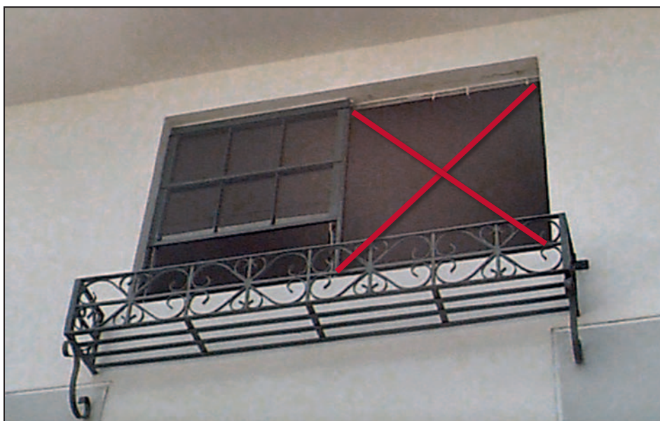
Figure 11-8. Window frame pulled out of the wall because of inadequate window frame attachment. Hurricane Georges (Puerto Rico, 1998)
