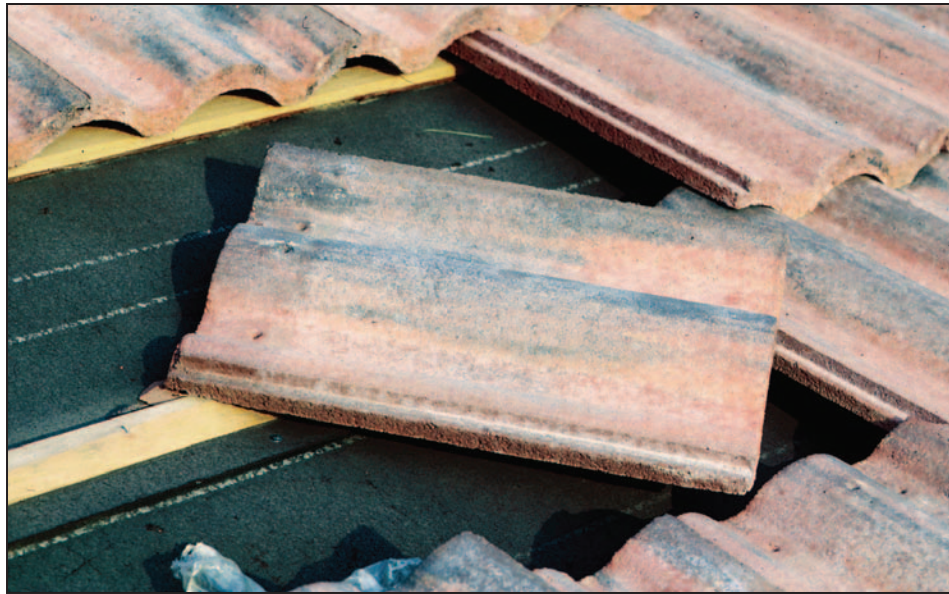
Figure 11-49. Area of the roof where tiles were not nailed to batten strips. Northridge Earthquake (California, 1994)
