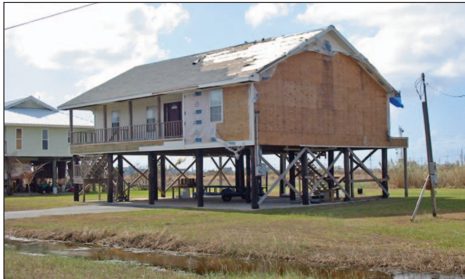
Figure 11-1. Good structural system performance but the loss of shingles, underlayment, siding, housewrap, and soffits resulted in significant interior water damage. Estimated wind speed: 125 mph. 3 Hurricane Katrina (Louisiana, 2005)
