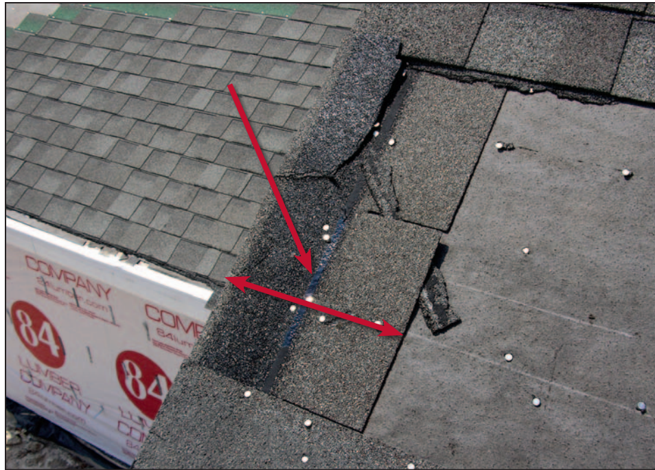
Figure 11-34. A bleeder strip (double-arrow) that was used at a rake blow-off; lack of contact between the tab of the overlying shingle and the bleeder's self-seal adhesive (upper arrow). Estimated wind speed: 125 mph. Hurricane Katrina (Mississippi, 2005)
