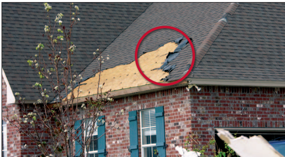
Figure 11-30. Loss of shingles and underlayment along the eave and loss of a few hip shingles. Estimated wind speed: 115 mph. Hurricane Katrina (Louisiana, 2005)
