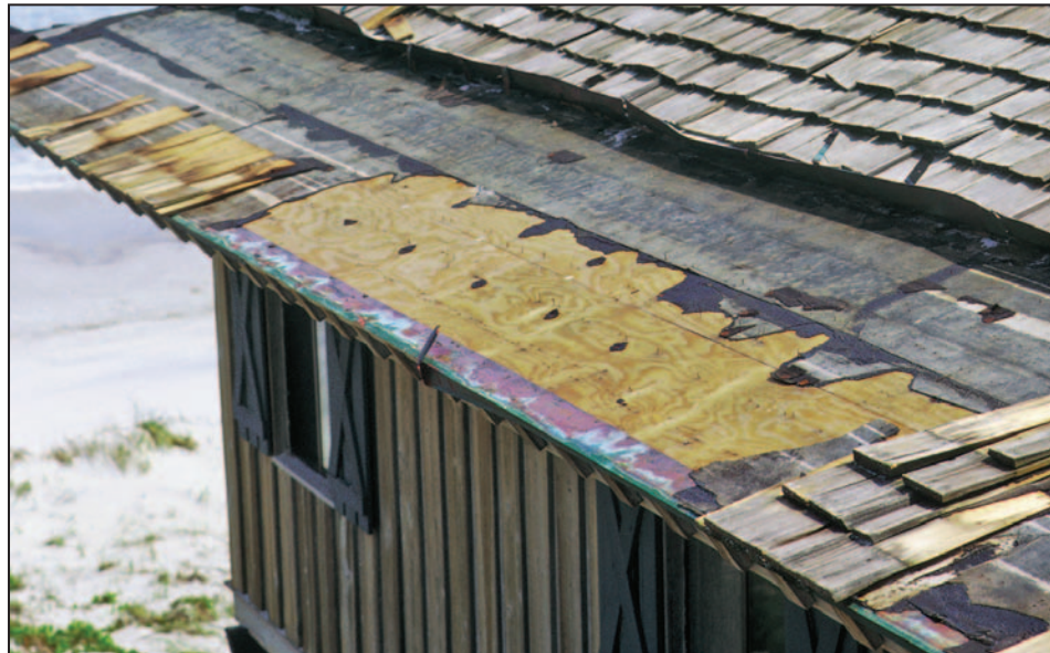
Figure 11-54. Loss of wood shingles due to fastener corrosion. Hurricane Bertha (North Carolina, 1996)
