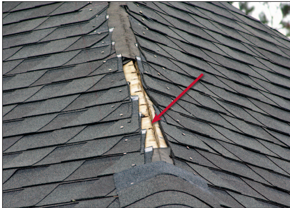
Figure 11-29. Underlayment that was not lapped over the hip; water entry possible at the sheathing joint (arrow). Estimated wind speed: 130 mph. Hurricane Katrina (Mississippi, 2005)
