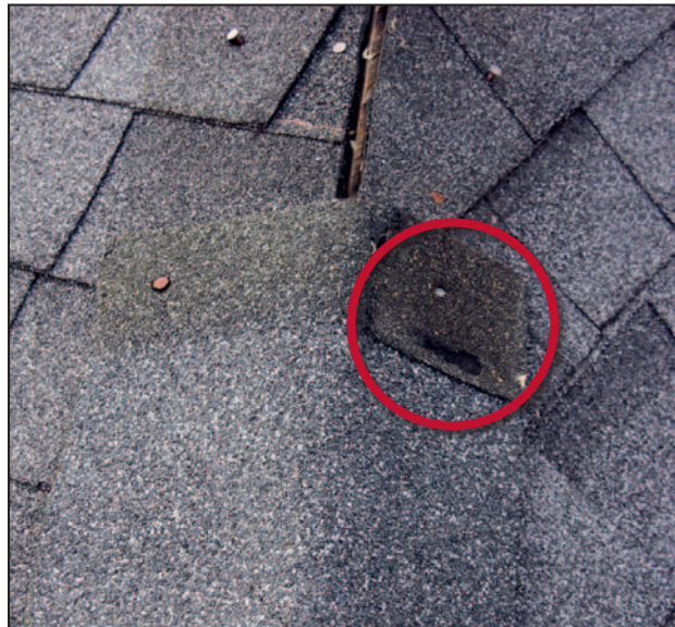
Figure 11-35. Inadequate sealing of the self-sealing adhesive at a hip as a result of the typical hip installation procedure. Estimated wind speed: 105 mph. Hurricane Katrina (Mississippi, 2005)
