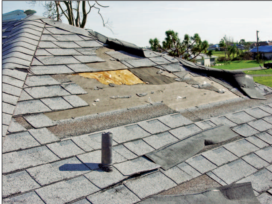
Figure 11-24. Small area of sheathing that was exposed after loss of a few shingles and some underlayment. Estimated wind speed: 140 to 160 mph. Hurricane Charley (Florida, 2004)
