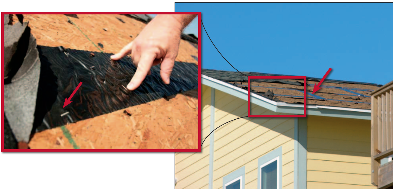
Figure 11-28. House that used enhanced underlayment Option 3 with taped sheathing joints (arrow). The self-adhering modified bitumen tape (inset) was stapled because of bonding problems. Estimated wind speed: 110 mph. Hurricane Ike (Texas, 2008)
