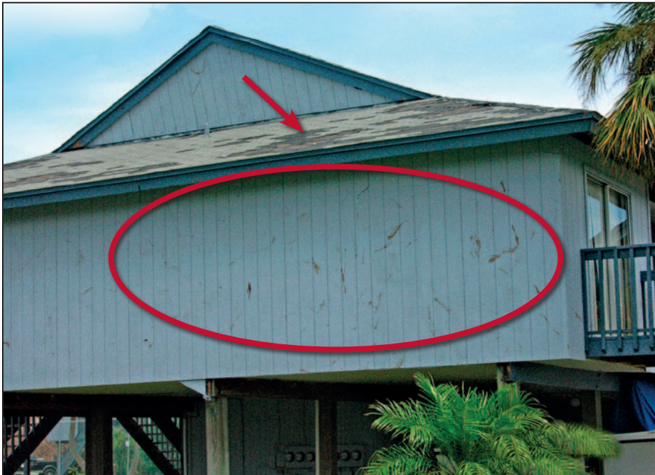
Figure 11-2. Numerous wind-borne debris scars on the wall of this house and several missing asphalt shingles. Estimated wind speed: 140 to 150 mph. Hurricane Charley (Florida, 2004)
