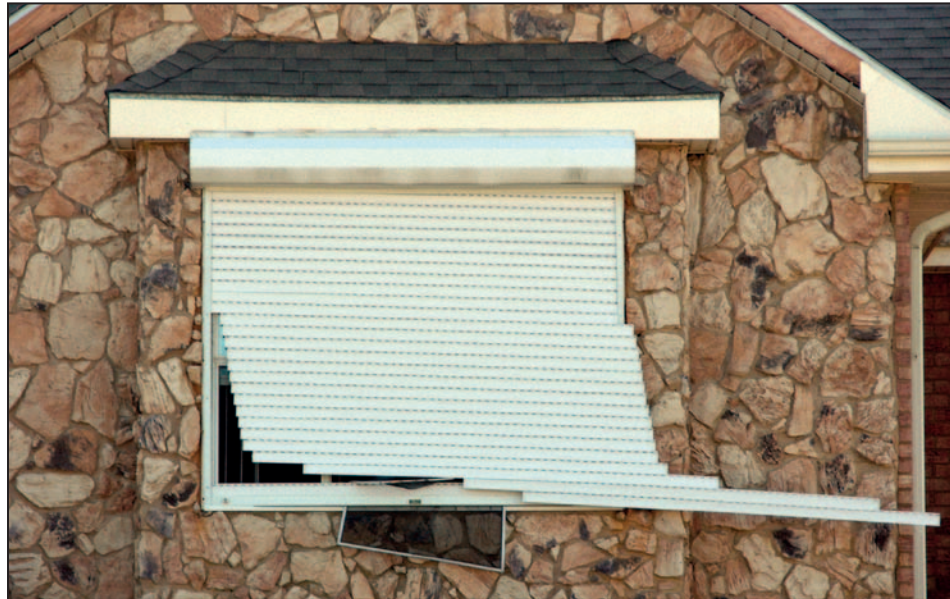
Figure 11-12. Roll-up shutter slats that detached from the tracks. The lack of a label makes it unclear whether the shutter was tested in accordance with a recognized method. Estimated wind speed: 110 mph. Hurricane Katrina (Louisiana, 2005)
