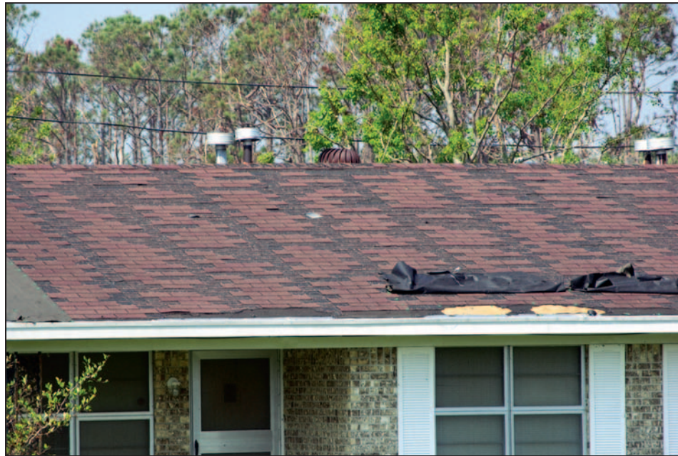
Figure 11-38. Shingles that unzipped at the band lines because the raking method was used to install them. Estimated wind speed: 135 mph. Hurricane Katrina (Mississippi, 2005)
