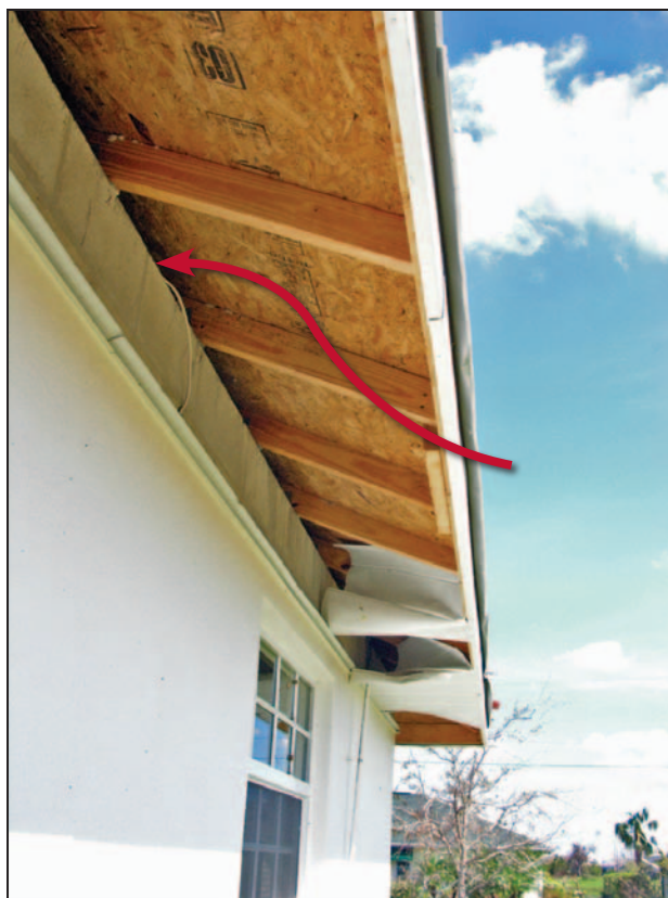
Figure 11-22. Blown-away soffit (arrow), which allowed wind-driven rain to enter the attic. Estimated wind speed: 140 to 160 mph. Hurricane Charley (Florida, 2004)
