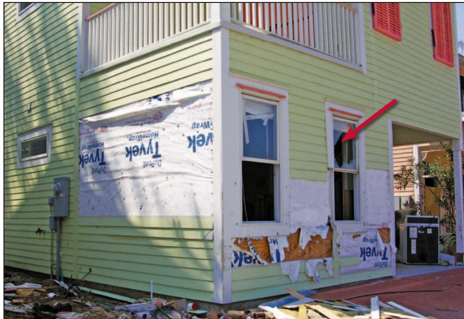
Figure 11-16. Blown-off fiber cement siding; broken window (arrow). Estimated wind speed: 125 mph. Hurricane Katrina (Mississippi, 2006)
