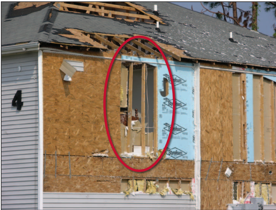
Figure 11-15. Blown-off vinyl siding and foam sheathing; some blow-off of interior gypsum board (circle). Estimated wind speed: 130 mph. Hurricane Katrina (Mississippi, 2006)
