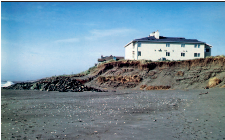
Figure 3-42. Buildings threatened by erosion at Ocean Shores, WA, in 1998. The rock revetments were built in response to shore erosion along an area adjacent to a jetty and thought to be accretional
