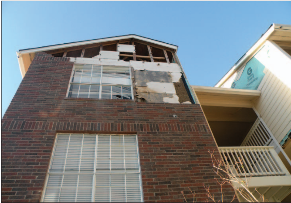
Figure 3-11. Apartment building with gable end wind damage from Hurricane Ike as a result of poor connection between brick veneer and wall structure (Galveston, TX, 2008)
