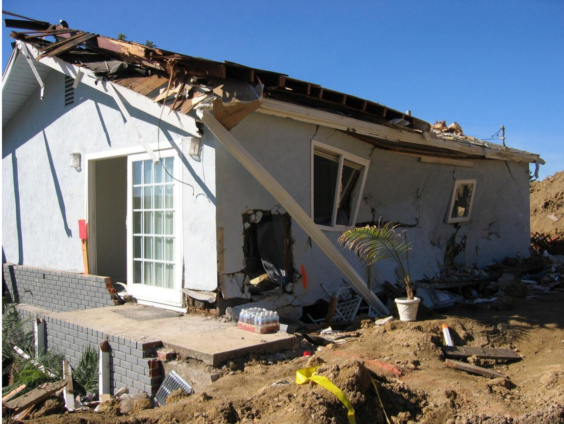
Figure 28. Damaged building braced for structural support in La Conchita, CA, after January 2005 storm event.
