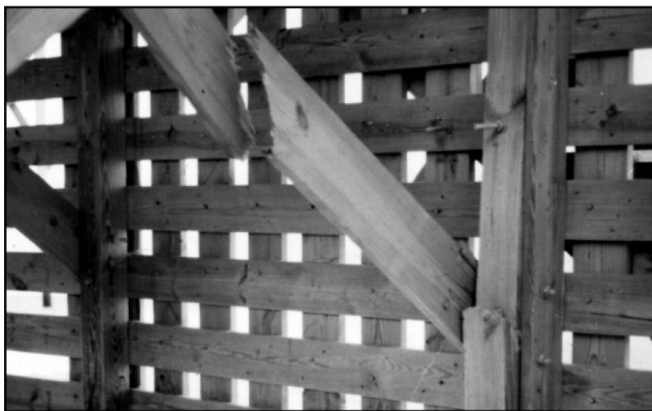
Figure 7. March 1989 nor'easter. Failure of cross-bracing.
