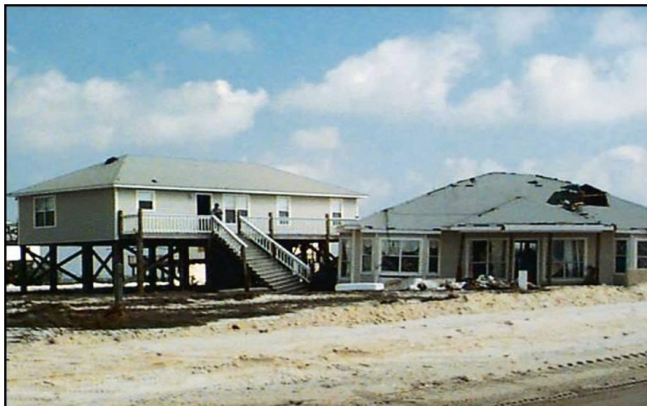
Figure 19. Hurricane Georges (1998), Dauphin Island, AL. As a result of erosion, scour, and inadequate pile embedment, the house on the right was washed off its foundation and into the house on the left.
