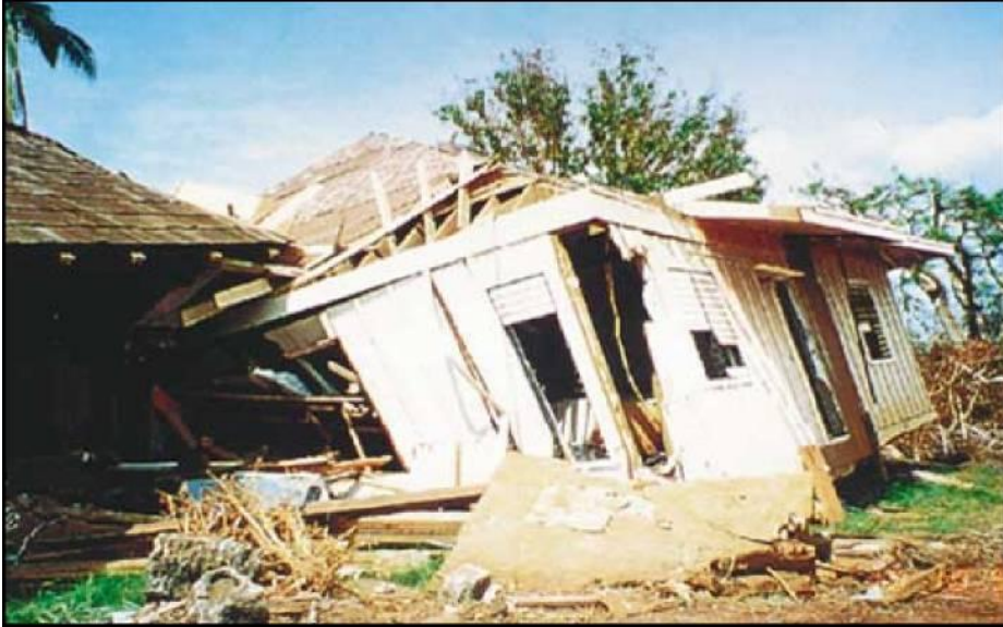
Figure 29. Hurricane Iniki (1992). Non-elevated house at Poipu Beach that floated off its foundation and was pinned against another house and destroyed by waves.
