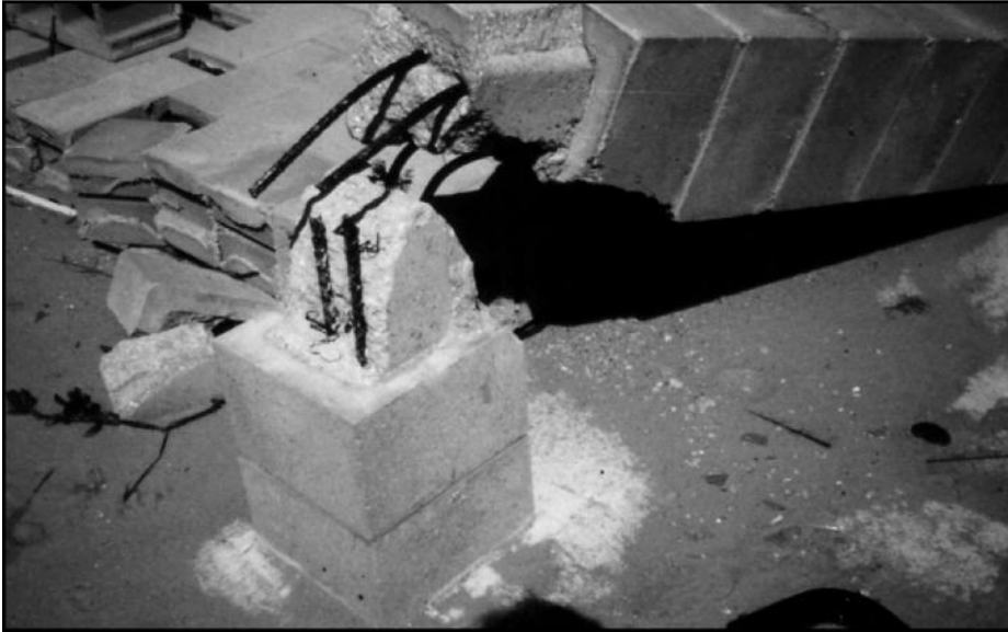
Figure 12. Hurricane Hugo (1989), South Carolina. Failure of reinforced masonry column.
