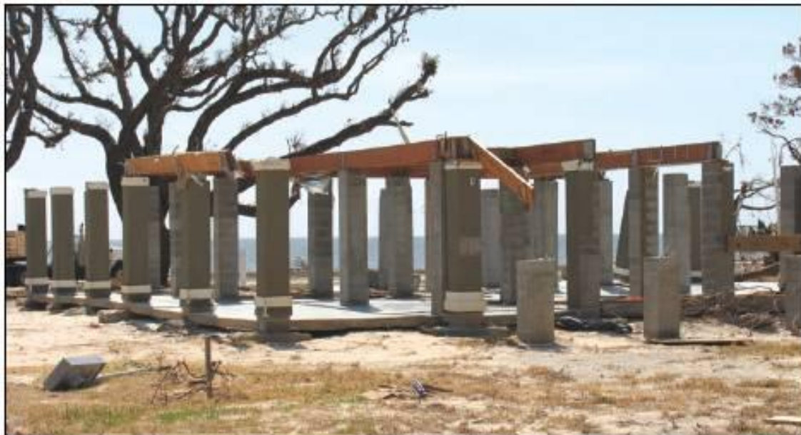
Figure 21. This elevated house on a masonry pier foundation was lost, probably due to waves and storm surge overtopping the foundation (Long Beach, MS, 2005).
