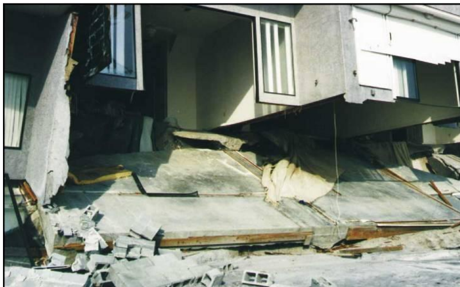
Figure 18. Hurricane Opal (1995), Bay County, Florida. Building damage from erosion and undermining.
