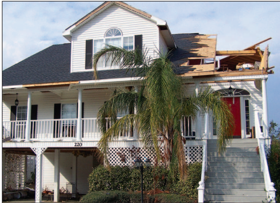
Figure 9-5. Newer home damaged from internal pressurization and inadequate connections, Hurricane Katrina (Pass Christian, MS, 2005)
