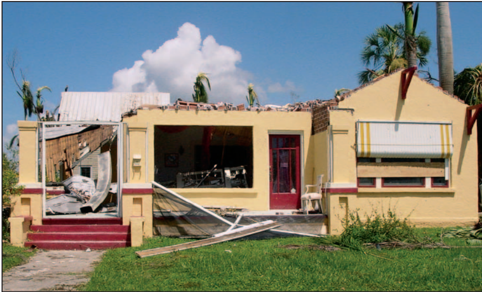
Figure 9-3. Roof framing damage and loss due to load path failure at top of wall/roof structure connection, Hurricane Charley (Punta Gorda, FL, 2004)
