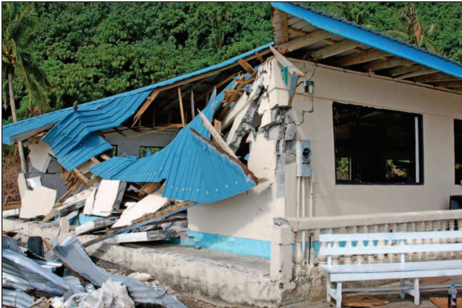
Figure 2-9. Tsunami damage at Poloa, American Samoa SOURCE: ASCE, USED WITH PERMISSION
