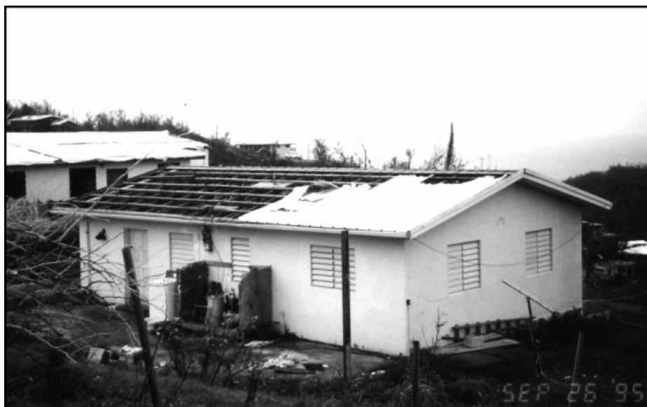
Figure 22. Hurricane Marilyn (1995). This house lost most of the metal roof covering.
