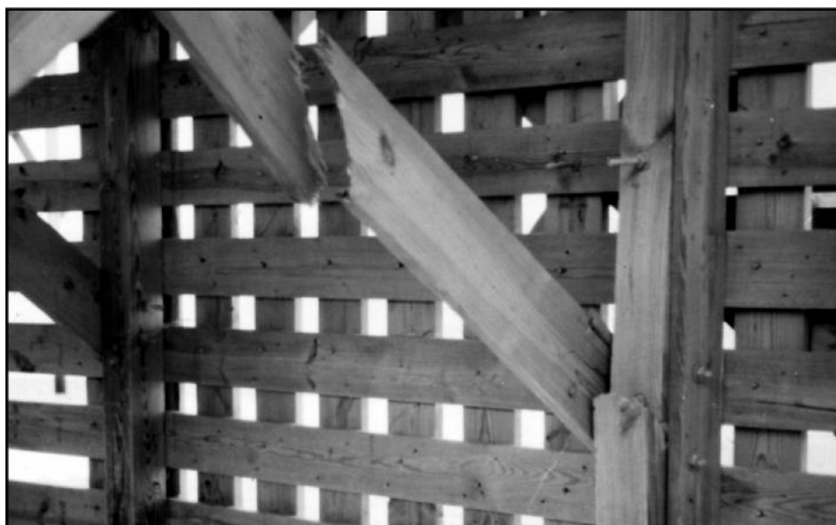
Figure 7. March 1989 nor'easter. Failure of cross-bracing.
