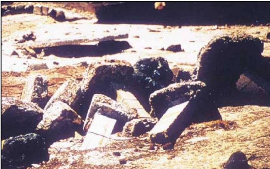
Figure 30. Hurricane Iniki (1992). Undermining of shallow footings supporting columns at Poipu Beach due to lack of sufficient embedment below erosion level.
