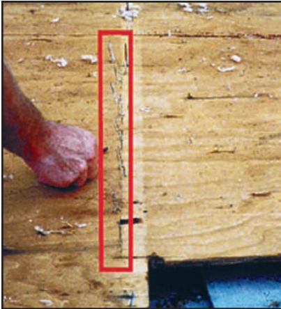
Figures 7-5 and 7-6. Exterior and interior views of connection issues between the roof sheathing and the top chords of the roof truss system. (Source: FEMA 55)
