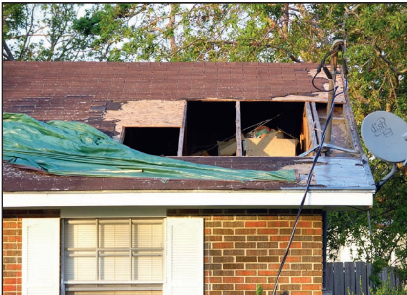
Figure 7-4. Loss of roof sheathing due to inadequate fastening between roof sheathing and framing. (Source: FEMA 549)
