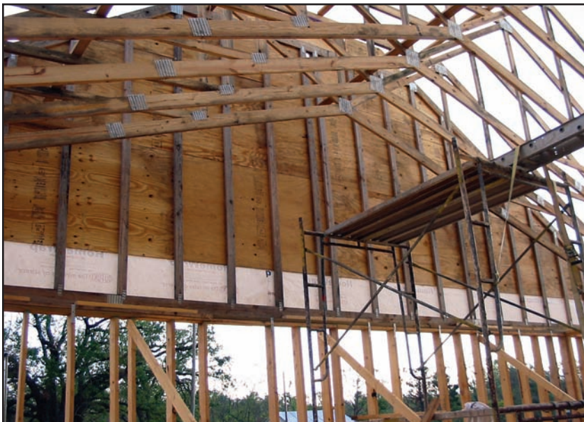
Figure 7-14. Improperly braced gable walls. The ceiling diaphragm (i.e., the bottom chords of the scissor truss) is located several feet above the top of the end wall top plate and no wall-to-truss bracing is provided. (Source: FEMA 549)
