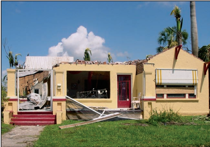
Figure 10-1. PUNTA GORDA, FLORIDA: Failure of a roof structure from pressurization of a house when the window failed on the windward face. (Source: FEMA 488)
