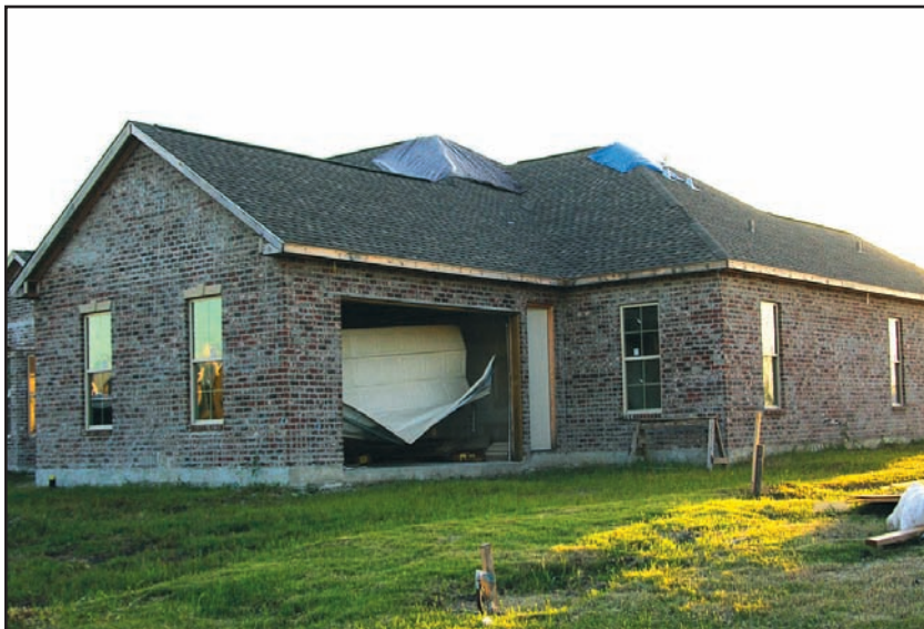
Figure 10-9. Positive pressure failure of garage door. (Source: FEMA 549)
