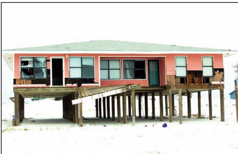
Figure 10-4. Glazing failure due to windborne debris. An oceanfront home damaged during Hurricane Ivan due to windows being broken by windborne debris. (Source: FEMA 489)
