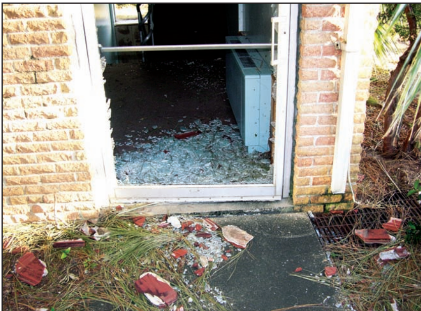
Figure 10-6. PENSACOLA, FLORIDA: Failure of glazing from windborne debris created by dislodged tile roofing. (Source: FEMA 489)
