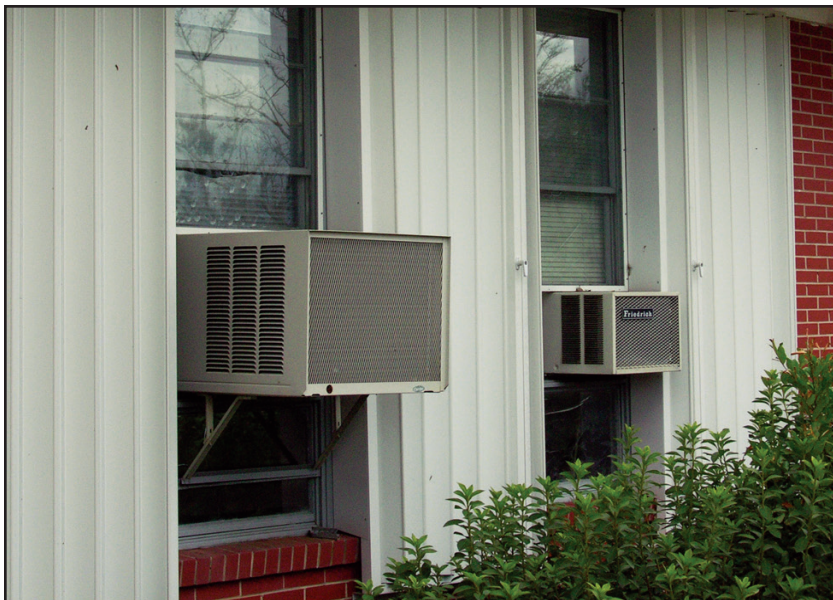
Figure 10-5. PENSACOLA, FLORIDA: Shutters had been attached to this building in order to protect it from windborne debris. However, areas above and below the air conditioning units were left unprotected. (Source: FEMA 489)
