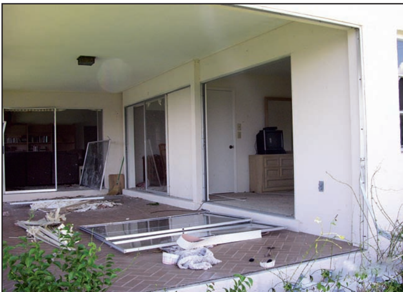
Figure 10-7. PUNTA GORDA ISLES, FLORIDA: Anchorage failure in sliding glass door failure. (Source: FEMA 488)
