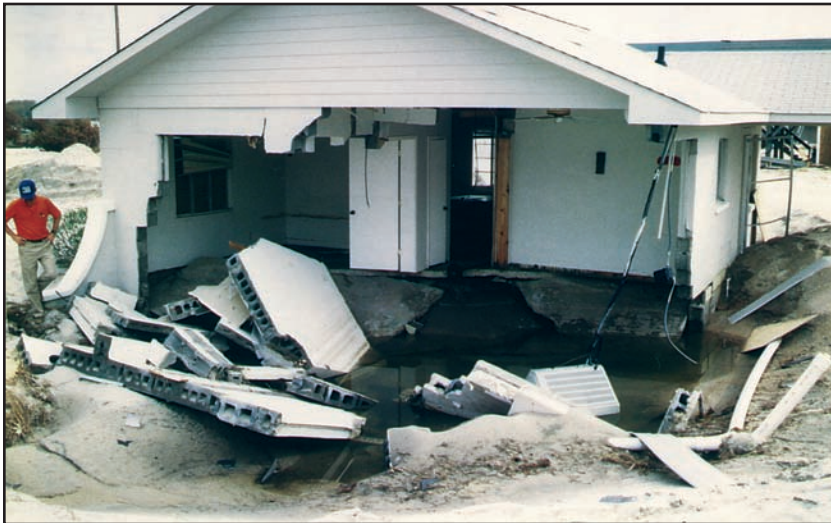
Figure 6-5. Building failure caused by undermining of crawlspace foundation during Hurricane Fran. Breaking waves may also have contributed to foundation failure. (Source: FEMA 290)
