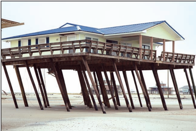
Figure 6-11. DAUPHIN ISLAND, ALABAMA: Structure near collapse due to insufficient pile embedment. (Source: FEMA 549)
