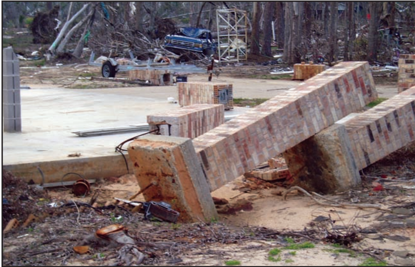
Figure 6-20. PASS CHRISTIAN, MISSISSIPPI: Performance comparison of shallow, open foundations founded on discrete footings (foreground) failed by rotating and overturning, while piers located on more substantial footings—in this case, a concrete mat (background)—survived. (Source: FEMA 549)
