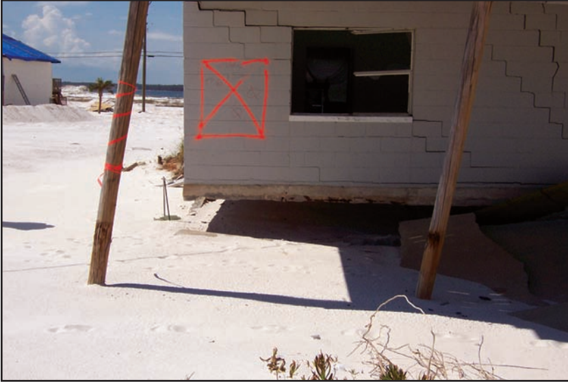
Figure 6-3. NAVARRE BEACH, FLORIDA: Close-up of foundation failure shown in Figure 6-2. (Source: FEMA 489)
