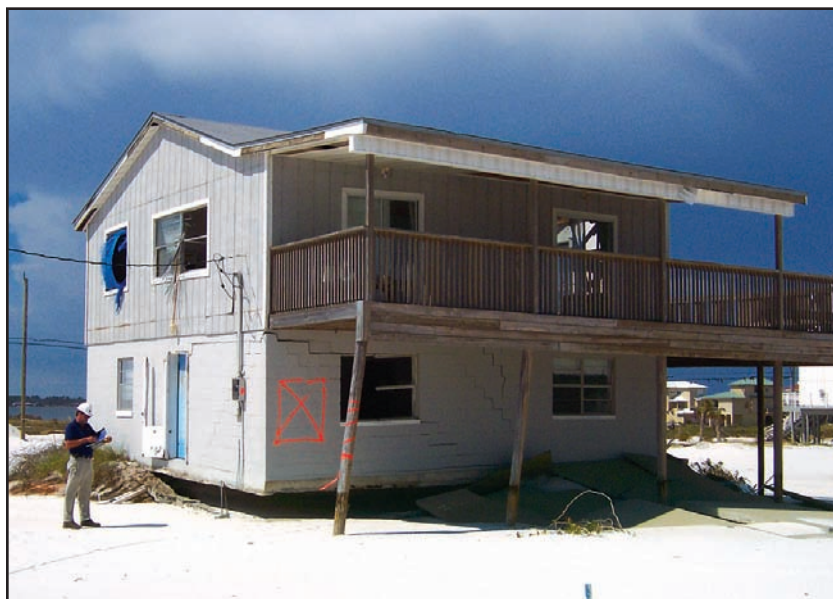
Figure 6-2. NAVARRE BEACH, FLORIDA: Slab-on-grade foundation failure due to erosion and scour undermining. (Source: FEMA 489)
