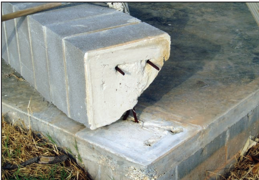
Figure 6-21. BELLE FONTAINE POINT, JACKSON COUNTY, MISSISSIPPI: Column connection failure. (Source: FEMA 549)
