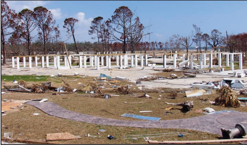
Figure 6-12. LONG BEACH, MISSISSIPPI: Structure removed from its foundation when waves exceeded the foundation height and connections between the elevated building and its foundation failed. The building was located within a mapped V Zone. (Source: FEMA 549)
