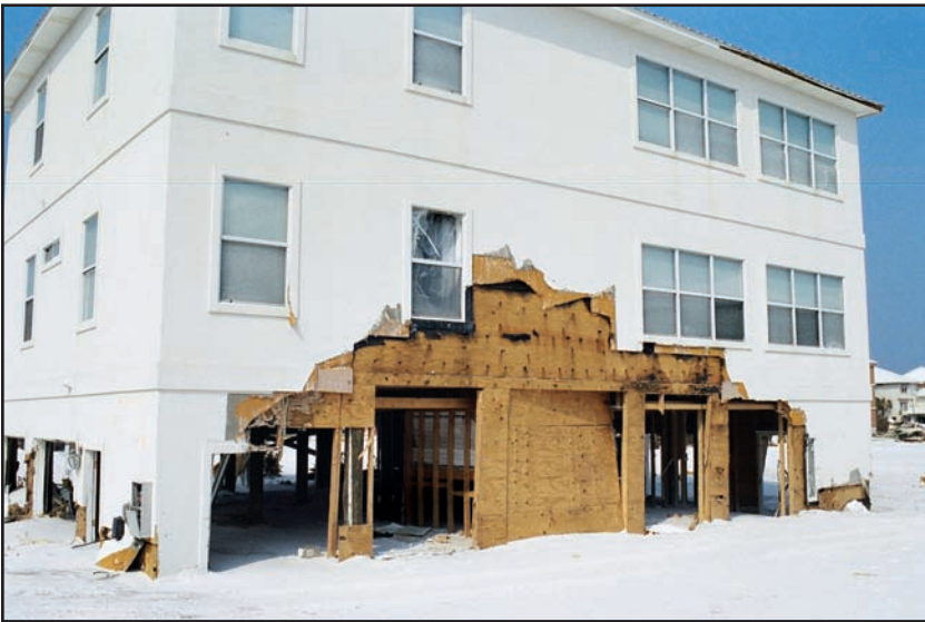
Figure 6-18. Building damages due to the incorrect construction of a breakaway wall. (Source: FEMA 489)
