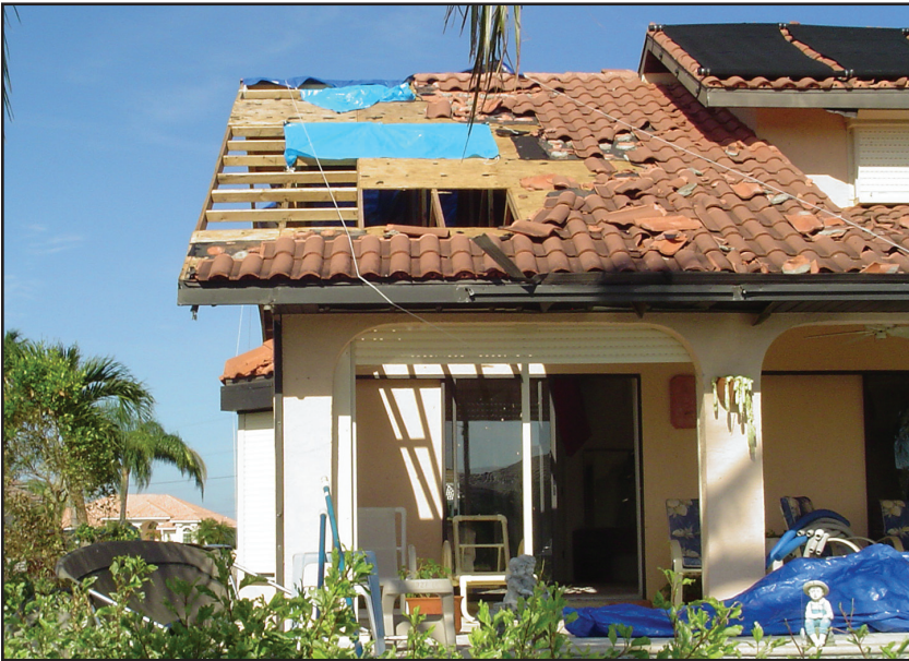
Figure 5-4. PUNTA GORDA, FLORIDA: Load path failure in connections between roof decking and roof framing. (Source: FEMA 488)
