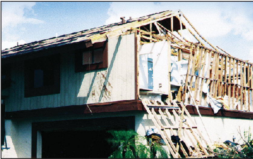
Figure 5-1. DADE COUNTY, FLORIDA, HURRICANE ANDREW (1992): Second-story wood framing (on first-story masonry). Load path failure at end gable. (Source: FEMA 55)
