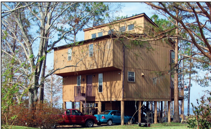
Figure 5-11. BIG LAGOON, FLORIDA: This house was elevated on piles, preventing major flood damage. (Source: FEMA 489)
