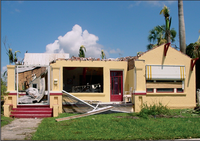
Figure 5-3. PUNTA GORDA, FLORIDA: Roof framing damage and loss due to load path failure at top of wall/roof structure connection. (Source: FEMA 488)
