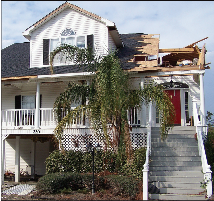
Figure 5-5. PASS CHRISTIAN, MISSISSIPPI: Newer home damaged from internal pressurization and inadequate connections. (Source: FEMA 549)
