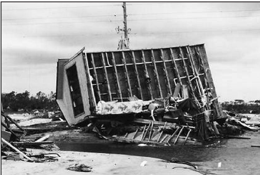
Figure 5-2. NORTH CAROLINA, HURRICANE FRAN (1996): Load path failure in connections between home and its foundation. (Source: FEMA 55)
