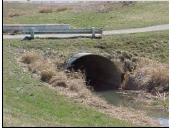
Undersized Culvert (Potential Area of Mitigation Interest)
