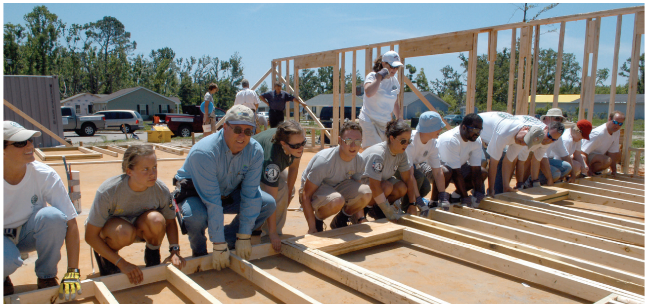
Gulfport, Miss., April 27, 2006 - AmeriCorps NCCC partnering with Harrison County Habitat for Humanity to build bunkhouses for volunteers assisting in recovery efforts on the Gulf Coast. George Armstrong/FEMA
