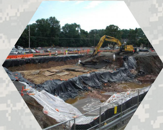
FUSRAP, Maywood, NJ
