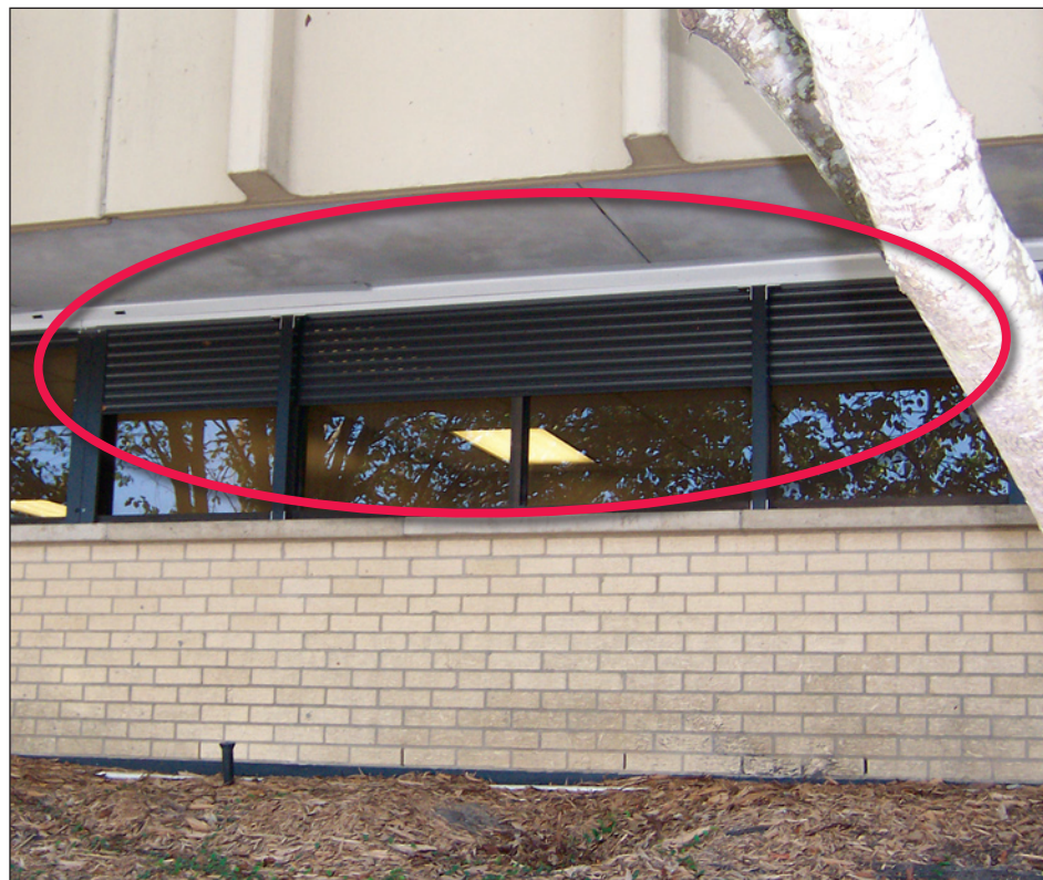
Figure 9-12. Closeup of the roll-down metal shutters on the Harrison County Courthouse building. Note the partially lowered shutters on the middle windows (circle) (estimated wind speed: 130 mph. Gulfport, Mississippi).
