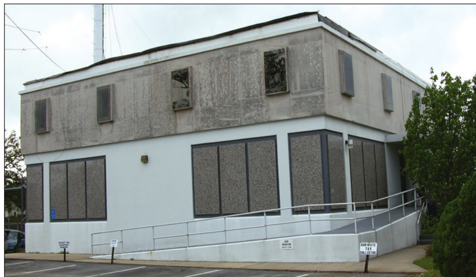
Figure 9-15. Exterior view of the Jackson County EOC. Note the polycarbonate shutters over the windows (estimated wind speed: 105 mph. Pascagoula, Mississippi).
