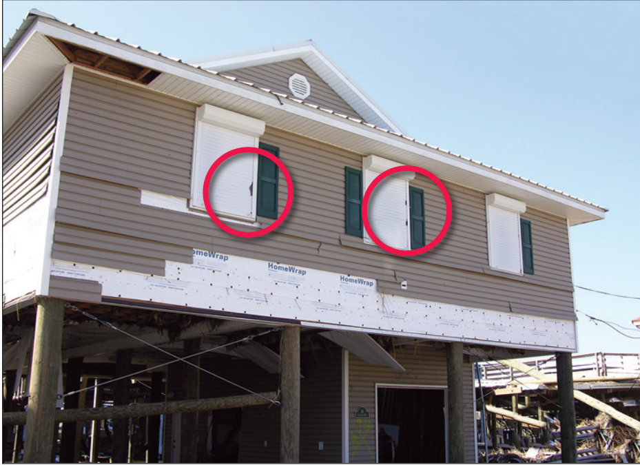
Figure 9-19. The black area at the left window and the two black areas at the middle window (circles) are pieces of asphalt shingle debris. Had the windows not been protected by shutters, they would have likely been broken by windborne debris (estimated wind speed: 125 mph. Shell Beach, Louisiana).
