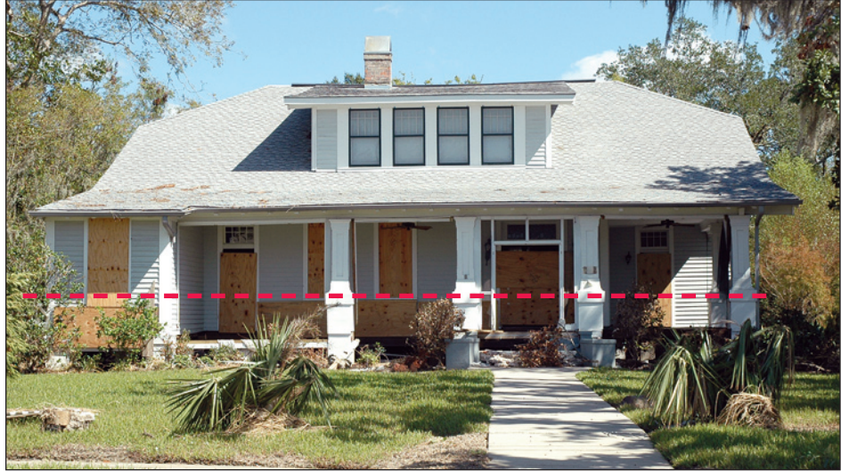
Figure 9-7. This building, elevated only a few feet above ground level, was heavily damaged by storm surge and flooding during Hurricane Katrina. Note the estimated flood depth in relation to the first floor (red line) (Mandeville, Louisiana).
