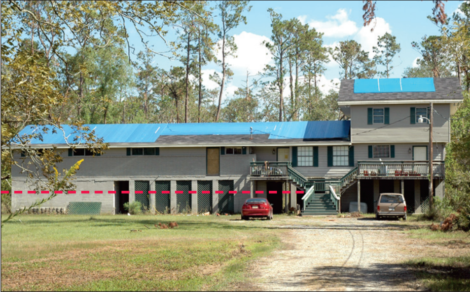
Figure 9-5. Post-Katrina photo of an HMGP-elevated house. Note the estimated water line associated with Hurricane Katrina (red line) (Lacombe, Louisiana).
