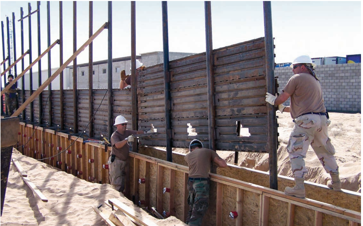
Air National Guard airmen of the 188th Fighter Wing, Arkansas Air National Guard, install a fence along the U.S.-Mexico border east of San Luis, Arizona. The Guardsmen were working in partnership with the U.S. Border Patrol as part of Operation Jump Start, October 3, 2006. (Photographer: SSgt Dan Heaton, USAF Air Force Photo.)
