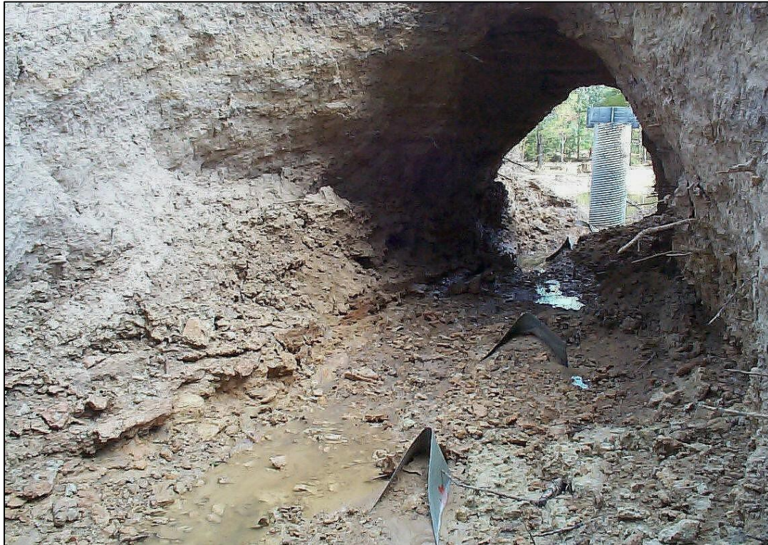
Figure 10-8.—Failure of an earth embankment in Louisiana along the principal spillway conduit, looking upstream toward riser. Notice damaged anti-seep collars on conduit. (Photo courtesy of NRCS, Louisiana)
