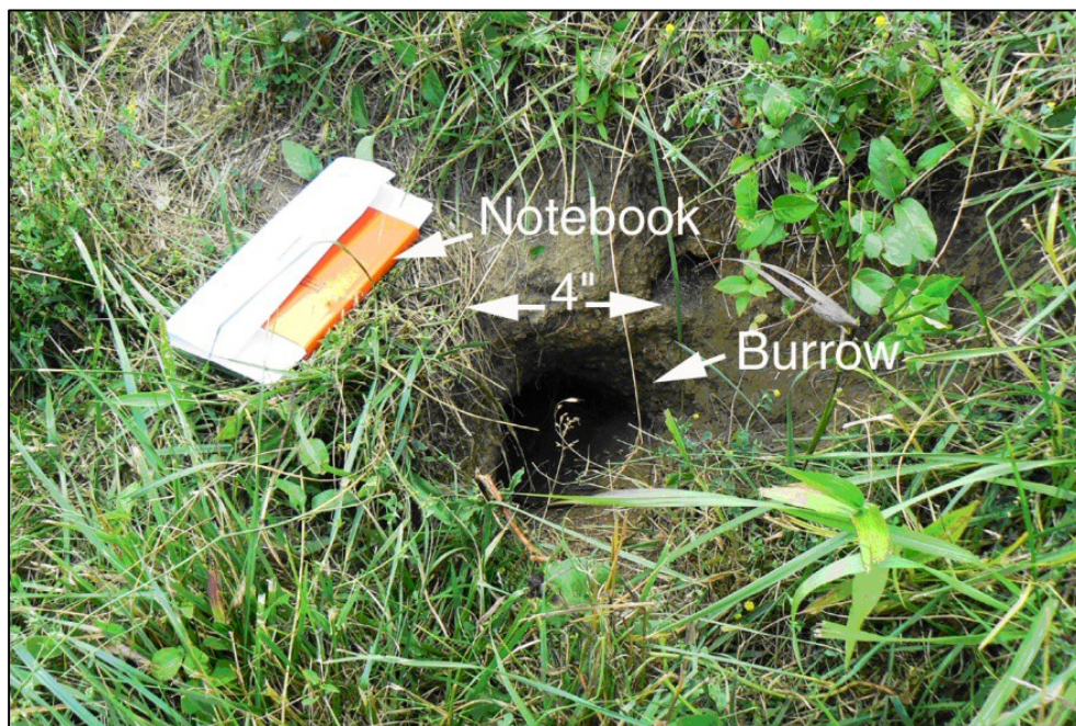
Figure 6-7.—Surface deformation indicative of animal activity observed on the downstream slope.
