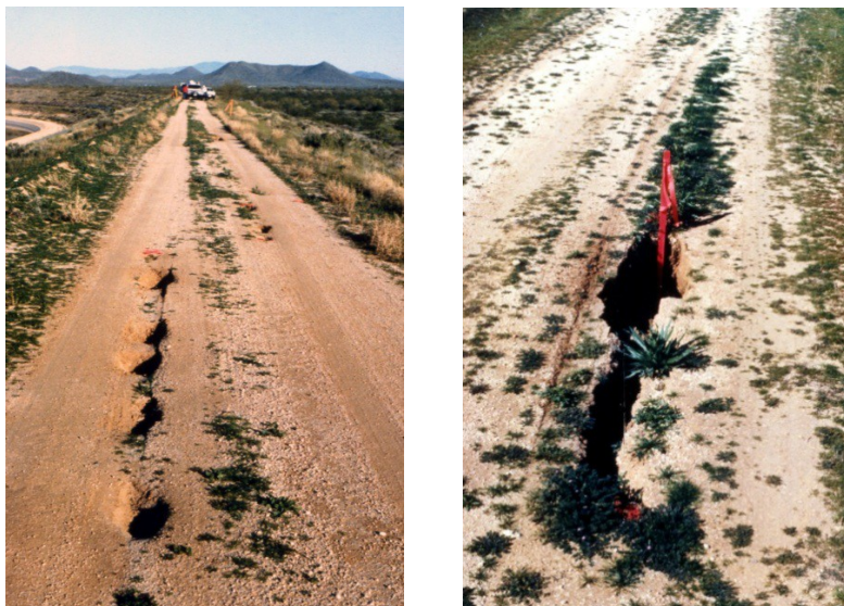
Figure 2.—Typical longitudinal cracking observed on crest of Reach 11 Dikes.
