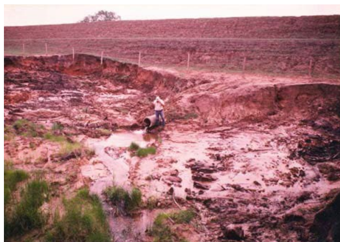
Figure 3.—Sloughing of downstream area near plunge pool.
