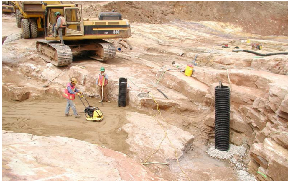
Figure 8.—Foundation cleanup and construction of downstream filter and berm at Spring Canyon Dam.
