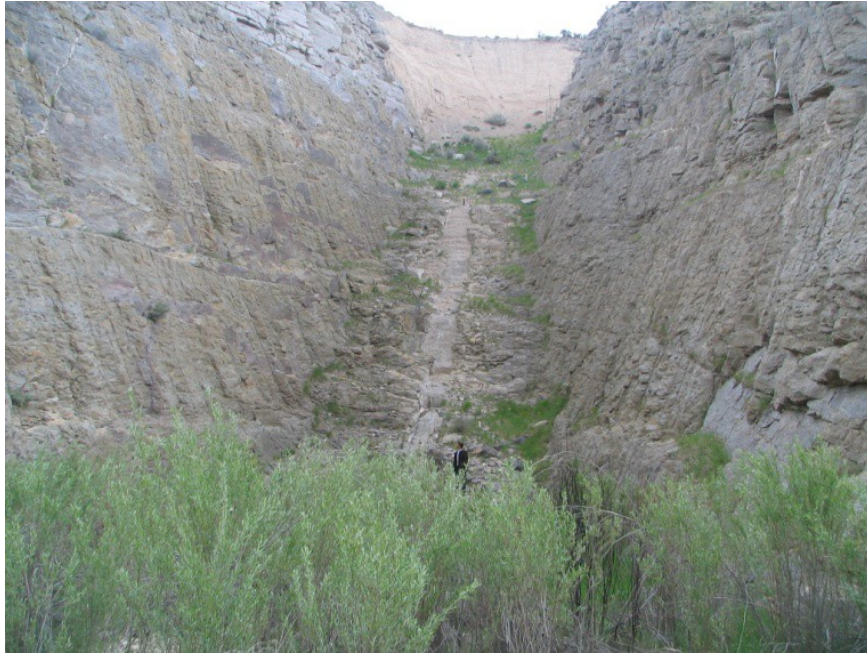
Figure 4.—Narrow, 70-ft-deep abutment cutoff trench. Man shown for scale (photo courtesy of James Wright 2007).
