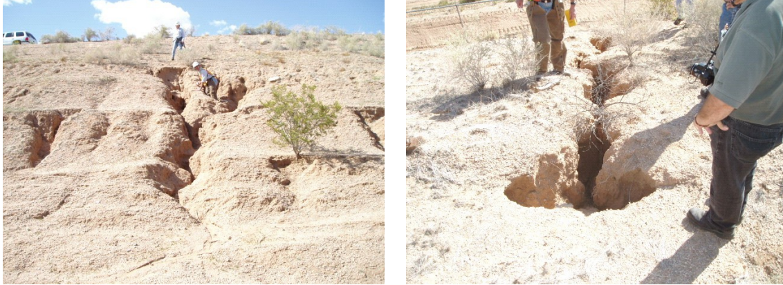
Figure 3.—Typical severe erosion of dispersive embankment soils comprising Reach 11 Dikes.
