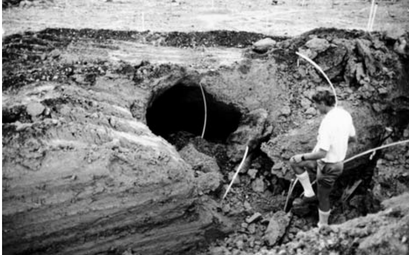
Figure 4.—Internal erosion in the dam core (Amos and Gillon, 2007).
