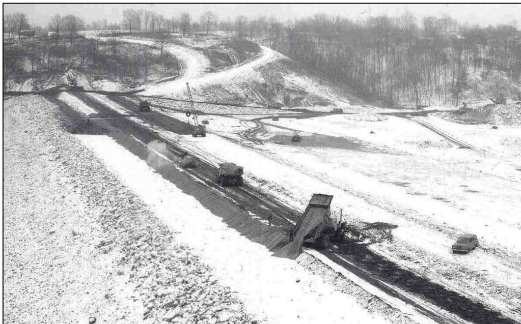
Figure 3-4.—Examples of winter construction at embankment dams prior to removal of snow and ice contamination. (Top) Blue blanket is insulated to prevent freezing of underlying soils. (Bottom) Placement of fill on improperly prepared frozen ground, snow, and ice.
