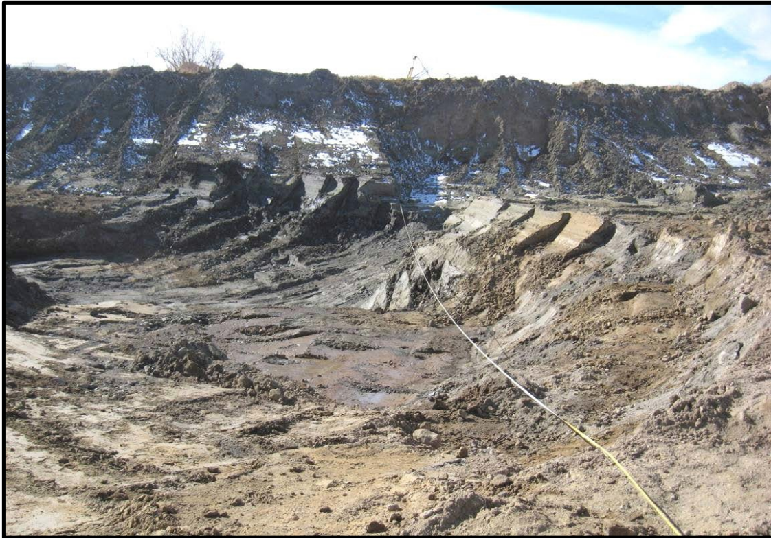
Figure 8.—View to the southwest (toward the right side canal embankment) of the final excavation of the scour hole site.
