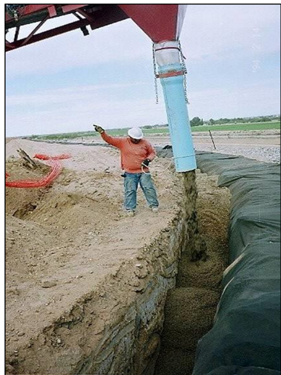
Figure 10-19.—Construction of a geotextile/aggregate chimney filter in Florence Dam in Arizona. Geotextile drape is on right (downstream) side of trench. (Photo courtesy of NRCS, Arizona)
