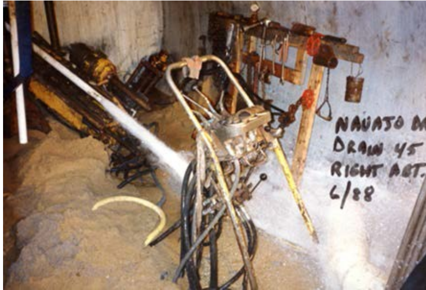
Figure 8.—High flows and sand washing into drain hole No. 45.
