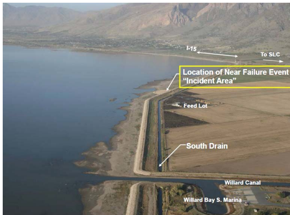
Figure 4.—Aerial view of the western portion of the dam showing the incident location in relation to the South Drain and feedlot.
