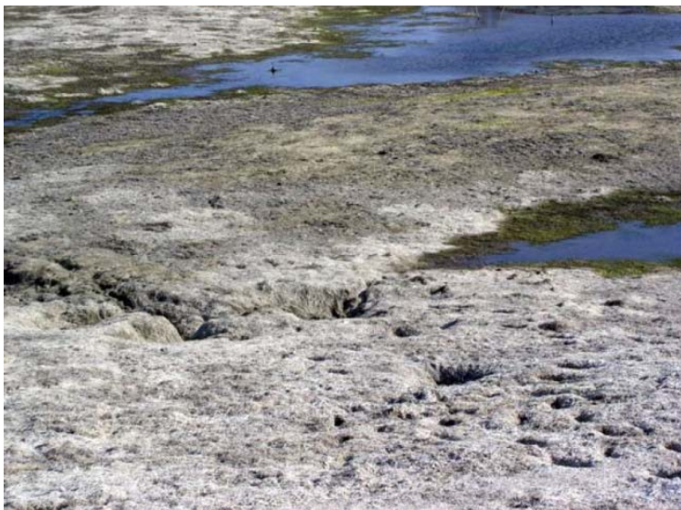
Figure 9.—Sinkholes in reservoir bottom.
