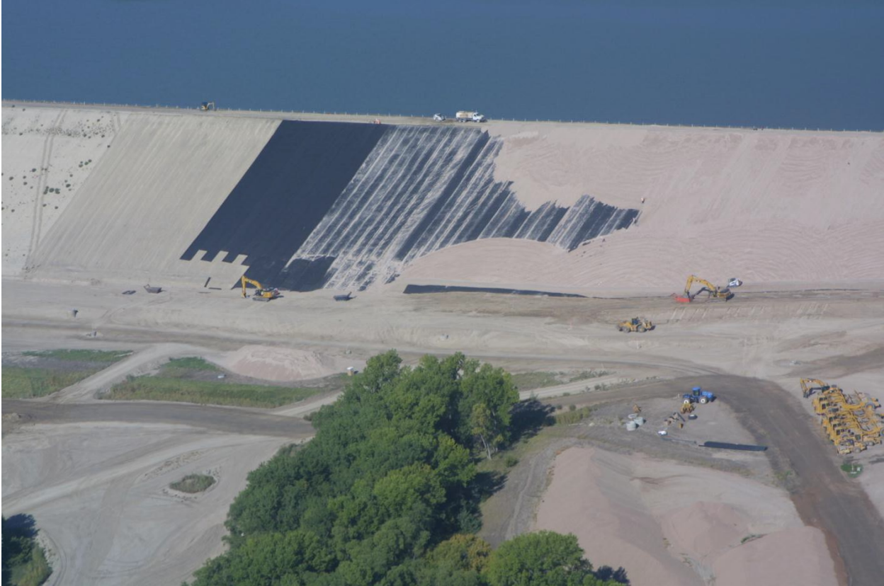
Figure 11.—Aerial photo of Red Willow Dam showing geo-net installation and protection with sand.
