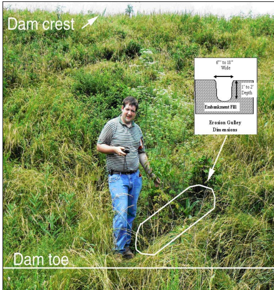
Figure 6-8.—Surface erosion (gully).
