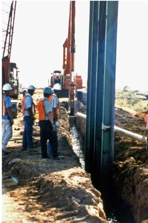
Figure 7.—Excavation of trench using biopolymer slurry. Steel frame was used to install the geomembrane panels.
