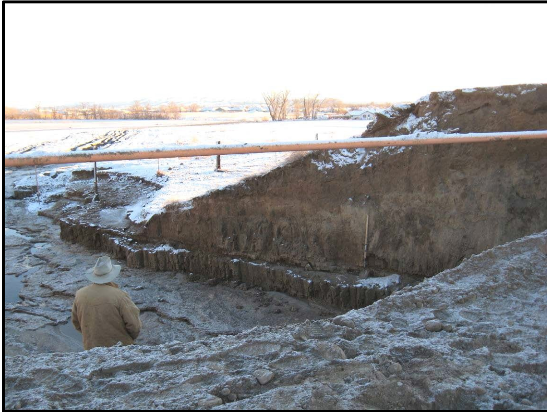
Figure 3.—View through the breach toward Fernley, Nevada. The downstream breach face cut into the left canal embankment is 17½ ft high.
