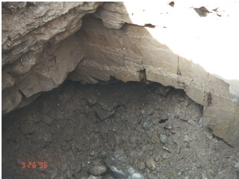
Figure 4.—Looking into sinkhole from foundation contact.
