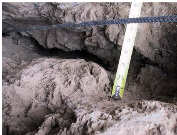
Figure 3.—Up to 5-in-wide cracks under holes.
