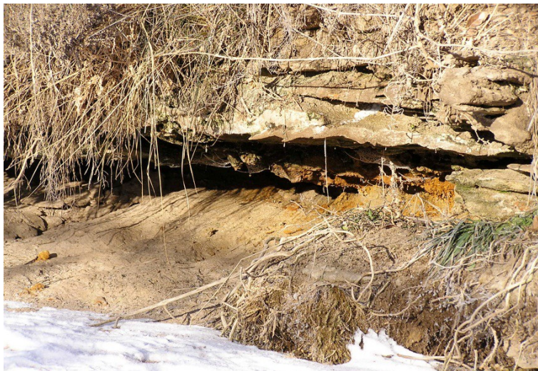
Figure 6.—Hardpan that formed a roof for the developing pipe.
