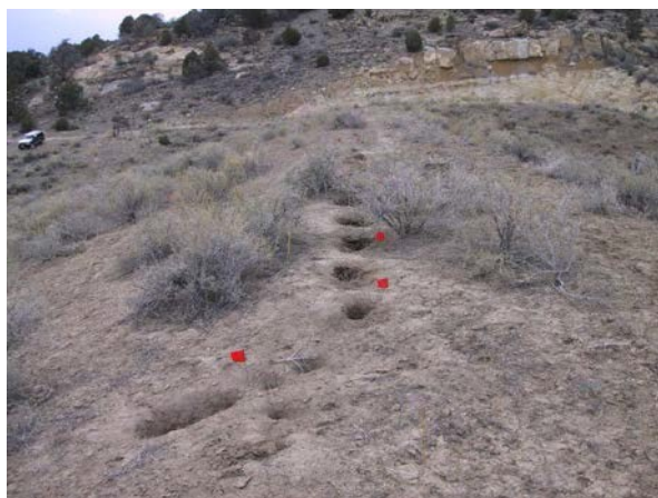
Figure 2.—Holes observed in crest.
