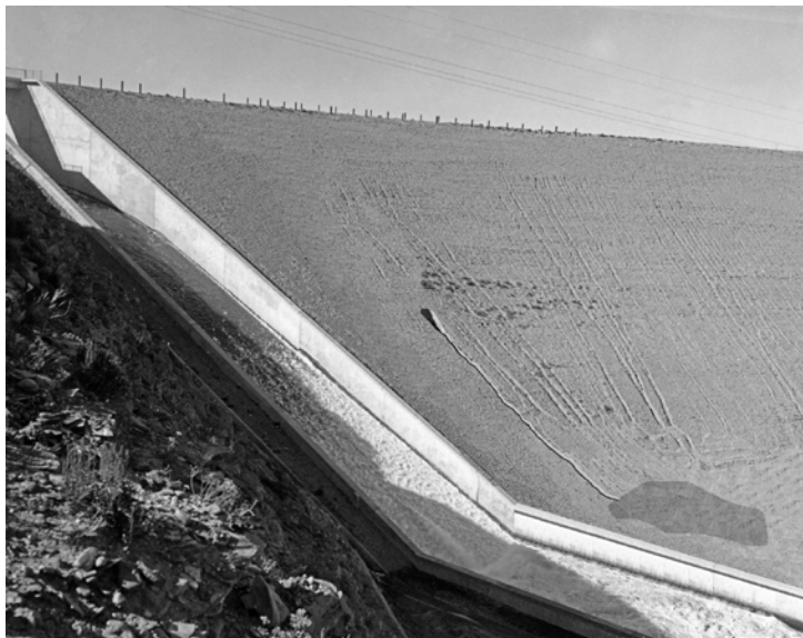
Figure 3.—First appearance of sinkhole, with drainage.
