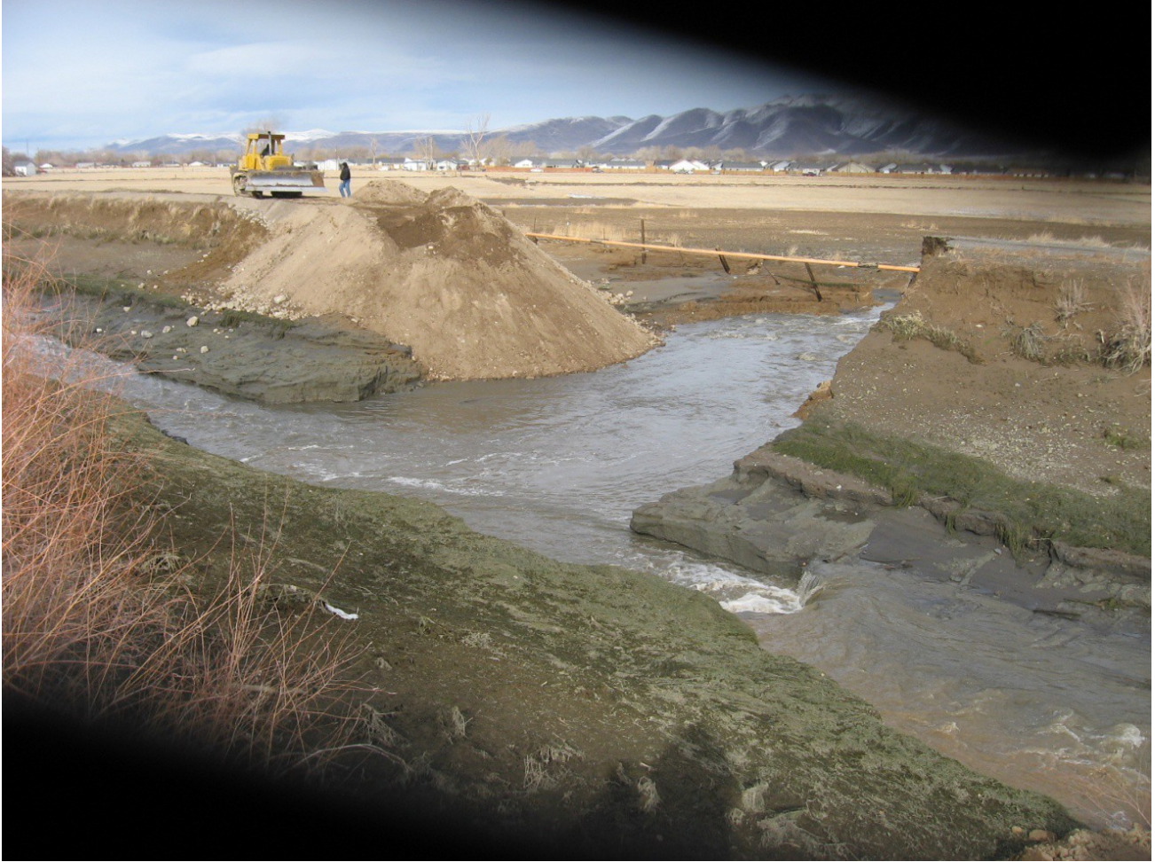
Figure 1.—Photo of the breach during early phases of temporary breach repair on the morning of January 5, 2008. Normal canal flow is from left to right in this photo. The breach is being filled by pushing fine-grained soil into the gap in the canal embankment. Some of the scour of the canal bottom can be seen along with some scour of the area immediately downstream from the breach. The pipeline shown is an abandoned natural gas pipeline that had been buried in the canal embankment. The pipe remained in place after the breach despite eroding all support provided by the original embankment.
