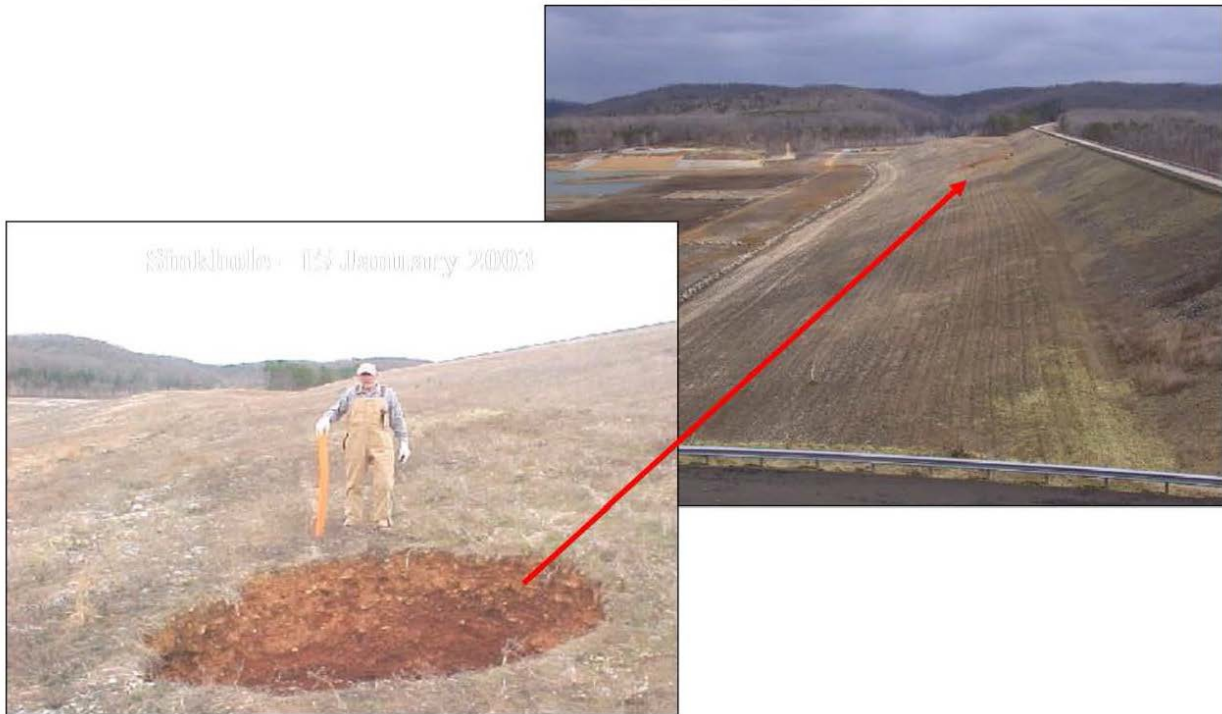
Figure 5.—Sinkhole through upstream impervious blanket.
