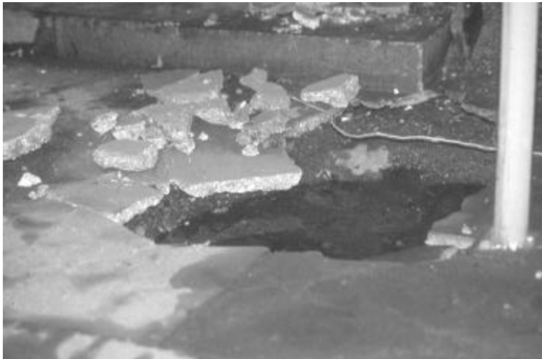
Figure 1-19. This basement floor broke from hydrostatic pressure
