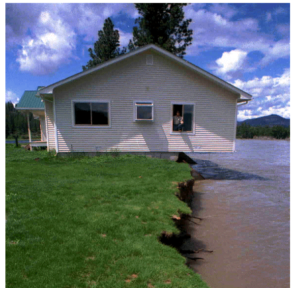
Figure 1-5. Riverine erosion can undercut structures
