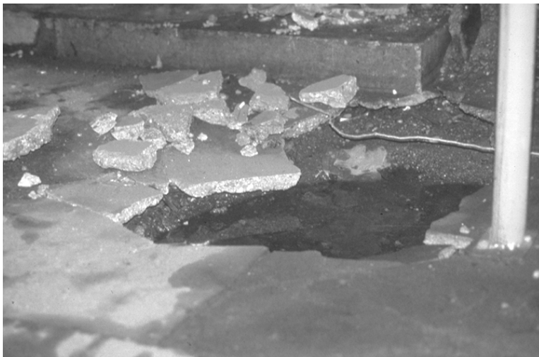
Figure 1-19. This basement floor broke from hydrostatic pressure
