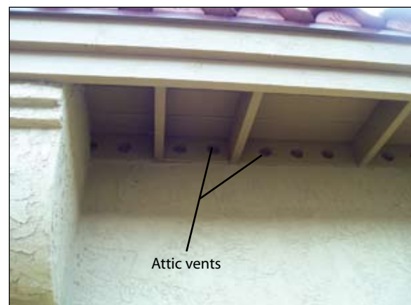
Figure 1. An open overhang. The exposed timber rafters and decking are susceptible to ignition, and embers and hot gases can enter the attic through unprotected vents.
