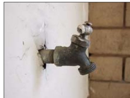
Figure 1. The gap around utility penetrations such as this one should be filled.
