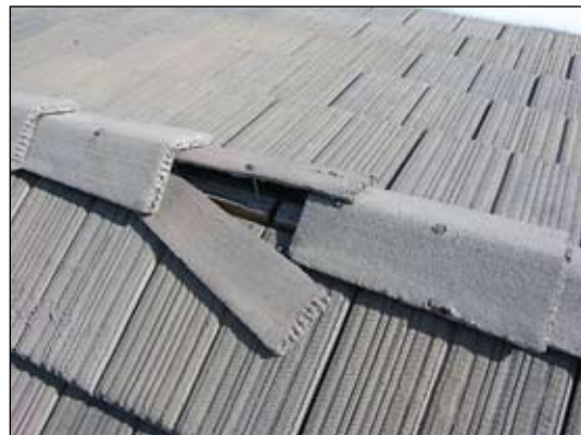
Figure 3. Displaced tiles allow ember entry.
