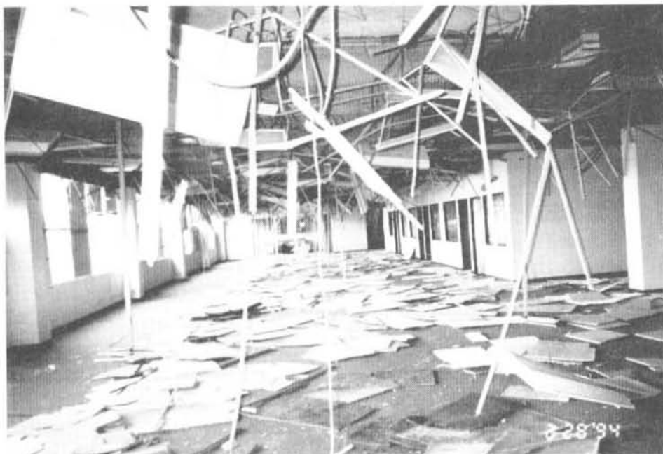
Complete loss of suspended ceiling and light fixtures Earthquake Damage: 1994, Northridge, California Photo Credit: Wiss, Janney, Elstner Associates, Inc.
