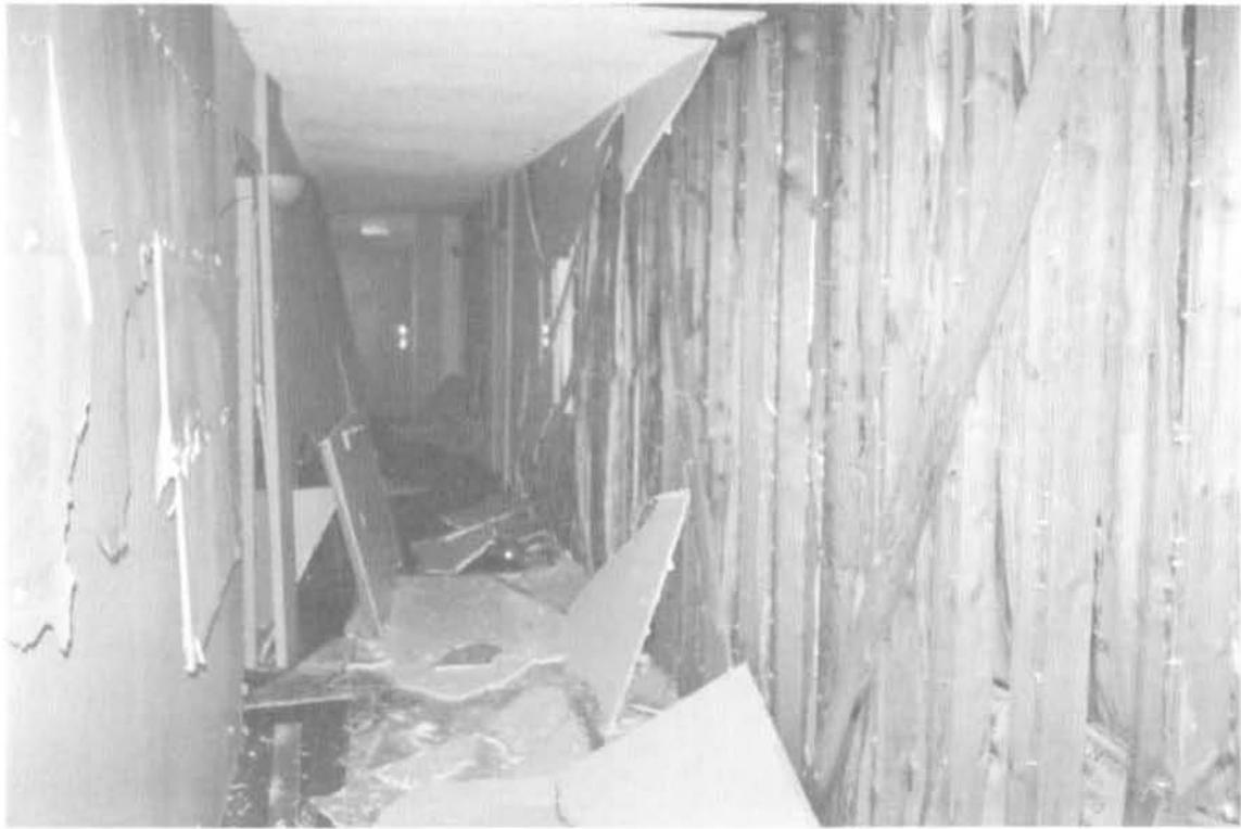
Earthquake Damage: 1994, Northridge, California Photo Credit: Wiss, Janney, Elstner Associates, Inc.
