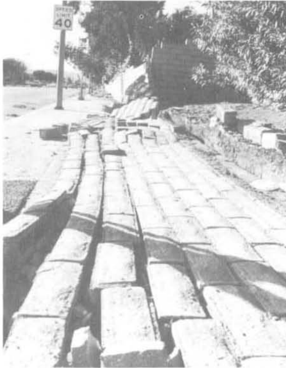
Earthquake Damage: 1994, Northridge, California Photo Credit: Robert Reitherman
