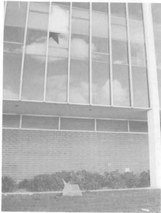
Earthquake Damage: 1994, Northridge, California Photo Credit: Wiss, Janney, Elstner Associates, Inc.
