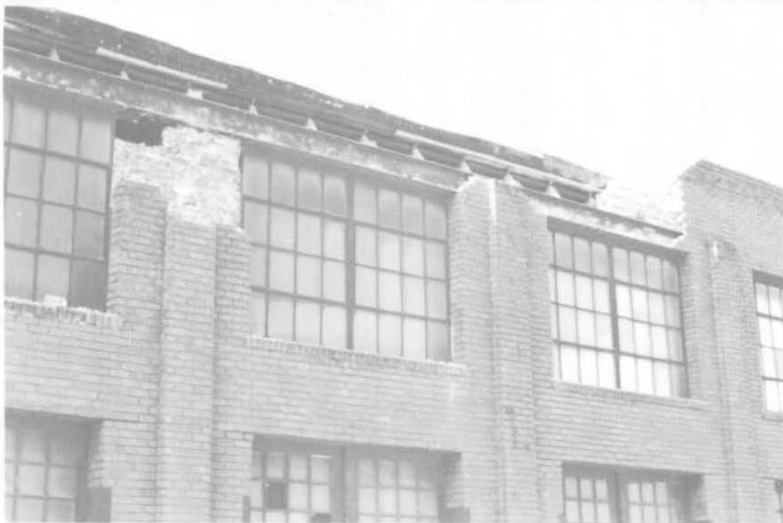
Earthquake Damage: 1989, Loma Prieta, California Photo Credit: Wiss, Janney, Elstner Associates, Inc.
