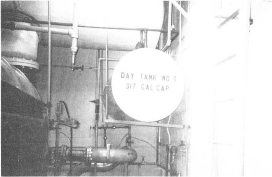
Unbraced Day Tank, Hospital, Puerto Rico Photo Credit: Wiss, Janney, Elstner Associates, Inc.
