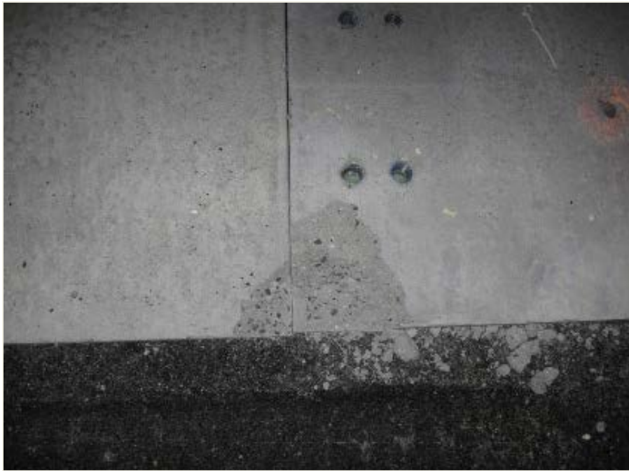
Figure 58. Spalling at joints on the ramp. Note panels were in contact.
