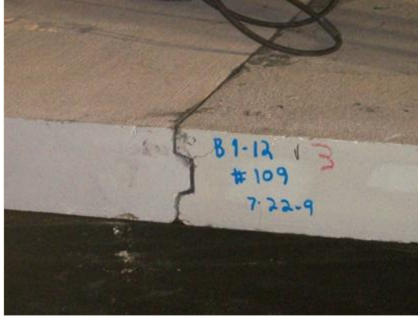
Figure 51. Crack in slab #109 at keyway. Note top of keyway rests on lower slab.
