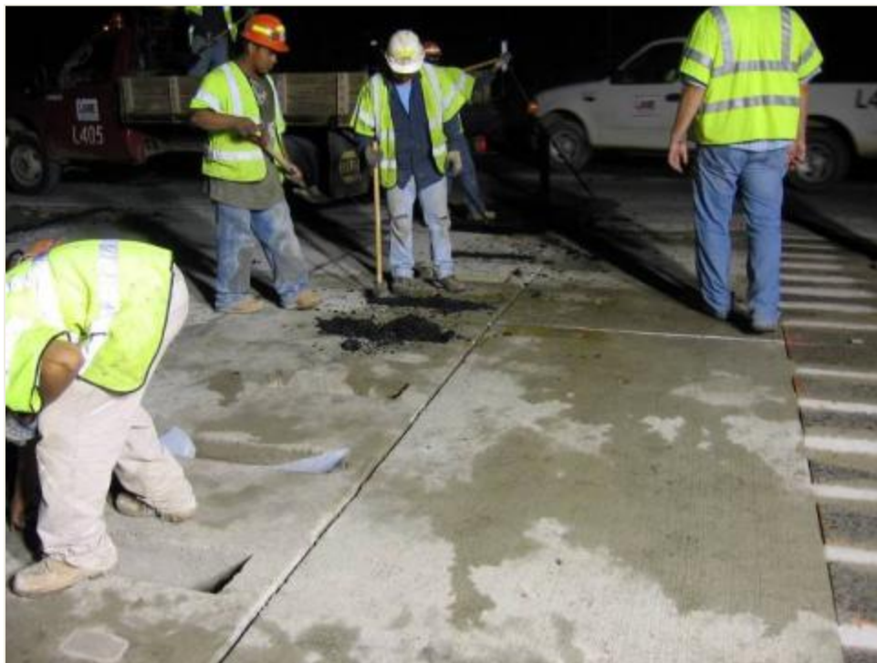
Figure 46. Cold patch in blockouts.
