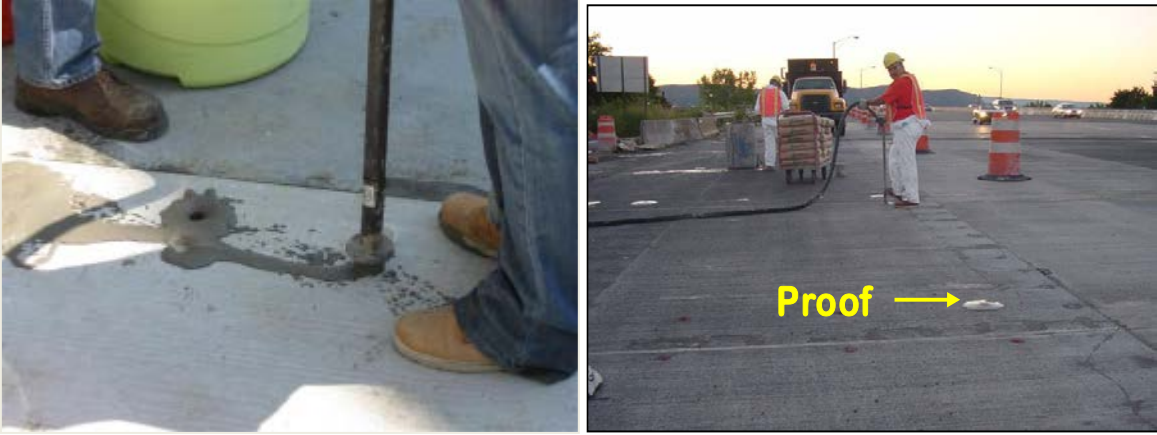
Figure 23. Verification of dowel grout and bedding grout distribution for uniform support (image from project in New York State, 2002).
