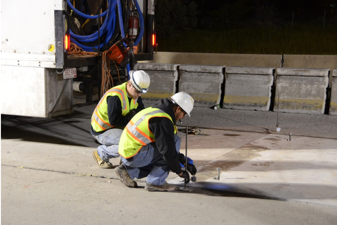
Figure 26. Panels leveled using leveling bolts to within final grade tolerance of 0.25 in.
