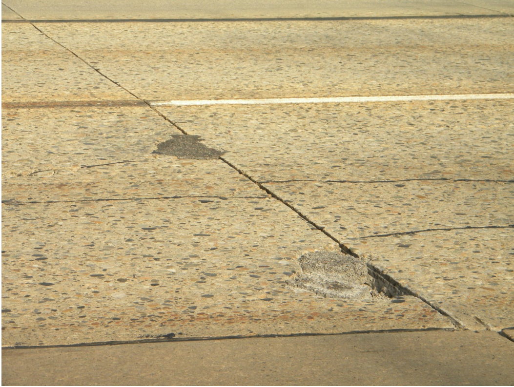
Figure 5. High-severity spalling and polishing of PCC surface on I-215.
