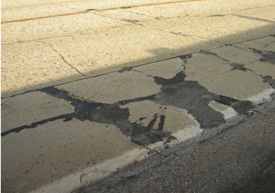
Figure 7. Severely deteriorated cracks and spalls filled with HMA on I-215.
