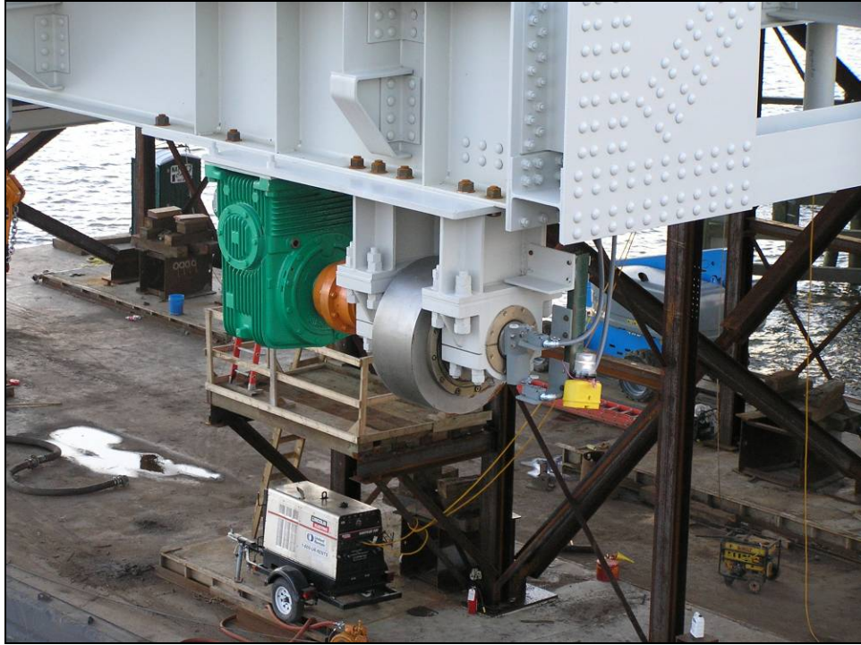
Figure 10. New swing span machinery.
