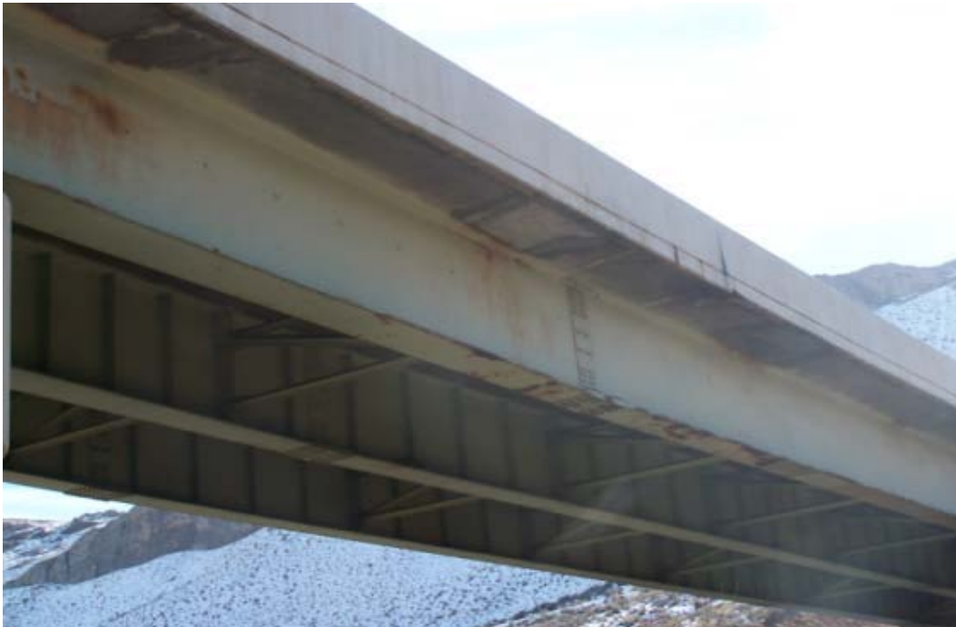
Figure 5. Photo. Corrosion of the existing bridge steel girders.
