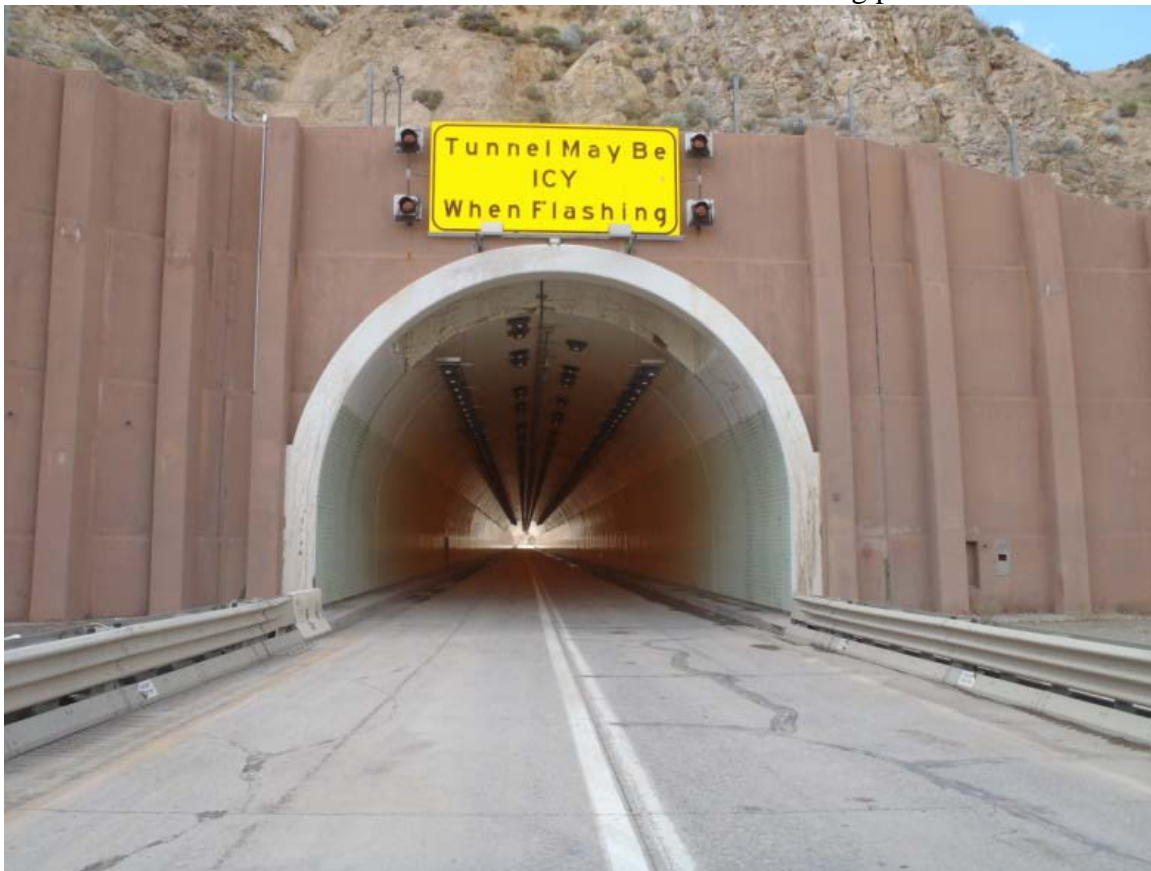
Figure 3. Photo. Existing Carlin Tunnel and the approach slabs with surface distress.
