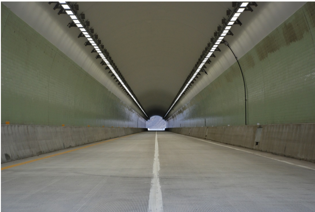
Figure 14. Photo. New LED lighting system.
