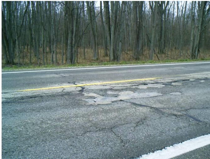
Figure 6. Typical delamination of HMA overlay.
