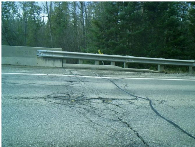
Figure 7. Deteriorated bridge leave joint over Doc and Tom Creek.
