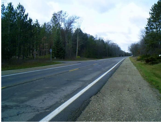
Figure 2. Overview of deteriorated pavement showing structural distress in the wheelpath.
