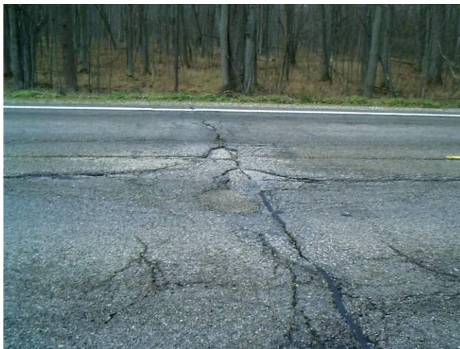
Figure 4. Typical deteriorated PCC joint reflecting through the HMA overlay.
