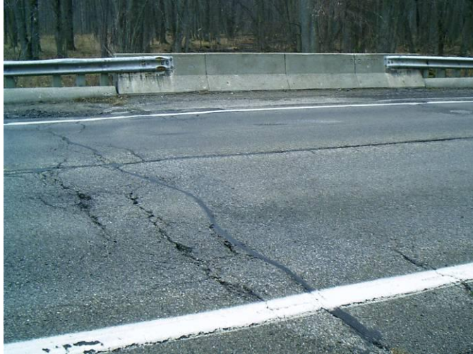
Figure 5. Deteriorated bridge approach joint over Doc and Tom Creek.
