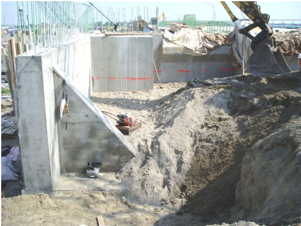
Figure 12. Granular material behind the abutment.
