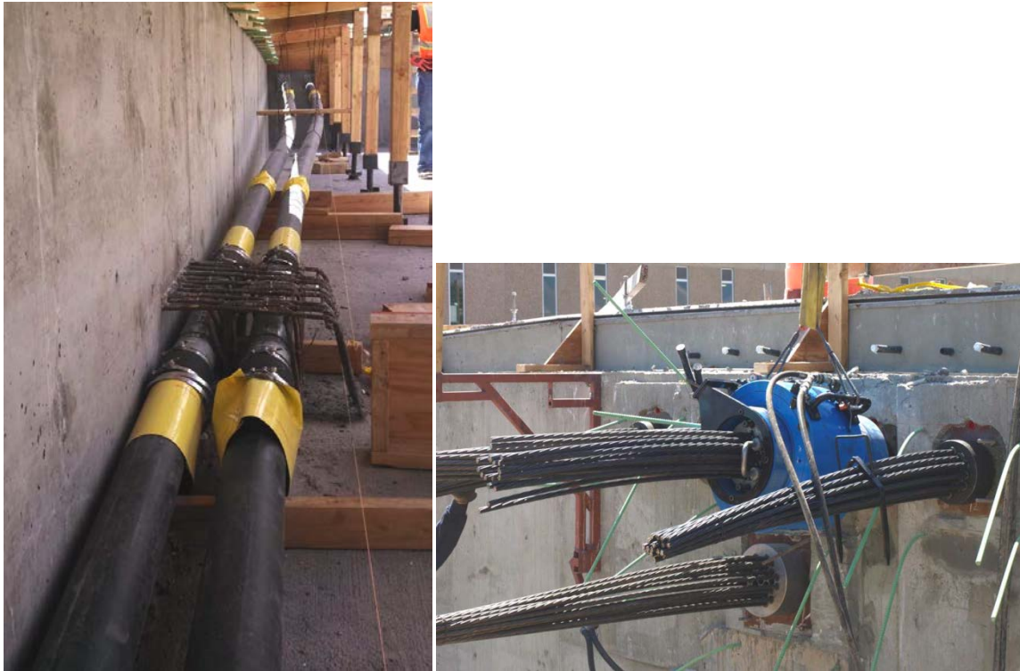
Figure 18. Photos. Longitudinal external tendons (courtesy: Colorado DOT).
