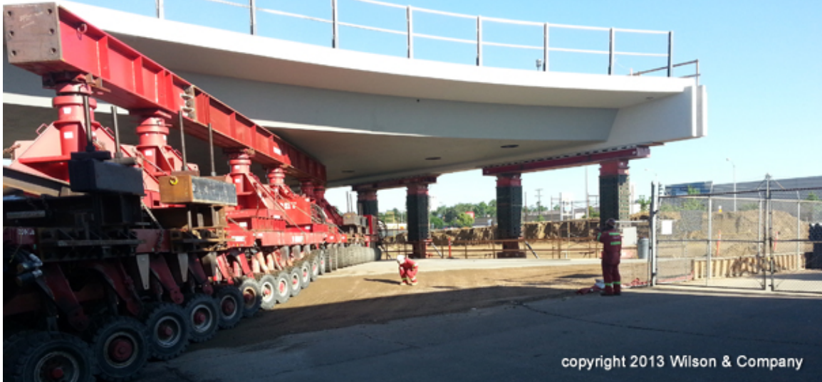
Figure 24. Photo. Operator rolling SPMT into position under the lifting diaphragms (courtesy: Colorado DOT).
