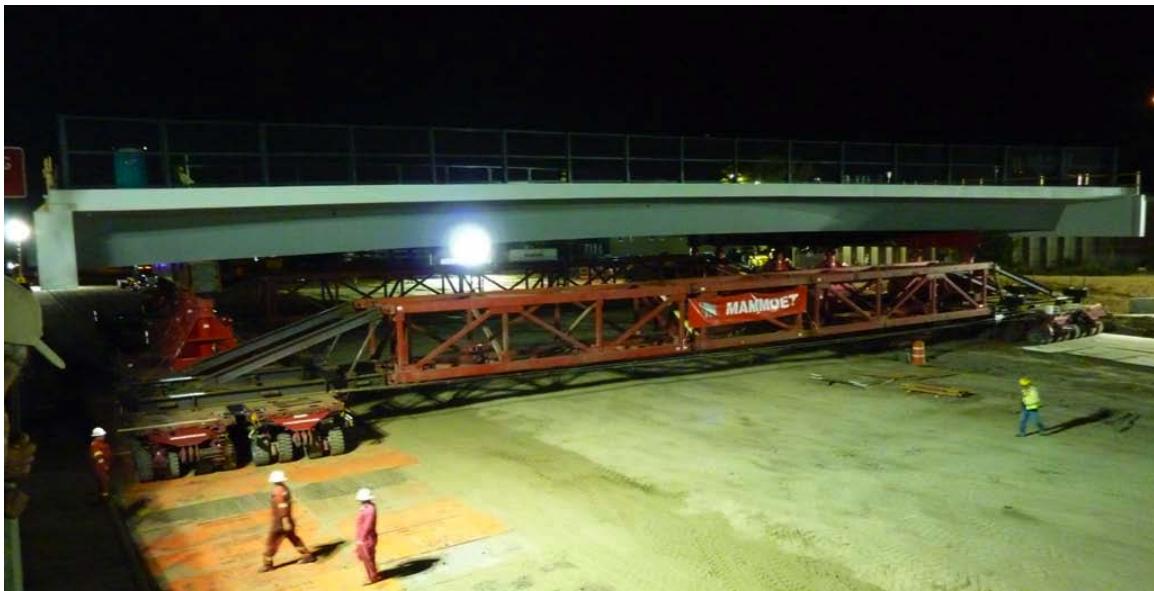
Figure 31. Photo. SPMT traveling over steel plates westward on I-70 (courtesy: Colorado DOT).
