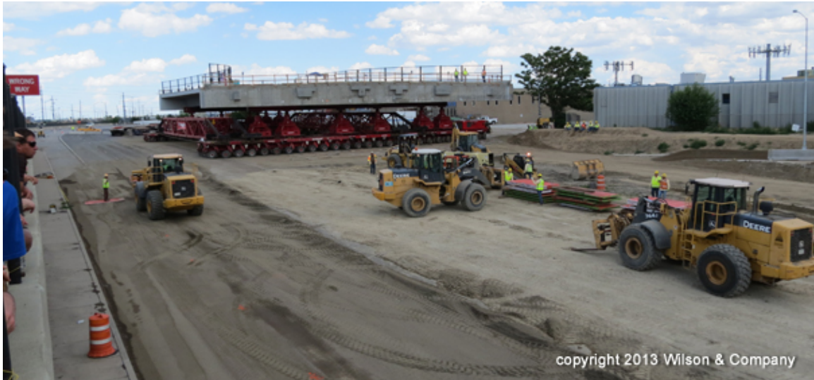
Figure 30. Photo. Superstructure on SPMT preparing to get on to I-70 (courtesy: Colorado DOT).
