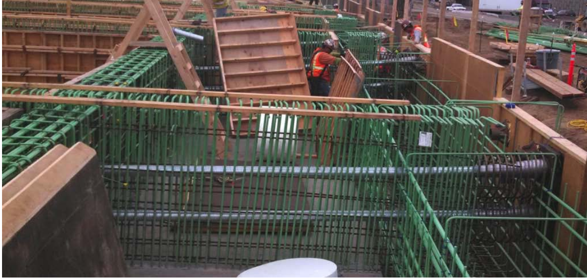
Figure 17. Photo. Longitudinal internal tendons (courtesy: Colorado DOT).
