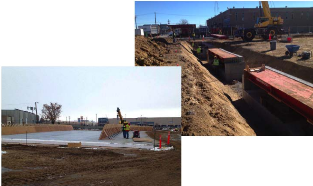
Figure 11. Photos. “Trench and “rat slab” construction in bridge staging area (courtesy: Colorado DOT).
