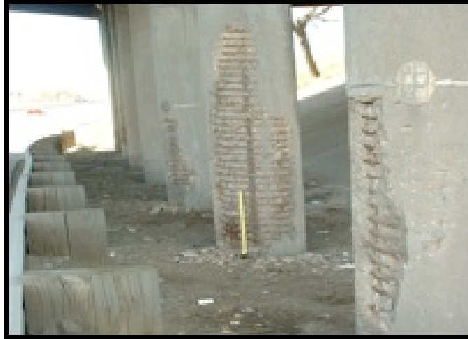
Figure 4. Photo. Spalling of columns (courtesy: Colorado DOT).
