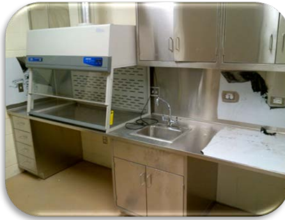
Exhibit 3. New agriculture laboratory being installed with fume hood (to mix chemicals) to the left of the sink.
