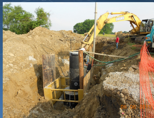
This project on U.S. 231 impacted 15 separate utilities on the western edge of Purdue University in West Lafayette, IN.
