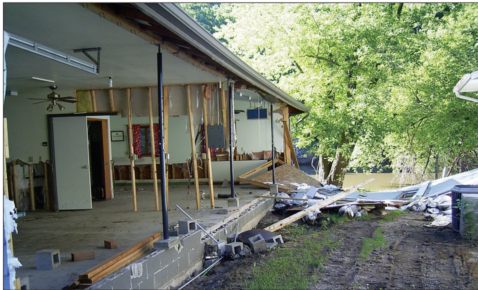
Figure 2-10. Water moving at high velocity destroyed the wall of this home and caused the building to shift on its foundation.
