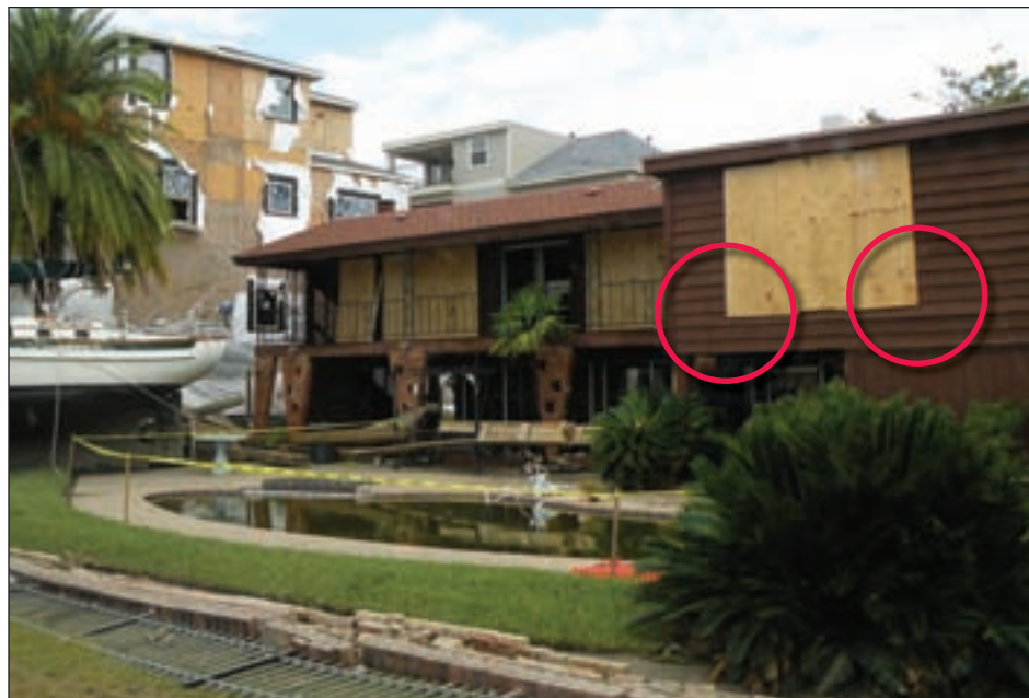
Figure 3-103. Plywood shutters installed into the wall cladding (red circles) in Clear Lake, TX (Hurricane Ike estimated wind speed in this area: 90 mph, Exposure B)
