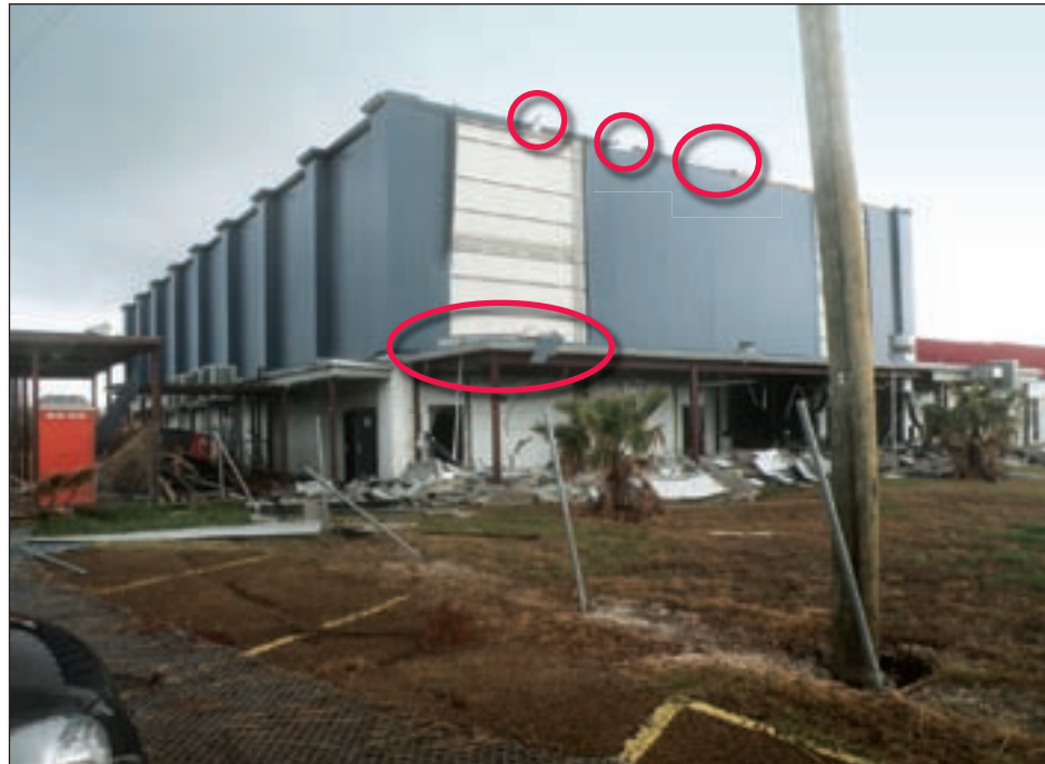
Figure 4-13. Johnson's Bayou School gymnasium. The red ovals indicate damage to canopy and roof.
