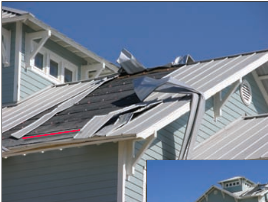
Figure 3-70. These architectural metal panels unlatched from the concealed clips. The red line shows location of the first row of clips (Galveston Island, TX; Hurricane Ike estimated wind speed in this area: 110 mph).
