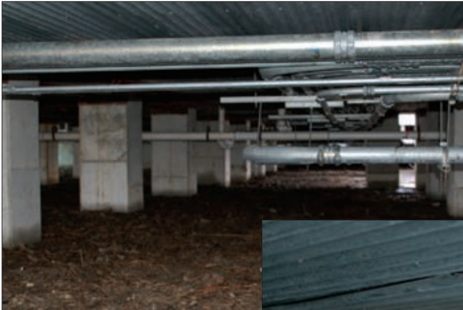
Figure 4-33. Conduits and pipes beneath South Cameron Parish Hospital. Vegetation was noted between the floor system and the steel plate of the foundation. A connection between the plate and the floor system was not visible.
