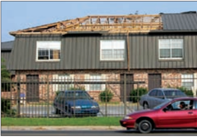
Figure 6. Blow-off of nailers caused these panels to progressively fail. The nailers were installed directly over the trusses. In an assembly such as this where there is no decking, there is no opportunity to incorporate an underlayment. With loss of the panels, rainwater was free to enter the building.
