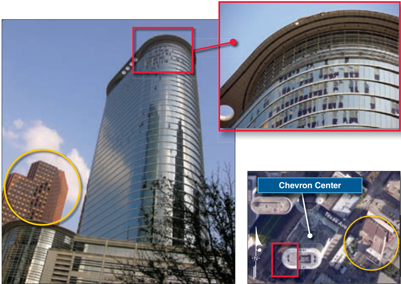
Figure 5-17. Chevron Center glazing damage. At the building beyond (yellow circle), at least 35 windows were boarded up. Bottom inset shows location.
