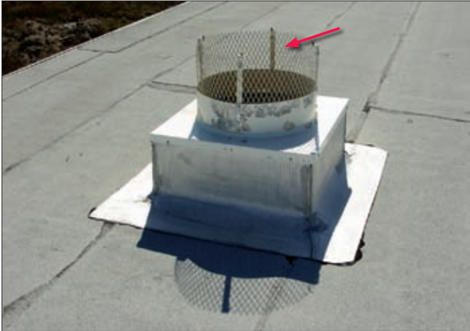
Figure 4-5. Wind blew off the hood, allowing rain to directly enter the building
