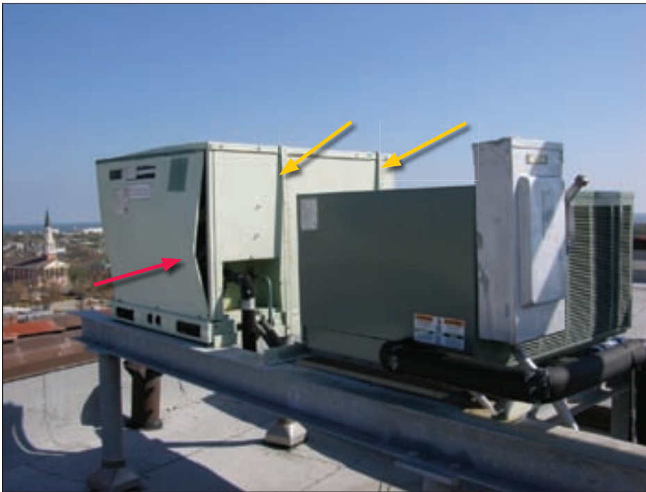
Figure 4-64. The access panel (red arrow) nearly blew away; the yellow arrows indicate supplementary anchor straps
