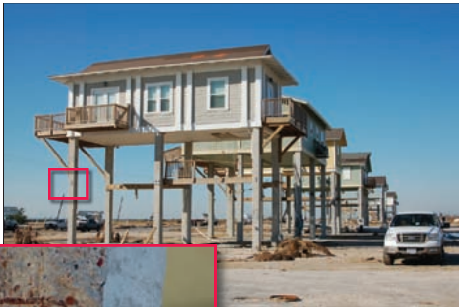
Figure 3-14. Ground-level view of elevated houses with inset showing typical column damage where the timber deck broke away (Bolivar Peninsula, TX)
