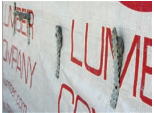
Figure 5. These four ties were never embedded into the mortar joint.
