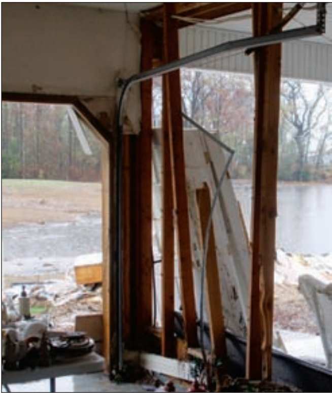
Figure 6. Damage attributed to small waves and approximately 5' of stillwater depth (Bridge City, TX, Hurricane Ike).
