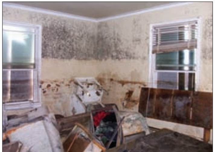
Figure 6. Other concerns when flood levels rise above the lowest floor are mold and biological/chemical contamination. These may render an otherwise repairable building unrepairable, or will at least make the cleanup, restoration, and repairs much more expensive and time-consuming.
