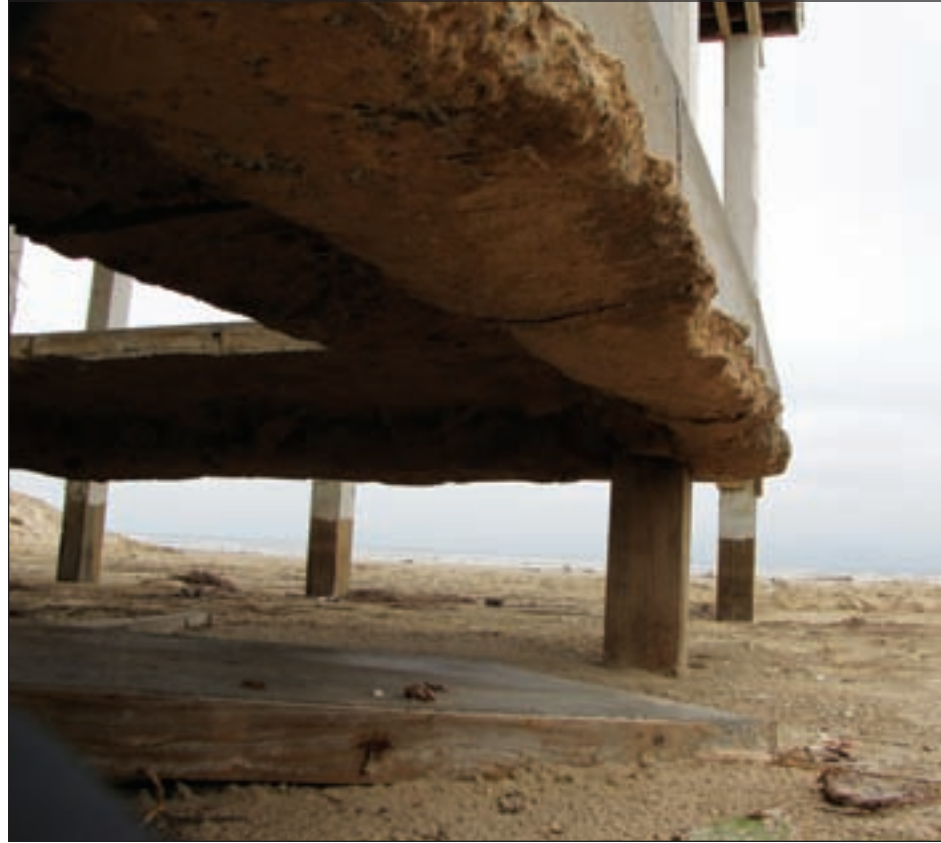
Figure 3-125. Pile-founded house with a slab thickened to create grade beams. The unthickened portion of the slab collapsed when undermined (Galveston Island, TX).
