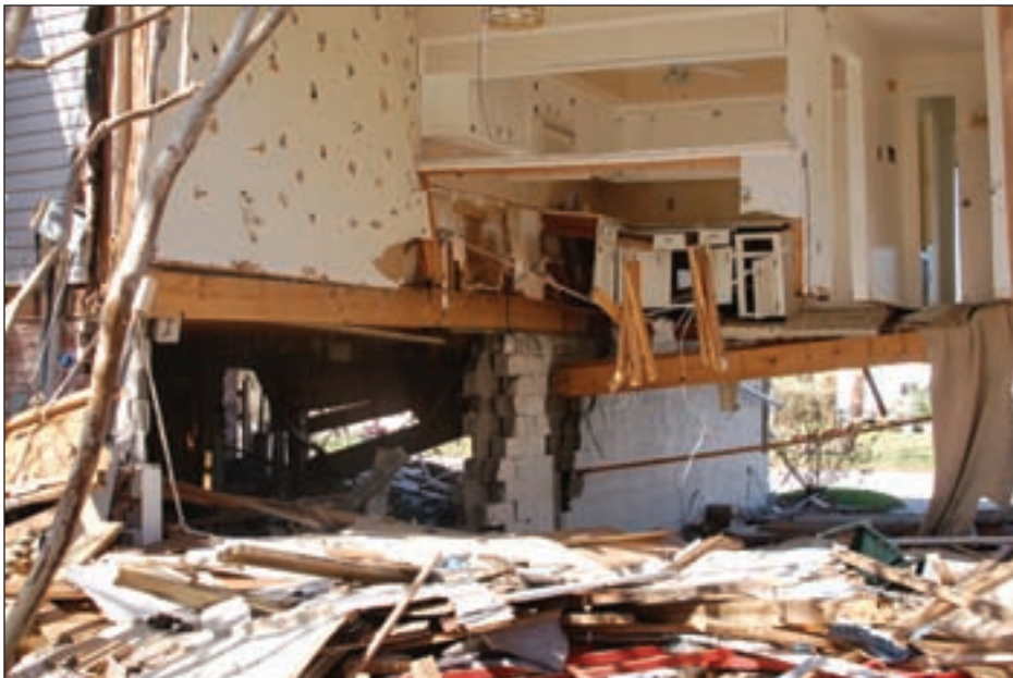
Figure 3-36. Likely wave and debris damage to townhouse building along the western Galveston Bay in Seabrook, TX. The building was supported on shore-parallel masonry walls, and is landward of another building that was destroyed by Ike.
