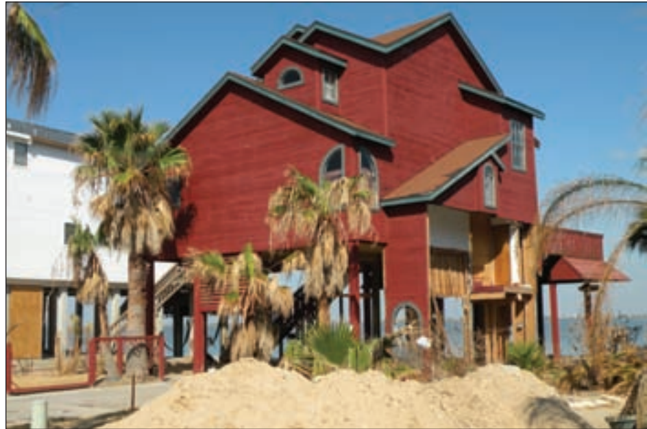
Figure 3-93. Clapboard-sided house with siding that performed well; damage resulted from failure of a non-breakaway wall (Tiki Island, TX; Hurricane Ike estimated wind speed in this area: 103 mph, Exposure C)
