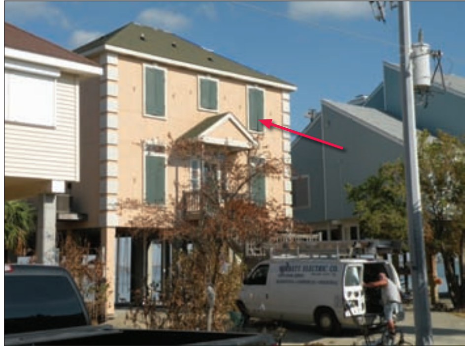
Figure 3-99. Traditional wood swinging shutters on Tiki Island, TX (Hurricane Ike estimated wind speed in this area: 103 mph, Exposure B)
