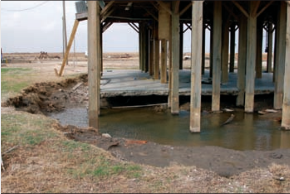
Figure 3-19. Foundation scour observed at Holly Beach, LA (Zone V, ABFE = 16 feet)
