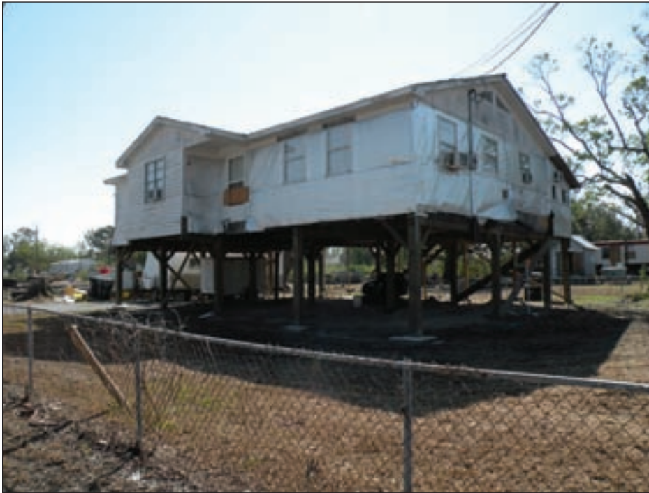
Figure 3-73. Loss of siding due to winds, Chauvin, LA (Terrebonne Parish; Hurricane Ike estimated wind speed in this area: 50 to 60 mph, Exposure B)
