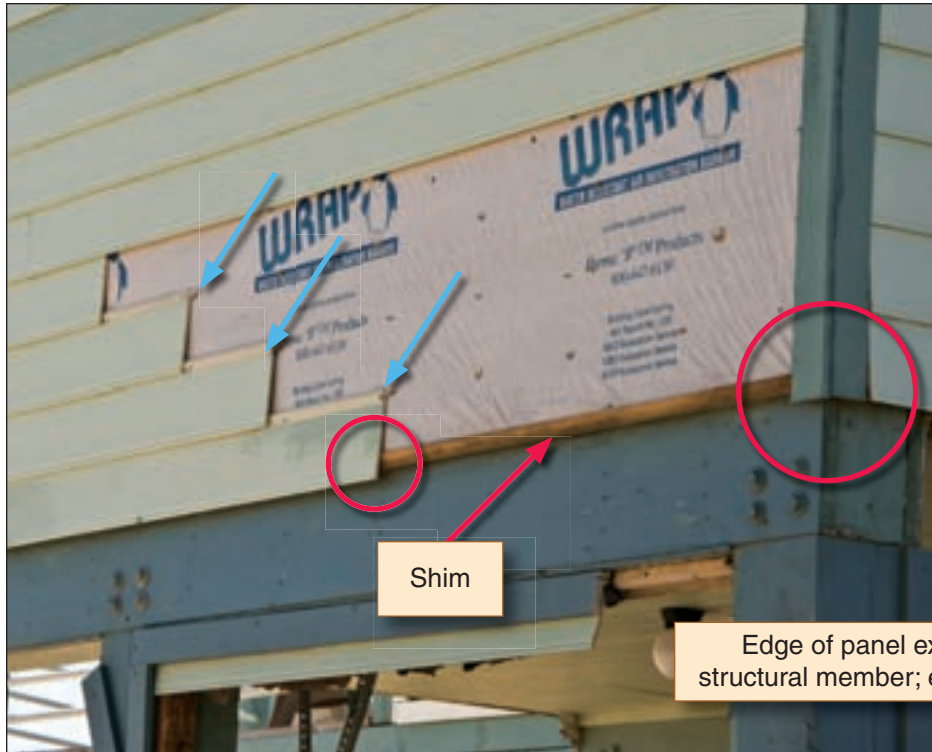
Figure 3-91. Shim placement (red arrow) allowed the lower edge (red circles) of siding to be exposed, resulting in loss of siding at several locations around this elevated structure on Bolivar Peninsula, TX. Note the blind nailing shown by blue arrows (Hurricane Ike estimated wind speed in this area: 110 mph, Exposure C).
