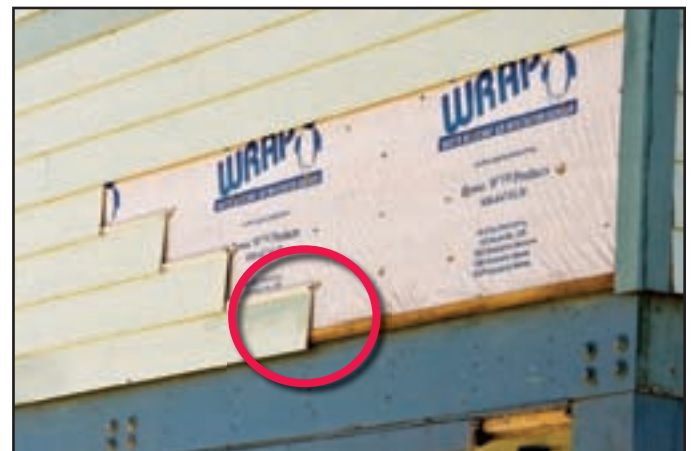
Figure 12. Blind nailed siding installed with exposed gap at bottom (red circle) is vulnerable to failure.
