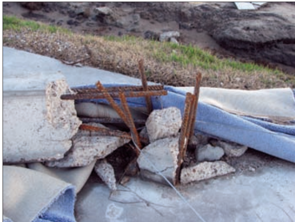
Figure 3-4. This concrete column failed due to lateral loads. Note limited overlap of reinforcing steel at the bottom of the column.
