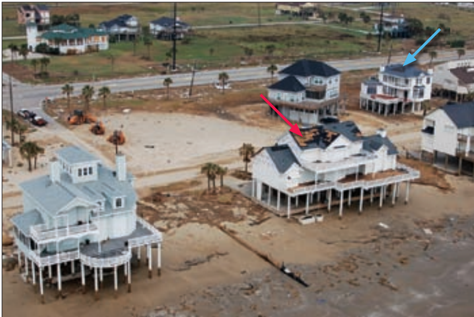
Figure 3-60. Some of the roofs on these Jamaica Beach, TX, houses had no roof covering damage, while one had moderate damage (blue arrow) and one had extensive damage, including loss of underlayment (red arrow) (Hurricane Ike estimated wind speed in this area: 90 mph)
