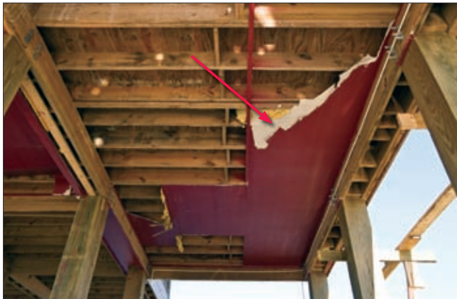
Figure 3-120. Fiber cement board sheathing (red arrow) was removed from the underside of this house, which was elevated approximately 12 feet above ground level (Bolivar Peninsula, TX)
