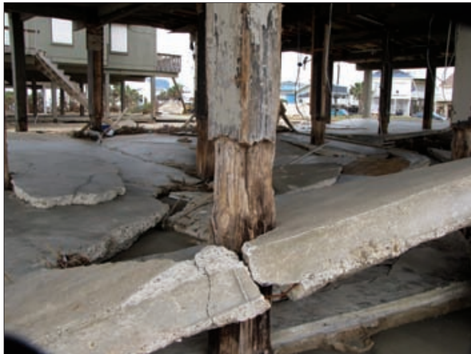
Figure 3-28. Deterioration in wood piling. The foundation did not fail during Ike, but it was weakened and will be more susceptible to failure in the future (Galveston Island, TX).
