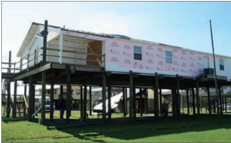
Figure 3-137. This elevated manufactured home in Grand Isle of Jefferson Parish, LA, had siding and roof damage, but did not move from its foundation
