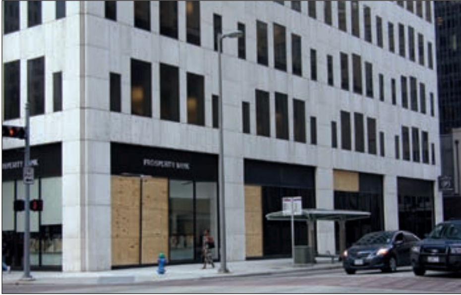
Figure 5-3. Random breakage of first floor glazing
