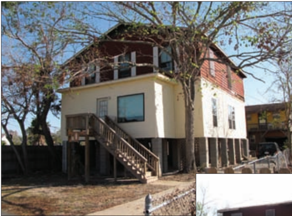
Figure 3-142. House elevated with Increased Cost of Compliance funds (Kemah, TX). Inset shows evidence of wind damage to roof (Hurricane Ike estimated wind speed in this area: 90 mph, Exposure B).
