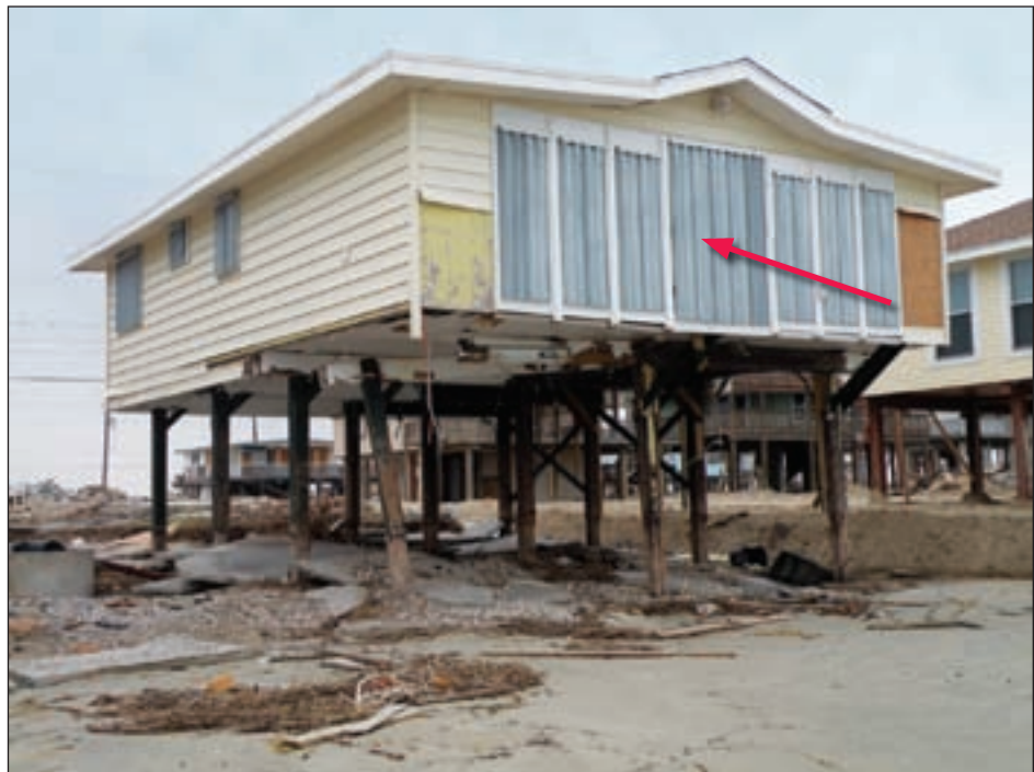
Figure 3-100. Corrugated metal shutters on house in West Galveston, TX (Hurricane Ike estimated wind speed in this area: 95 mph, Exposure C)
