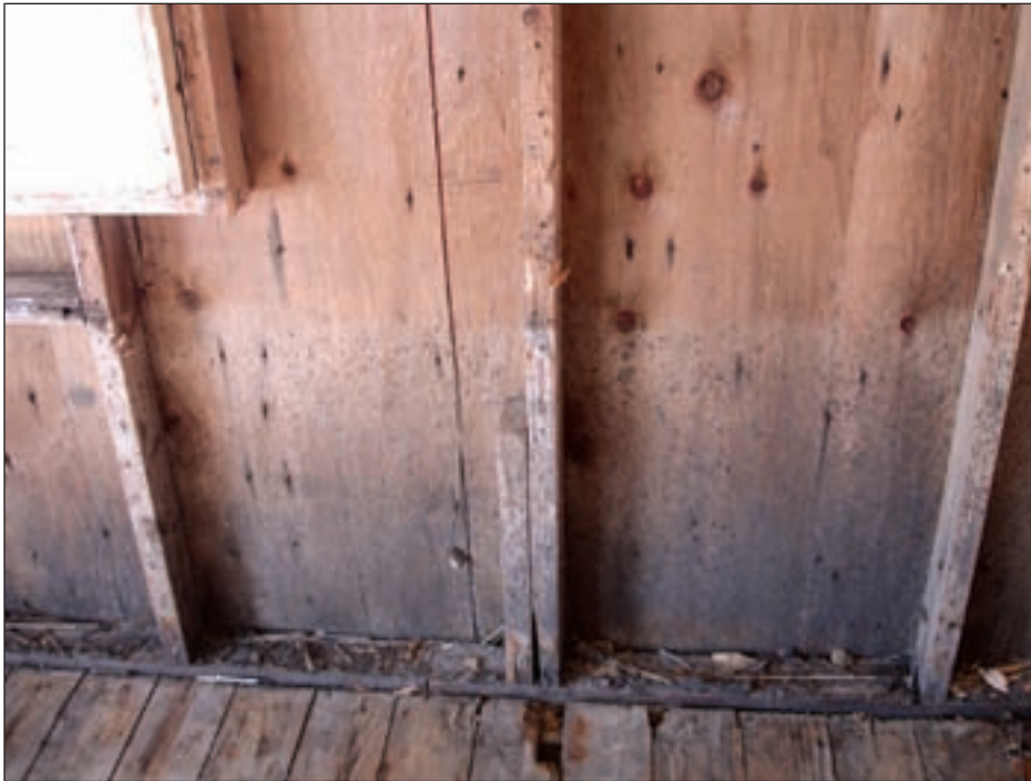
Figure 3-130. Mildew and mold forming on wall sheathing following flooding (Golden Meadow, LA)
