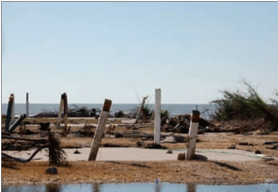
Figure 3-2. A house on timber piles was pushed over by wind and flood loads and the load path failed at the connection between the floor beam and the piles. Embedment and elevation were also insufficient at this Bolivar Peninsula, TX, site.
