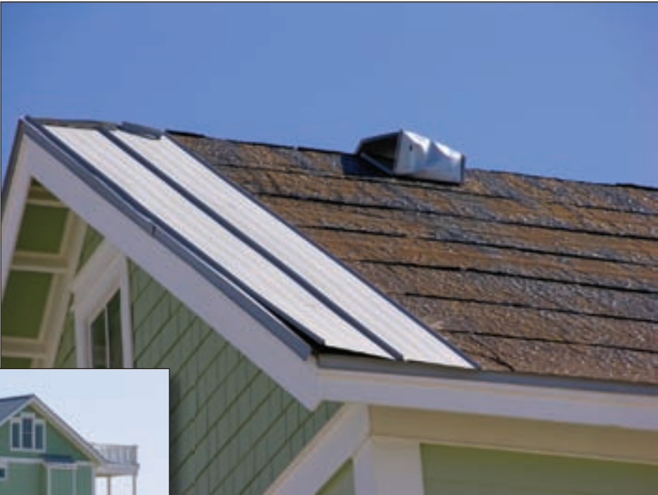
Figure 3-69. These snap-lock seam panels were attached with fasteners through one side of the seam (Galveston Island, TX; Hurricane Ike estimated wind speed in this area: 110 mph)
