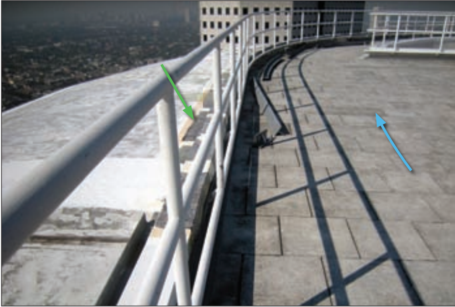
Figure 5-21. View of the damaged window washing track (green arrow). The concrete pavers (blue arrow) were not damaged.
