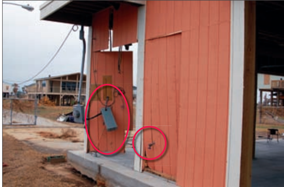
Figure 3-115. Attachment of utilities to breakaway wall may have prevented the wall from breaking away, thereby resulting in additional damage to the structure (Galveston Island, TX)
