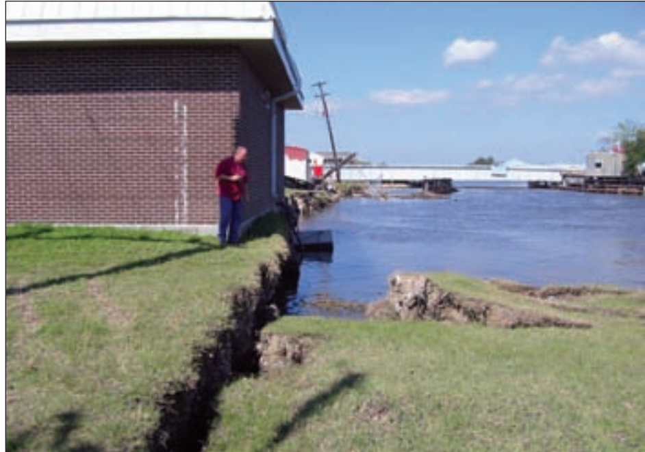
Figure 4-56. Rear of Dularge Fire Station; note canal bank erosion sustained during Hurricane Ike
