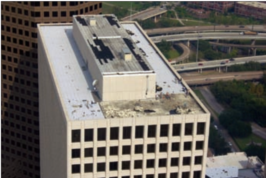
Figure 5-28. Roof covering damage on the main and penthouse roofs of building B-1
