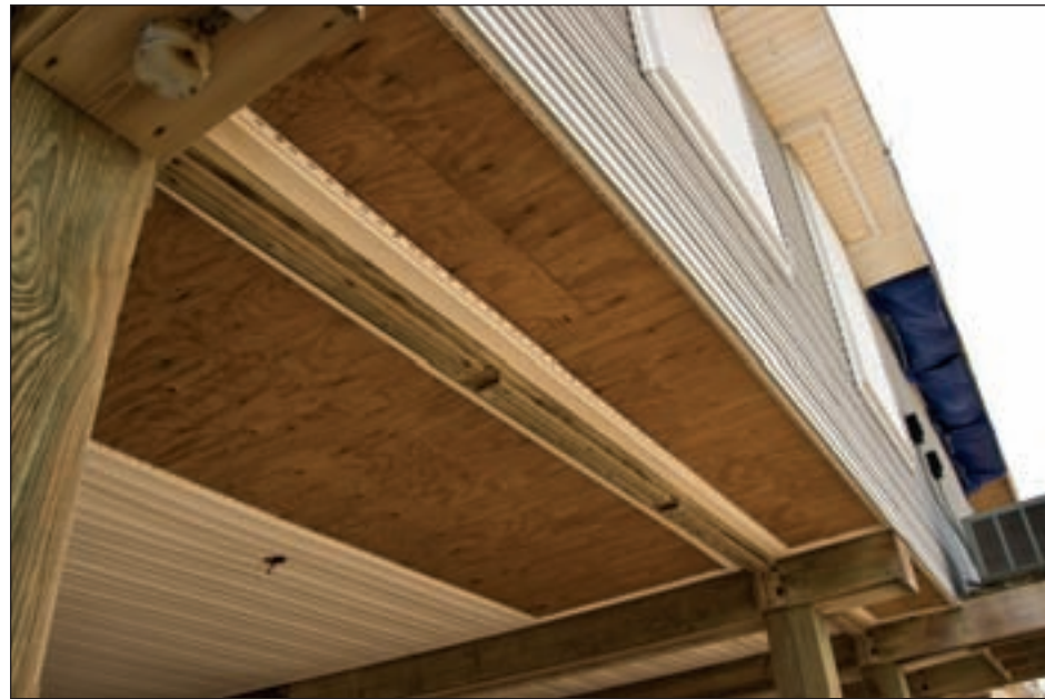
Figure 3-122. Vinyl soffit covering over plywood sheathing partially removed (Tiki Island, West Galveston Bay; Estimated Hurricane Ike wind speed: 103 mph, Exposure C)
