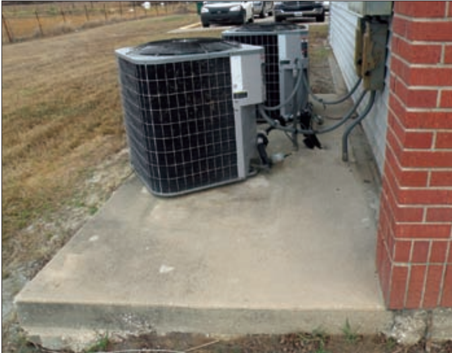
Figure 4-58. Condenser units were installed at Hackberry Fire Station after Ike and are vulnerable to future flooding
