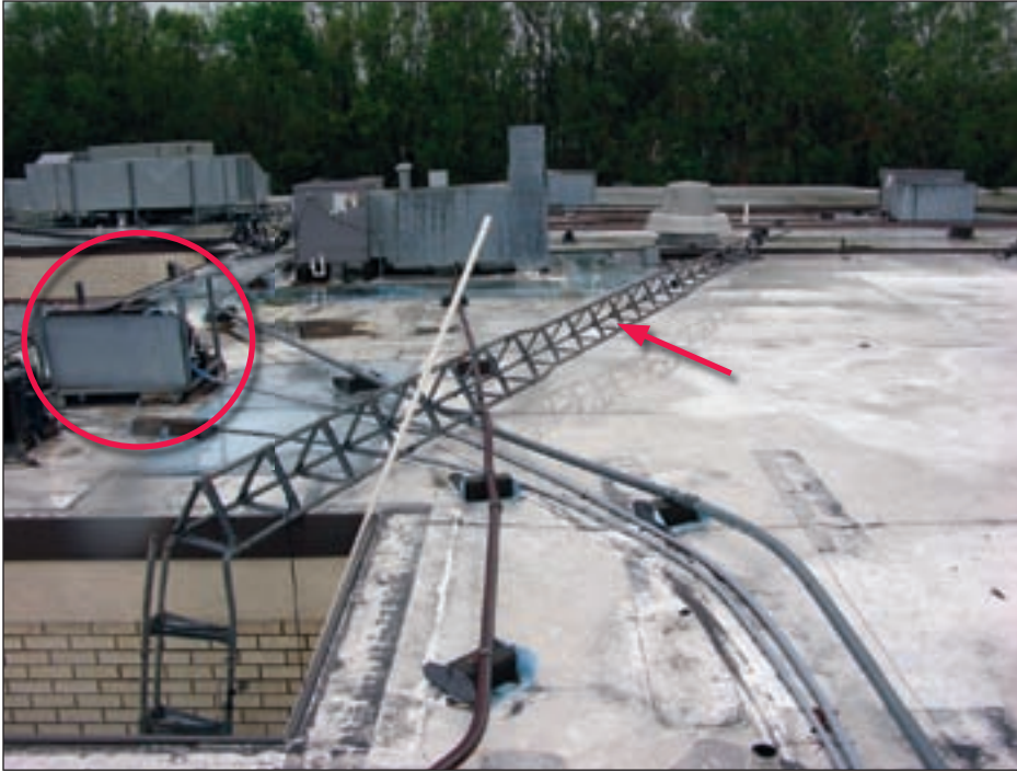
Figure 4-21. Collapsed communications tower and blown-away access panels (red circle)
