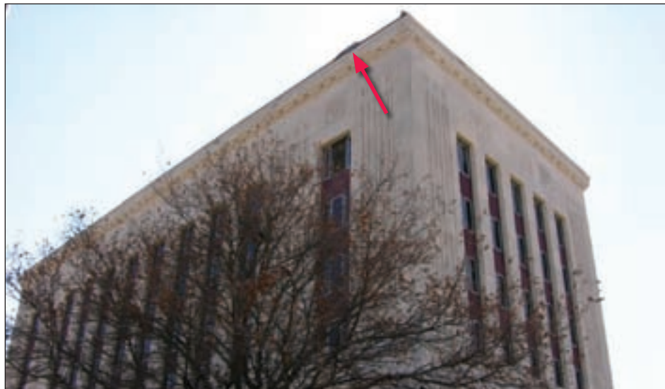
Figure 4-62. General view of Federal Courthouse and Post Office; some flashing damage occurred during Hurricane Ike (shown by red arrow)
