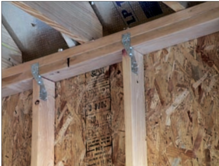
Figure 3-53. Studs clipped to double top plate; rafter-to-top-plate connector has yet to be installed. Better framing practices could have avoided some of the problems shown in this photo. Ceiling joists are not well nailed to the rafter and may twist in the future. The builder did not take advantage of aligning wall framing and rafter framing to simplify connections for wind loads.
