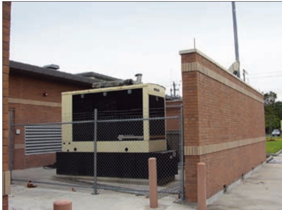
Figure 4-49. The emergency generator is inadequately protected from wind and windborne debris
