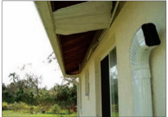
Figure 1. Missing soffit material.
