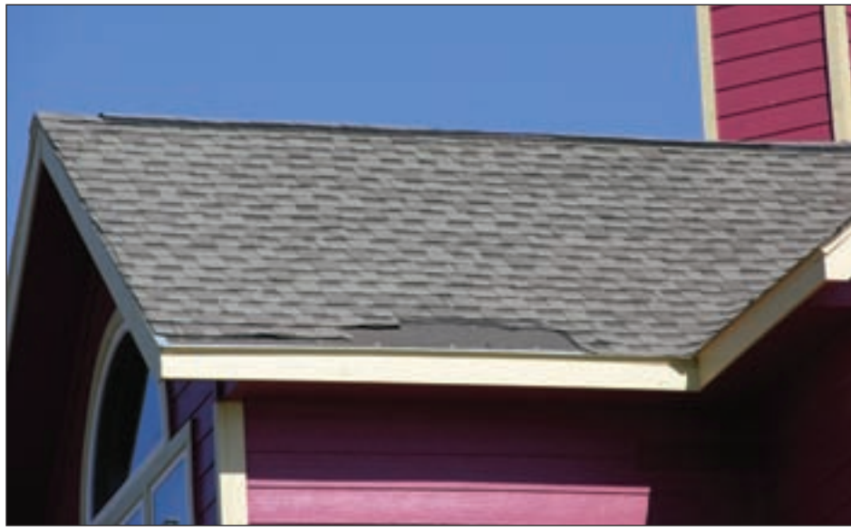
Figure 3-63. Loss of shingles along the eave in Bolivar Peninsula, TX (Hurricane Ike estimated wind speed in this area: 110 mph)
