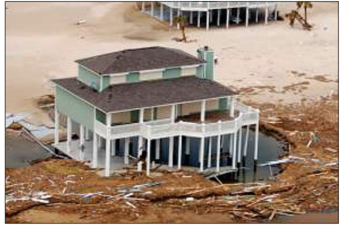
Figure 7. Extreme local scour around a Gulf-front pile foundation (Bolivar Peninsula, TX, Hurricane Ike).
