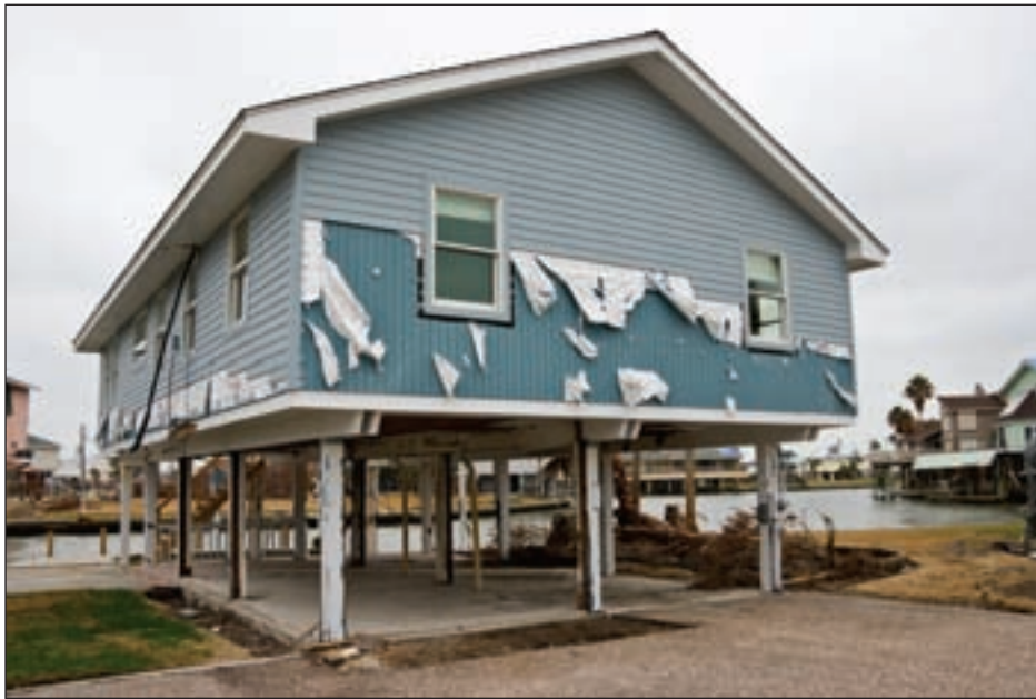
Figure 3-88. Fiber cement lap siding was blown off this West Bay, Galveston Island, TX, house (Hurricane Ike estimated wind speed in this area: 100 mph, Exposure B)
