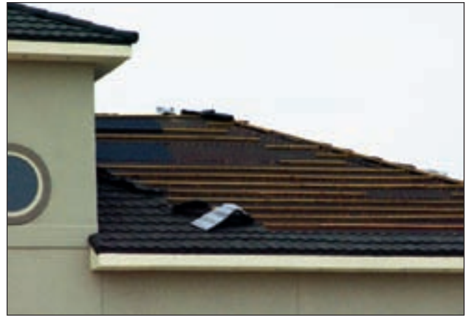
Figure 7. This residence had metal shingles that simulated the appearance of tile. The shingles typically blew off the battens, but some of the battens were also blown away.
