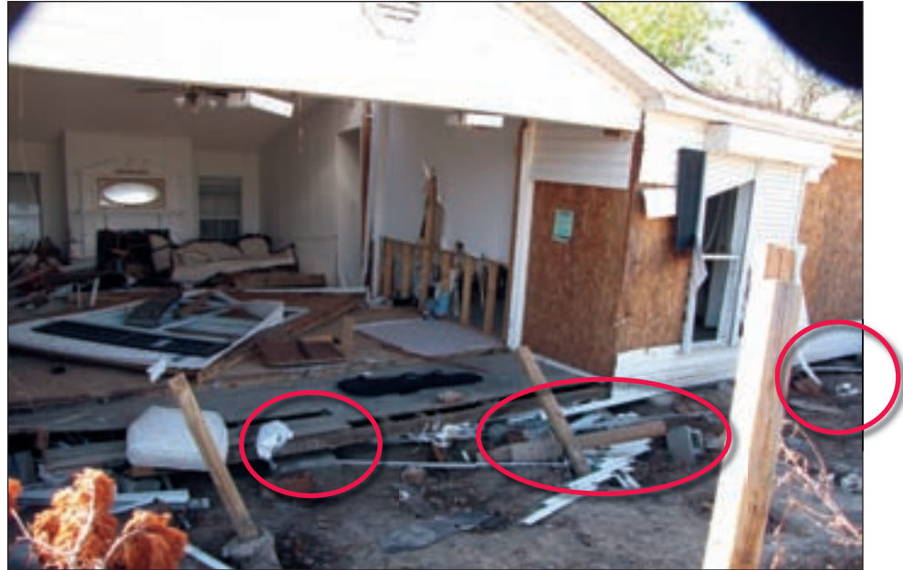
Figure 3-134. Scour depressions existed around the masonry piers, pads, and ground anchor stabilizer plates (San Leon, TX)
