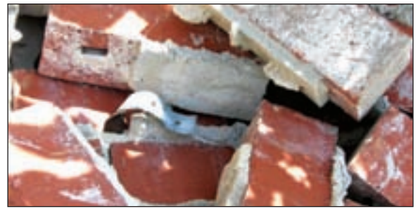
Figure 4. This tie remained embedded in the mortar joint while the smooth-shank nail pulled out from the stud.
