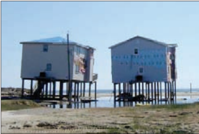
Figure 8. Differential settlement of buildings thought to be a result of inadequate foundation embedment coupled with erosion, scour, and/or soil liquefaction (Surfside Beach, TX, Hurricane Ike).
