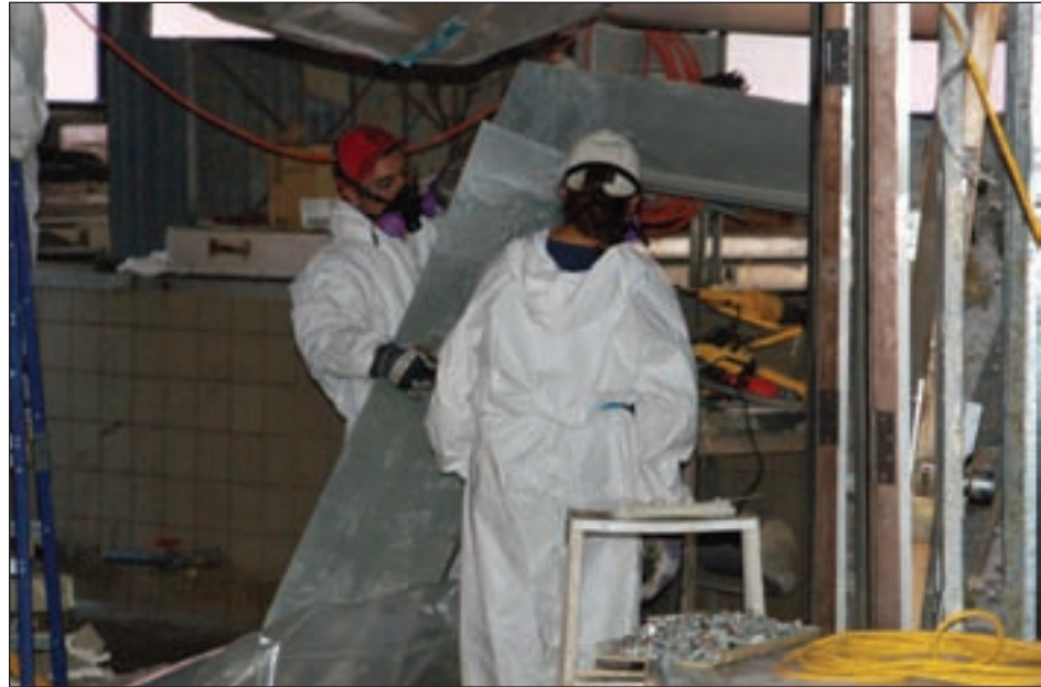
Figure 4-24. Clean-up underway inside the basement of UTMB Building 1. All the laboratory equipment, office and classroom contents, and interior finishes had to be decontaminated and removed for disposal.
