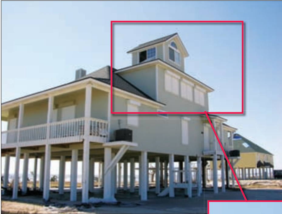
Figure 6-2. The upper windows on this Seabrook, TX, residence were not shuttered and were vulnerable to windborne damage
