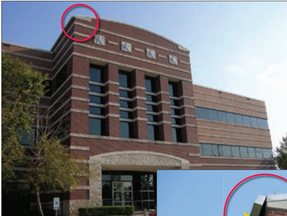
Figure 4-41. Houston Transtar Regional EOC; significant permanent outward deformation occurred at the gutter shown in the inset
