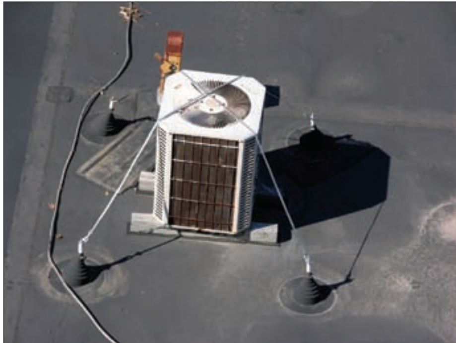
Figure 4-15. Condenser with tie-down cables
