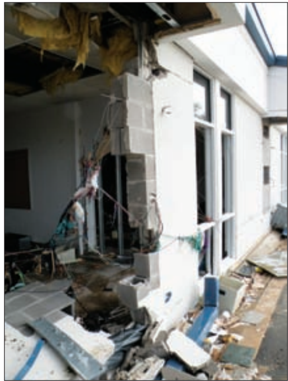
Figure 7. Damage believed to have resulted from Coastal A-zone conditions (Johnson Bayou, LA, Hurricane Ike).
