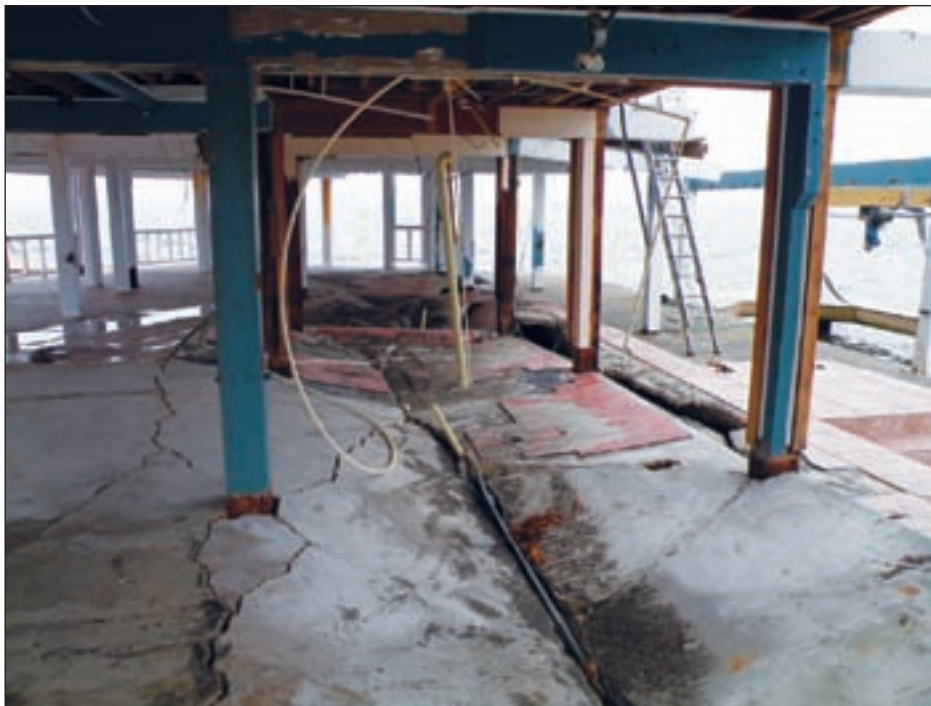
Figure 2-9. First floor walls removed and floor slab undermined by flooding and waves at this Jamaica Beach house (number 2480 in 1990 Galveston study)
