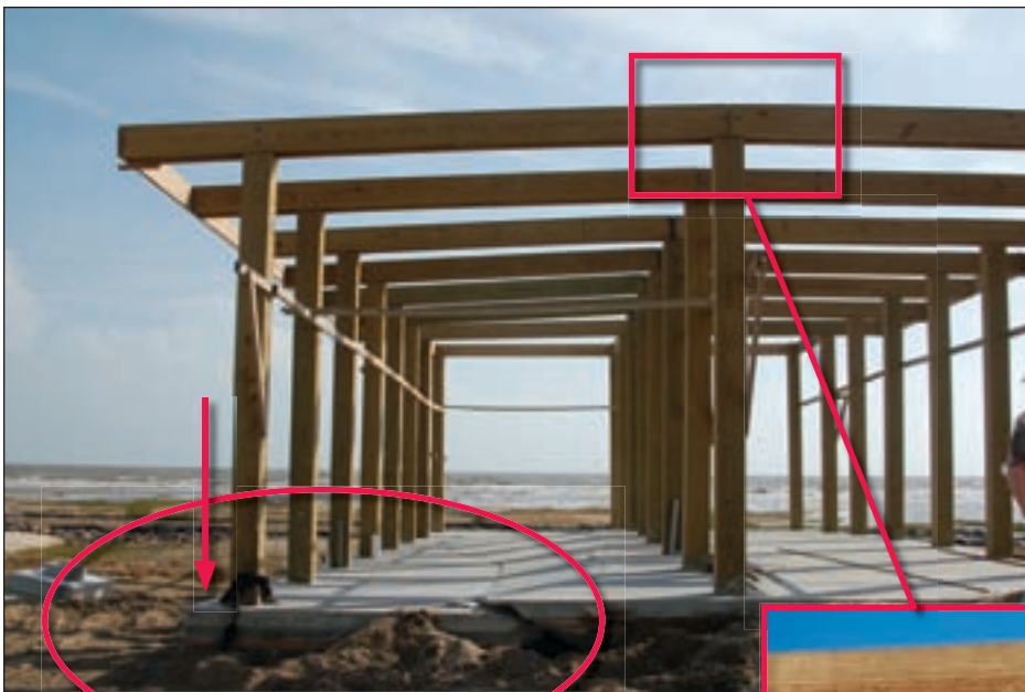
Figure 3-127. Slab undermining and settlement during Ike probably pulled piles downward. Inset shows that the dropped piles also caused the floor beam to deflect (Holly Beach, LA).
