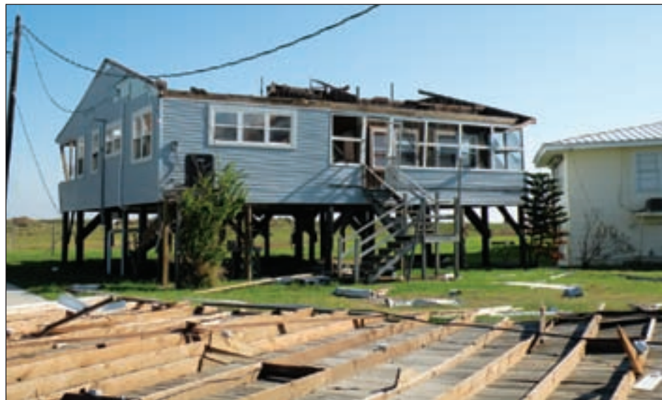
Figure 3-41. The roof structure was poorly connected to this house in Grand Isle (Jefferson Parish, LA) and was blown off by 50-mph Ike winds (Exposure B)
