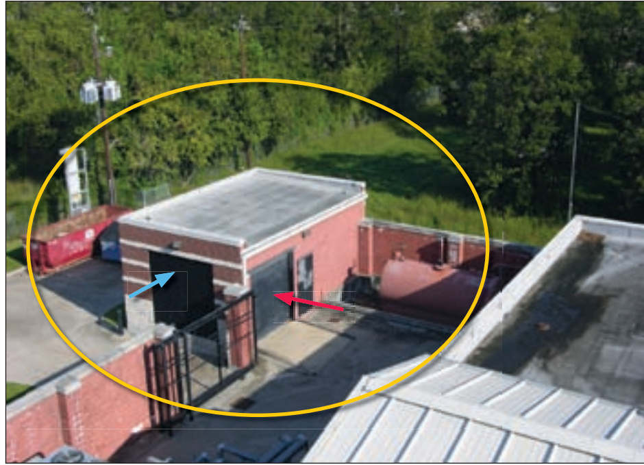
Figure 4-46. The emergency generator is housed in the circled building; the coiling door (red arrow) and the louver (blue arrow) appeared to provide inadequate protection for the generator
