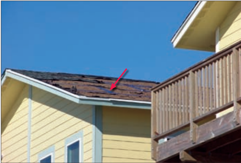
Figure 3-67. This Fortified...for safer living ® house had taped sheathing joints (red arrow)
