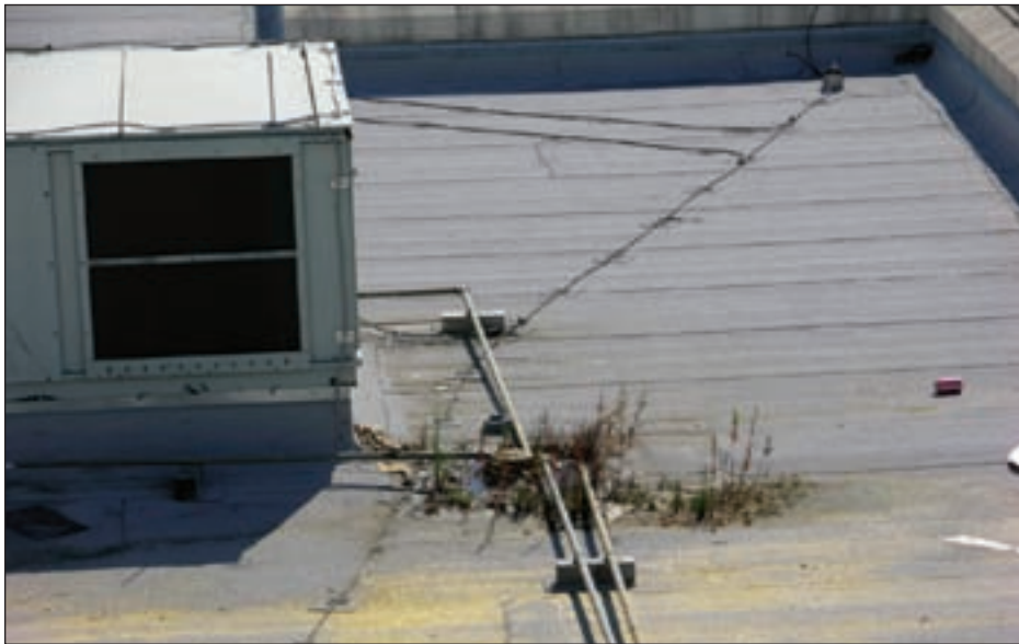
Figure 4-18. View of one of the mitigated roofs. Note the vegetation growth in the vicinity of the roof drain, indicating a lack of maintenance.
