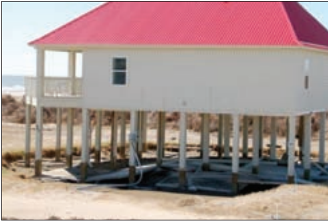
Figure 6. Local scour around a 3rd row house's pile foundation (Bolivar Peninsula, TX, Hurricane Ike).
