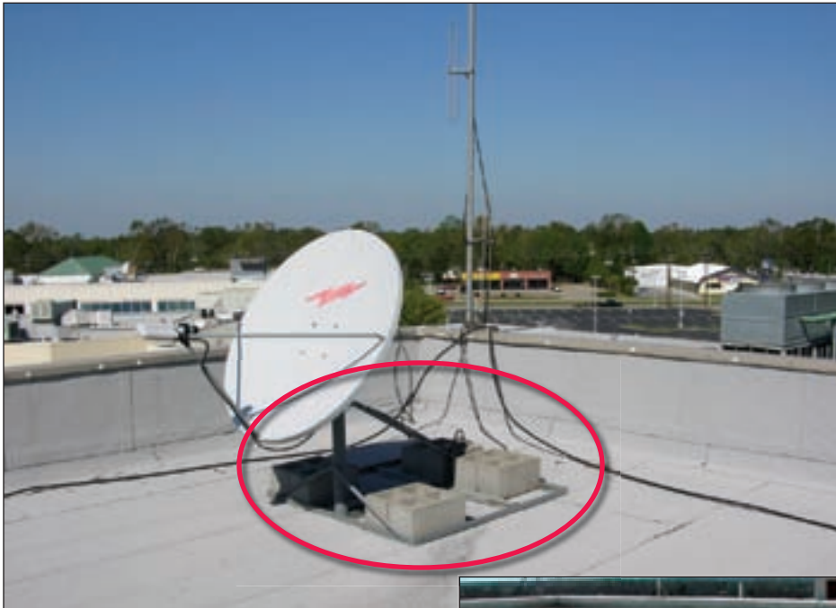
Figure 4-17. This satellite dish was held down with CMU only; inset shows all that remains from a similarly mounted dish after a strong hurricane
