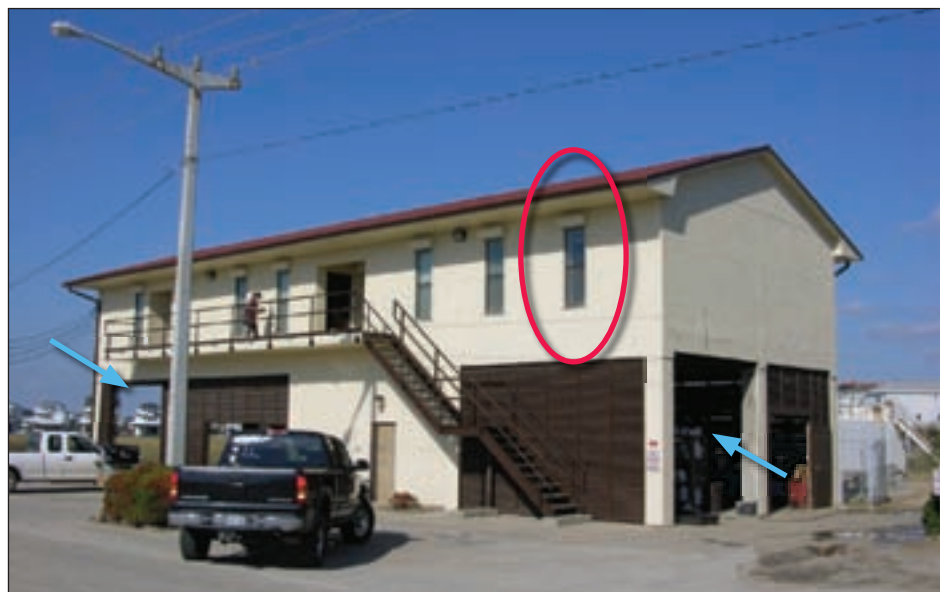
Figure 4-66. One of the shutters at the Tiki Island City Hall is shown in the red oval; blue arrows indicate breakaway walls that performed successfully by breaking away
