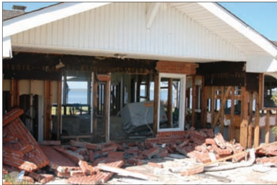
Figure 3-35. Damage to at-grade house in Zone V likely caused by wave and surge along the northern Galveston Bay shoreline in Baytown, TX
