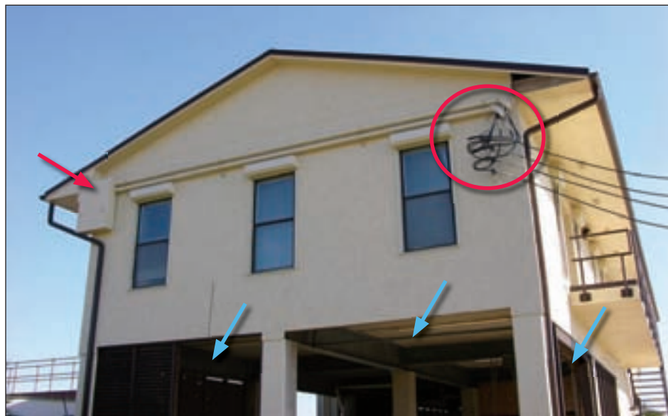
Figure 4-68. The electrical service entered through the wall rather than the roof; the blue arrows indicate missing breakaway walls
