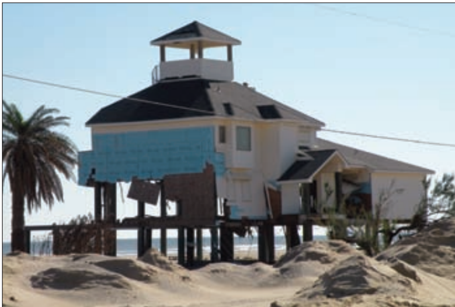
Figure 3-48. Though much of the cladding and structural sheathing was destroyed by Ike's surge, the MWFRS of this Bolivar Peninsula, TX, beach house remained intact and connected
