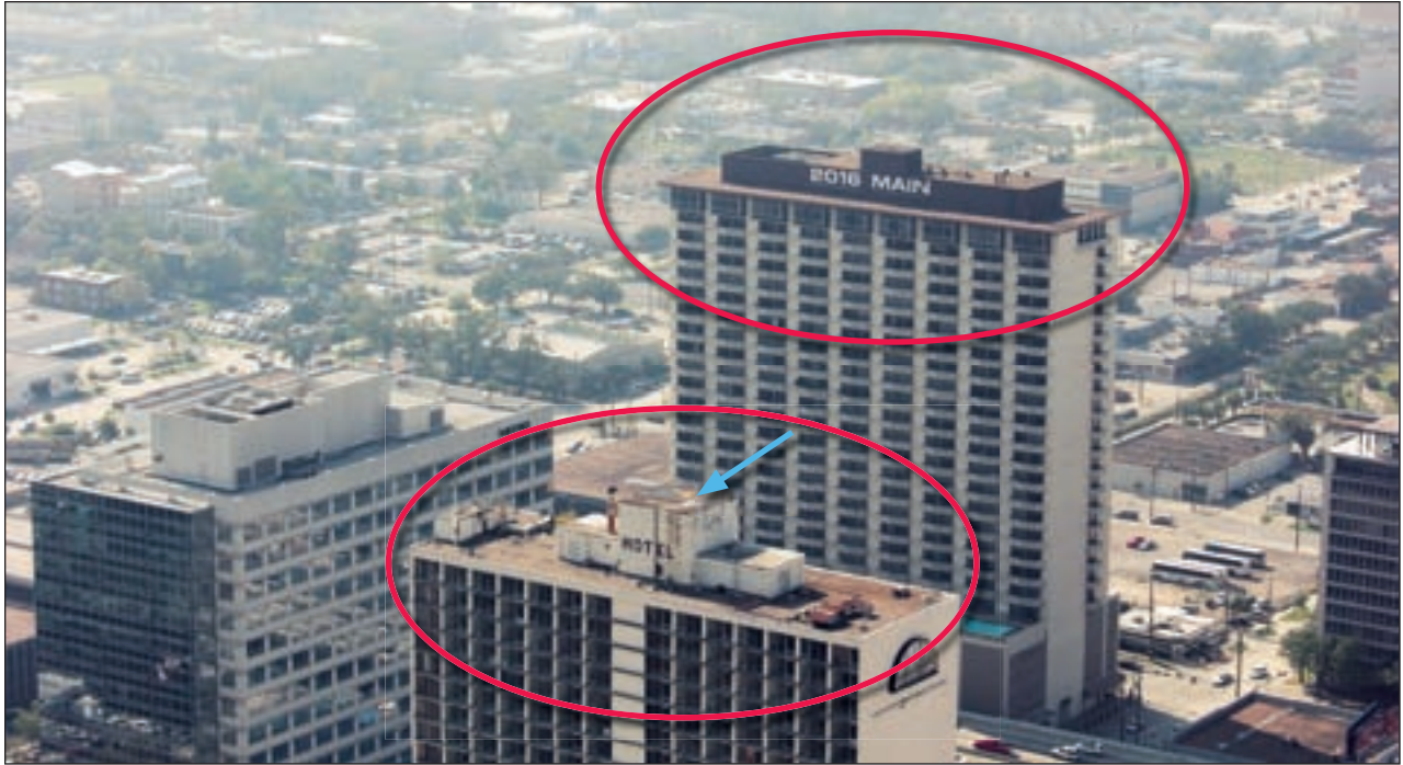
Figure 6-4. Aggregate-surfaced BURs on two mid-rise buildings on the periphery of Houston’s central business district. The roof membrane blew off the penthouse roof, shown by the blue arrow (Figure 5-19 inset shows building locations).
