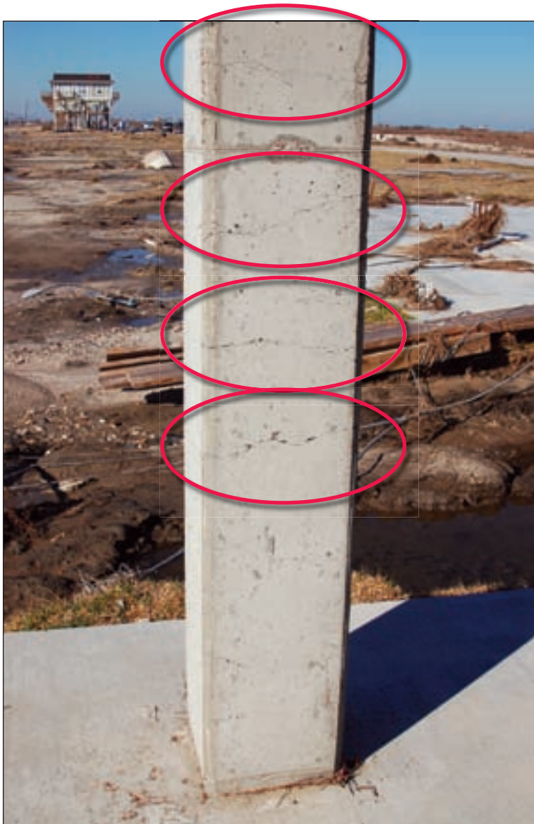
Figure 3-15. Concrete column showing cracking that was likely caused by extreme column bending stresses due to lateral loads on the elevated house and foundation (Bolivar Peninsula, TX)
