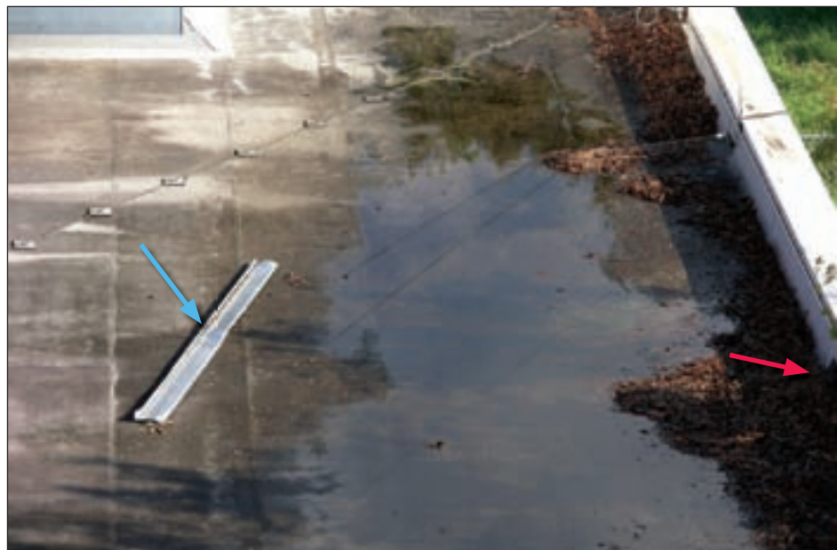
Figure 4-44. Coping debris (blue arrow) on a lower roof; note leaf debris near the scupper (red arrow)
