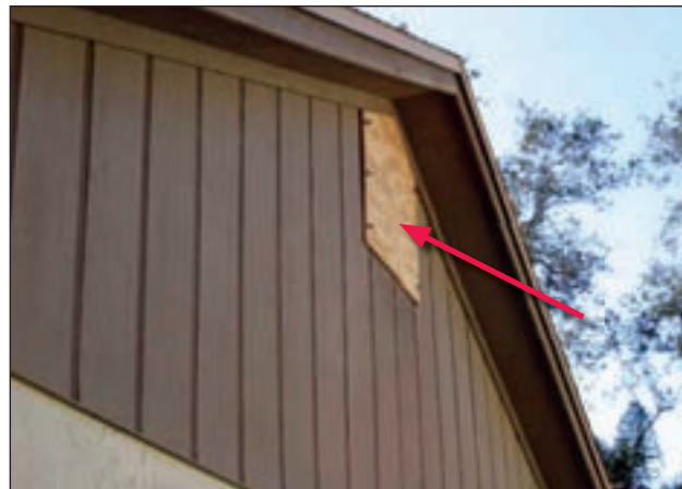
Figure 3-109. Shuttered gable end vent (red arrow)
