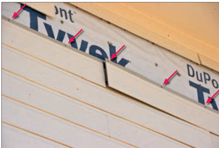
Figure 3-89. Damaged fiber cement plank siding. Note that blind nailing alone (red arrows) is recommended only for 90-mph or less installation. Higher wind zone installations should include both blind and face nailing (Hurricane Ike estimated wind speed in this area: 93 mph, Exposure B).
