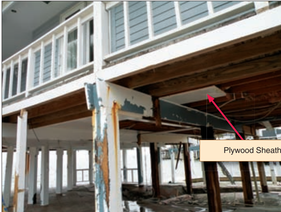
Figure 3-119. Plywood sheathing removed by storm surge (Jamaica Beach, TX, house on West Bay)
