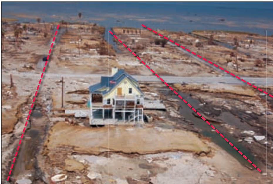
Figure 3-22. Linear scour features tend to align with canals and roads as storm surge returns to the Gulf. Houses such as this one were fortunate not to be undermined and lost during Ike, as many homes undoubtedly were (Bolivar Peninsula, TX).
