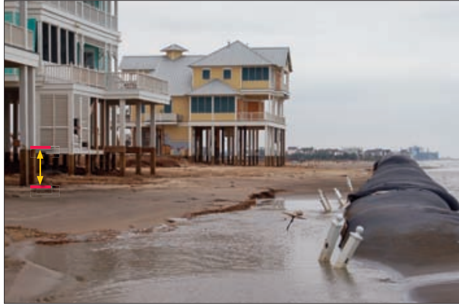
Figure 3-17. Exposed geotextile tubes formerly covered by sand and dune vegetation. Note erosion behind the tubes and under Zone V (BFE = 18 feet) buildings (yellow arrow at left).
