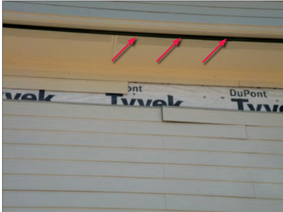
Figure 3-104. Fiber cement soffit remained connected; soffit vent slots shown with red arrows. Fiber cement plank siding was damaged (Tiki Island, TX; Hurricane Ike estimated wind speed in this area: 88 mph, Exposure B).
