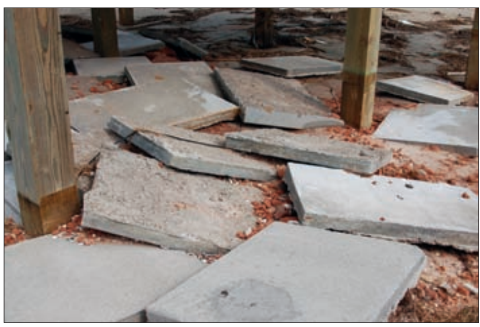
Figure 3-129. Thin, unreinforced parking slab sections separated when undermined and collapsed in place, with no apparent adverse impact to the foundation (Galveston Island, TX)
