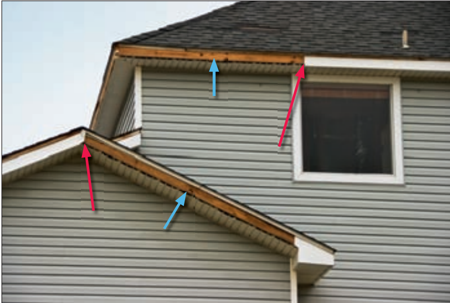
Figure 3-105. Loss of aluminum fascia cover (red arrows) exposed ends of vinyl soffit (blue arrows) to direct entry of wind-driven rain (Tiki Island, TX; Hurricane Ike estimated wind speed in this area: 88 mph)
