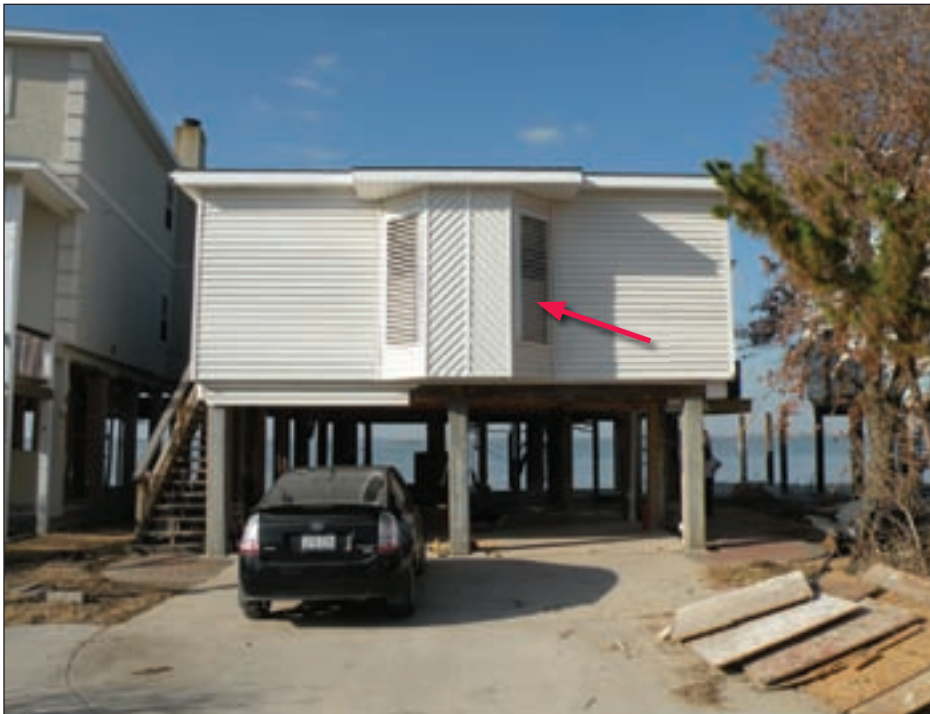
Figure 3-97. Tiki Island, TX, house with adjustable shutters (Hurricane Ike estimated wind speed in this area: 103 mph, Exposure C)
