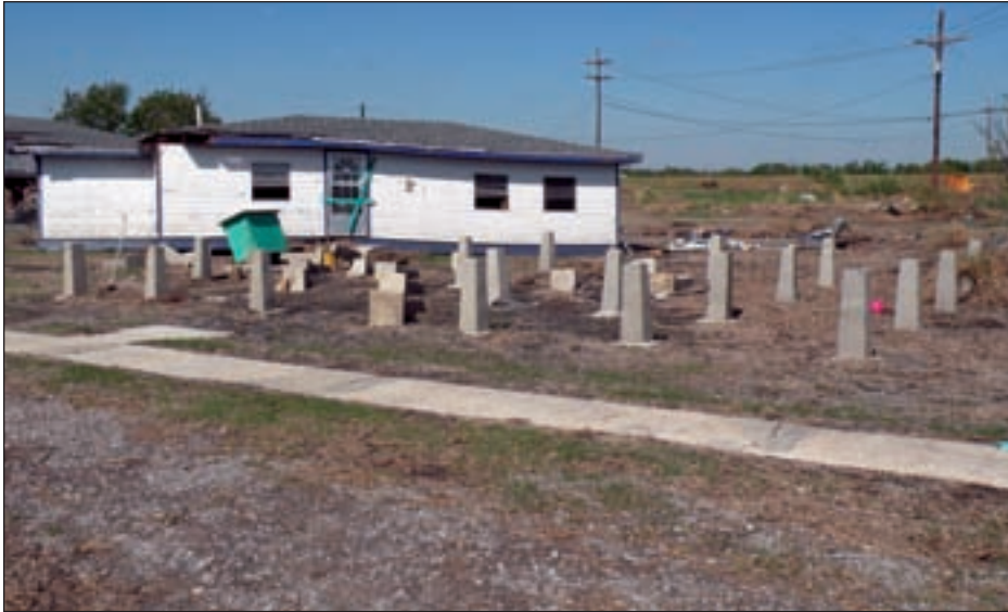
Figure 3-12. This house floated off its foundation due to insufficient elevation and inadequate connections between the foundation and the house (Golden Meadow, LA)
