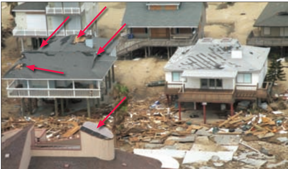
Figure 3-43. Galveston, TX, West End Beach house with roof damage in high pressure zones (Hurricane Ike estimated wind speed in this area: 95 mph, Exposure C)
