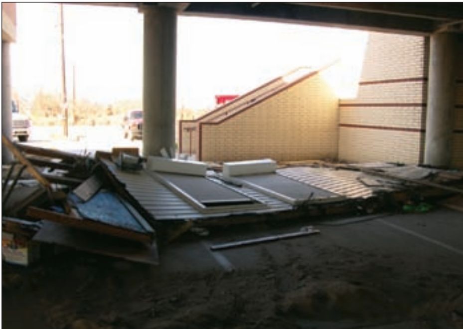
Figure 4-3. Wall of house washed underneath Crenshaw School during Ike (note shutters still attached to wall)
