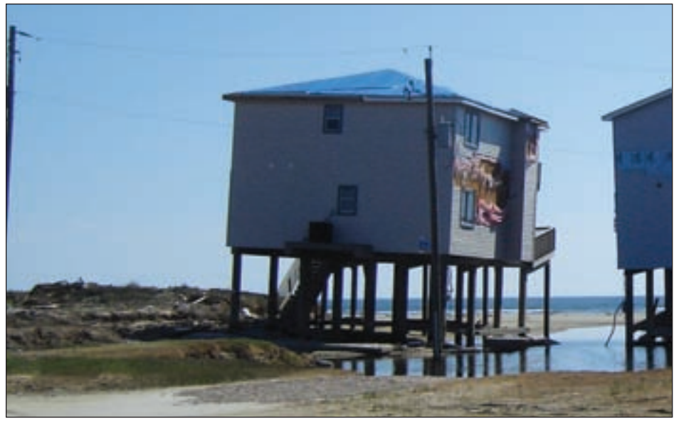
Figure 3-128. The weight of this slab, undermined due to scour and erosion, could have contributed to settlement and racking of this elevated house (Surfside Beach, TX)
