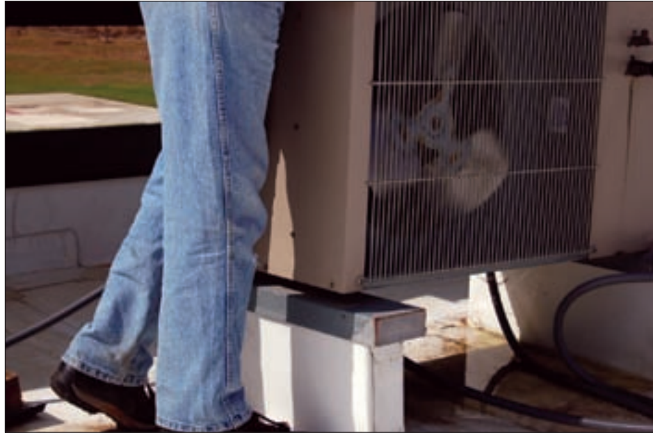
Figure 4-35. Lack of proper fastening of rooftop equipment—a MAT member was able to easily lift this condenser unit off the curb. All equipment should be fastened to resist uplift and blow-off.
