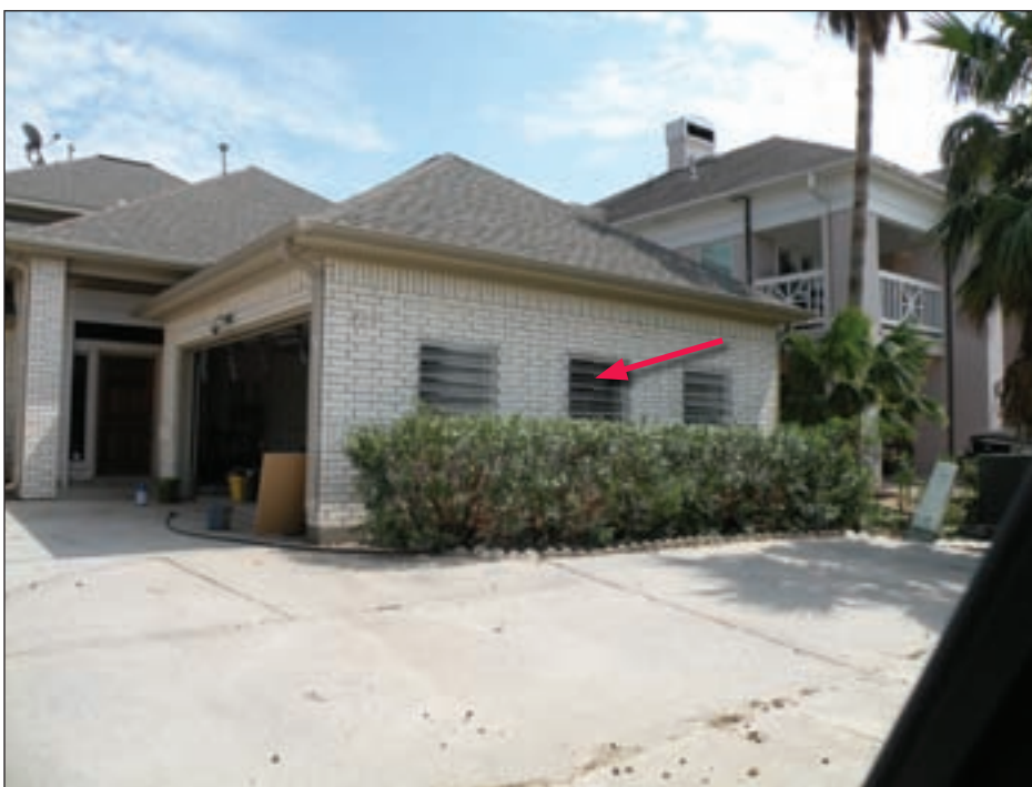
Figure 3-98. Texas City, TX, house with corrugated clear plastic shutters (Hurricane Ike estimated wind speed in this area: 88 mph, Exposure B)
