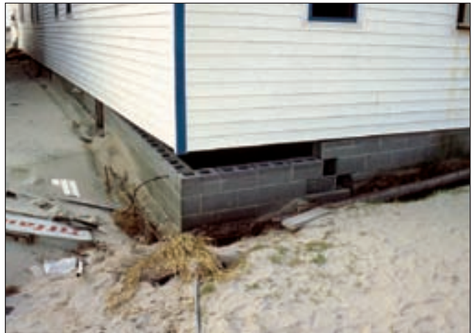
Figure 3. Failure of A-zone type foundation in coastal area, not subject to V-zone conditions (Topsail Island, NC, Hurricane Fran).
