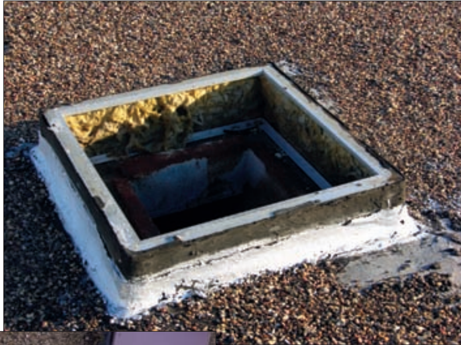
Figure 4-39. The fan shown in the inset blew off of this curb
