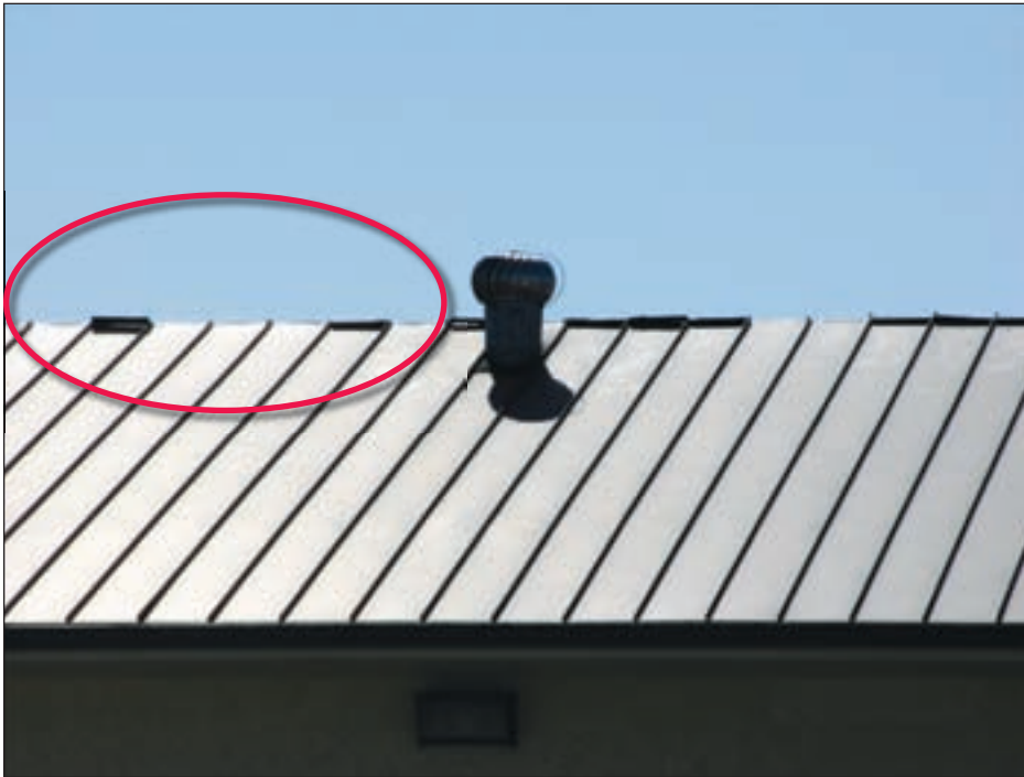
Figure 4-67. The oval shows where ridge flashing blew away
