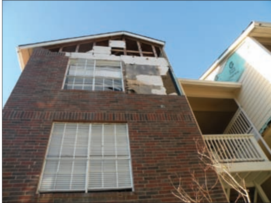
Figure 3-40. This West Bay, Galveston Island, TX, apartment experienced gable-end wind damage as a result of sheathing failure and poor connection of the brick veneer to the stud walls (Hurricane Ike estimated wind speed in this area: 90 mph, Exposure B)
