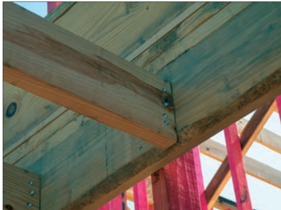
Figure 3-55. Toe-nailed connection of floor joists on band beam on house under construction. Floor joist should be installed using either galvanized metal joist hangers or ledger beams (LaPorte, TX).
