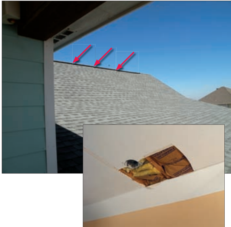
Figure 3-107. The roof ridge vent (red arrows) on this Bolivar Peninsula, TX, home leaked, and it is presumed that the water was shed down the underside of the roof decking and/or structure, thereby producing ceiling damage along the wall of this second story room (Hurricane Ike estimated wind speed in this area: 110 mph, Exposure C)
