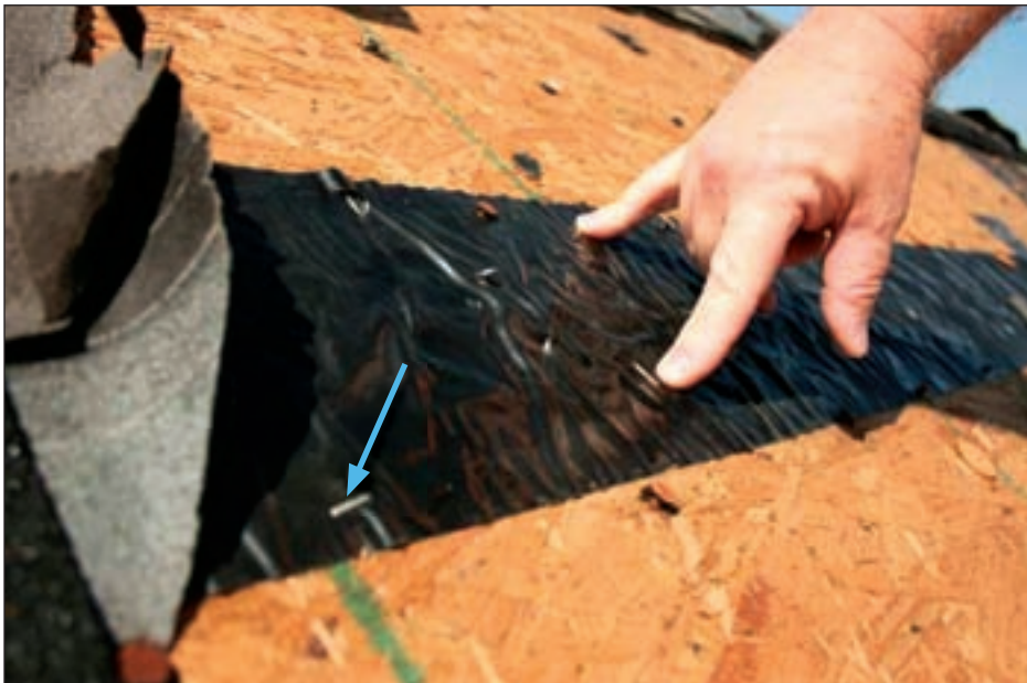
Figure 3-68. This tape did not provide a watertight seal. Note the wrinkles (which allow water migration) and the staples (blue arrow) that were used to attach the tape (Audubon Village, TX). CREDIT: IBHS
