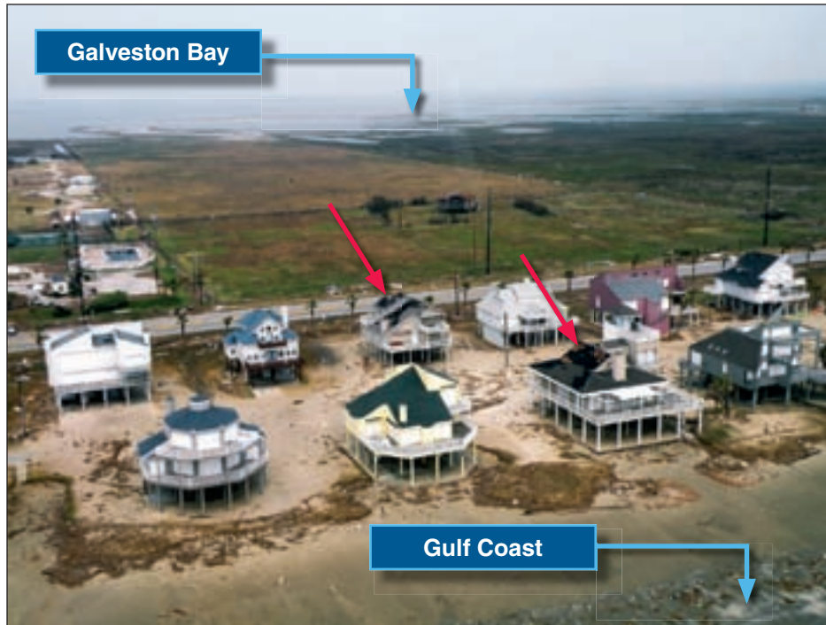
Figure 1-12. Roofing damage to north and west exposures produced by Hurricane Ike backside winds
