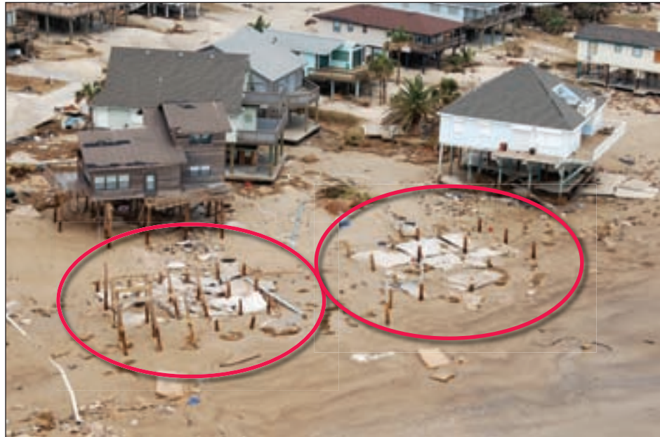
Figure 3-34. Broken piles beneath destroyed Gulf-front houses, Galveston Island, TX (west of the seawall)
