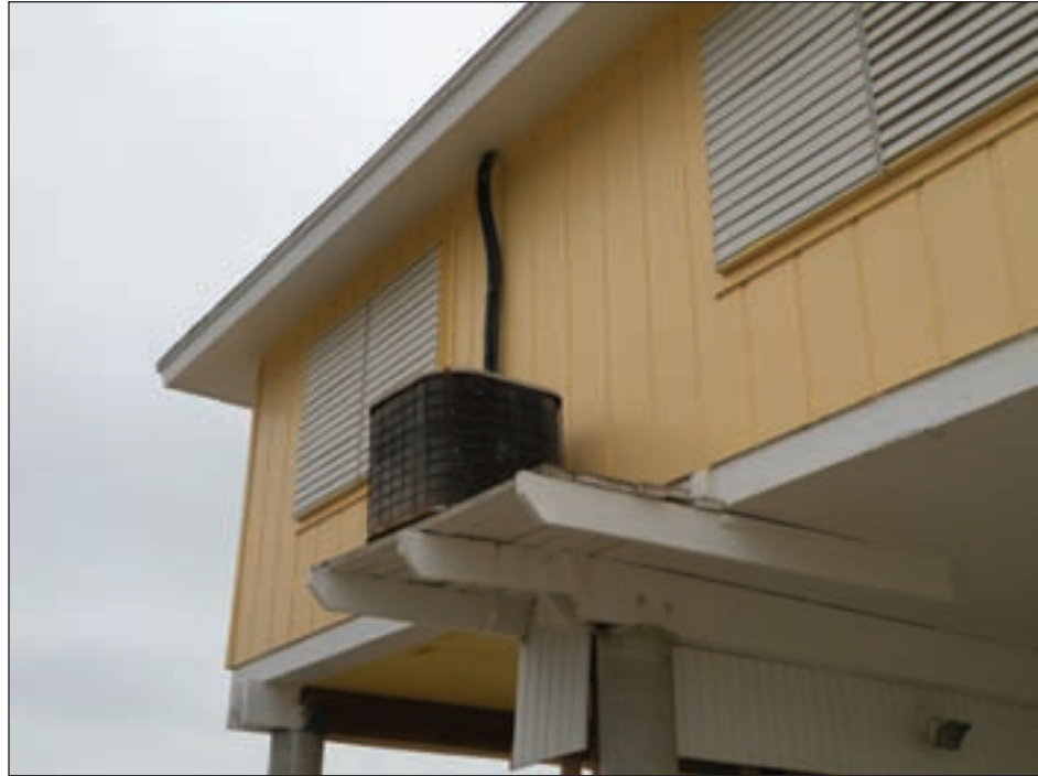
Figure 3-111. Typical cantilevered condenser (Jamaica Beach, TX; Hurricane Ike estimated wind speed in this area: 80 mph, Exposure B)
