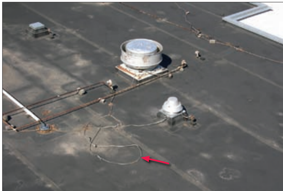
Figure 4-16. Detached LPS conductor
