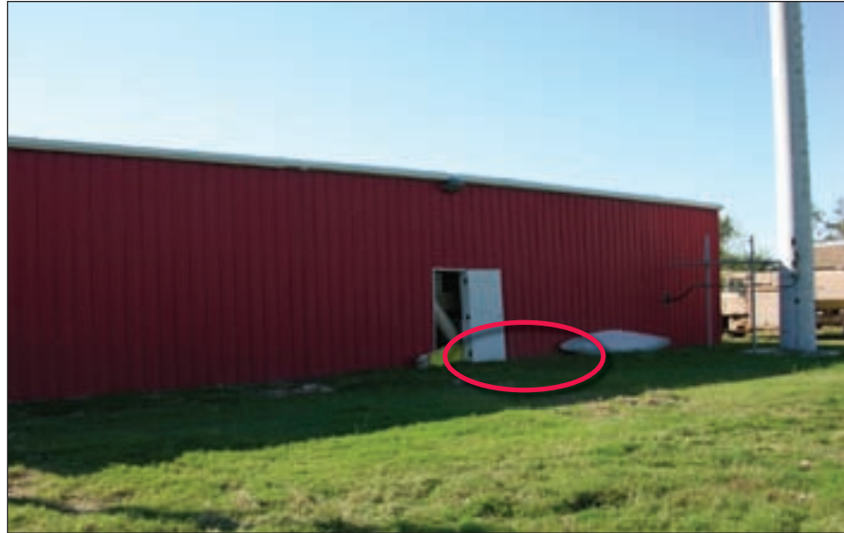
Figure 4-54. The metal wall at the red oval area was pushed outward because of inadequate attachment of the wall angle to the slab
