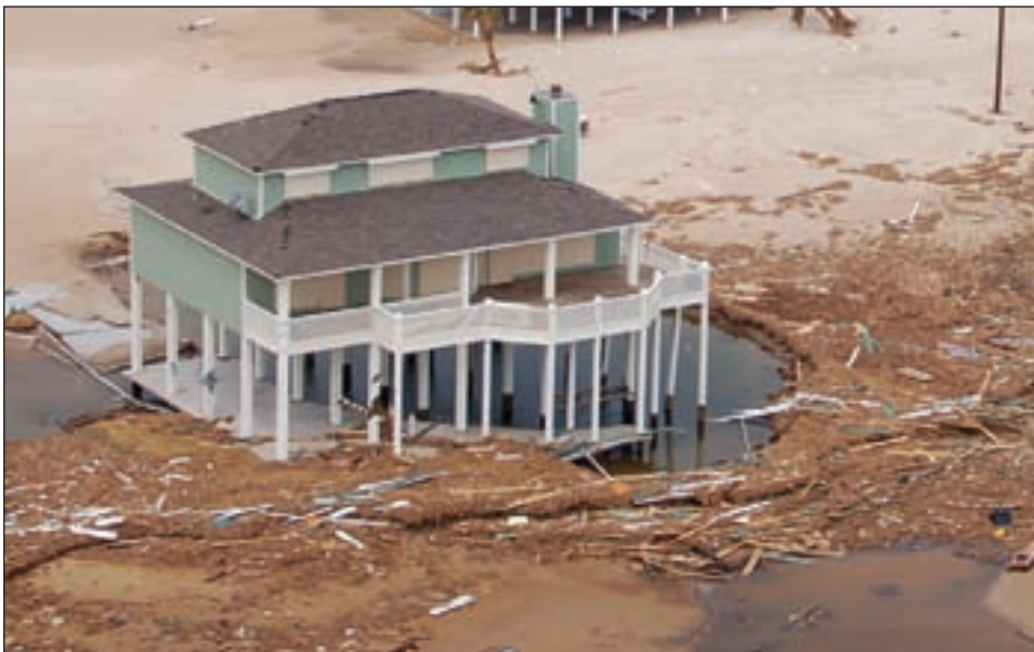
Figure 3-20. Foundation scour was reported to be 10 feet deep—note the bottoms of the piles on the right side of building that have been pushed toward the building (Bolivar Peninsula, TX; Zone V)
