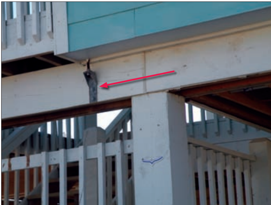
Figure 3-56. Existing house shear wall connector incorrectly located (red arrow). Connector should be located on column line or the beam and beam-to-column connection should be designed to resist the uplift load, which is carried by a nailed connection in the absence of bolts (Sunset Crystal Beach, Bolivar Island, TX).
