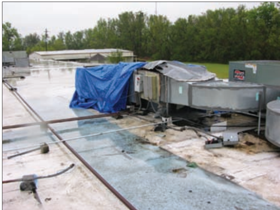
Figure 4-20. Water entered the building where ductwork blew away
