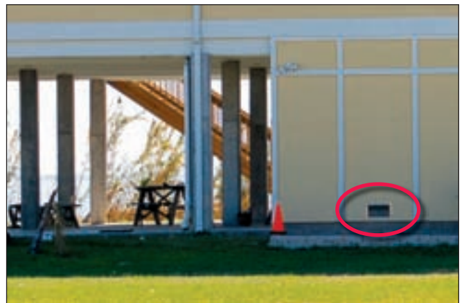
Figure 5. Flood opening in a below-BFE enclosure wall.
