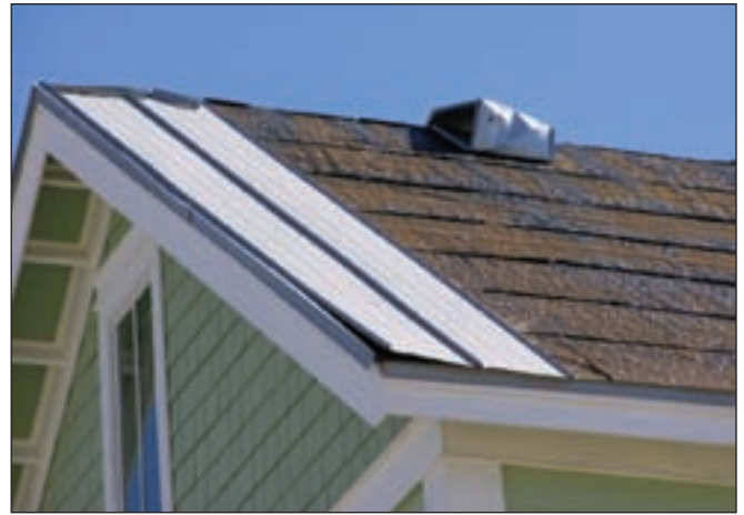
Figure 3. These architectural panel system have snap-lock seams. One side of the seam is attached with a concealed fastener. Although a large number of panels blew away, the underlayment did not.
