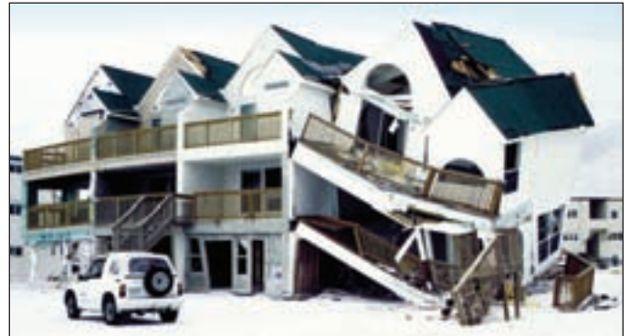
Figure 1. Failure of wood-frame walls used to support a coastal building, which was subjected to shallow flooding, small waves, and floating debris (Fort Walton Beach, FL, Hurricane Opal).
