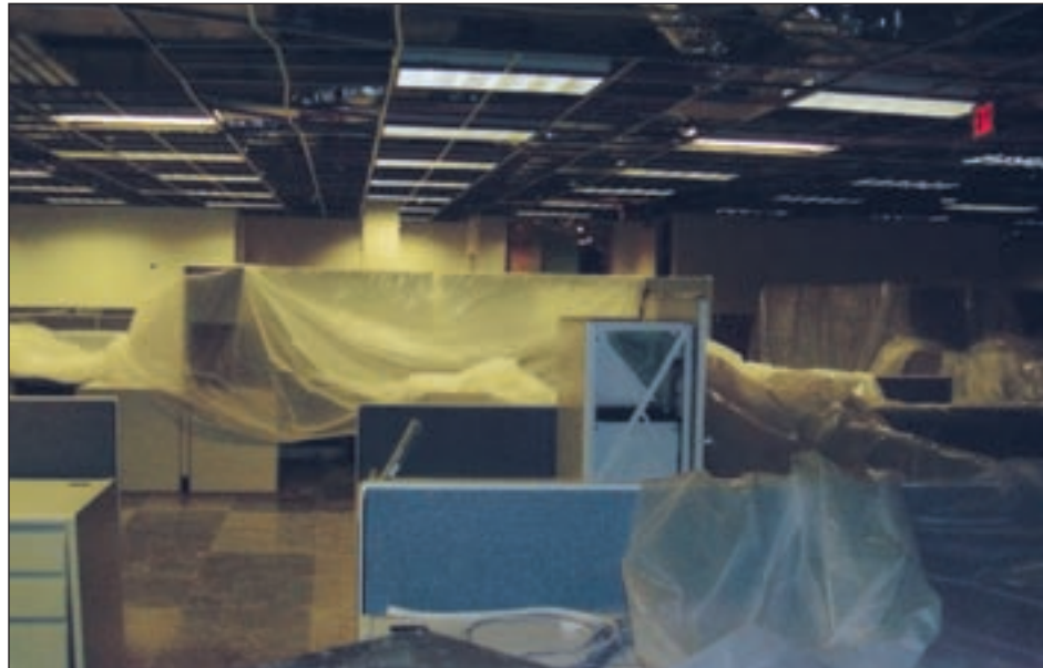
Figure 5-9. View of repairs to an office damaged in the JP Morgan Chase Center
