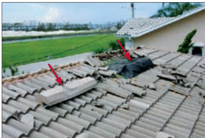
Figure 11. Two off-ridge vents are shown in this photograph. The vent that is covered with roofing felt flipped up and allowed a substantial amount of water to enter the residence. Carpeting, kitchen cabinets, and a large amount of gypsum board had to be replaced because of the water intrusion.
