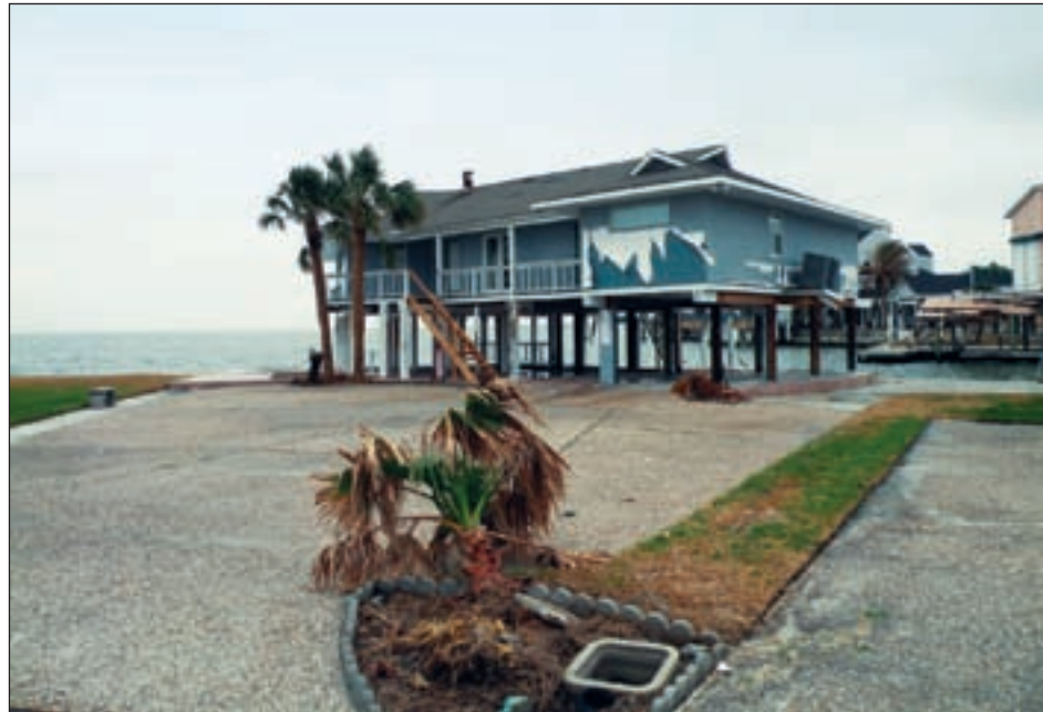
Figure 2-8. Jamaica Beach house on the West Bay with “backside” wind damage (number 2480 in 1990 Galveston study)
