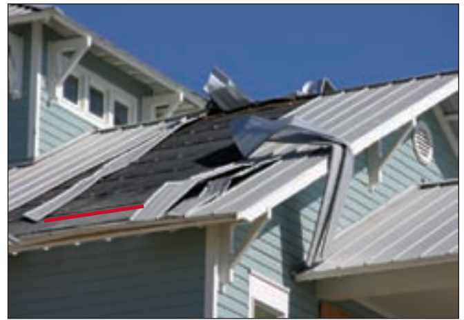
Figure 1. This architectural panel system has concealed clips. The panels unlatched from the clips. The first row of clips (just above the red line) was several inches from the end of the panels. The first row of clips should have been closer to the eave.
