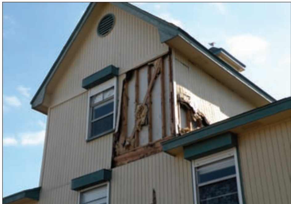
Figure 3-94. Decayed plywood siding removed by wind pressures (Tiki Island, TX; Hurricane Ike estimated wind speed in this area: 103 mph, Exposure C)
