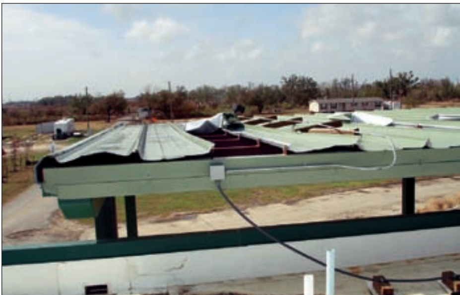
Figure 4-34. Damage to canopy over emergency room entrance driveway
