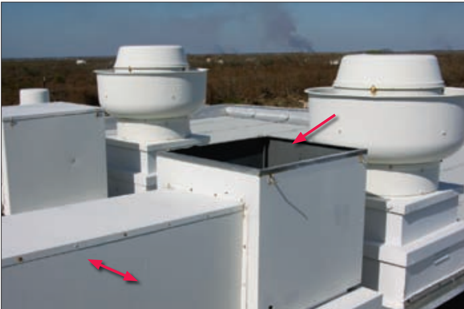
Figure 4-6. Missing access panel allowed rain intrusion; ductwork could be easily flexed
