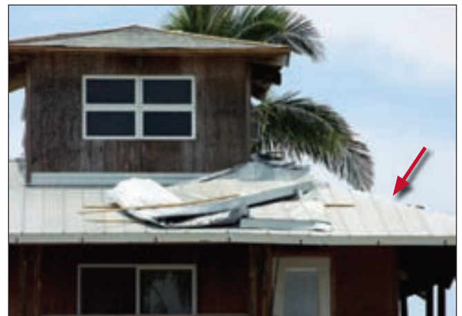
Figure 5. The panels blew off the upper roof and landed on the lower roof of this house. The upper asphalt shingle roof shown had been re-covered with 5V-Crimp panels that were screwed to nailers. The failure was caused by inadequate attachment of the nailers (which had widely-spaced nails) to the sheathing. Note that the hip flashing on the lower roof blew off.
