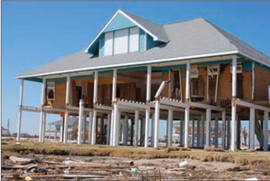
Figure 3-32. Seaward side of Zone V house struck by waves. The deck, the elevated floor system, and the seaward walls were destroyed or heavily damaged (Bolivar Peninsula, TX).
