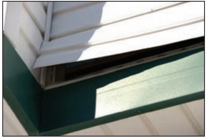
Figure 4. Utility trim was substituted for the starter strip and the bottom lock was cut off the siding. Siding was able to pull loose under wind pressure.
