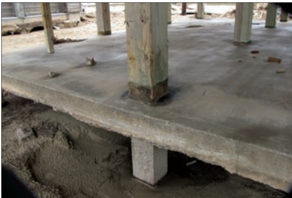
Figure 3-124. Undermining of concrete slab that settled but remained intact (Galveston Island, TX)
