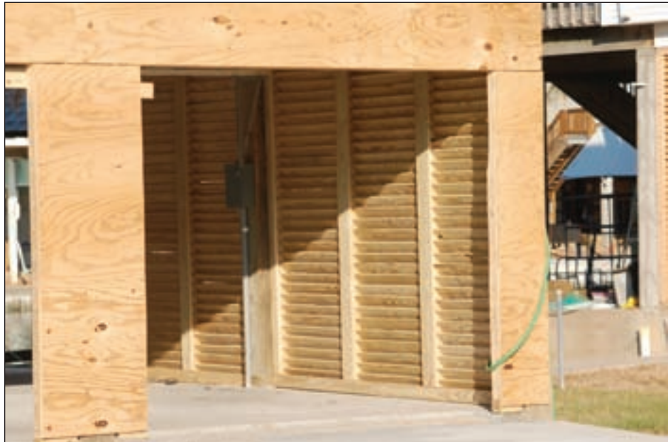
Figure 3-118. Solid breakaway walls lost during Ike are being replaced with louvered panels (Tiki Island, TX)
