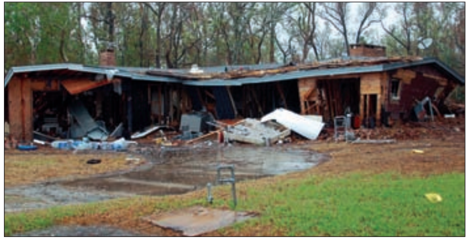
Figure 3-11. This house sustained significant structural damage due to storm surge and small waves above the 9-foot BFE in Zone A (Bridge City, TX). Note flood debris line on the roof.
