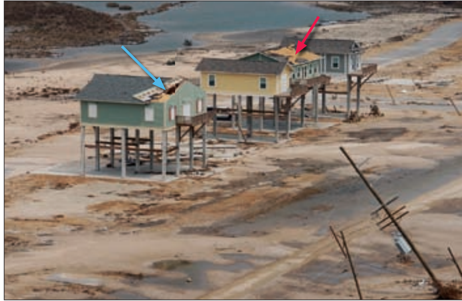
Figure 3-66. Roof covering and roof structure damage at Fortified...for safer living ® houses in the Audubon Village area on Bolivar Peninsula, TX (Hurricane Ike estimated wind speed in this area: 110 mph)
