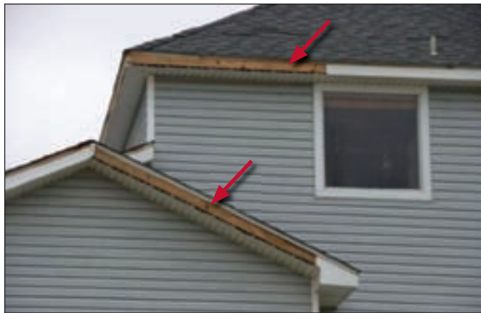
Figure 7. Loss of fascia cover exposes ends of vinyl soffit to direct entry of wind-driven rain.
