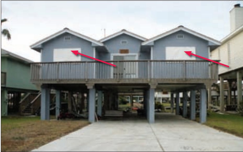
Figure 3-101. Snapped-on vinyl canvas window covers (red arrows) in West Bay, Galveston Island, TX (Hurricane Ike estimated wind speed in this area: 90 mph, Exposure B)
