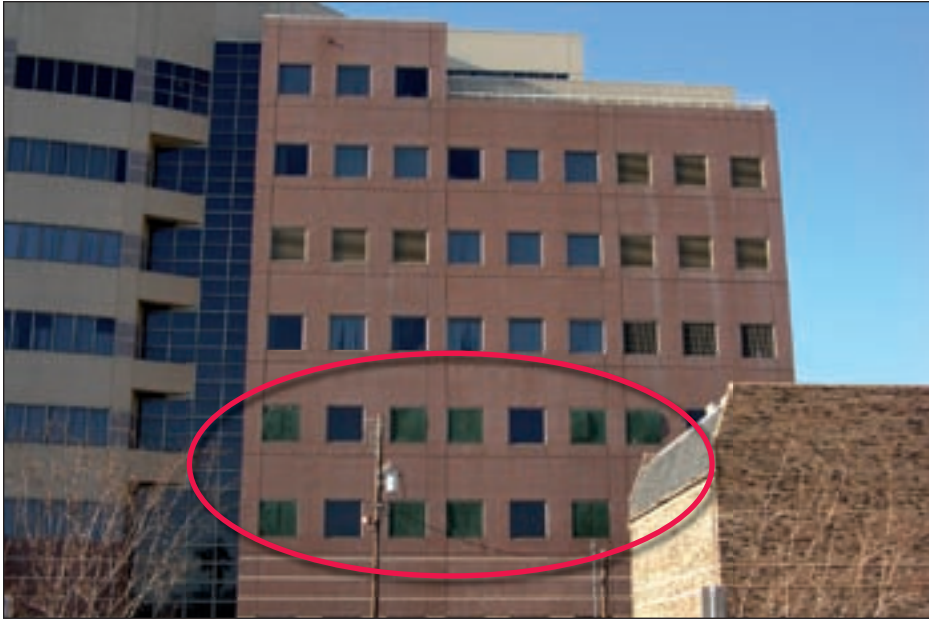
Figure 4-31. Nine broken windows are shown in the red oval; the brown openings above the oval are louvers
