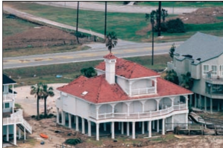
Figure 3-72. This tile roof on Galveston Island, TX, experienced hip, eave, and field damage (Hurricane Ike estimated wind speed in this area: 106 mph)
