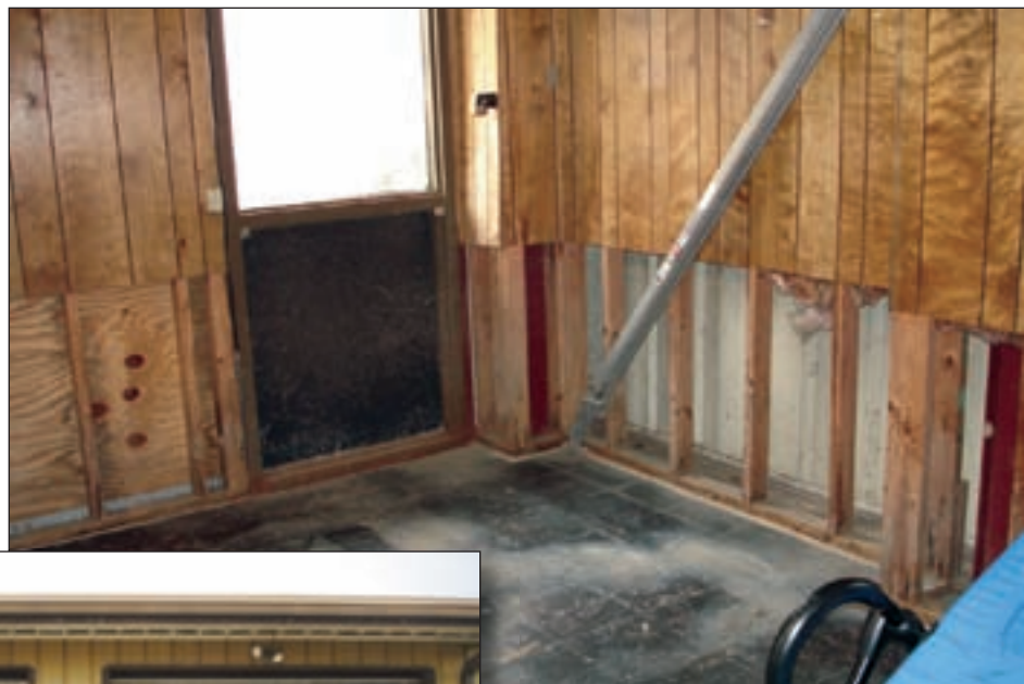
Figure 4-57. 7th Ward Fire District No.1 Fire Station; wall repairs were in progress during MAT inspection
