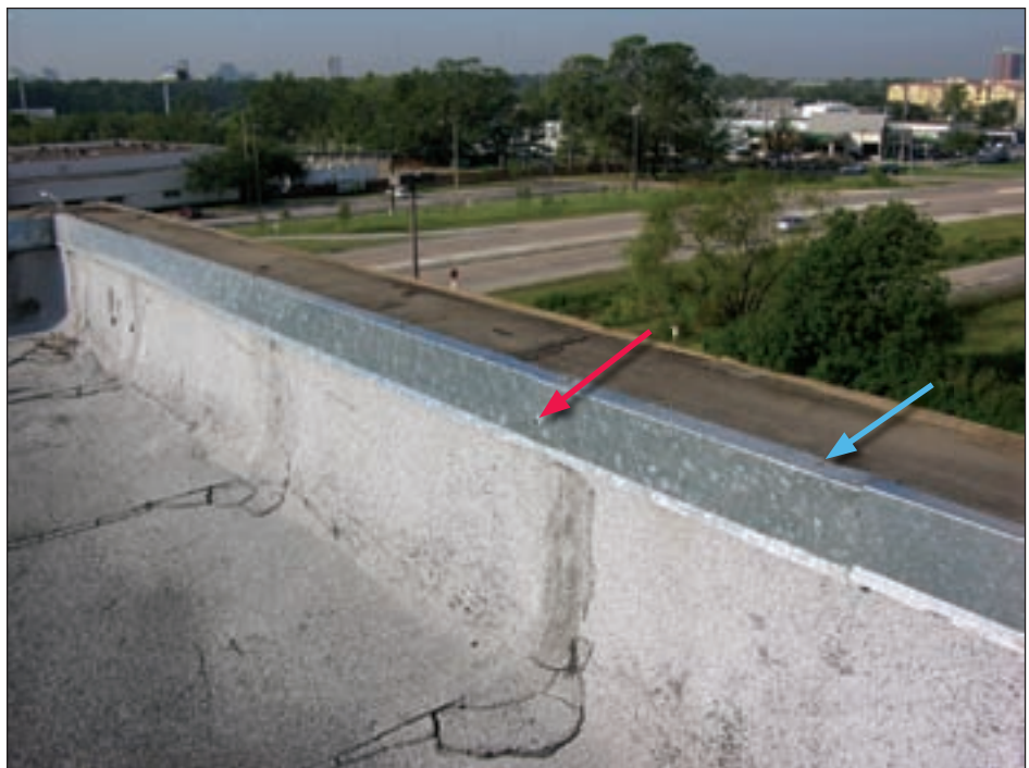
Figure 4-42. The coping blew off because of inadequate attachment of the cleats. The blue arrow shows roofing nails driven through the horizontal flange and the red arrow shows widely spaced nails through the vertical flange.
