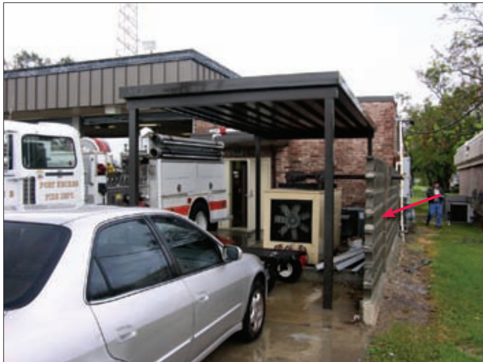
Figure 4-52. The emergency generator is susceptible to windborne debris and damage caused by collapse of the masonry screen wall
