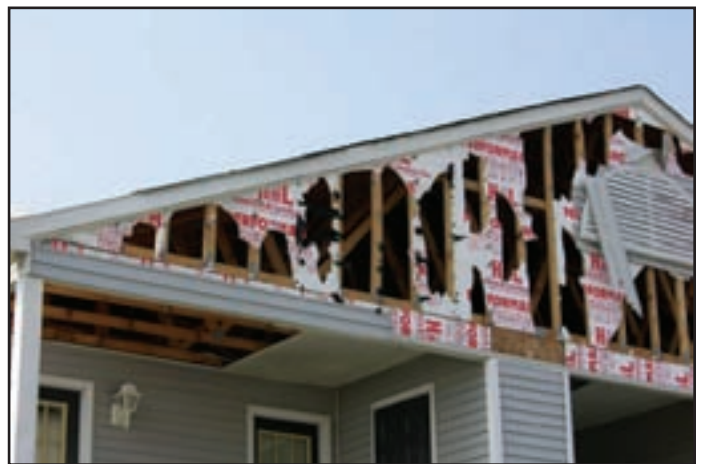
Figure 7. The vinyl siding at this gable was installed over plastic foam insulation. Without wood sheathing, the wind pressures on the vinyl are increased. Also, if the siding blows away, the foam insulation is very vulnerable to blow-off. With loss of the foam insulation, wind-driven rain can freely enter the attic, saturate the ceiling insulation, and cause collapse of the ceiling.
