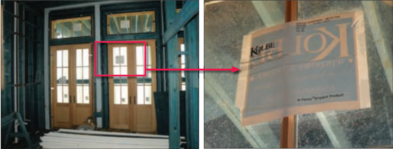
Figure 3-95. Impact-resistant door and window glazing in new East Galveston, TX, house. Inset shows manufacturer's label indicating glazing is impact resistant.
