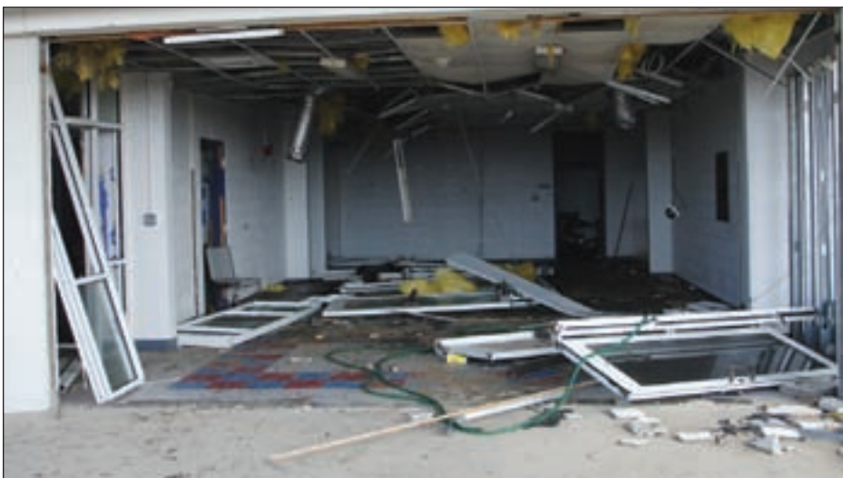
Figure 4-9. Johnson's Bayou School interior building damage
