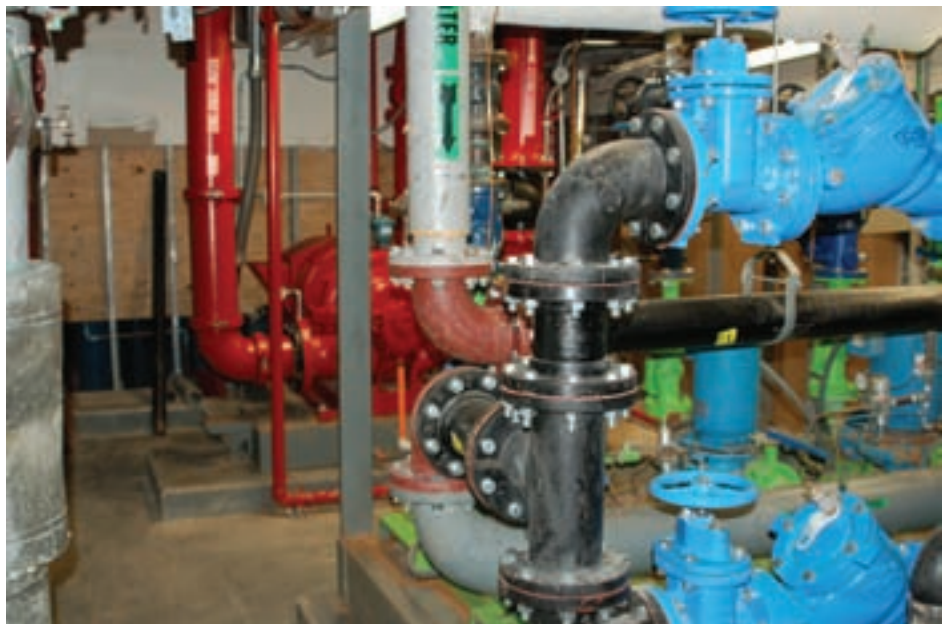
Figure 4-25. The Ike flood level in UTMB Building 56 pump room was approximately 30 inches above the floor, and controls and equipment were damaged.
