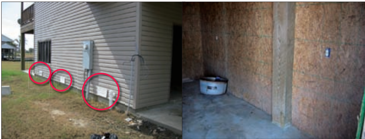
Figure 3-132. Flood vent openings (red circles) that do not extend through the walls (Hackberry, Cameron Parish, LA)
