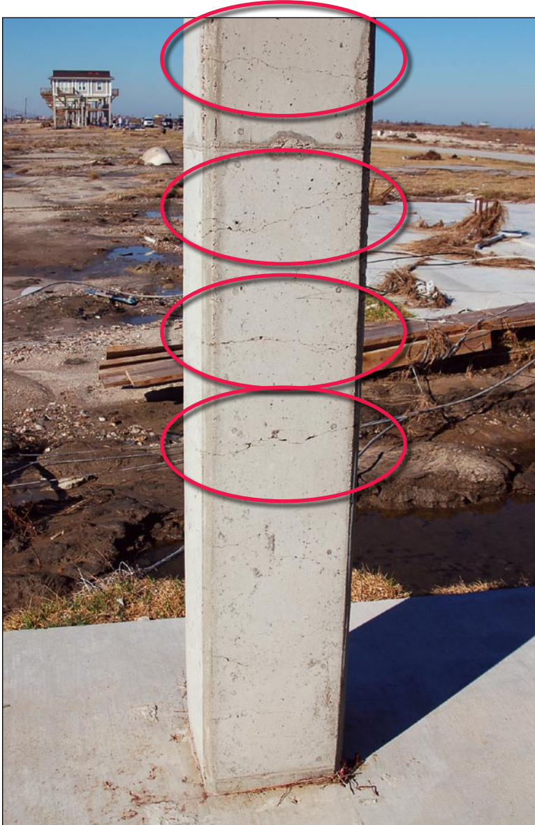
Figure 3-15. Concrete column showing cracking that was likely caused by extreme column bending stresses due to lateral loads on the elevated house and foundation (Bolivar Peninsula, TX)
