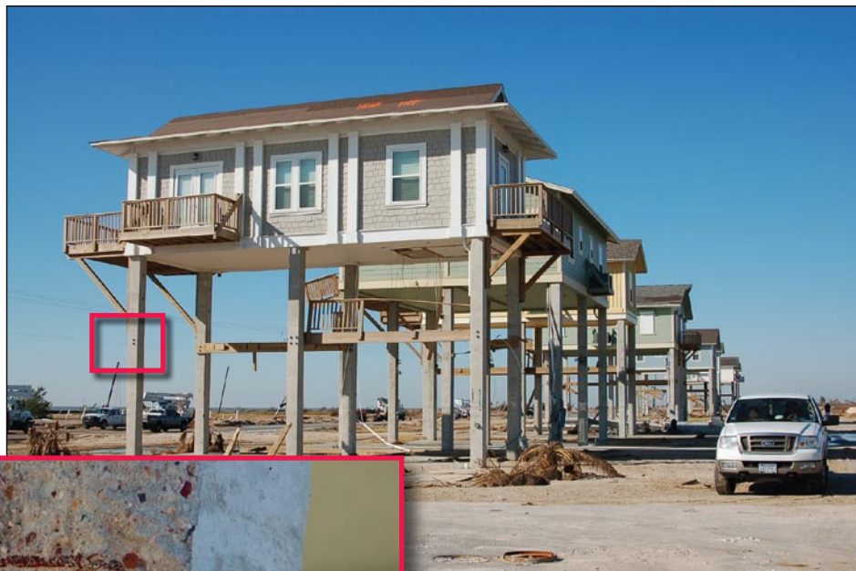
Figure 3-14. Ground-level view of elevated houses with inset showing typical column damage where the timber deck broke away (Bolivar Peninsula, TX).
