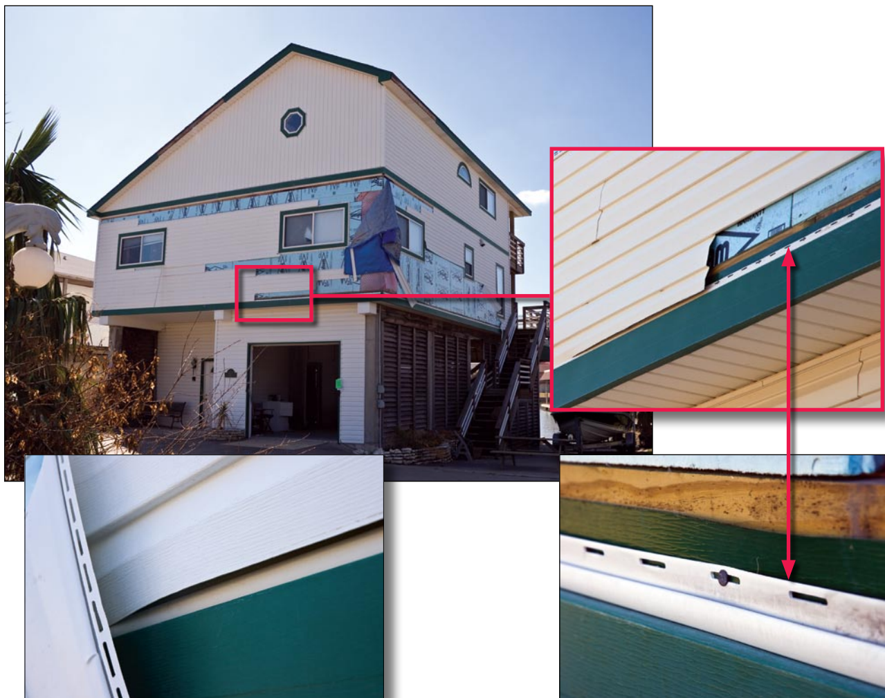
Figure 3-81. Improper installation led to extensive loss of siding up the house wall. The bottom lock of the lowest course of siding was cut off, and utility trim substituted for the correct starter strip. The poorly retained bottom edge pulled out under wind pressure, leading to extensive loss of siding up the house wall (Tiki Island, TX; Hurricane Ike estimated wind speed in this area: 88 mph, Exposure B).
