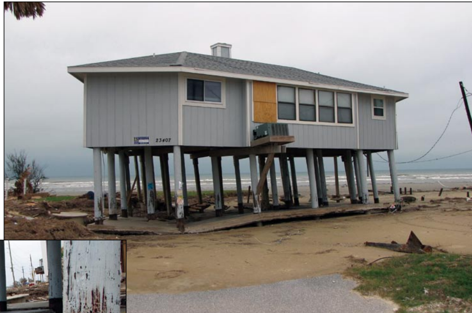
Figure 3-21. Failure of a timber pile foundation undermined by scour and erosion. Inset shows close-up of concrete slab failure and rotation of some of the foundation piles (Galveston Island, TX; Zone V).
