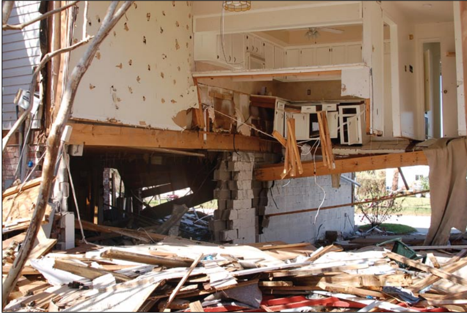
Figure 3-36. Likely wave and debris damage to townhouse building along the western Galveston Bay in Seabrook, TX. The building was supported on shore-parallel masonry walls, and is landward of another building that was destroyed by Ike.
