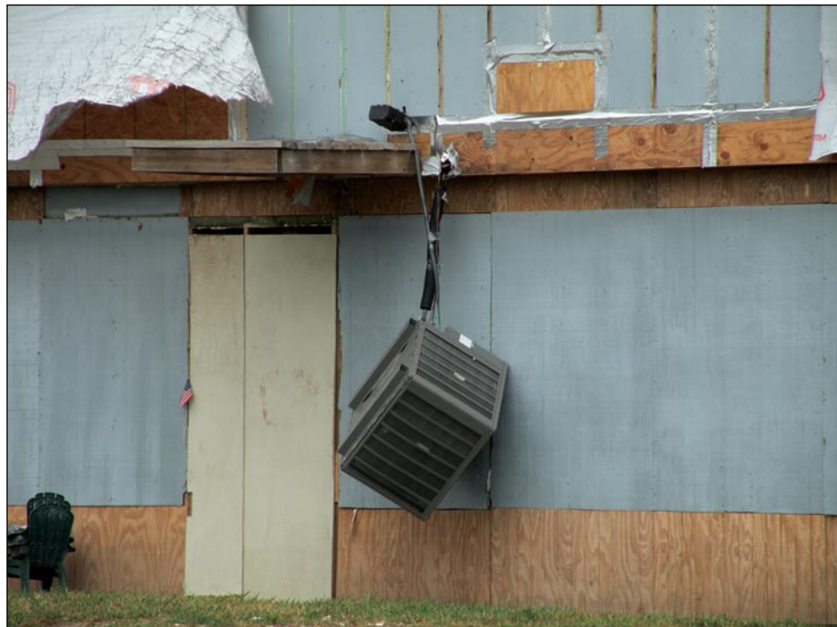
Figure 3-112. Improperly secured condensing unit was knocked from its platform (Kahala Beach, TX; Hurricane Ike estimated wind speed in this area: 80 mph, Exposure B)
