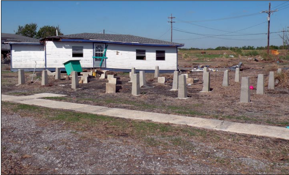
Figure 3-12. This house floated off its foundation due to insufficient elevation and inadequate connections between the foundation and the house (Golden Meadow, LA)
