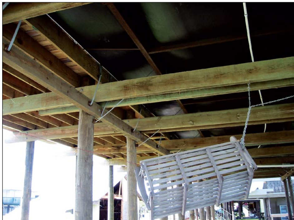
Figure 3-138. The framing and anchoring system of the house shown in Figure 3-137. Strapping secured the home's walls and frames to its foundation. While the strapping held the home to its foundation during Ike, it could not be determined if the strapping would resist a design wind event (Estimated wind speed during Ike: less than 60 mph, 3-second gust).
