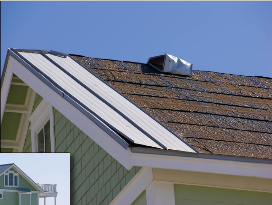
Figure 3-69. These snap-lock seam panels were attached with fasteners through one side of the seam (Galveston Island, TX; Hurricane Ike estimated wind speed in this area: 110 mph)
