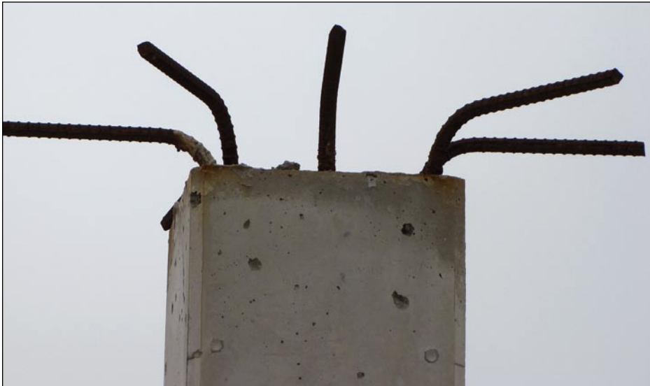
Figure 3-26. Reinforcing steel extending from the top of a concrete column (building under construction) (Galveston Island, TX)
