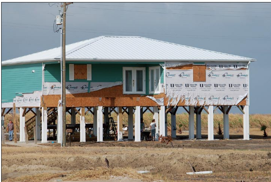
Figure 3-74. Loss of siding at Holly Beach, LA, home (Cameron Parish; Hurricane Ike estimated wind speed in this area 80 mph, Exposure C)
