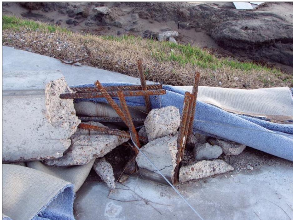
Figure 3-4. This concrete column failed due to lateral loads. Note limited overlap of reinforcing steel at the bottom of the column.
