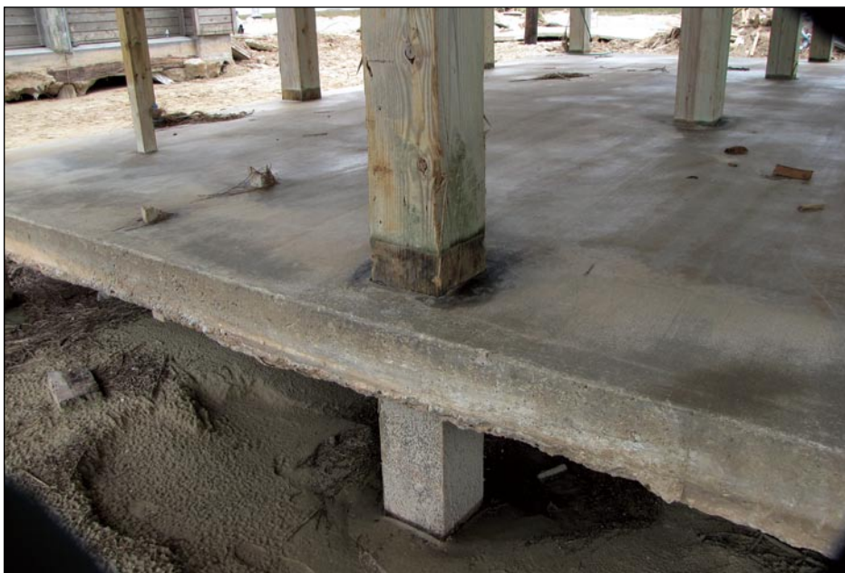
Figure 3-124. Undermining of concrete slab that settled but remained intact (Galveston Island, TX)
