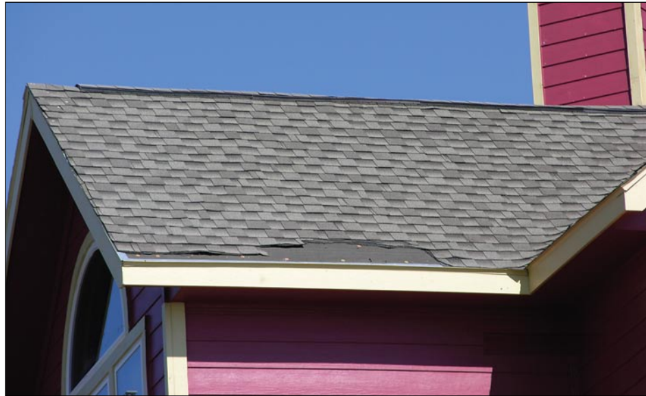
Figure 3-63. Loss of shingles along the eave in Bolivar Peninsula, TX (Hurricane Ike estimated wind speed in this area: 110 mph)
