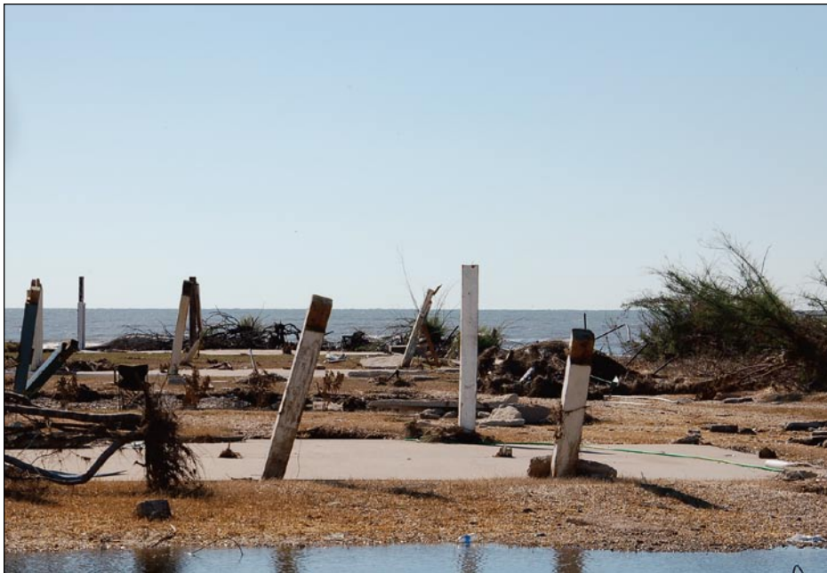
Figure 3-2. A house on timber piles was pushed over by wind and flood loads and the load path failed at the connection between the floor beam and the piles. Embedment and elevation were also insufficient at this Bolivar Peninsula, TX, site.
