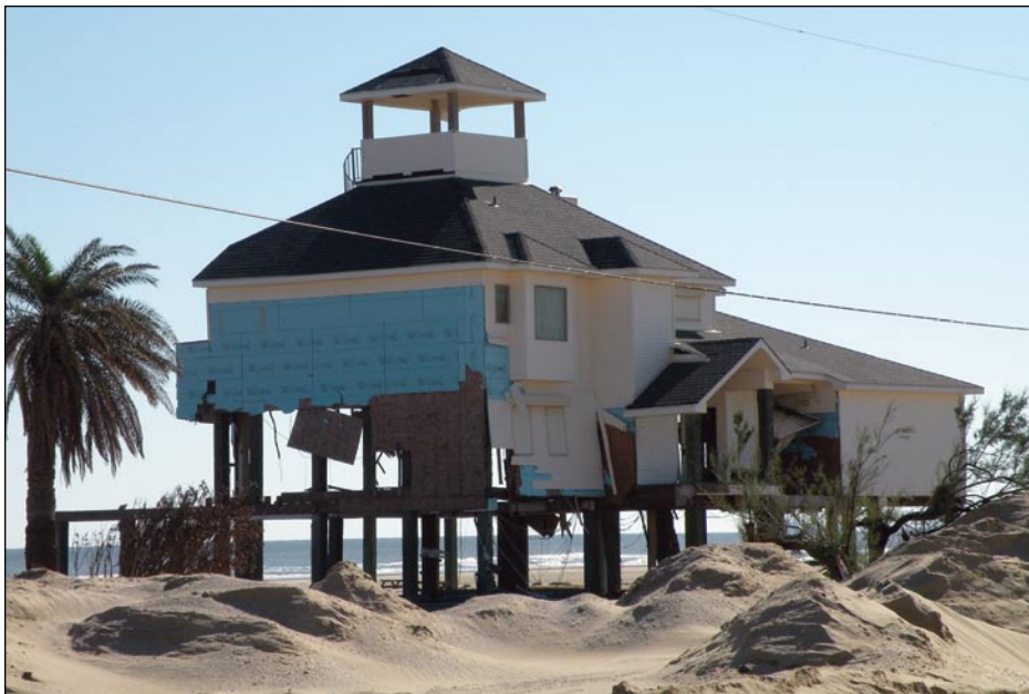
Figure 3-48. Though much of the cladding and structural sheathing was destroyed by Ike's surge, the MWFRS of this Bolivar Peninsula, TX, beach house remained intact and connected
