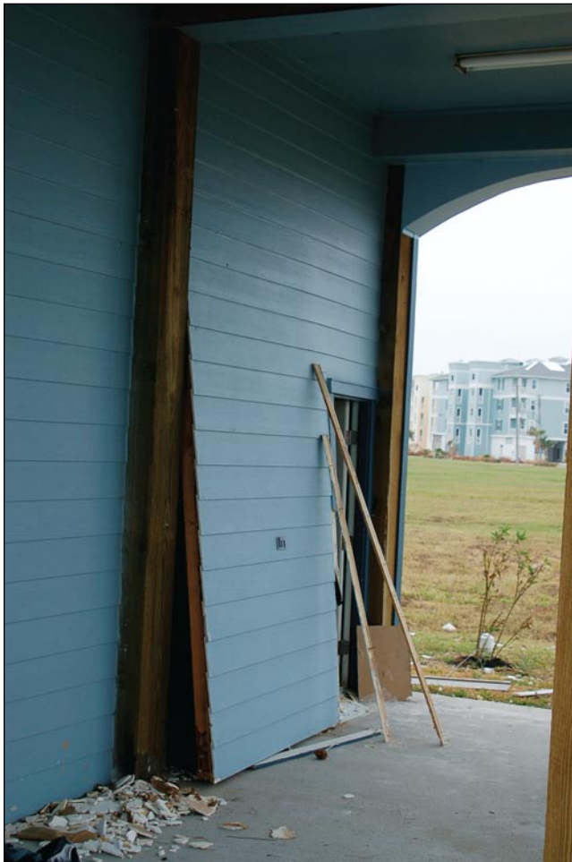
Figure 3-116. This 11-foot high breakaway wall panel was pushed out by floodwaters trapped inside the enclosure (Galveston Island, TX)
