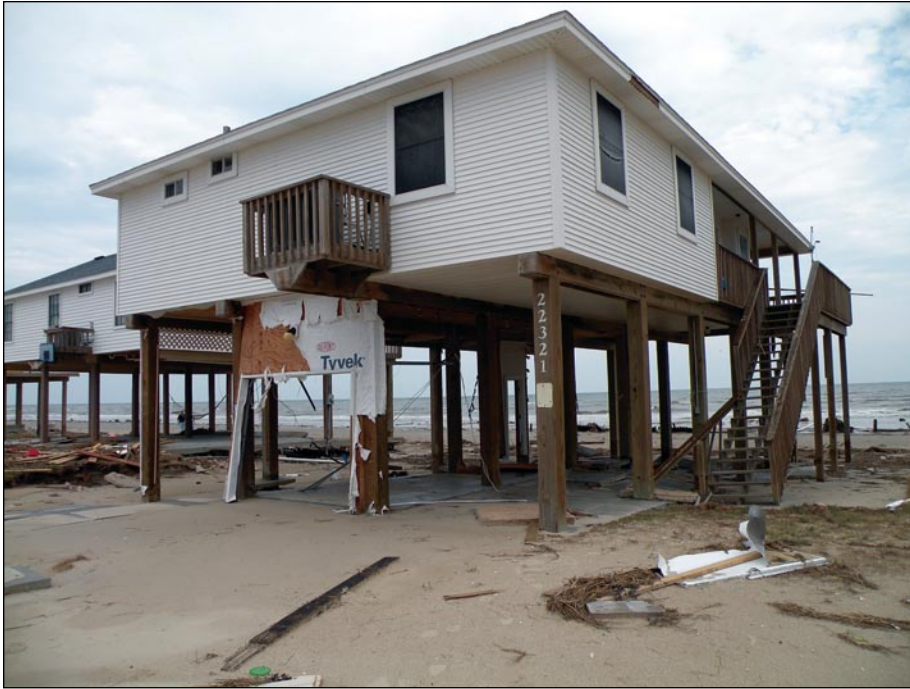
Figure 3-113. Elevated condenser is tightly enclosed, making service access difficult (Bermuda Beach, TX; Hurricane Ike estimated wind speed in this area: 95 mph, Exposure C)
