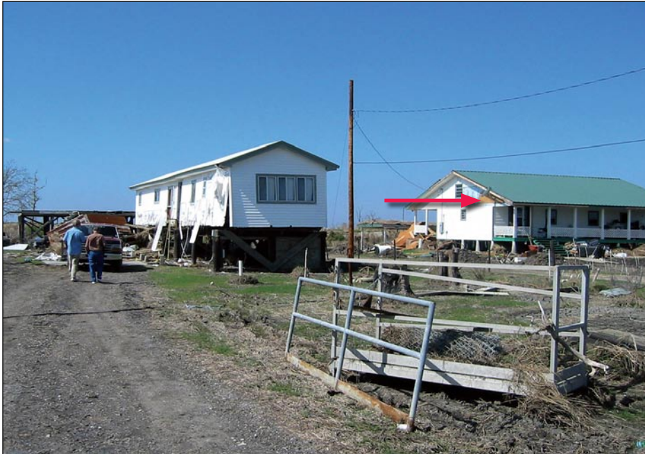
Figure 3-139. Zone A manufactured home in the Golden Meadows section of Lafourche Parish, LA, sustained 3 to 4 feet of flooding above the floor, but did not shift or float off of its foundation. The red arrow indicates the flood level reported by neighbors.
