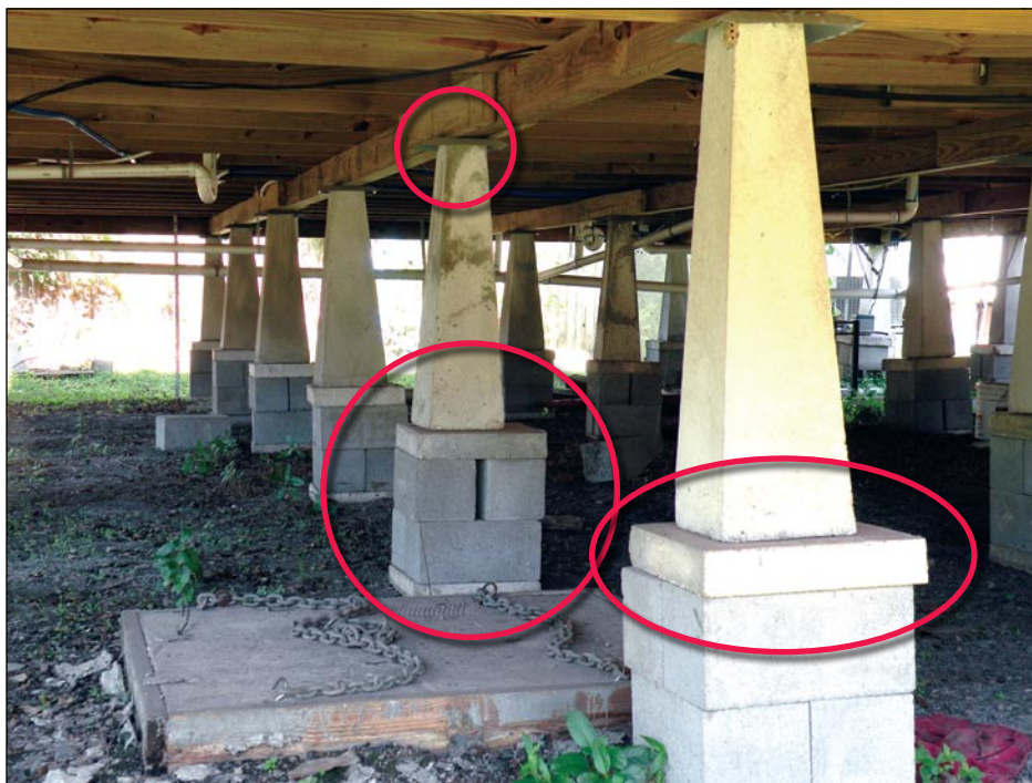
Figure 3-29. House resting (i.e., with no structural connection) on top of precast concrete piers, stacked CMUs, and shallow footing pads (New Iberia, LA)
