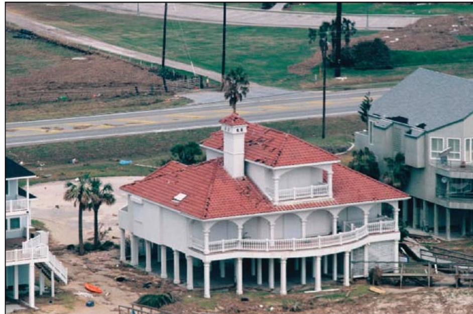
Figure 3-72. This tile roof on Galveston Island, TX, experienced hip, eave, and field damage (Hurricane Ike estimated wind speed in this area: 106 mph)
