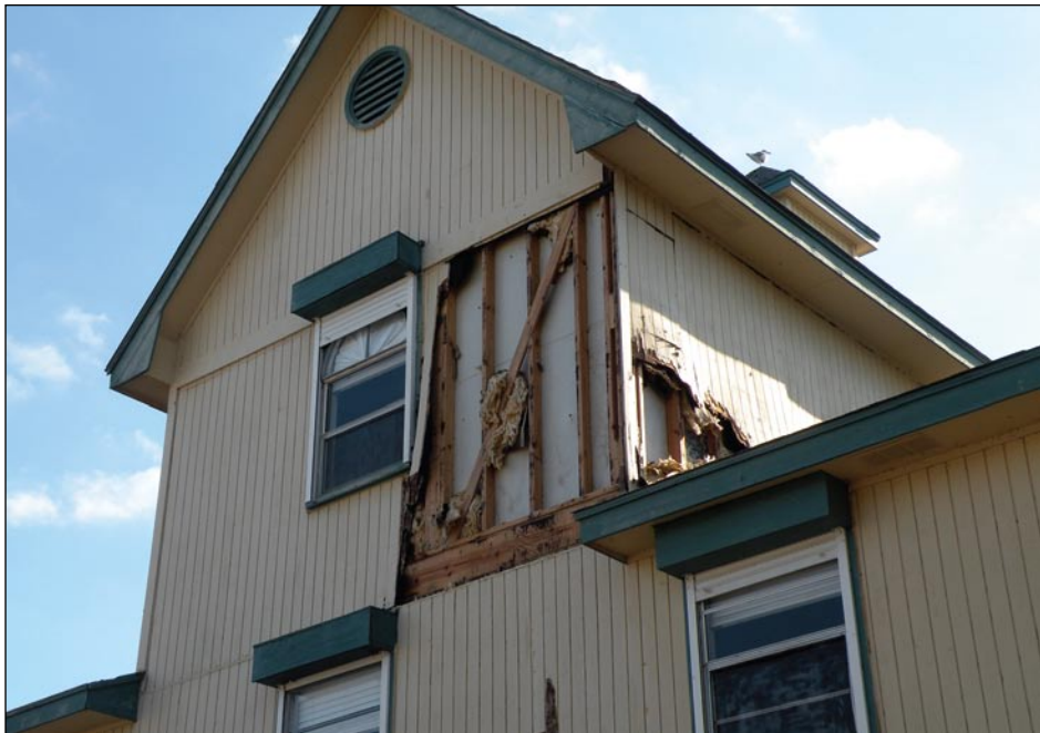
Figure 3-94. Decayed plywood siding removed by wind pressures (Tiki Island, TX; Hurricane Ike estimated wind speed in this area: 103 mph, Exposure C)
