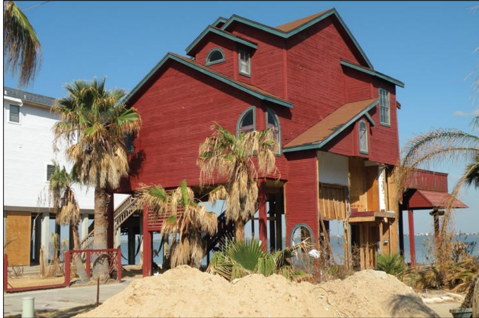
Figure 3-93. Clapboard-sided house with siding that performed well; damage resulted from failure of a non-breakaway wall (Tiki Island, TX; Hurricane Ike estimated wind speed in this area: 103 mph, Exposure C).
