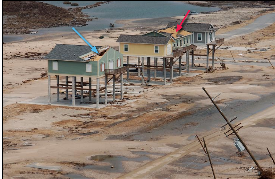
Figure 3-66. Roof covering and roof structure damage at Fortified... for safer living ® houses in the Audubon Village area on Bolivar Peninsula, TX (Hurricane Ike estimated wind speed in this area: 110 mph)
