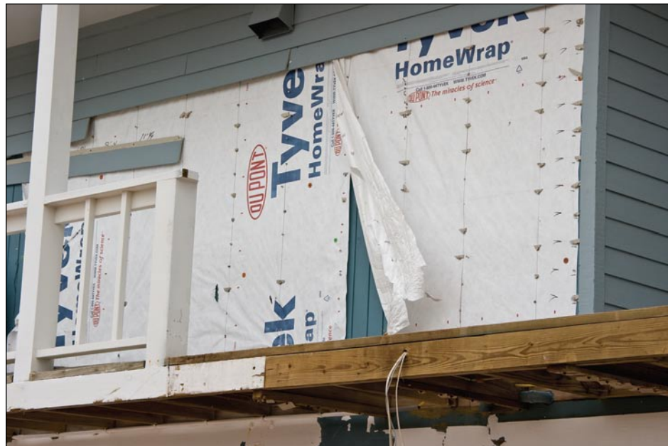
Figure 3-87. Fiber cement plank siding, installed as a reside over the original plywood siding, was torn from this West Bay, Galveston Island, TX, house (Hurricane Ike estimated wind speed in this area: 100 mph, Exposure C)
