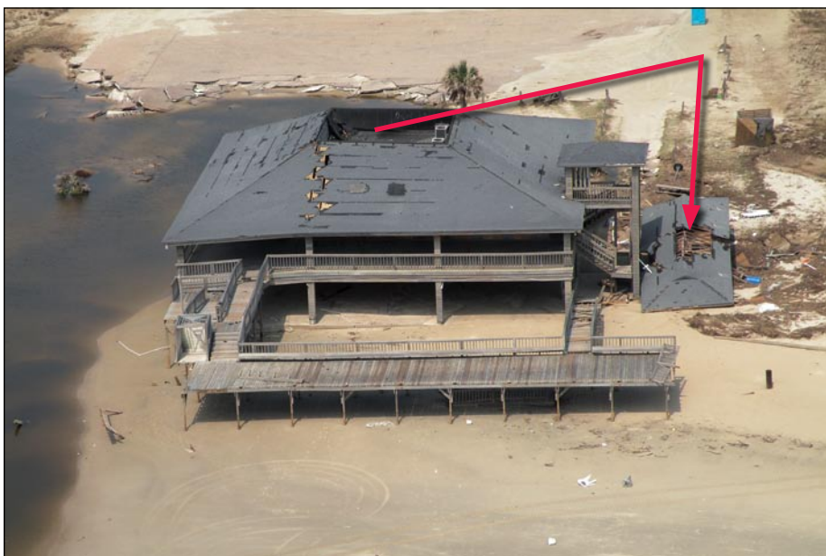
Figure 3-39. Galveston, TX, West End Beach house with roof structure removed by Hurricane Ike. The cause of the failure is unknown, but Ike wind speeds in this area were below design speeds (Hurricane Ike estimated wind speed in this area: 93 mph, Exposure C).
