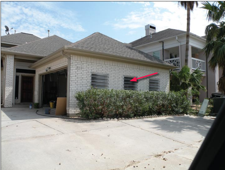
Figure 3-98. Texas City, TX, house with corrugated clear plastic shutters (Hurricane Ike estimated wind speed in this area: 88 mph, Exposure B)
