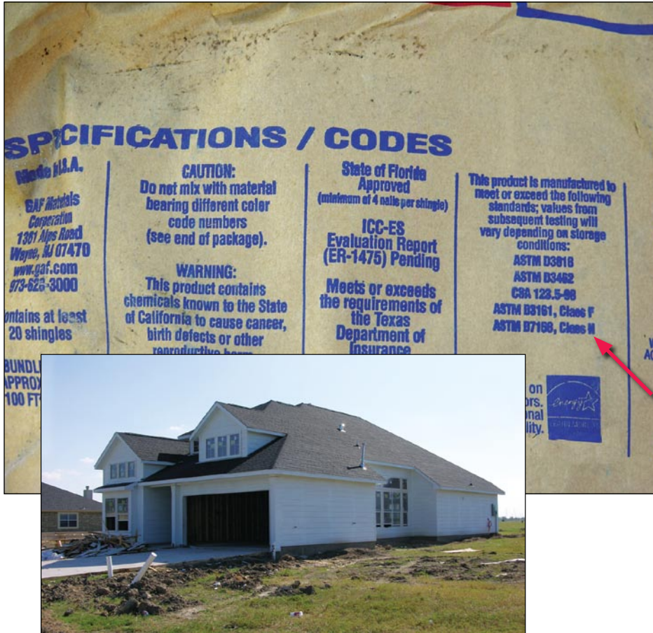
Figure 3-61. View of a shingle bundle wrapper at the Webster, TX, house shown in the inset. This shingle has a Class H rating (red arrow) (Hurricane Ike estimated wind speed in this area: 104 mph).
