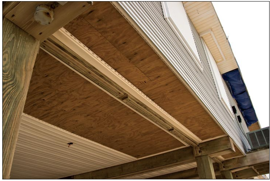
Figure 3-122. Vinyl soffit covering over plywood sheathing partially removed (Tiki Island, West Galveston Bay; Estimated Hurricane Ike wind speed: 103 mph, Exposure C)
