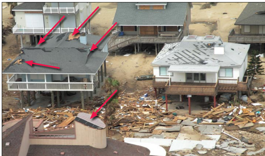
Figure 3-43. Galveston, TX, West End Beach house with roof damage in high pressure zones (Hurricane Ike estimated wind speed in this area: 95 mph, Exposure C)
