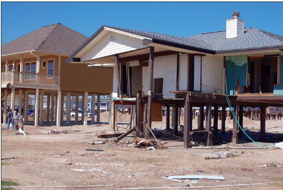
Figure 3-6. Unlike the older and lower house on the right, the Zone V house on the left was elevated approximately 5 feet above the 16-foot National Geodetic Vertical Datum (NGVD) BFE and sustained no structural damage due to flooding (Crystal Beach, TX)
