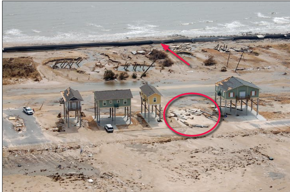
Figure 3-13. Looking toward the Gulf, past Zone V houses on tall concrete column foundations (with the lowest floor 10 feet above the 17-foot BFE). Four of the five tall houses shown in this photograph survived Ike (red circle indicates destroyed house). The red arrow points to exposed geotextile tube (under former dune). Note other destroyed houses (not on tall foundations) seaward of the highway (Bolivar Peninsula, TX).
