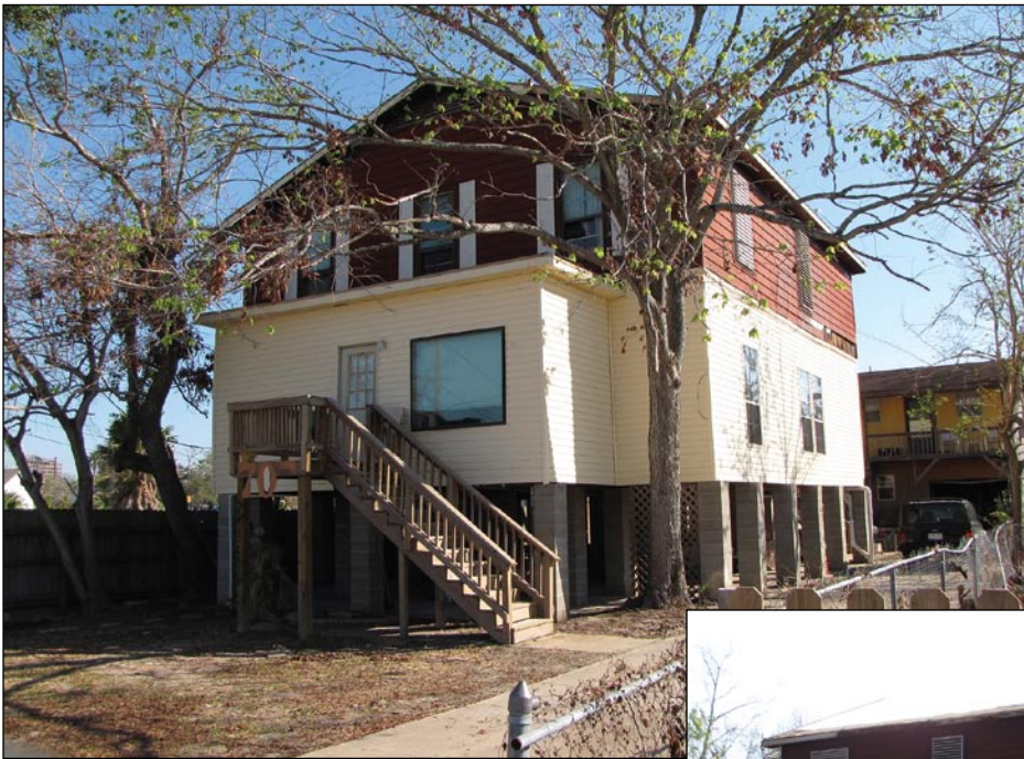
Figure 3-142. House elevated with Increased Cost of Compliance funds (Kemah, TX). Inset shows evidence of wind damage to roof (Hurricane Ike estimated wind speed in this area: 90 mph, Exposure B).
