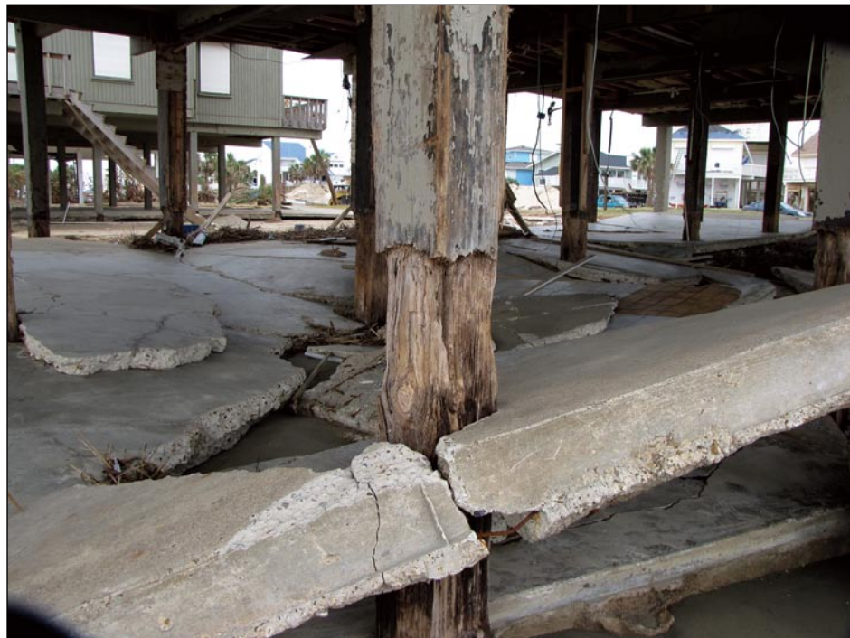
Figure 3-28. Deterioration in wood piling. The foundation did not fail during Ike, but it was weakened and will be more susceptible to failure in the future (Galveston Island, TX).
