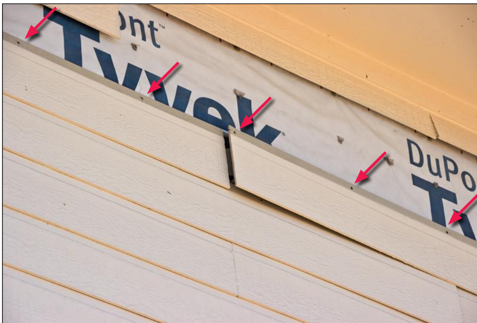
Figure 3-89. Damaged fiber cement plank siding. Note that blind nailing alone (red arrows) is recommended only for 90-mph or less installation. Higher wind zone installations should include both blind and face nailing (Hurricane Ike estimated wind speed in this area: 93 mph, Exposure B).
