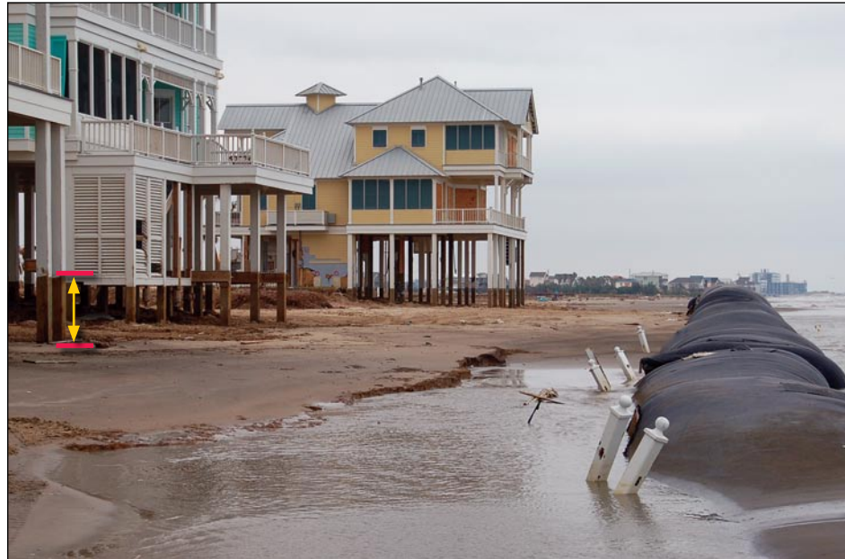
Figure 3-17. Exposed geotextile tubes formerly covered by sand and dune vegetation. Note erosion behind the tubes and under Zone V (BFE = 18 feet) buildings (yellow arrow at left).
