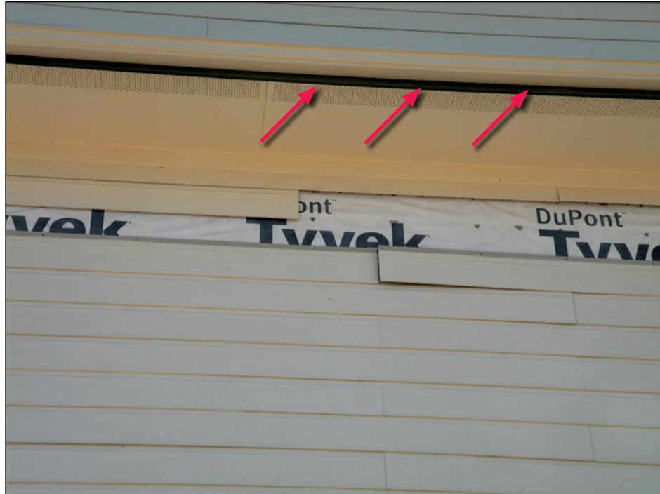
Figure 3-104. Fiber cement soffit remained connected; soffit vent slots shown with red arrows. Fiber cement plank siding was damaged (Tiki Island, TX; Hurricane Ike estimated wind speed in this area: 88 mph, Exposure B).
