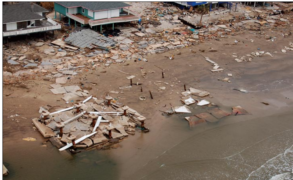
Figure 3-57. Post-Ike photograph of West Galveston Island, TX, illustrating increased severity of flood damage near the shoreline
