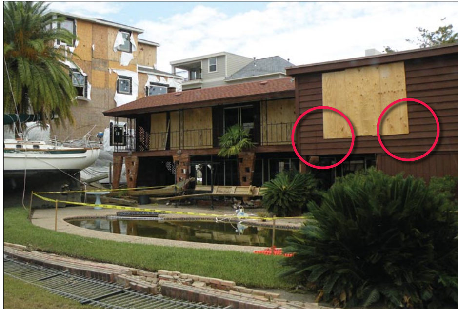
Figure 3-103. Plywood shutters installed into the wall cladding (red circles) in Clear Lake, TX (Hurricane Ike estimated wind speed in this area: 90 mph, Exposure B)
