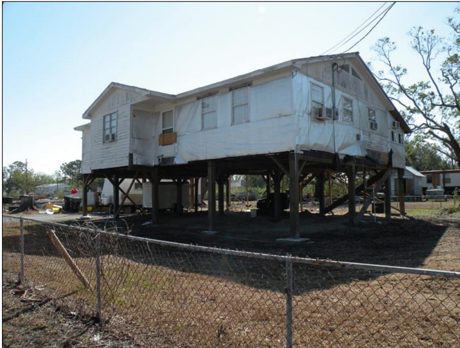
Figure 3-73. Loss of siding due to winds, Chauvin, LA (Terrebonne Parish; Hurricane Ike estimated wind speed in this area: 50 to 60 mph, Exposure B)
