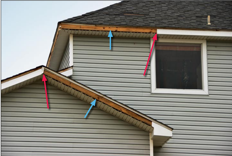
Figure 3-105. Loss of aluminum fascia cover (red arrows) exposed ends of vinyl soffit (blue arrows) to direct entry of wind-driven rain (Tiki Island, TX; Hurricane Ike estimated wind speed in this area: 88 mph)
