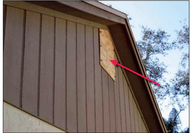
Figure 3-109. Shuttered gable end vent (red arrow)
