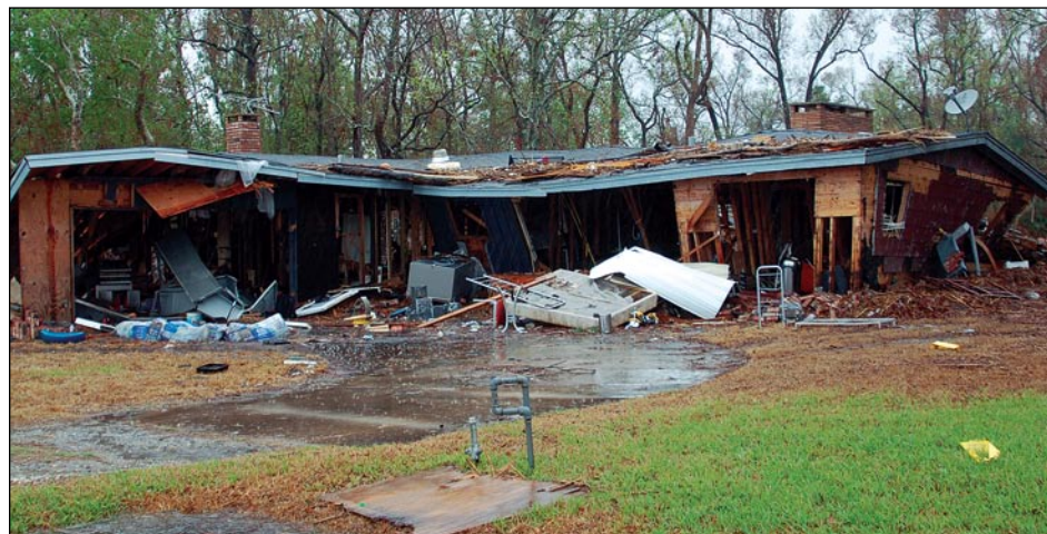
Figure 3-11. This house sustained significant structural damage due to storm surge and small waves above the 9-foot BFE in Zone A (Bridge City, TX). Note flood debris line on the roof.
