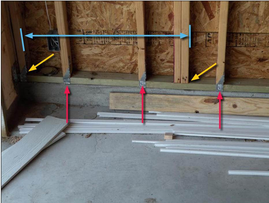
Figure 3-52. Studs and sill plate connected in new house (sill bolts yellow arrows and clips red arrows). However, sill bolts are spaced too far apart (2 feet is the maximum spacing allowed) and did not have 3-inch by 3-inch by 1/8-inch washers per 2003 IRC and TDI-adopted IBHS guidelines. Blue line shows 3-foot spacing (Webster, TX).
