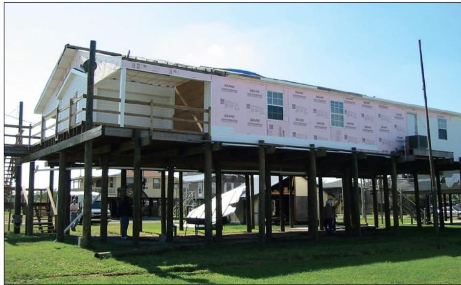
Figure 3-137. This elevated manufactured home in Grand Isle of Jefferson Parish, LA, had siding and roof damage, but did not move from its foundation
