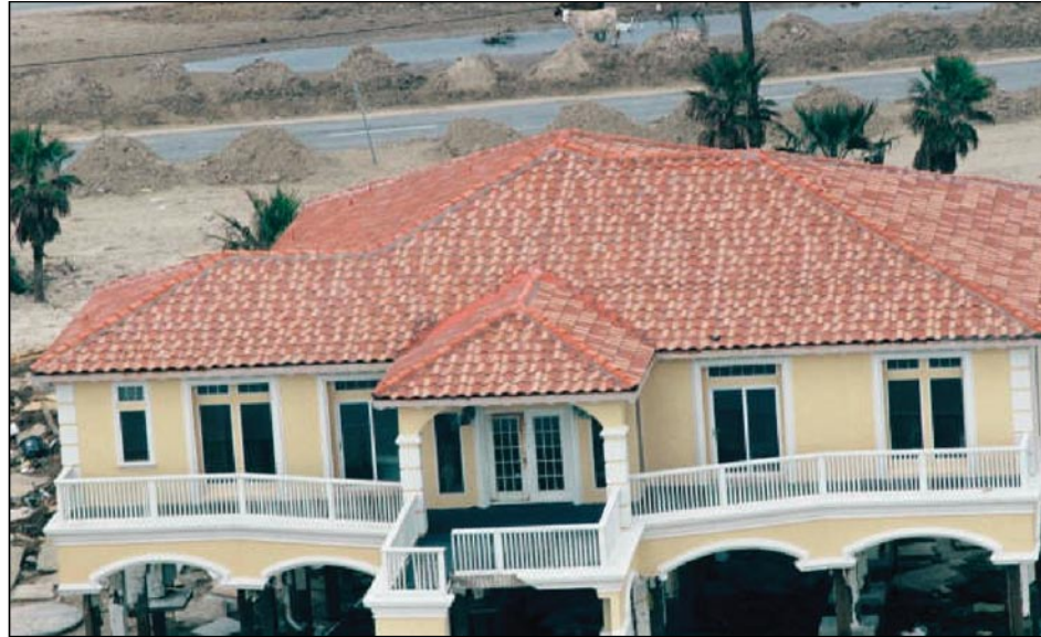
Figure 3-71. This tile roof on Galveston Island, TX, did not experience any wind damage (Hurricane Ike estimated wind speed in this area: 106 mph)
