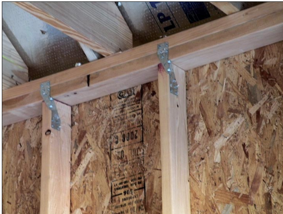
Figure 3-53. Studs clipped to double top plate; rafter-to-top plate connector has yet to be installed. Better framing practices could have avoided some of the problems shown in this photo. Ceiling joists are not well nailed to the rafter and may twist in the future. The builder did not take advantage of aligning wall framing and rafter framing to simplify connections for wind loads.
