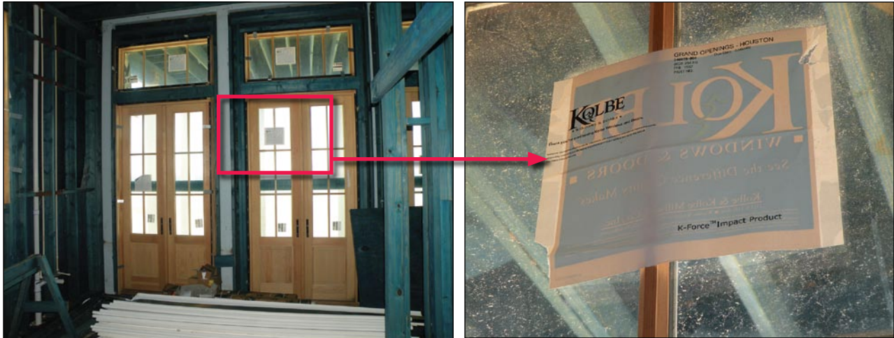
Figure 3-95. Impact-resistant door and window glazing in new East Galveston, TX, house. Inset shows manufacturer's label indicating glazing is impact resistant.
