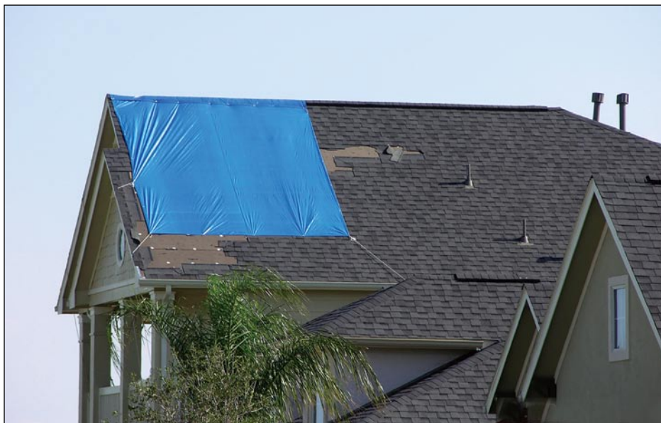
Figure 3-62. Shingle damage at a house near the one shown in Figure 3-61 (Webster, TX)
