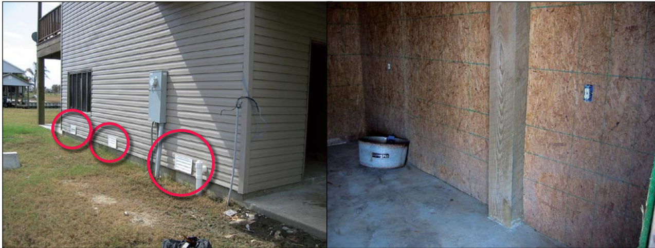
Figure 3-132. Flood vent openings (red circles) that do not extend through the walls (Hackberry, Cameron Parish, LA)
