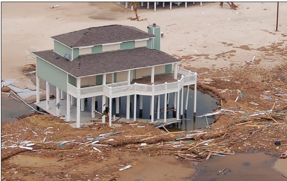
Figure 3-20. Foundation scour was reported to be 10 feet deep—note the bottoms of the piles on the right side of building that have been pushed toward the building (Bolivar Peninsula, TX; Zone V)
