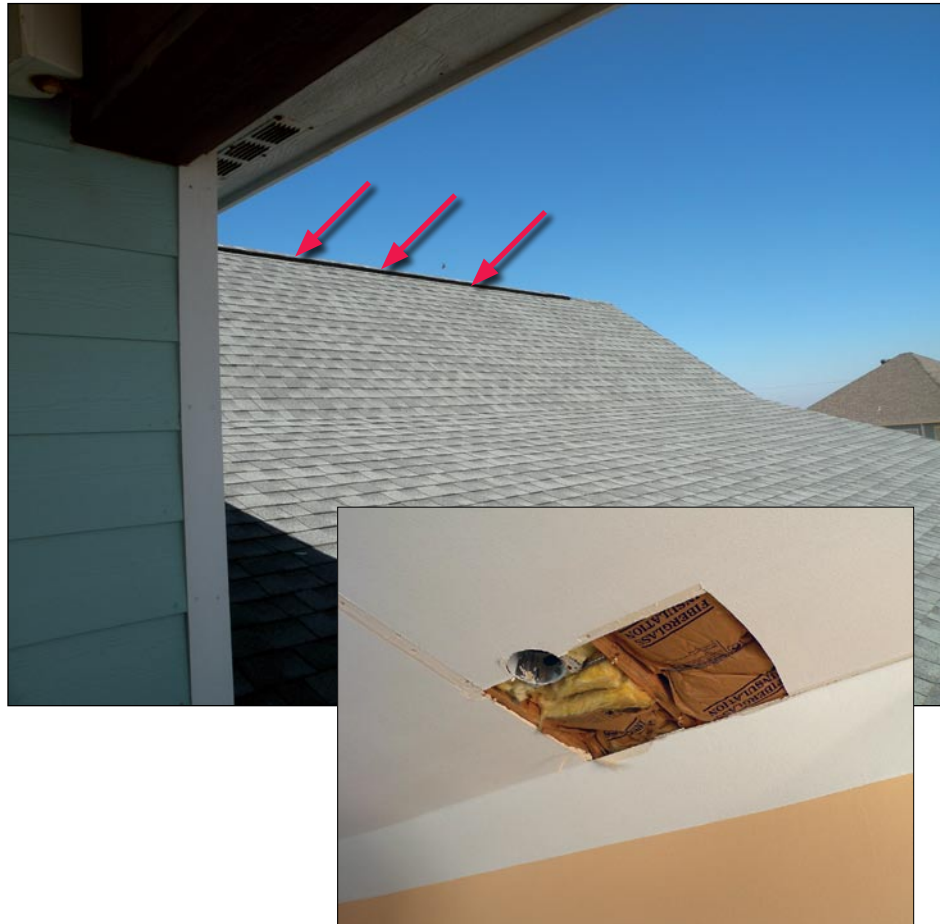
Figure 3-107. The roof ridge vent (red arrows) on this Bolivar Peninsula, TX, home leaked, and it is presumed that the water was shed down the underside of the roof decking and/or structure, thereby producing ceiling damage along the wall of this second story room (Hurricane Ike estimated wind speed in this area: 110 mph, Exposure C)
