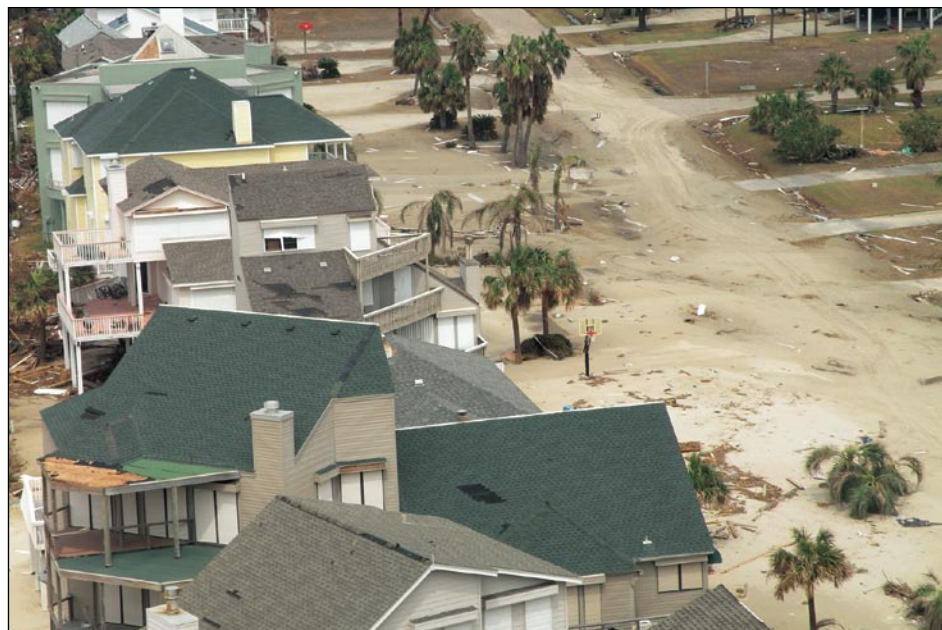
Figure 3-59. A substantial amount of siding (the white lines scattered around the ground), along with roofing materials, blew off these West Galveston, TX, houses (Hurricane Ike estimated wind speed in this area: 90 mph)
