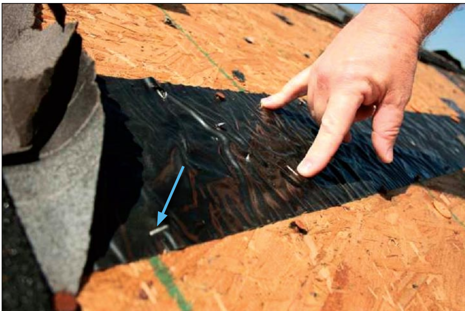
Figure 3-68. This tape did not provide a watertight seal. Note the wrinkles (which allow water migration) and the staples (blue arrow) that were used to attach the tape (Audubon Village, TX). CREDIT: IBHS
