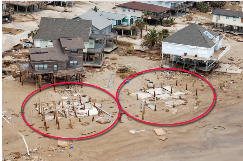
Figure 3-34. Broken piles beneath destroyed Gulf-front houses, Galveston Island, TX (west of the seawall)
