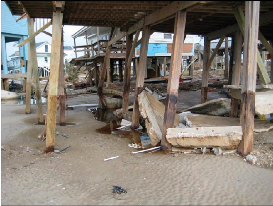
Figure 3-126. Slab failure probably contributed to foundation damage (West Galveston Island, TX)
