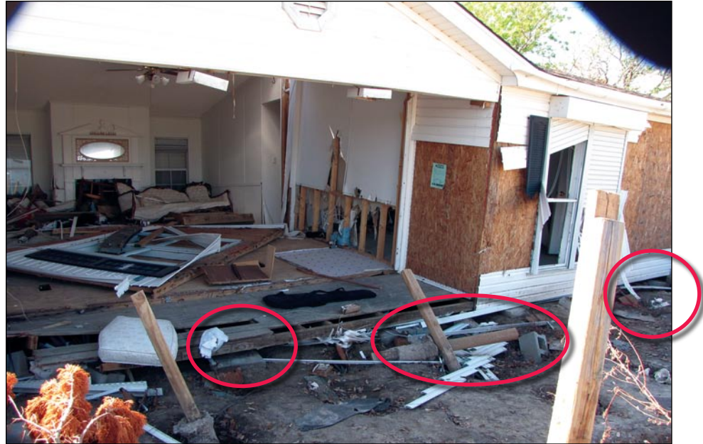
Figure 3-134. Scour depressions existed around the masonry piers, pads, and ground anchor stabilizer plates (San Leon, TX)
