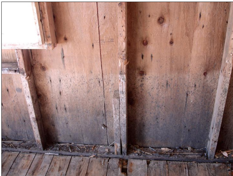
Figure 3-130. Mildew and mold forming on wall sheathing following flooding (Golden Meadow, LA)
