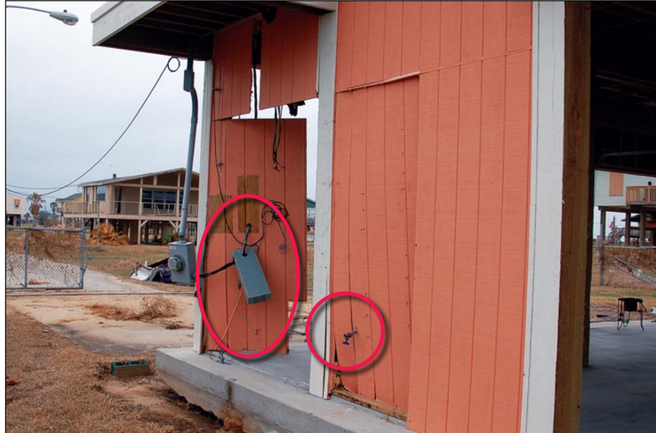
Figure 3-115. Attachment of utilities to breakaway wall may have prevented the wall from breaking away, thereby resulting in additional damage to the structure (Galveston Island, TX)
