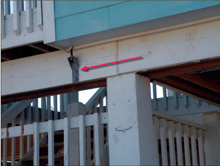
Figure 3-56. Existing house shear wall connector incorrectly located (red arrow). Connector should be located on column line or the beam and beam-to-column connection should be designed to resist the uplift load, which is carried by a nailed connection in the absence of bolts (Sunset Crystal Beach, Bolivar Island, TX).
