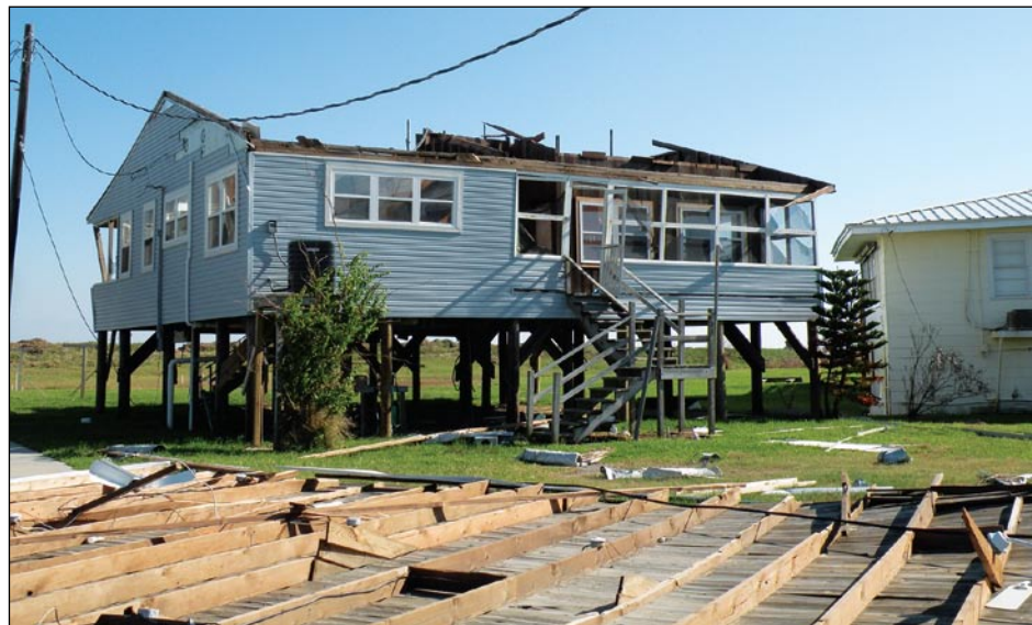
Figure 3-41. The roof structure was poorly connected to this house in Grand Isle (Jefferson Parish, LA) and was blown off by 50-mph Ike winds (Exposure B)
