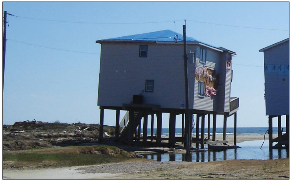
Figure 3-128. The weight of this slab, undermined due to scour and erosion, could have contributed to settlement and racking of this elevated house (Surfside Beach, TX)
