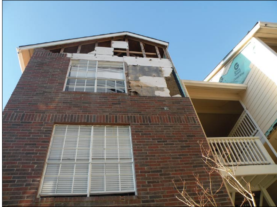
Figure 3-40. This West Bay, Galveston Island, TX, apartment experienced gable-end wind damage as a result of sheathing failure and poor connection of the brick veneer to the stud walls (Hurricane Ike estimated wind speed in this area: 90 mph, Exposure B)
