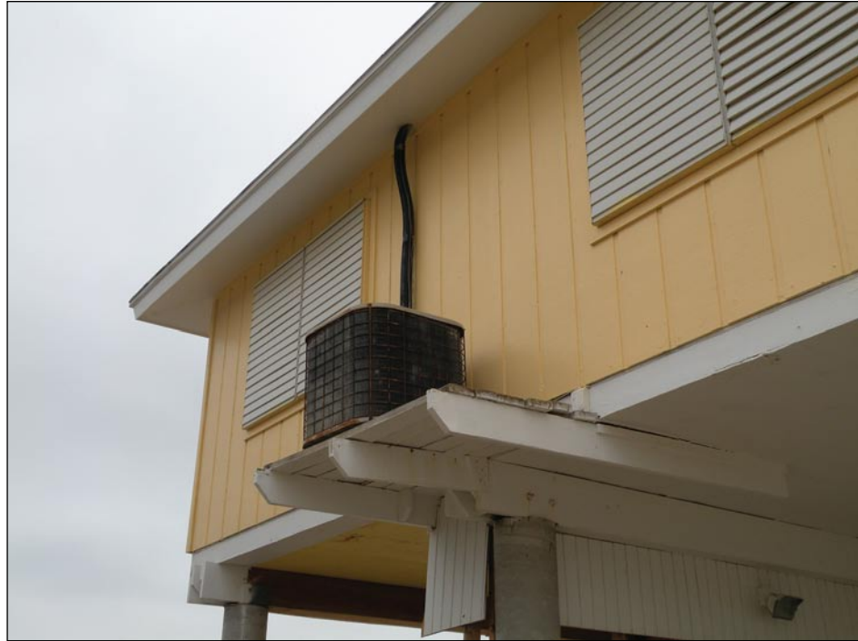
Figure 3-111. Typical cantilevered condenser (Jamaica Beach, TX; Hurricane Ike estimated wind speed in this area: 80 mph, Exposure B)
