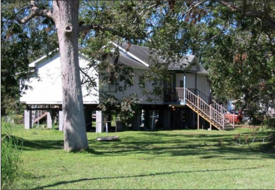
Figure 3-141. Zone A house elevated with Increased Cost of Compliance funds on masonry piers (Iberia Parish, LA). There was no evidence of pier reinforcement, mortar between masonry blocks, or ties between the piers and the elevated home.
