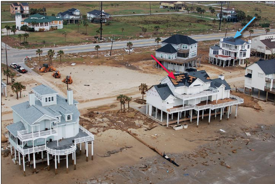
Figure 3-60. Some of the roofs on these Jamaica Beach, TX, houses had no roof covering damage, while one had moderate damage (blue arrow) and one had extensive damage, including loss of underlayment (red arrow) (Hurricane Ike estimated wind speed in this area: 90 mph)
