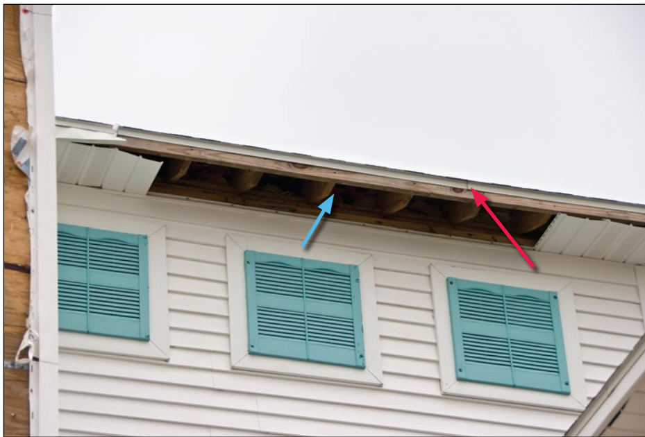
Figure 3-106. Loss of fascia cover (red arrow) led to loss of soffit (blue arrow), exposing the attic to wind-driven rain (San Luis, TX; Hurricane Ike estimated wind speed in this area: 93 mph, Exposure C)
