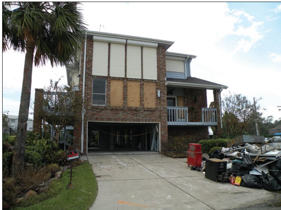
Figure 3-96. Clear Lake, TX, house with plywood shutters installed on the accessible first floor and roll-down shutters installed on the less accessible second floor (Hurricane Ike estimated wind speed in this area: 90 mph, Exposure B)
