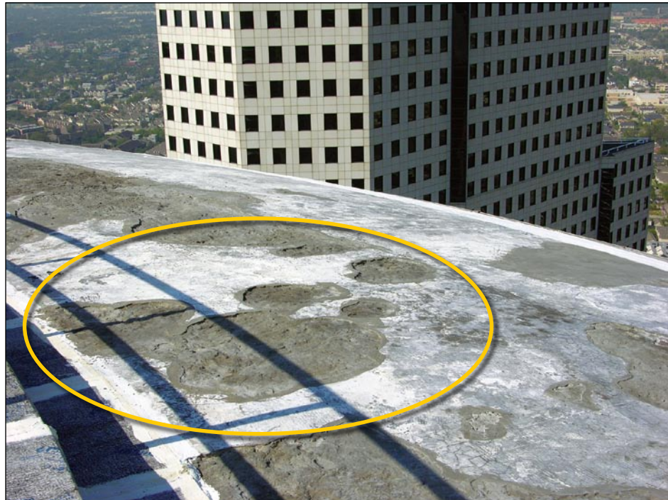
Figure 5-20. The lightweight insulating concrete deck was gouged in many locations
