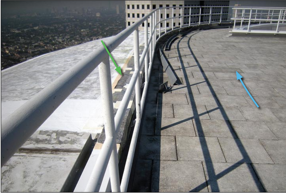
Figure 5-21. View of the damaged window washing track (green arrow). The concrete pavers (blue arrow) were not damaged.
