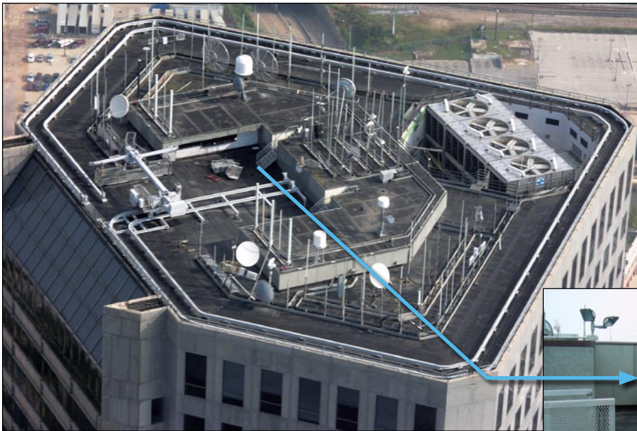
Figure 5-12. View of the JP Morgan Chase Tower roof. Inset shows damaged window washing equipment.
