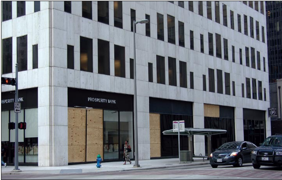
Figure 5-3. Random breakage of first floor glazing
