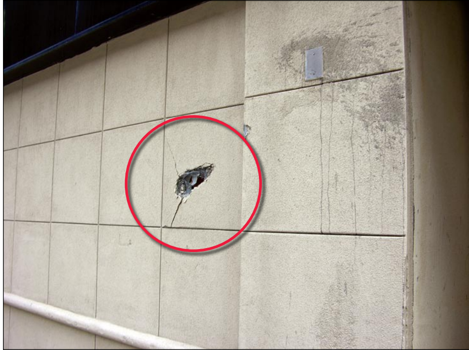
Figure 5-5. The wire mesh of this stucco wall was penetrated by windborne debris. The impact location is about 5 feet above the sidewalk.
