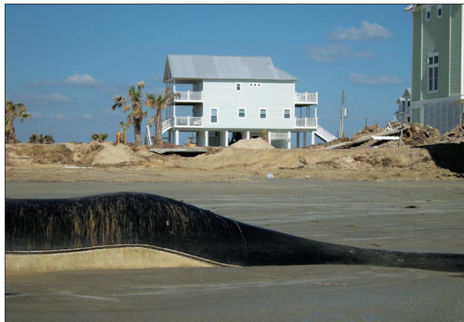
Figure 8-4. Broken geotextile tube at Beachside Drive, Galveston Island, TX
