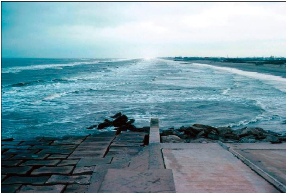
Figure 8-5. West end of the seawall at Galveston, TX. The concrete ramp (right foreground) was the road leading to the beach in the mid-1960s. Since then, the beach has eroded more than 492 feet.
