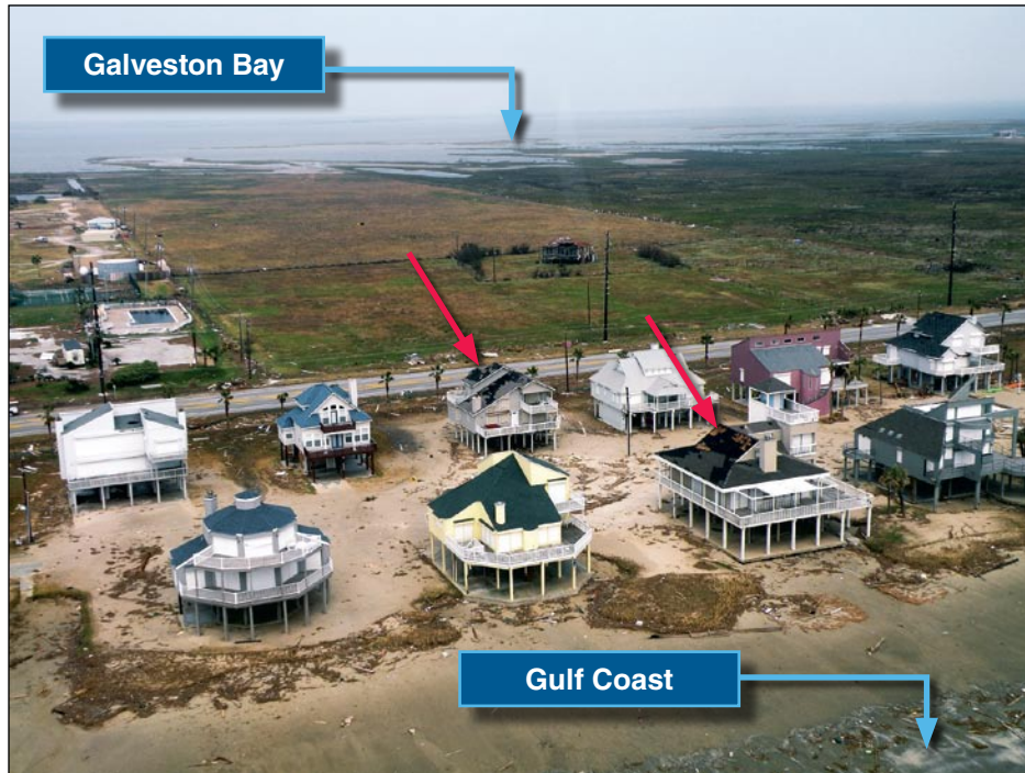
Figure 1-12. Roofing damage to north and west exposures produced by Hurricane Ike backside winds
