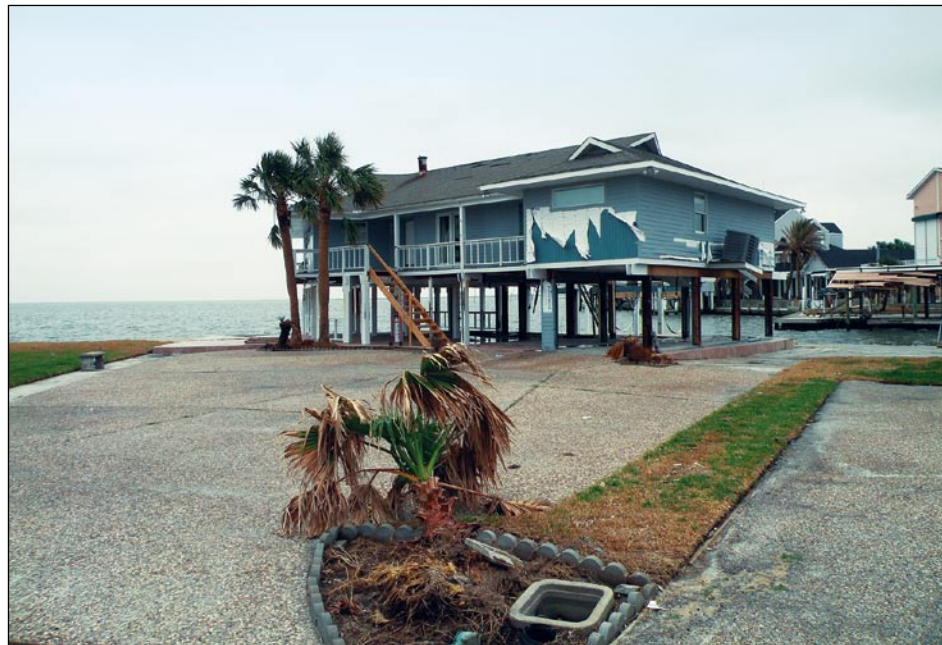
Figure 2-8. Jamaica Beach house on the West Bay with “backside” wind damage (number 2480 in 1990 Galveston study)
