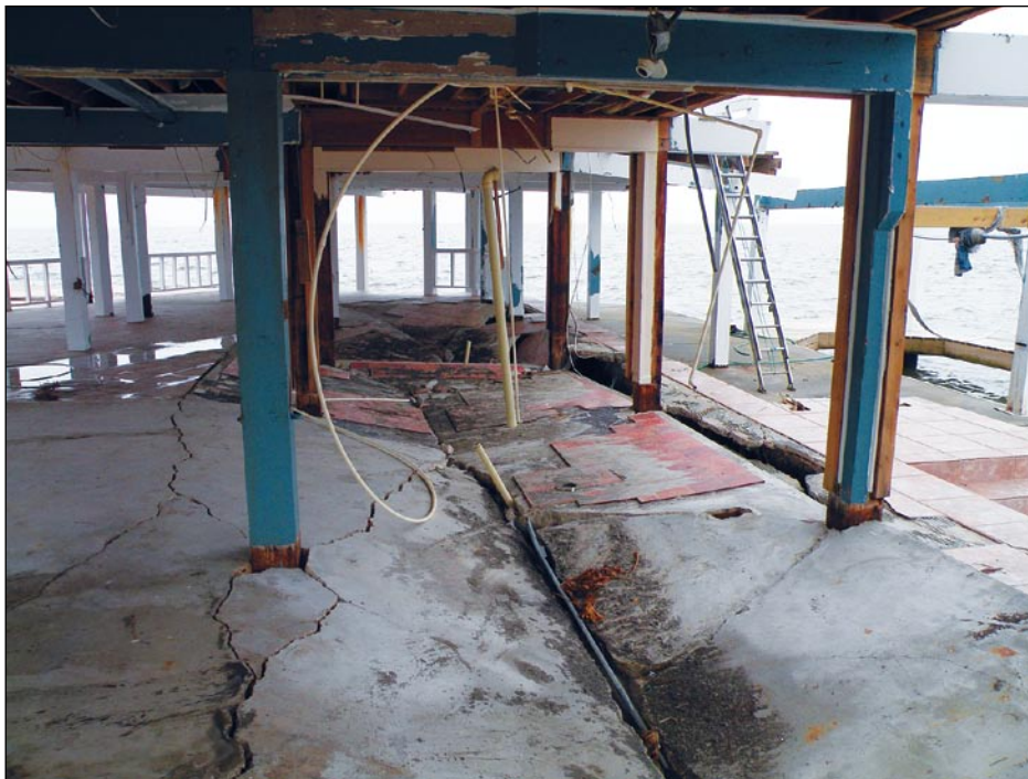
Figure 2-9. First floor walls removed and floor slab undermined by flooding and waves at this Jamaica Beach house (number 2480 in 1990 Galveston study)
